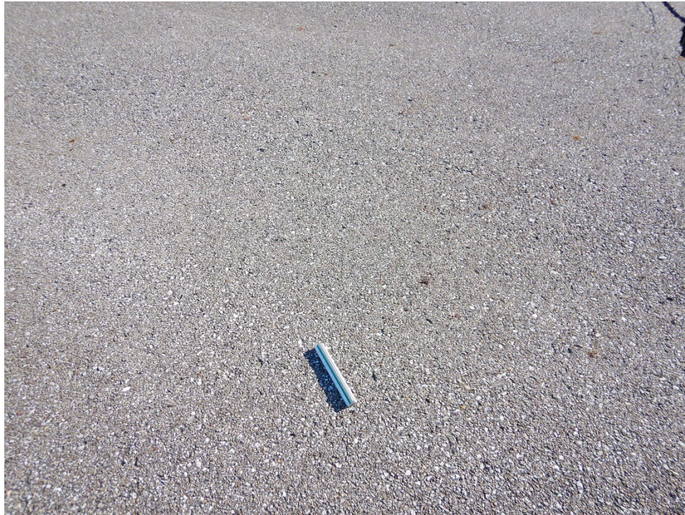
T03AL-01. Raveling (Sample Unit No. 01).
