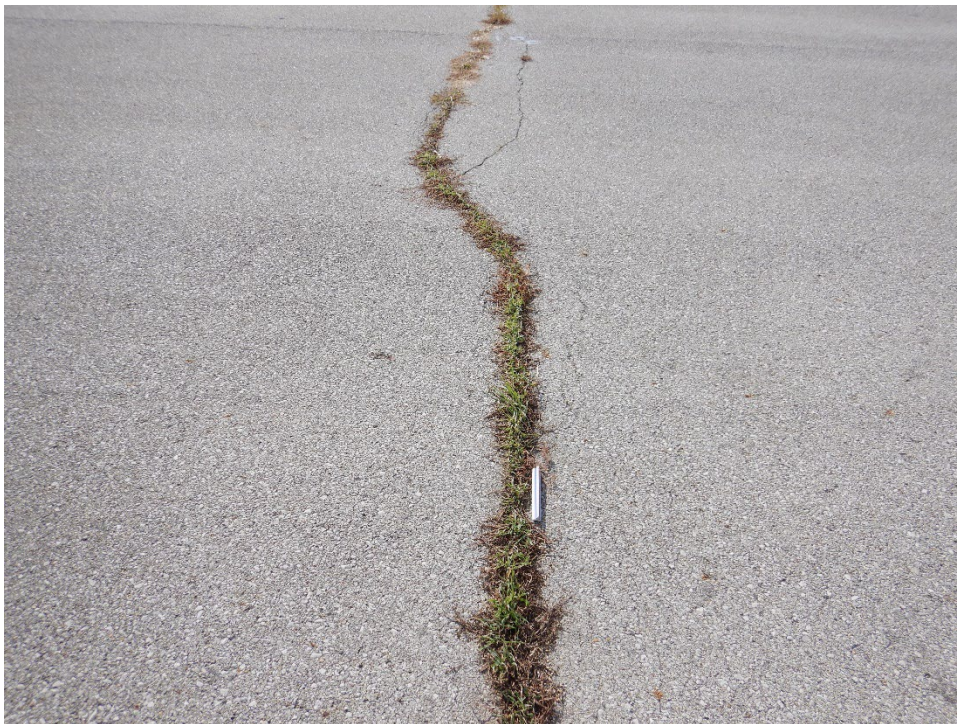
A01AL-01. L&T Cracking (Sample Unit No. 02).
