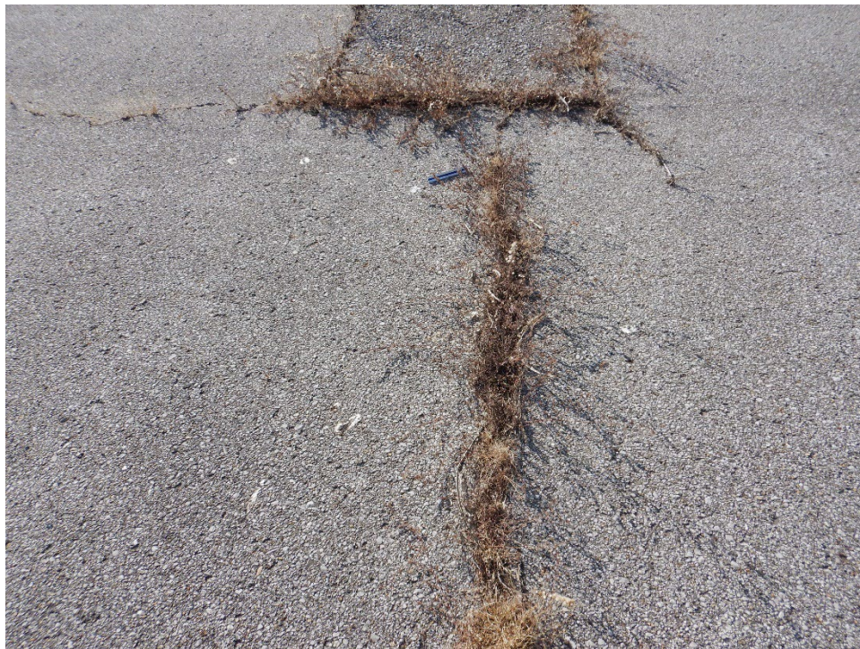
R13AL-05. L&T Cracking (Sample Unit No. 01).
