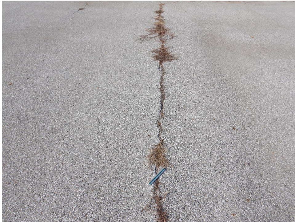
A01AL-02. L&T Cracking (Sample Unit No. 01).
