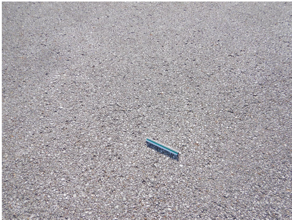
R13AL-02. Raveling (Sample Unit No. 01).
