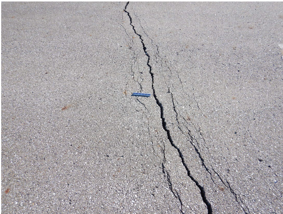
T03AL-01. L&T Cracking (Sample Unit No. 01).
