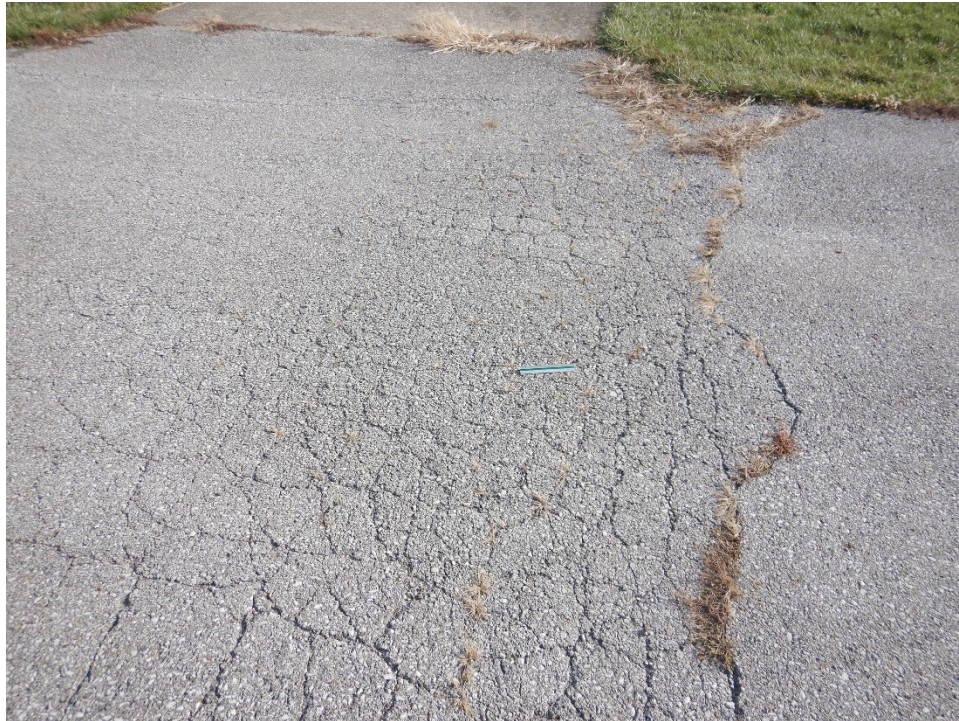
TH01AL-01. Alligator Cracking (Sample Unit No. 01).
