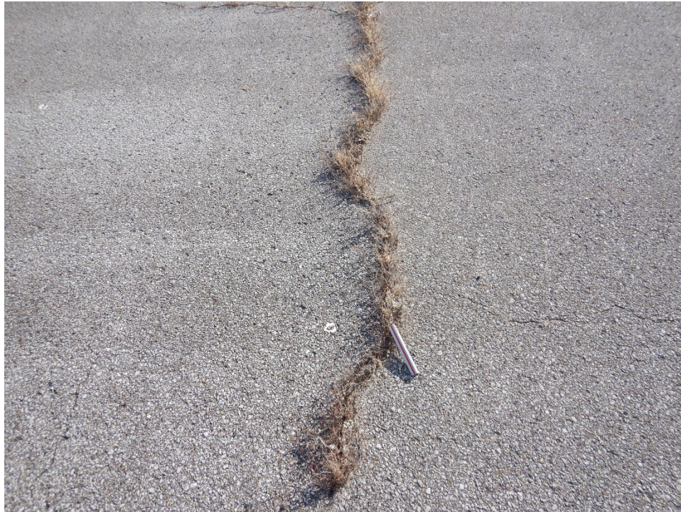
R13AL-02. L&T Cracking (Sample Unit No. 01).
