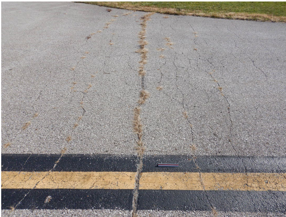
T01AL-01. Alligator Cracking (Sample Unit No. 01).
