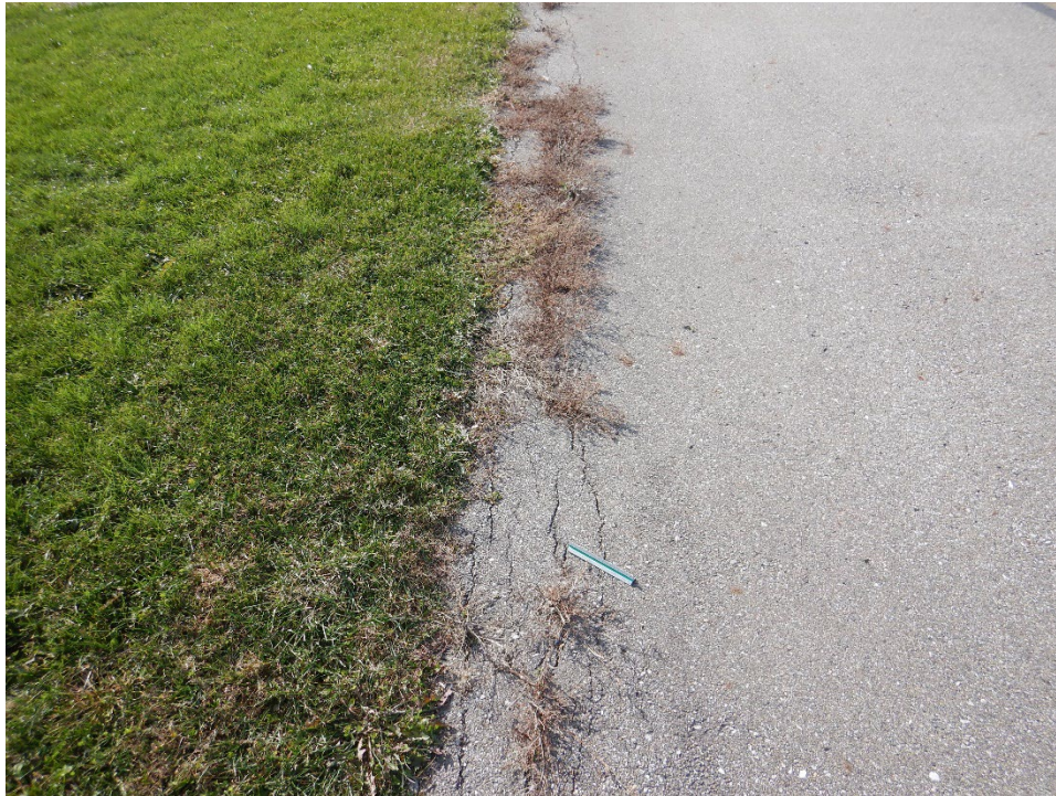
T02AL-01. Alligator Cracking (Sample Unit No. 01).
