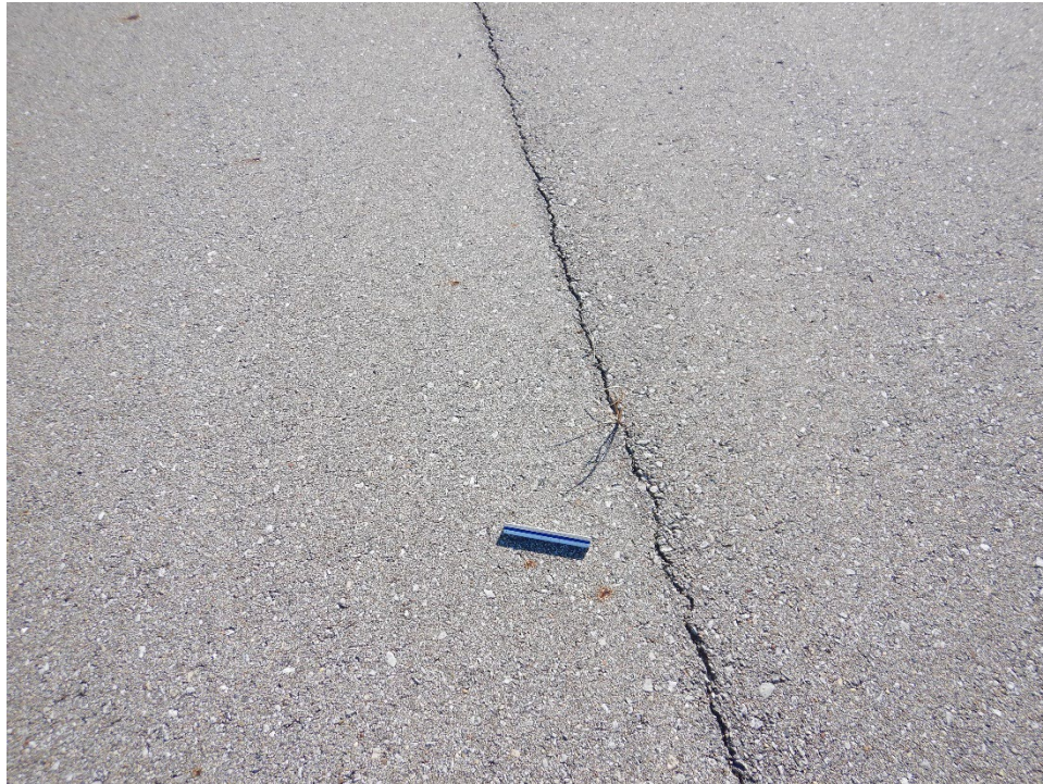
R13AL-01. L&T Cracking (Sample Unit No. 04).
