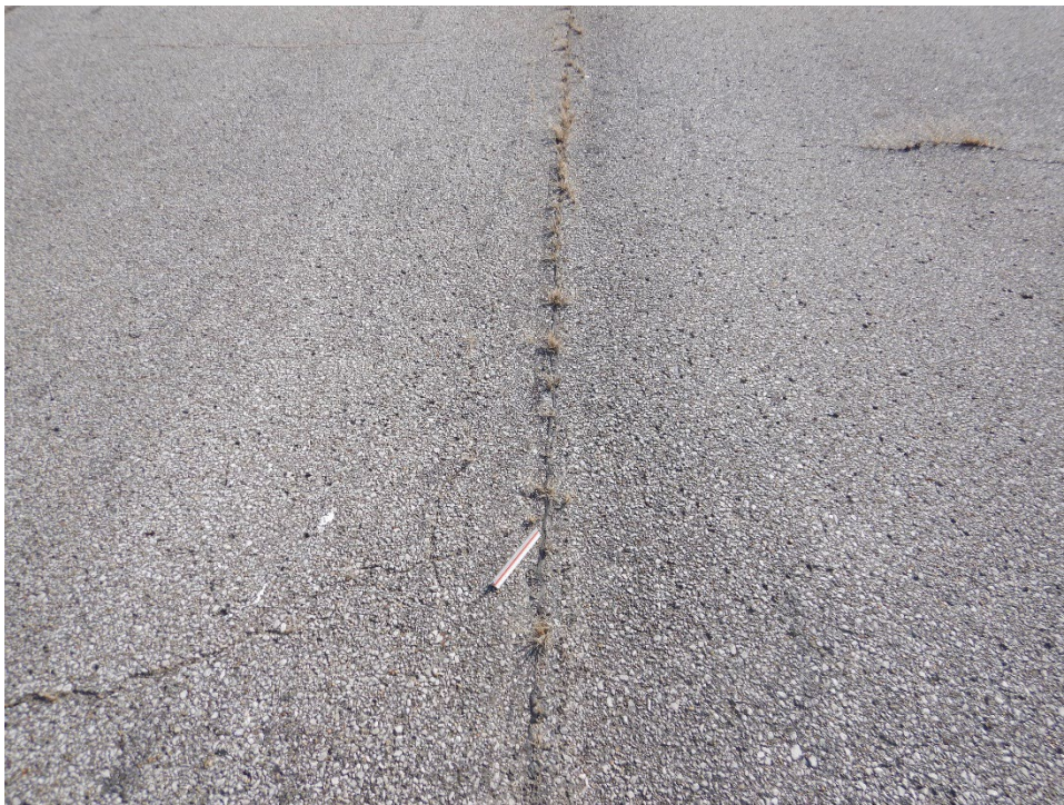
R13AL-03. L&T Cracking (Sample Unit No. 01).
