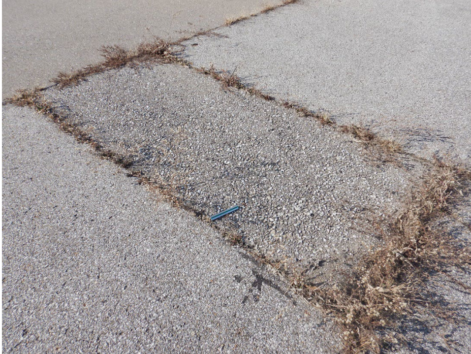
R13AL-05. Patching (Sample Unit No. 01).
