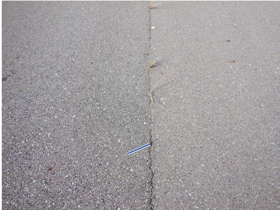
R13AL-04. L&T Cracking (Sample Unit No. 04).
