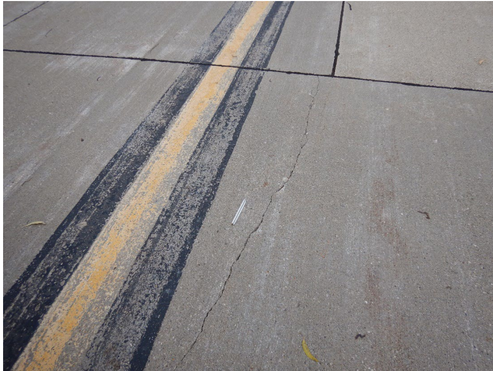
T06AN-01. LTD Cracking (Sample Unit No. 15).
