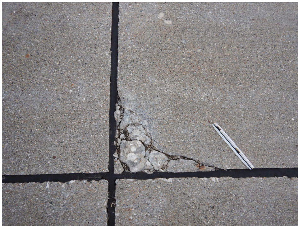
T04AN-01. Corner Spalling (Sample Unit No. 08).
