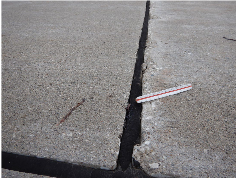
T07AN-01. Faulting (Sample Unit No. 04).
