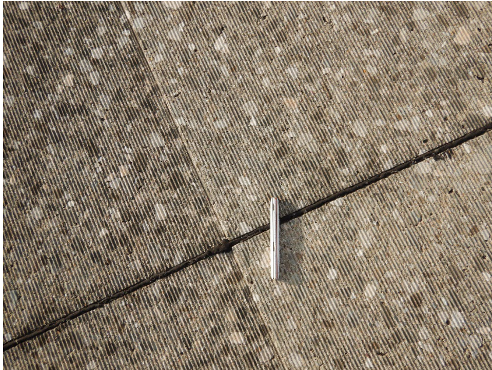
T01AN-02. Joint Seal Damage (Sample Unit No. 12).
