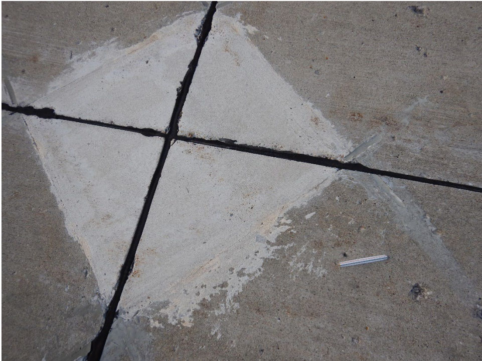
R04AN-03. Small Patching (Sample Unit No. 06).
