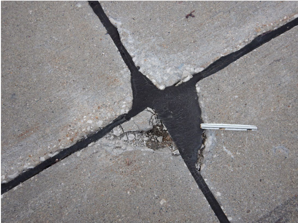
R18AN-02. Corner Spalling (Sample Unit No. 06).
