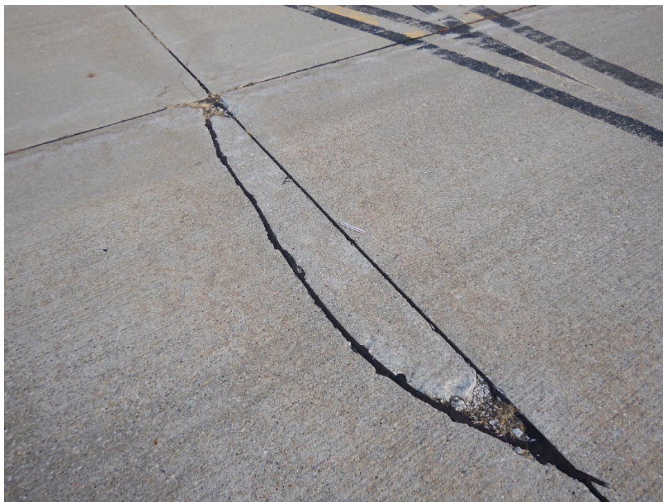
A01AN-01. Joint Spalling (Sample Unit No. 30).
