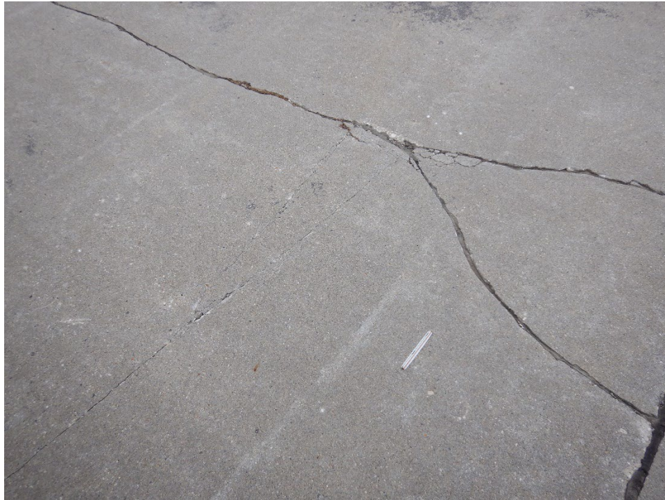
TH01AN-02. Shattered Slab (Sample Unit No. 18).
