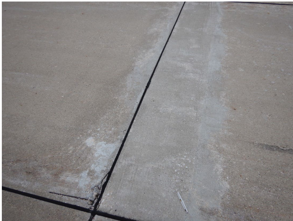
R18AN-01. Large Patching (Sample Unit No. 09).
