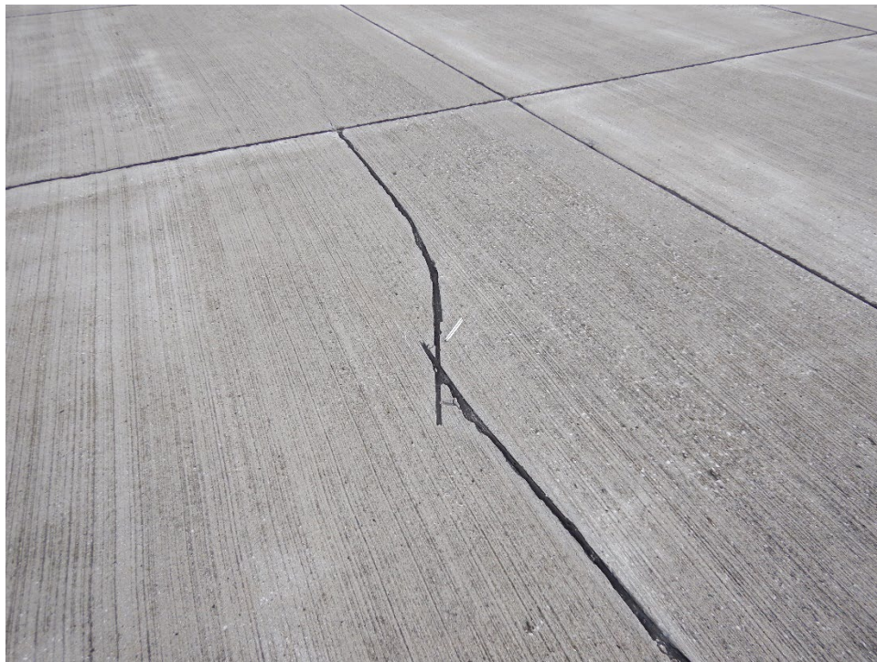
T08AN-01. LTD Cracking (Sample Unit No. 04).
