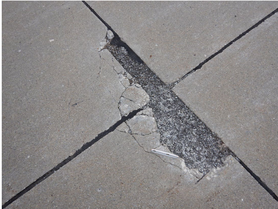
T04AN-01. Small Patching (Additional Sample Unit No. 18).
