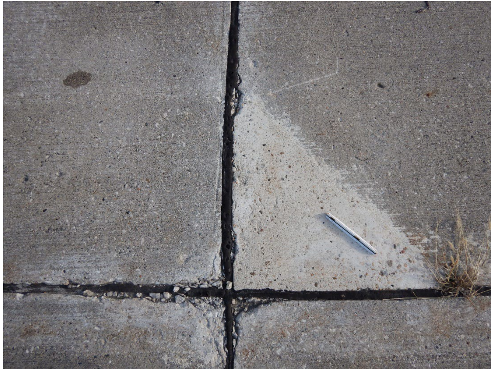
R04AN-01. Small Patching (Sample Unit No. 01).
