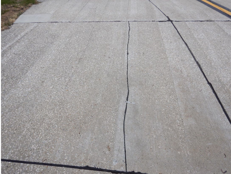
T03AN-01. LTD Cracking (Sample Unit No. 02).
