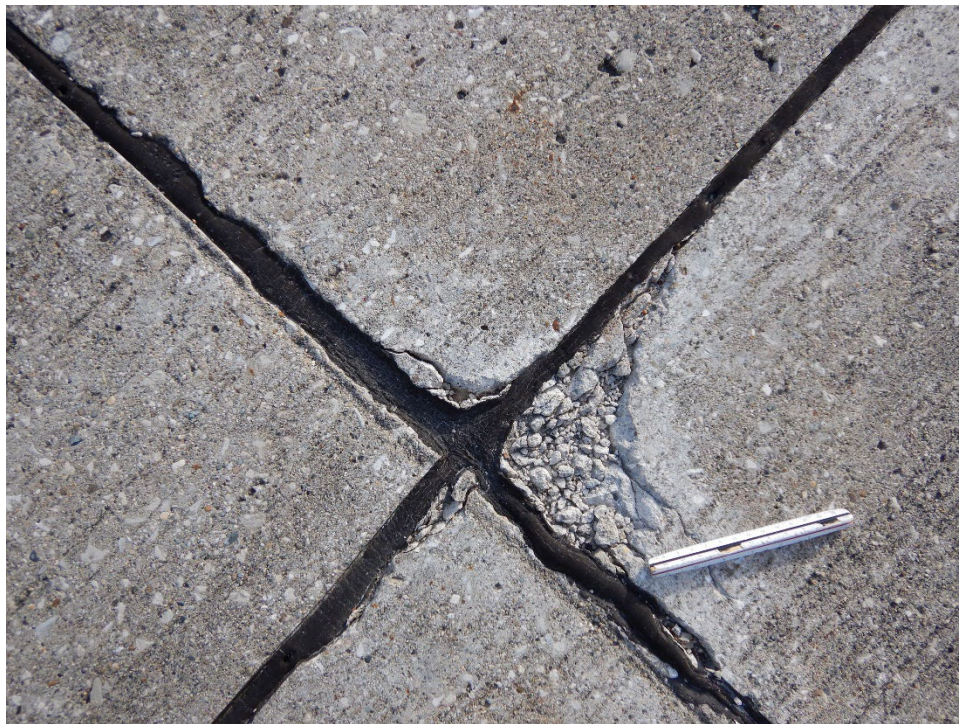
R04AN-01. Corner Spalling (Sample Unit No. 01).
