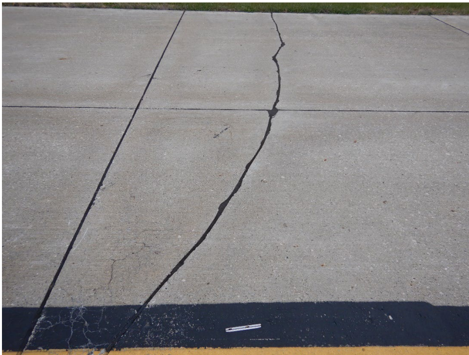
T02AN-01. LTD Cracking (Sample Unit No. 03).
