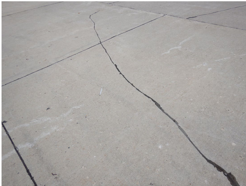
TH01AN-01. LTD Cracking (Sample Unit No. 09).
