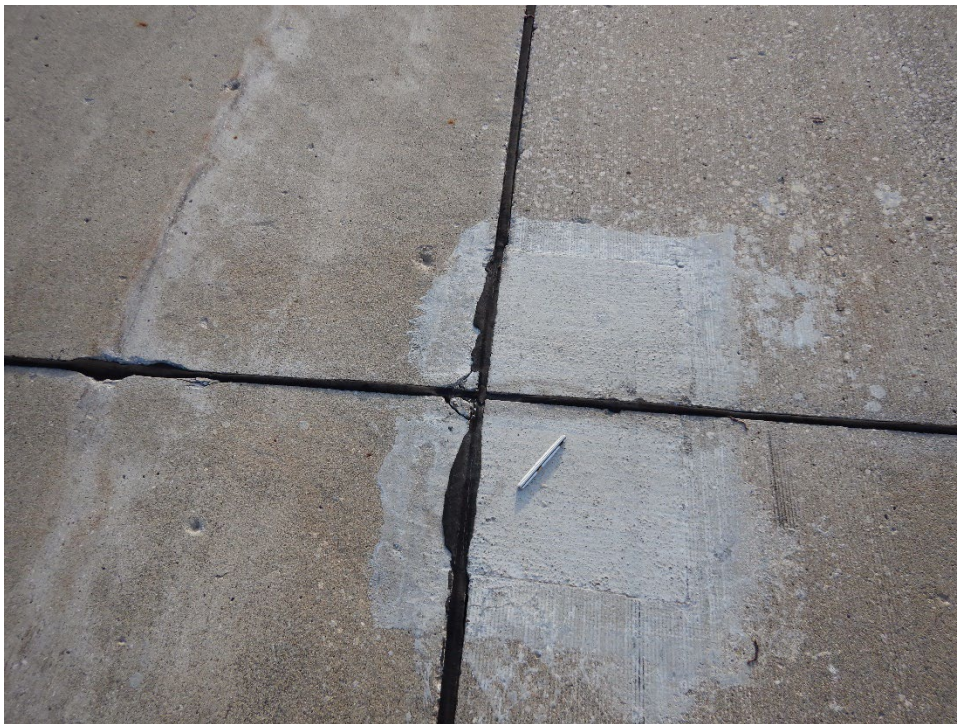
R04AN-02. Small Patching (Sample Unit No. 02).
