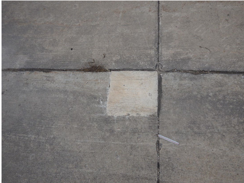
TH01AN-01. Small Patching (Sample Unit No. 09).
