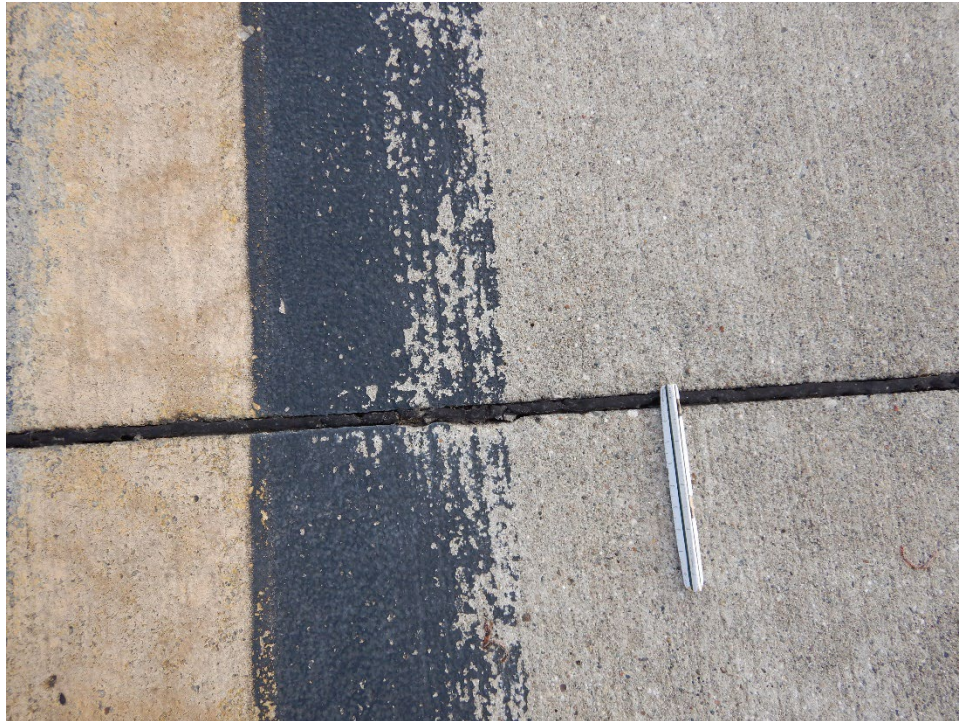
T13AN-01. Joint Seal Damage (Sample Unit No. 13).
