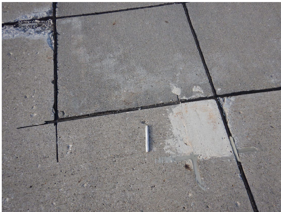
R04AN-04. Small Patching (Sample Unit No. 43).
