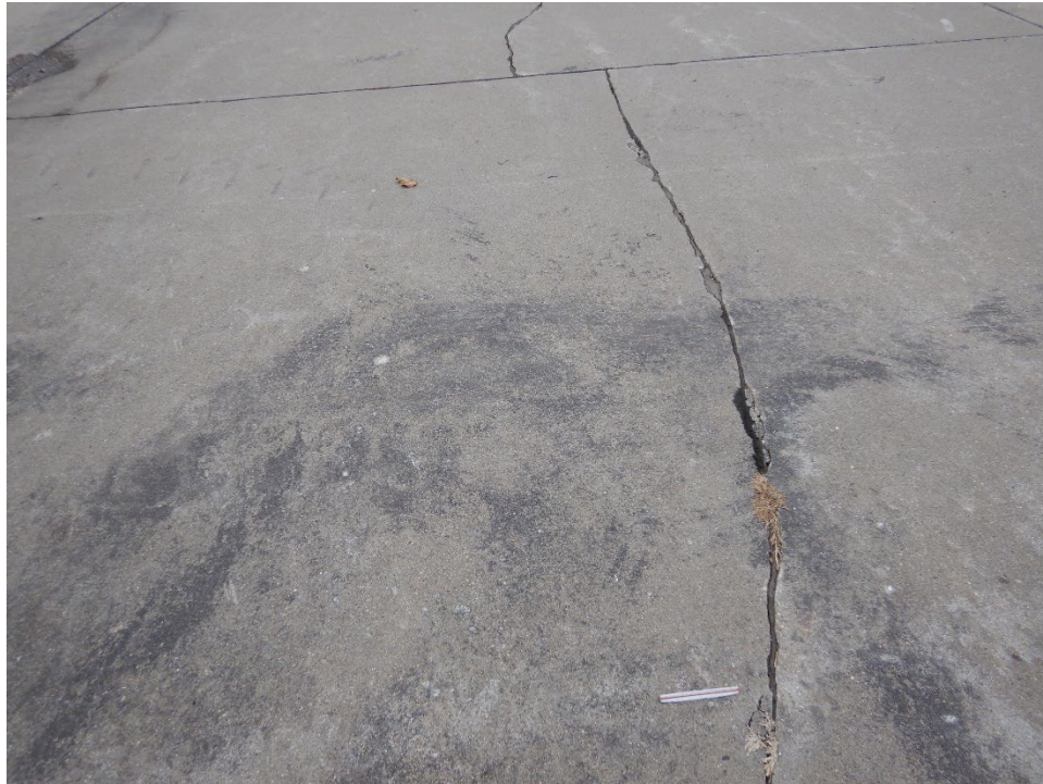
TH01AN-02. LTD Cracking (Sample Unit No. 18).
