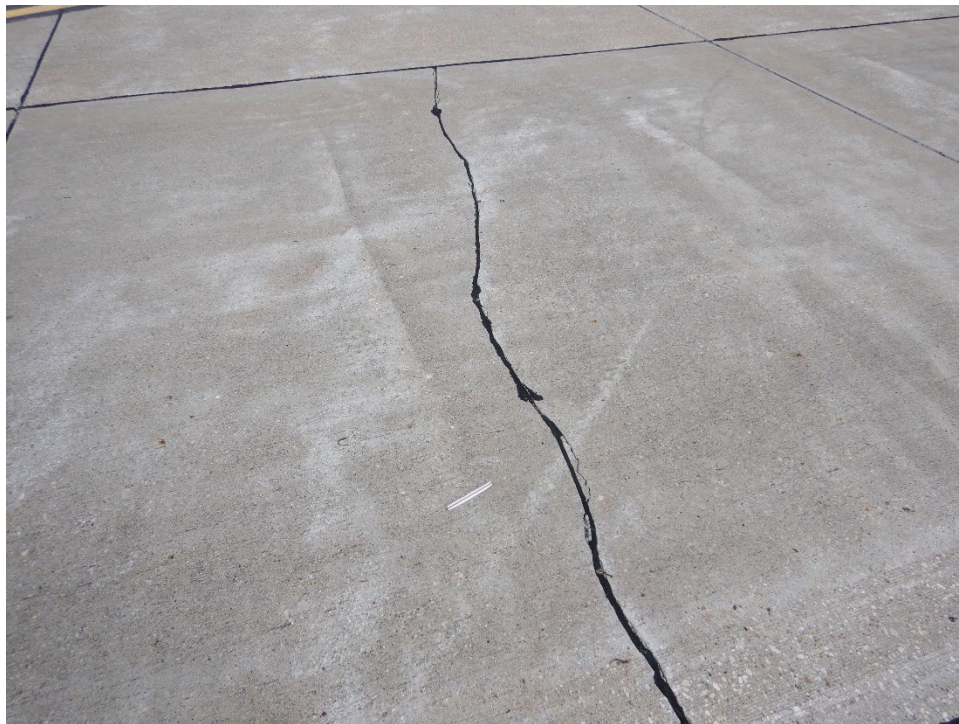
T05AN-01. LTD Cracking (Sample Unit No. 05).
