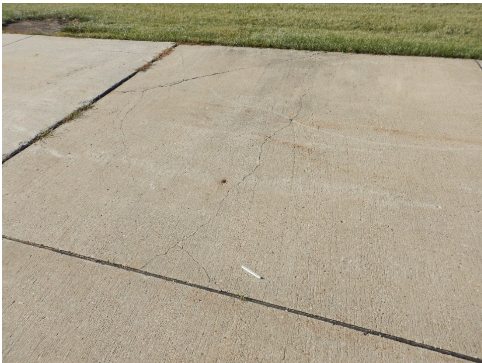
A02AU-01. Shattered Slab (Sample Unit No. 03).
