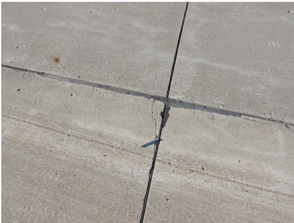
T02AU-01. Joint Spalling (Sample Unit No. 02).
