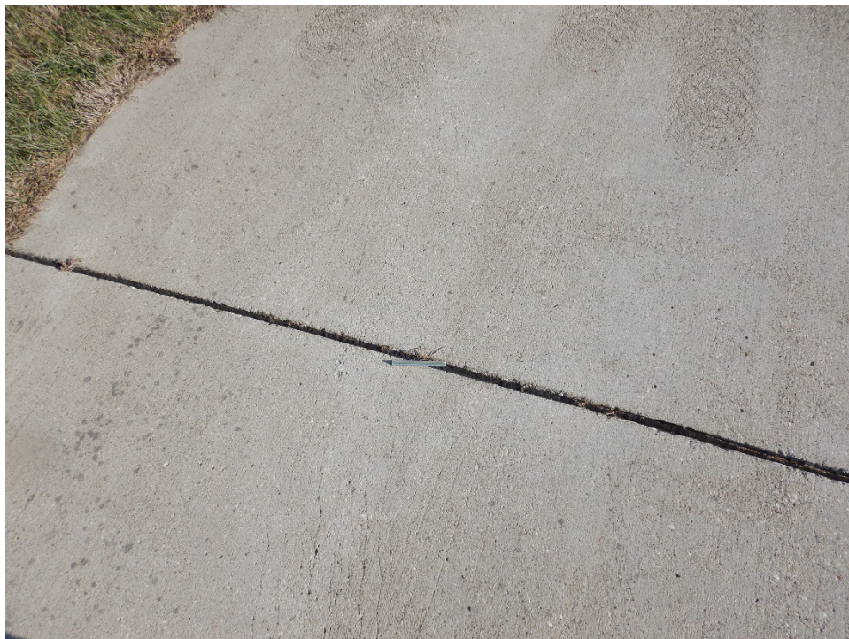
T01AU-03. Joint Seal Damage (Sample Unit No. 01).
