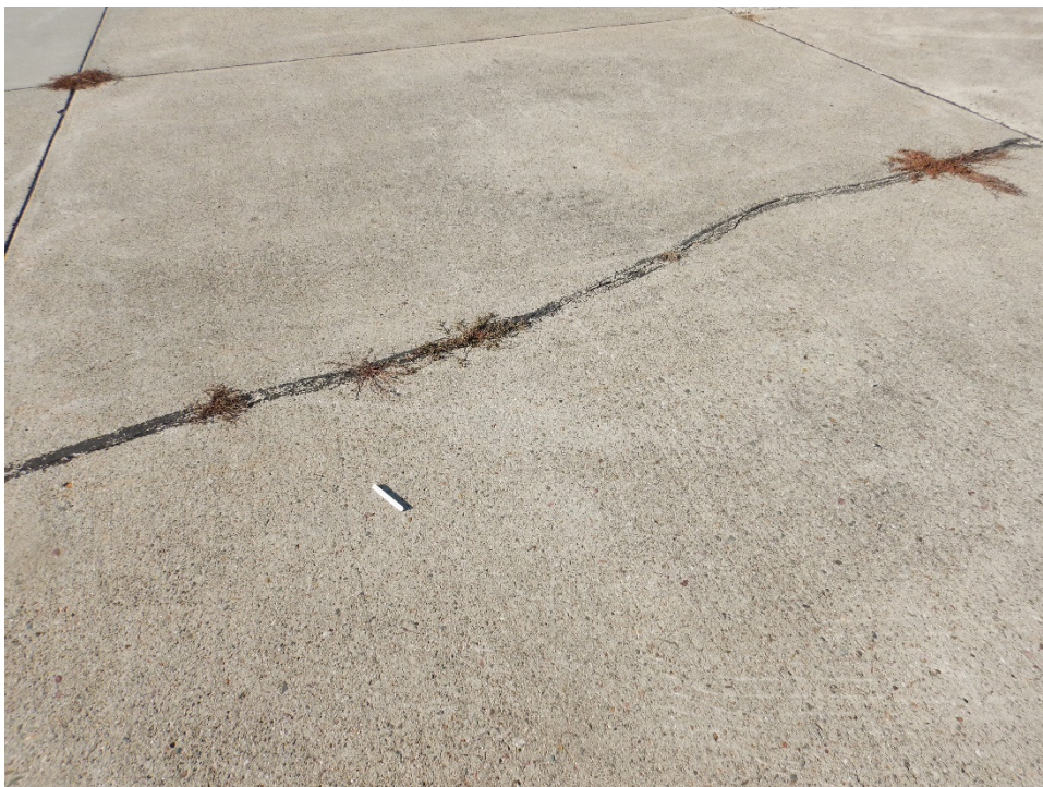
T01AU-01. LTD Cracking (Sample Unit No. 01).
