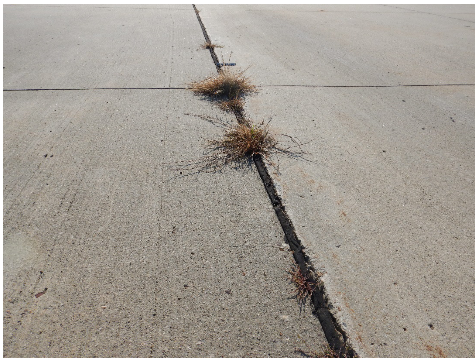
A02AU-02. Faulting (Sample Unit No. 03).
