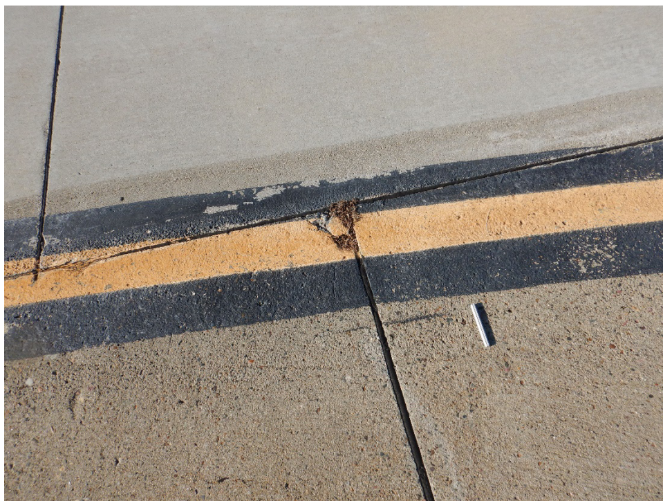
T01AU-02. Corner Spalling (Sample Unit No. 01).
