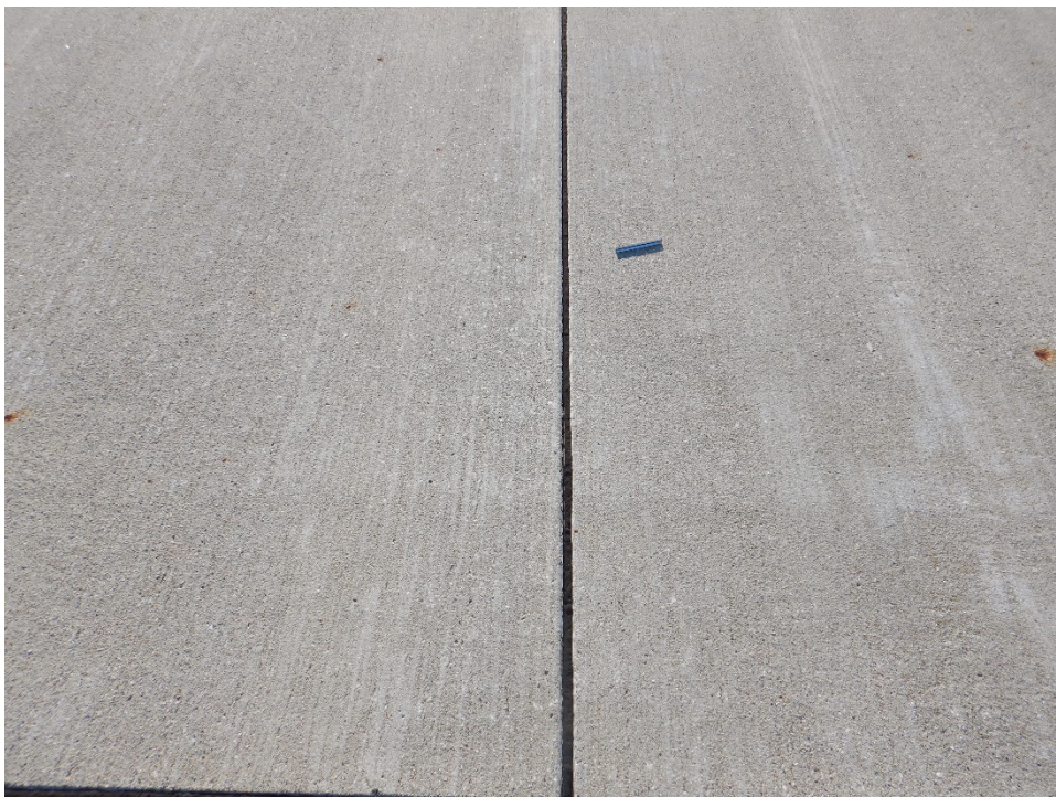
R14AU-01. Joint Seal Damage (Sample Unit No. 55).
