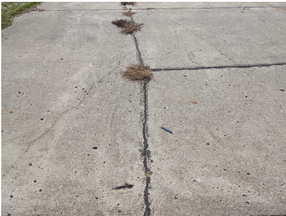
A01AU-01. Shattered Slab (Sample Unit No. 02).
