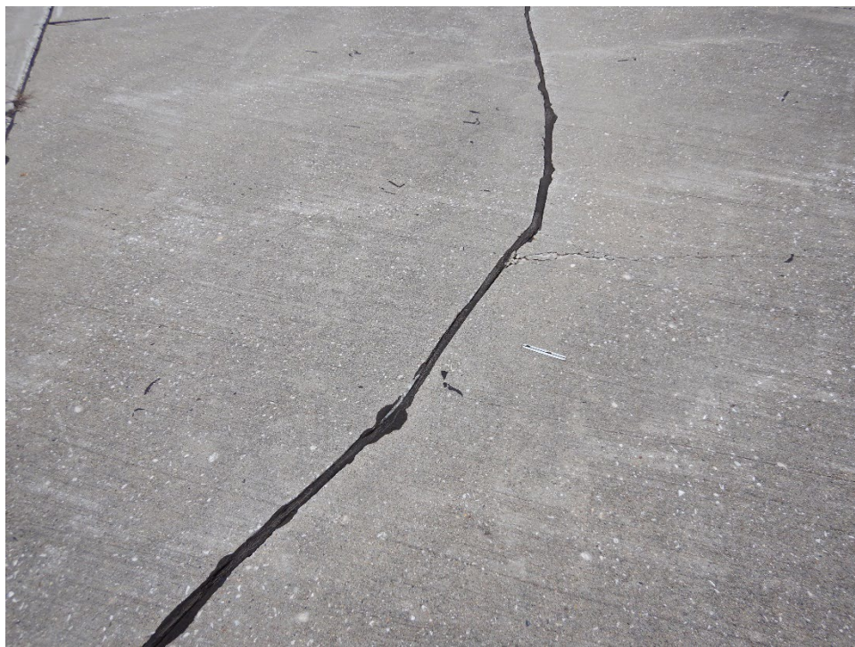
T01BP-01. LTD Cracking (Sample Unit No. 01).
