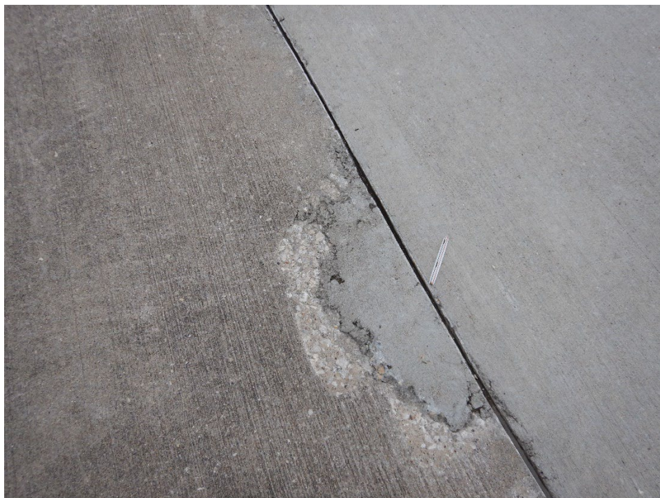
R18BP-01. Joint Spalling (Sample Unit No. 55).
