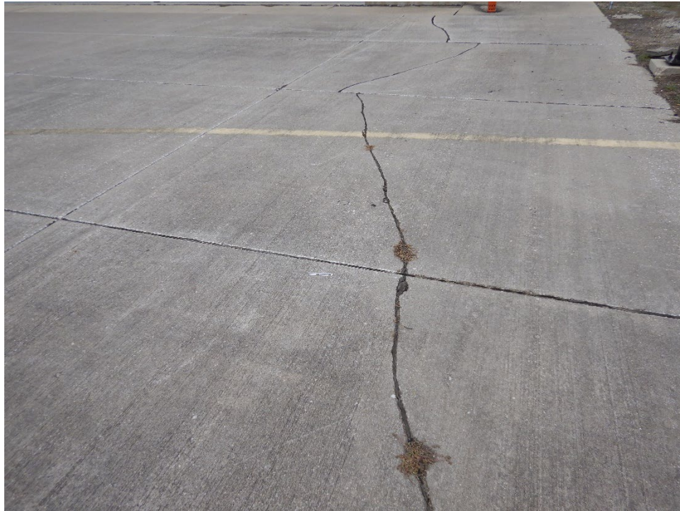
A01BP-01. LTD Cracking (Sample Unit No. 04).
