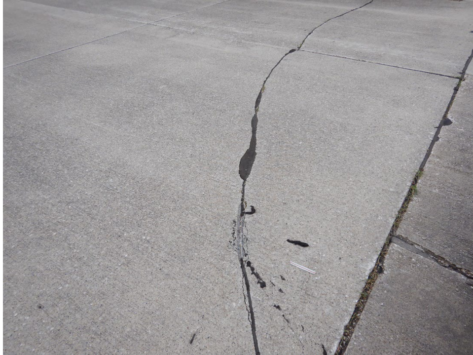
TH01BP-02. LTD Cracking (Sample Unit No. 01).
