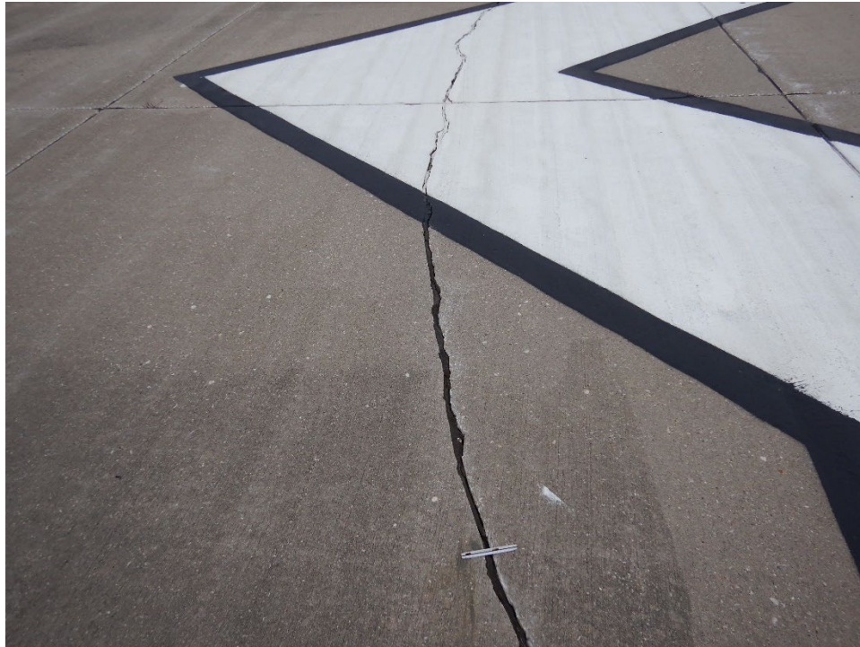
R18BP-01. LTD Cracking (Sample Unit No. 95).
