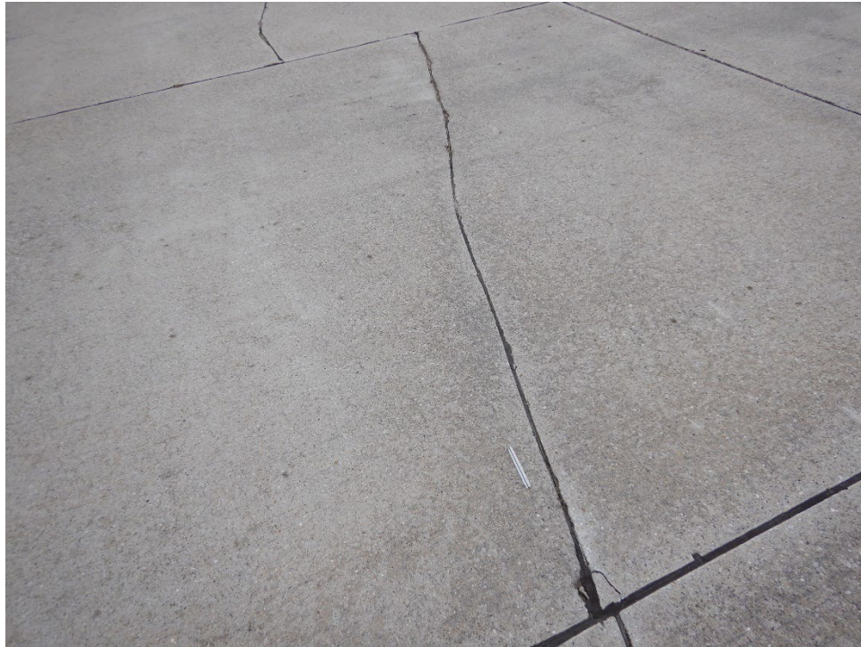
TH01BP-01. LTD Cracking (Sample Unit No. 01).
