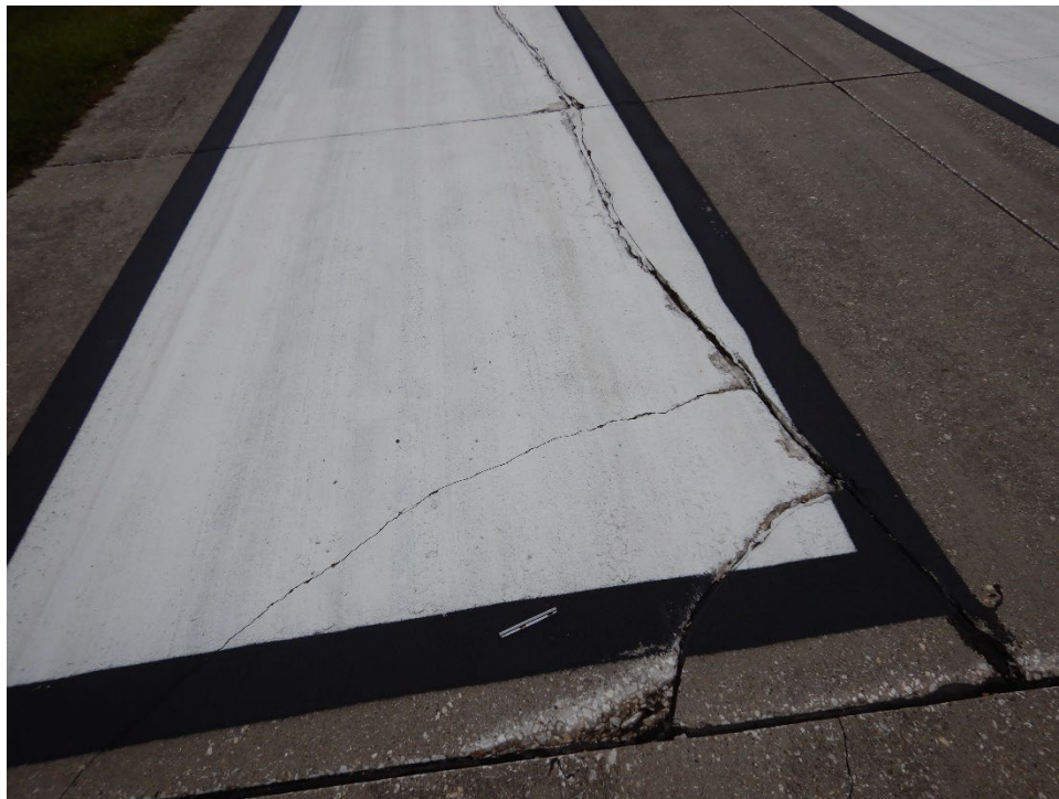
R18BP-01. Shattered Slab (Sample Unit No. 05).
