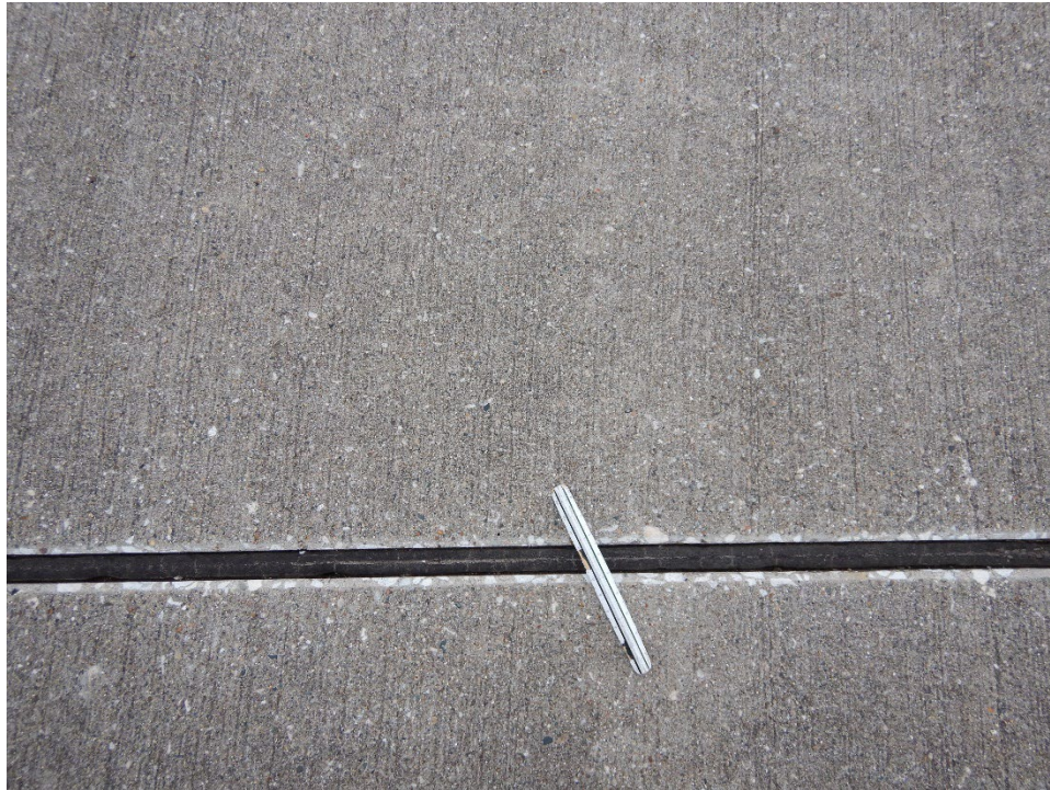
R18BP-01. Joint Seal Damage (Sample Unit No. 95).
