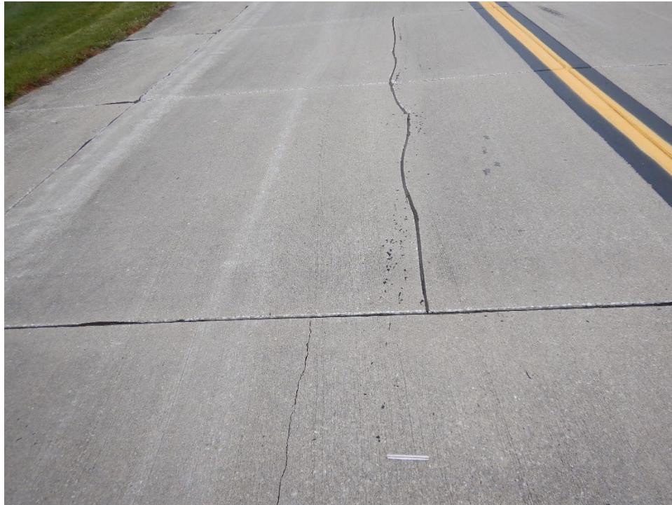
T01BP-01. LTD Cracking (Sample Unit No. 02).
