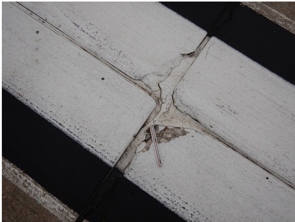
R18BP-01. Corner Spalling (Sample Unit No. 55).
