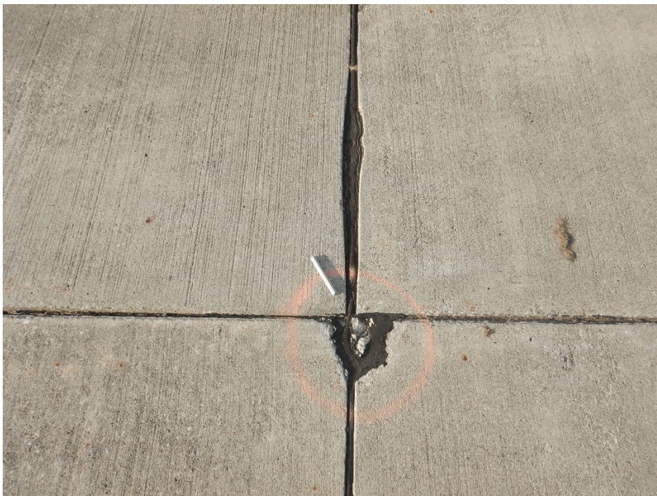
TA3BO-01. Corner Spalling (Sample Unit No. 02).
