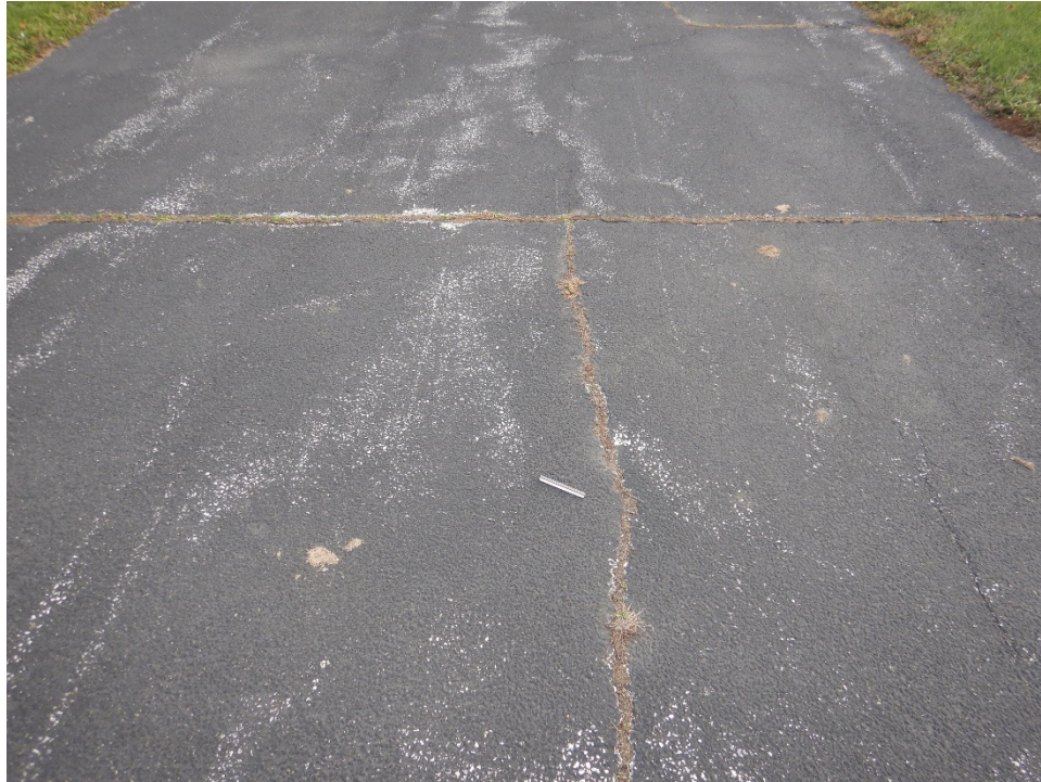
TH01BO-01. L&T Cracking (Sample Unit No. 02).
