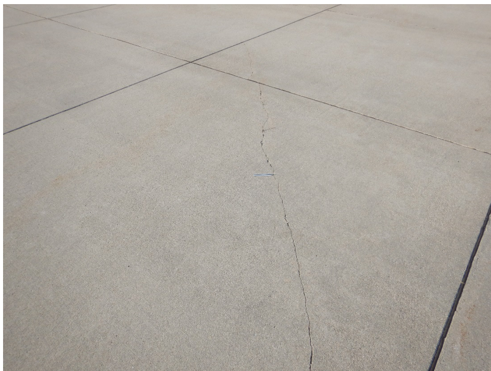
A01BO-04. LTD Cracking (Additional Sample Unit No. 07).
