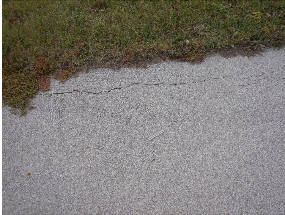
TH02BO-04. L&T Cracking (Sample Unit No. 02).
