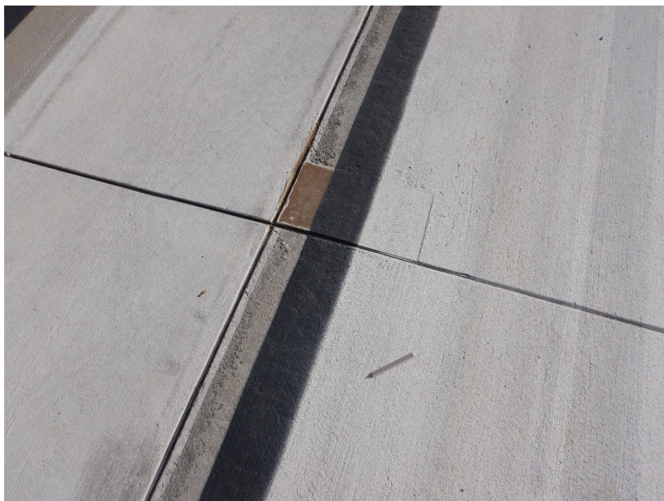
R15BO-02. Small Patching (Sample Unit No. 37).
