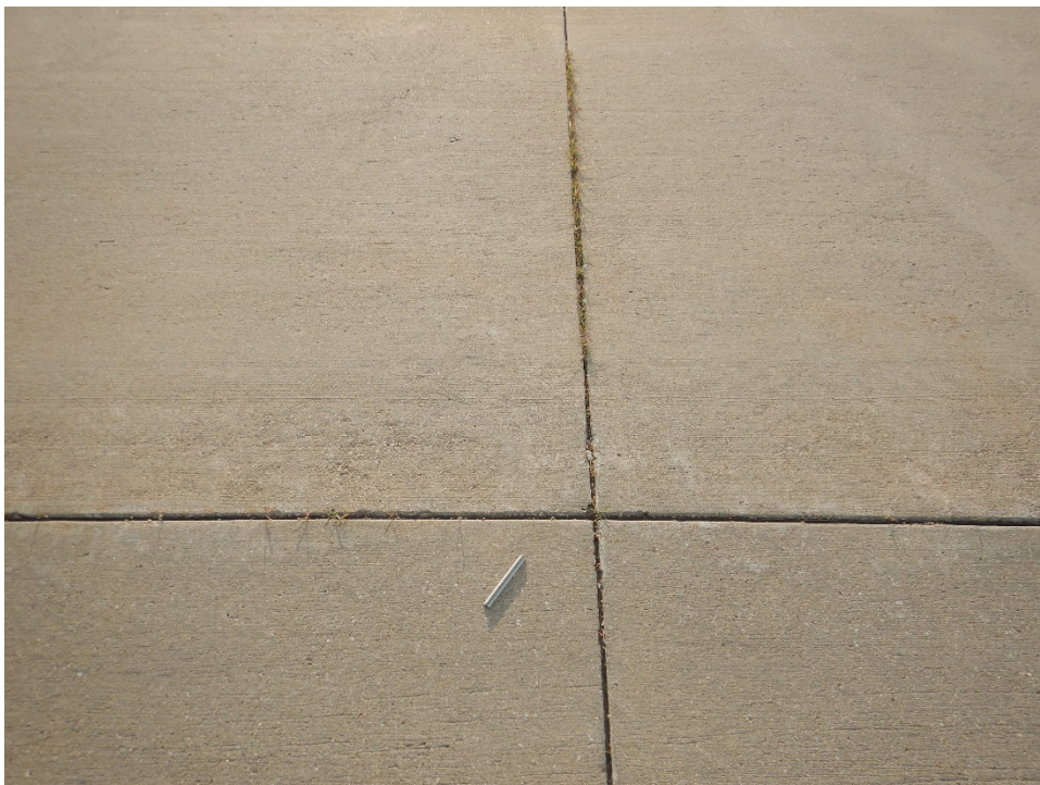
A01BO-02. Joint Seal Damage (Sample Unit No. 29).
