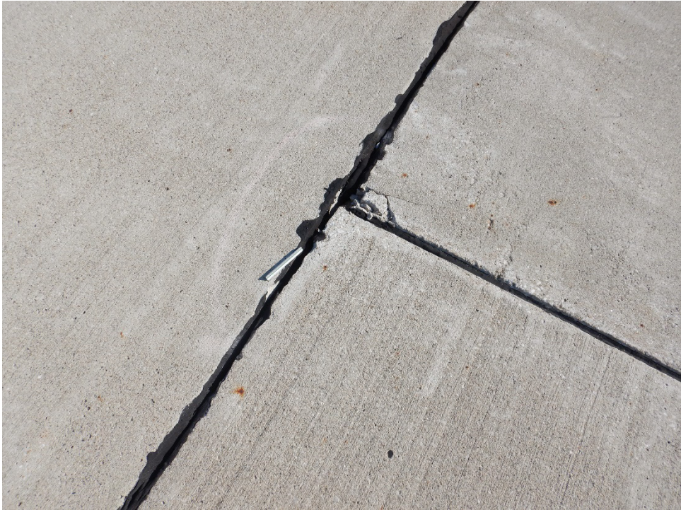
TA1BO-01. Corner Spalling (Sample Unit No. 01).
