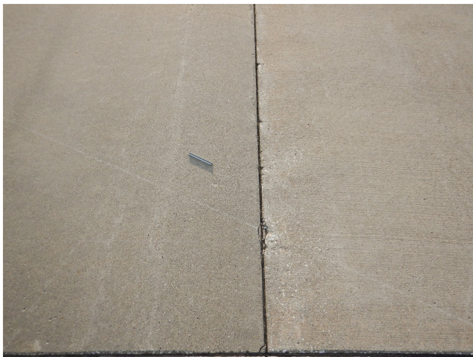
A01BO-03. Joint Seal Damage (Sample Unit No. 03).
