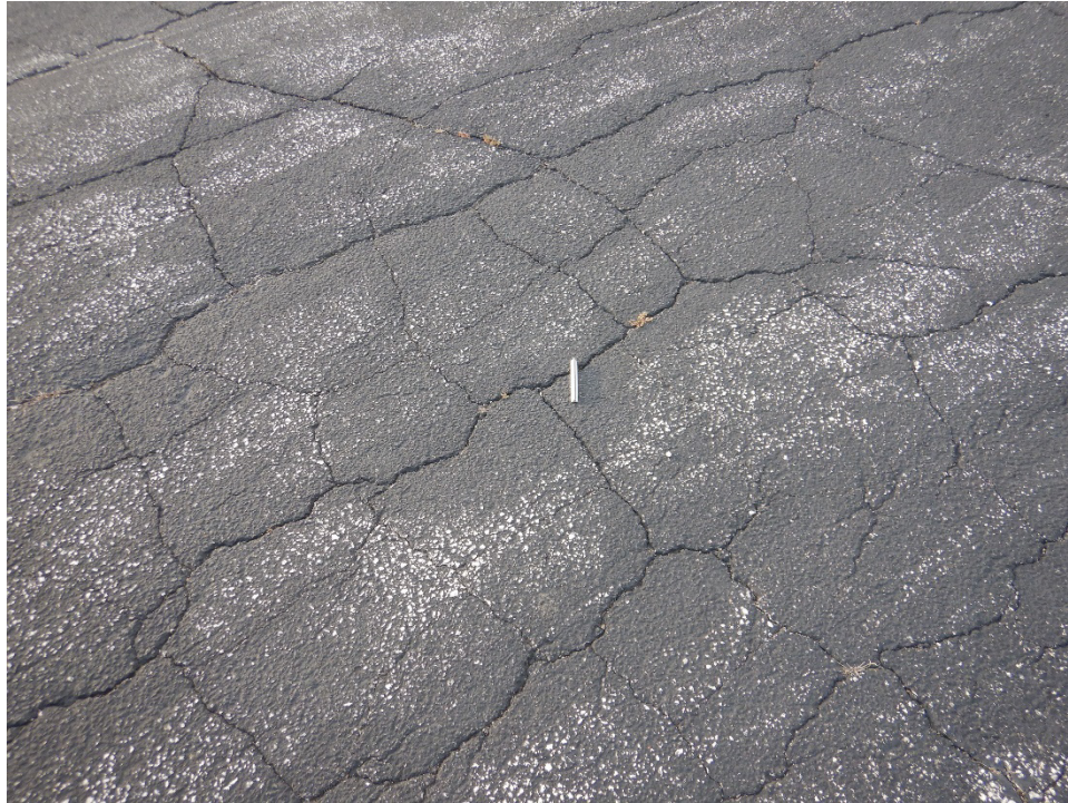
TH02BO-02. Alligator Cracking (Sample Unit No. 01).
