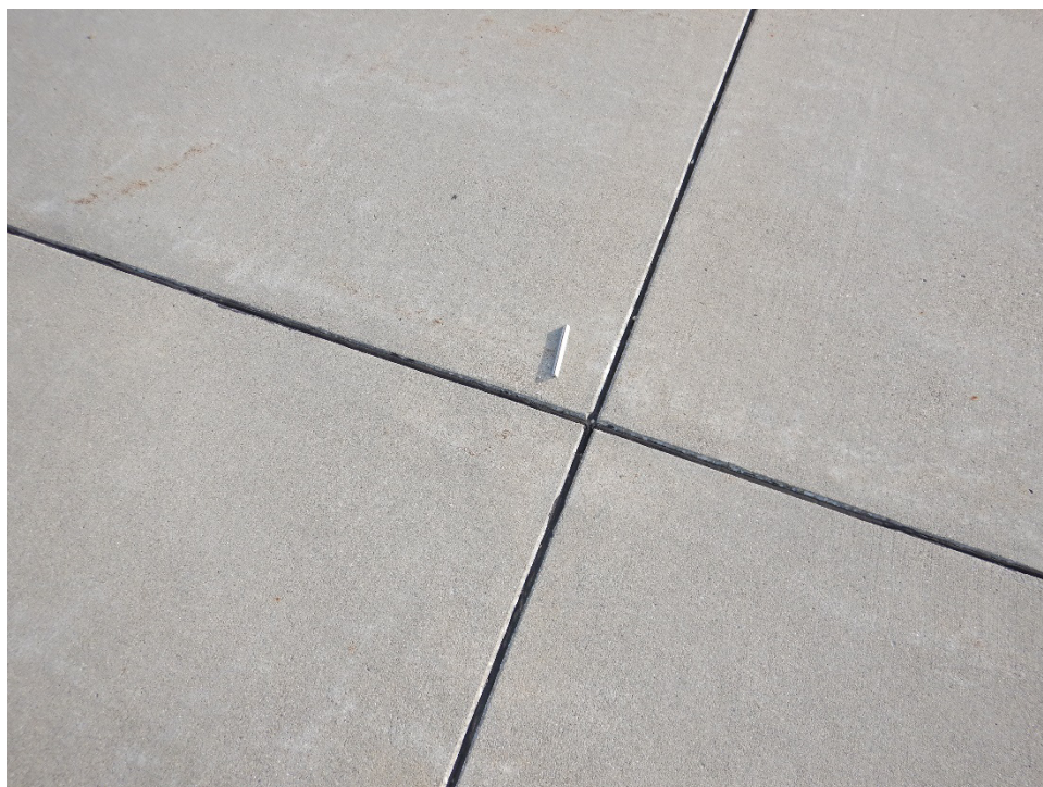
TA2BO-01. Joint Seal Damage (Sample Unit No. 02).
