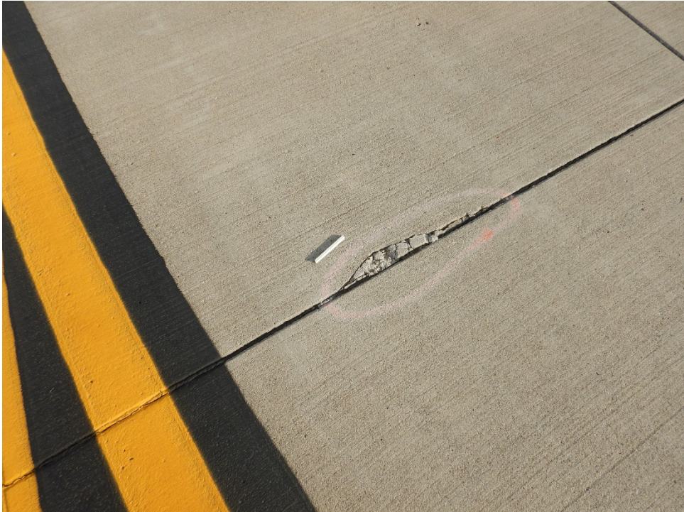
TA2BO-02. Joint Spalling (Sample Unit No. 04).
