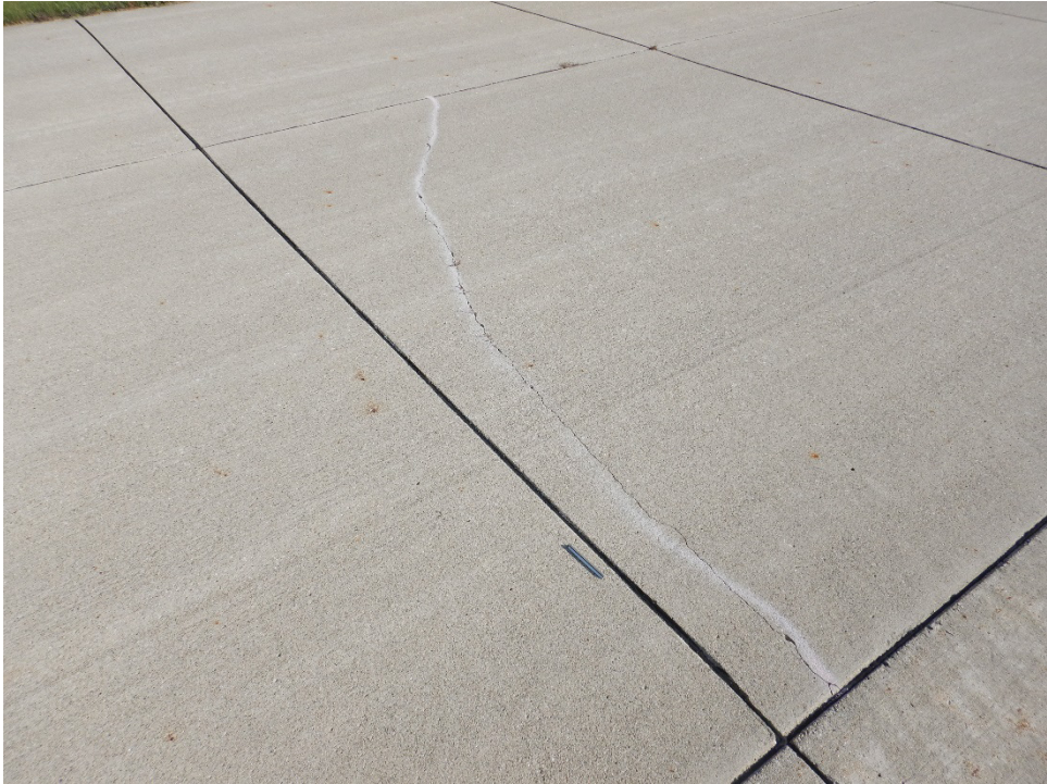
R15BO-01. LTD Cracking (Sample Unit No. 59).
