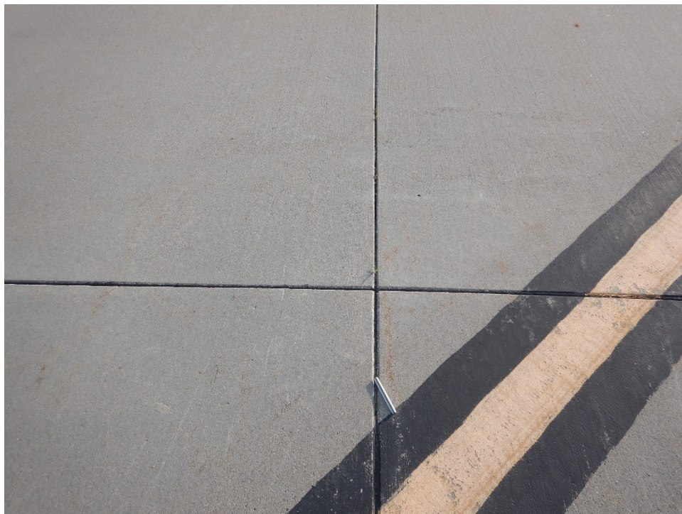
A01BO-01. Joint Seal Damage (Sample Unit No. 08).
