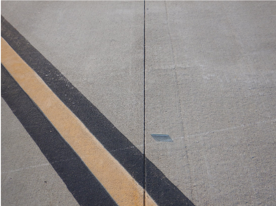
TH02BO-01. Joint Seal Damage (Sample Unit No. 03).
