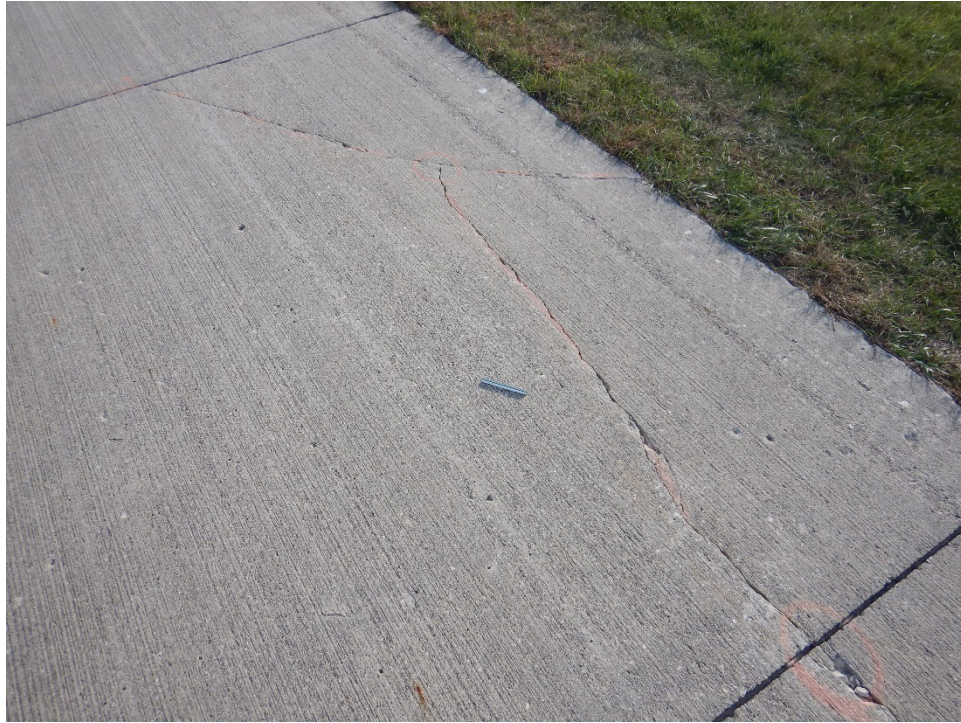
TABO-01. LTD Cracking (Sample Unit No. 33).
