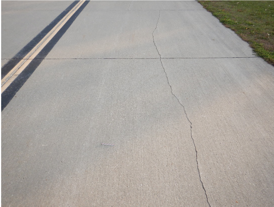
TH01BO-03. LTD Cracking (Sample Unit No. 10).
