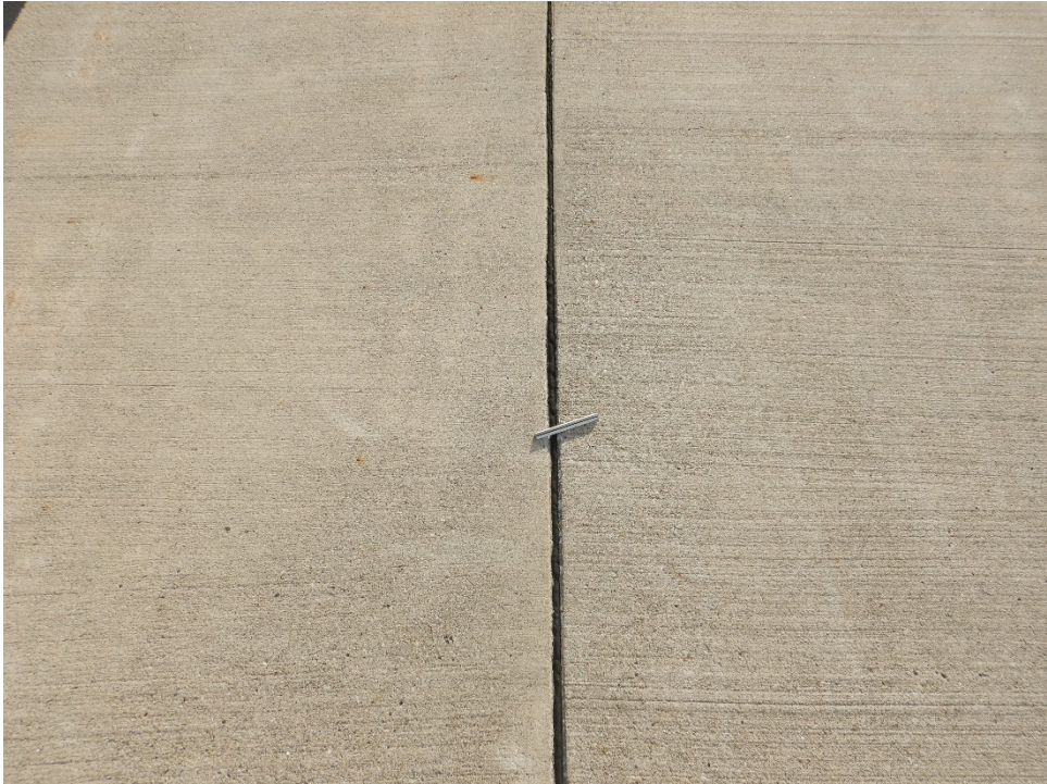
R02BO-01. Joint Seal Damage (Sample Unit No. 02).
