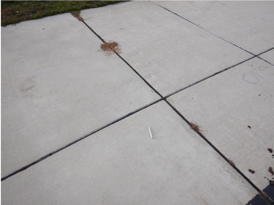
TH02BO-03. Joint Seal Damage (Sample Unit No. 05).
