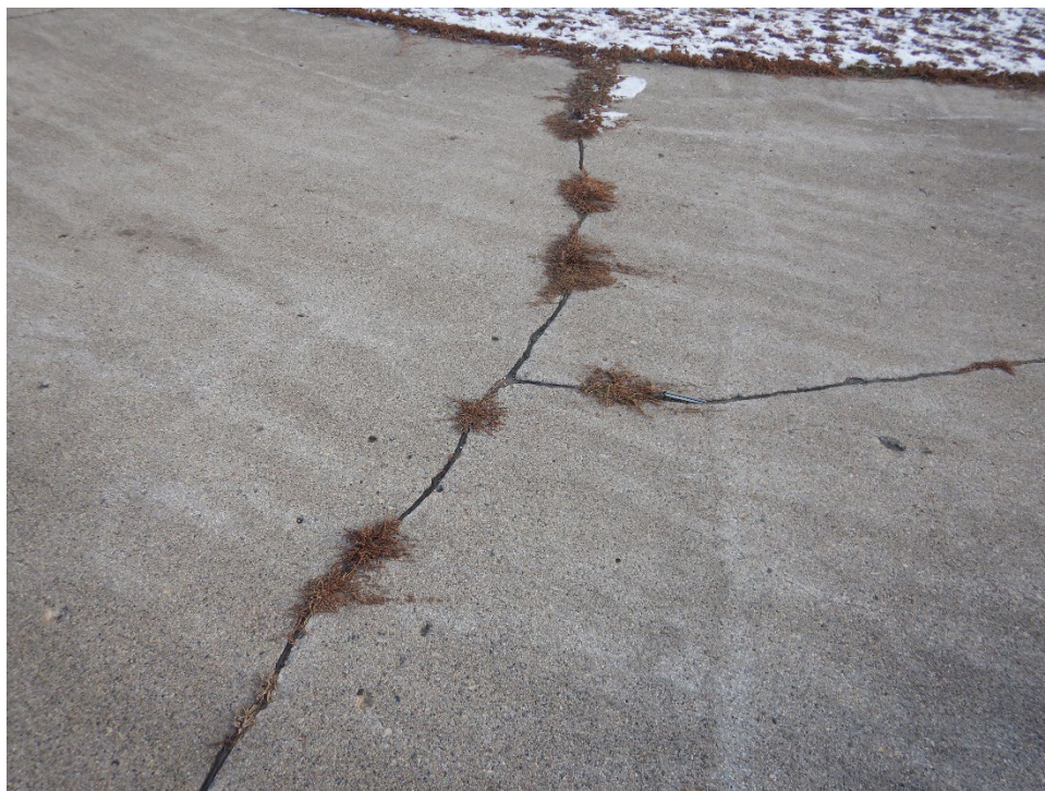
TH01CK-03. LTD Cracking (Sample Unit No. 04).
