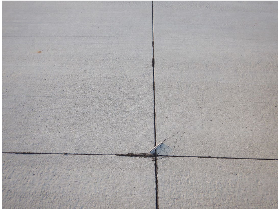
T02CK-01. Joint Seal Damage (Sample Unit No. 03).
