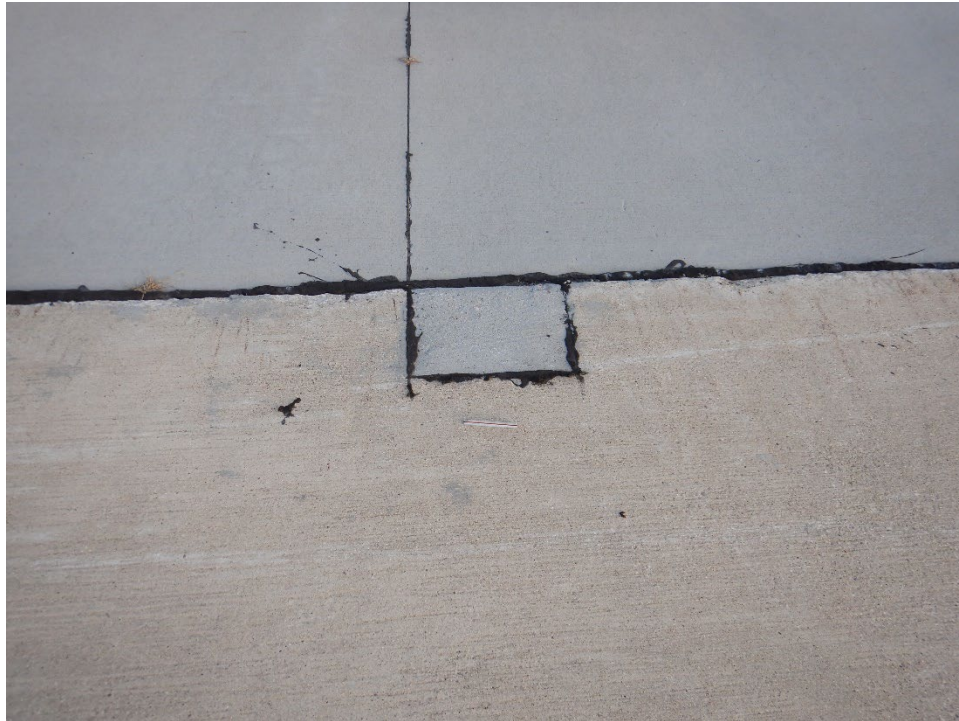
T01CK-01. Small Patching (Sample Unit No. 05).
