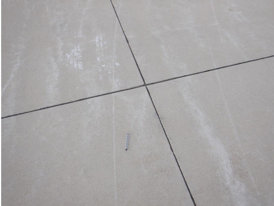
TH02CK-03. Joint Seal Damage (Sample Unit No. 01).
