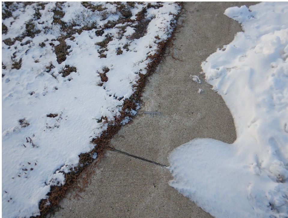
TH01CK-01. Joint Spalling (Sample Unit No. 02).
