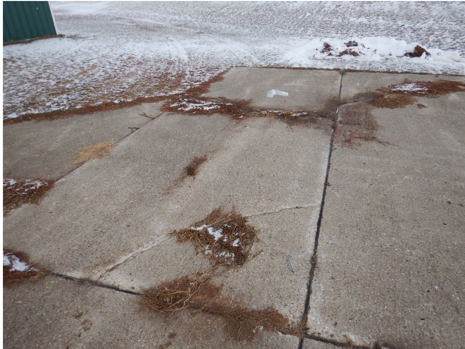
TH02CK-02. Shattered Slab (Sample Unit No. 03).
