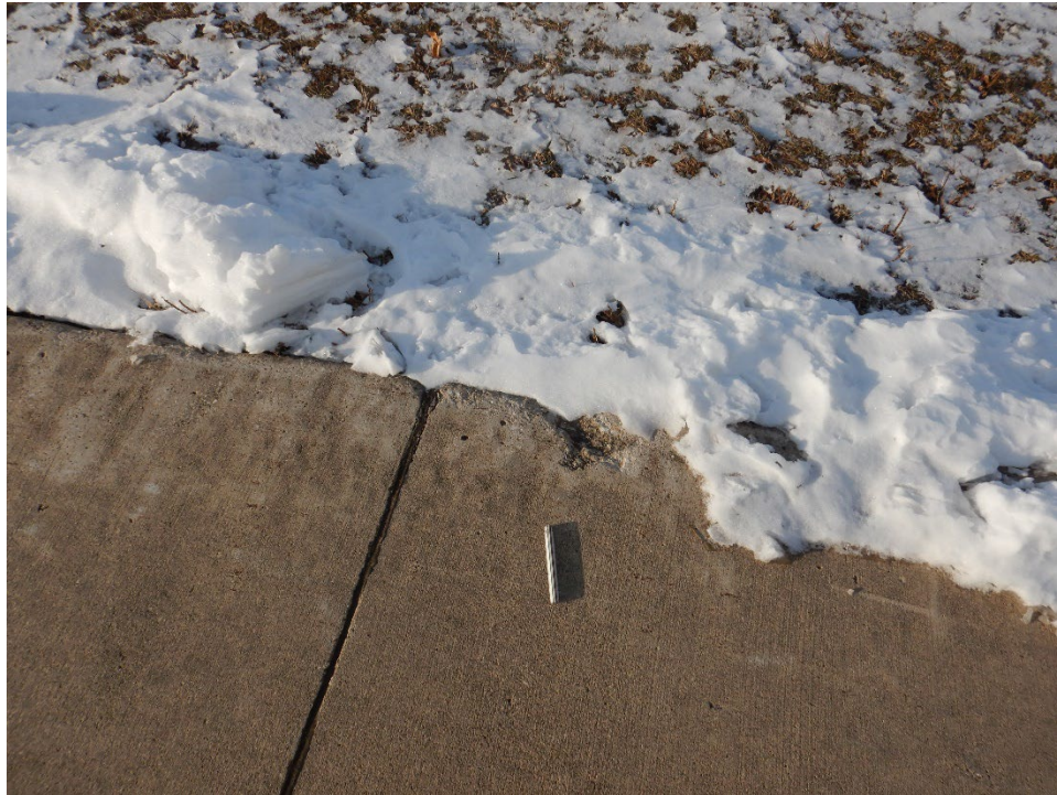
TH02CK-01. Joint Spalling (Sample Unit No. 01).
