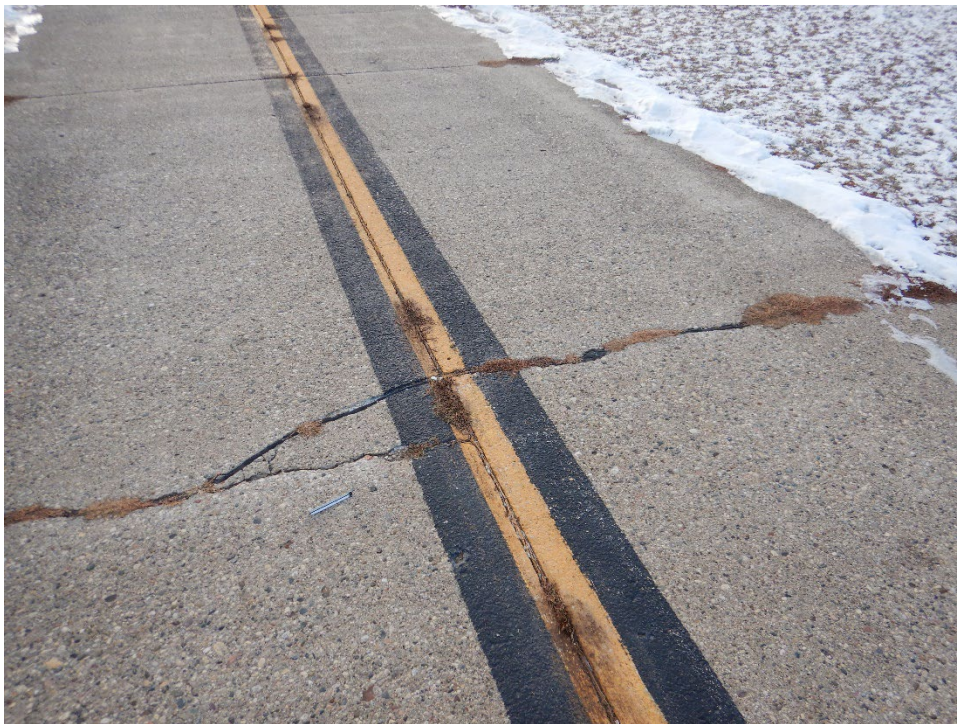
TH01CK-02. LTD Cracking (Sample Unit No. 01).
