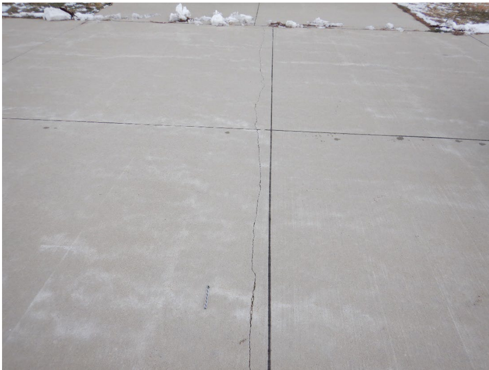
TH02CK-03. LTD Cracking (Sample Unit No. 02).
