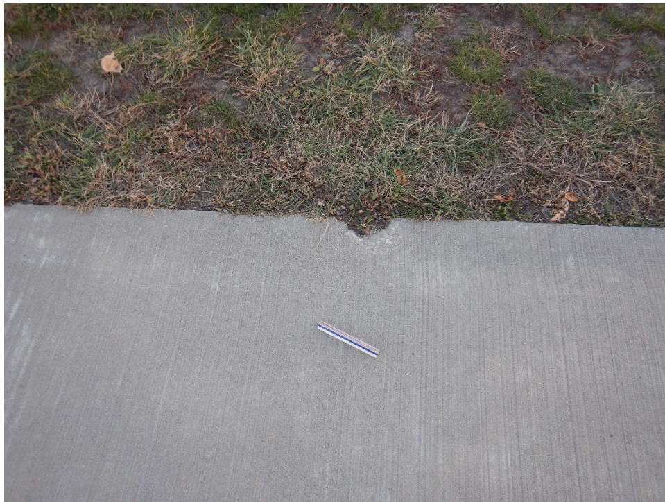
TH01CD-02. Joint Spalling (Sample Unit No. 05).
