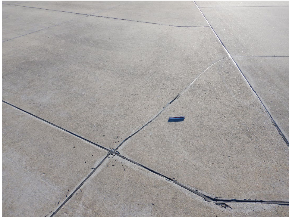
R13CD-02. LTD Cracking (Sample Unit No. 01).
