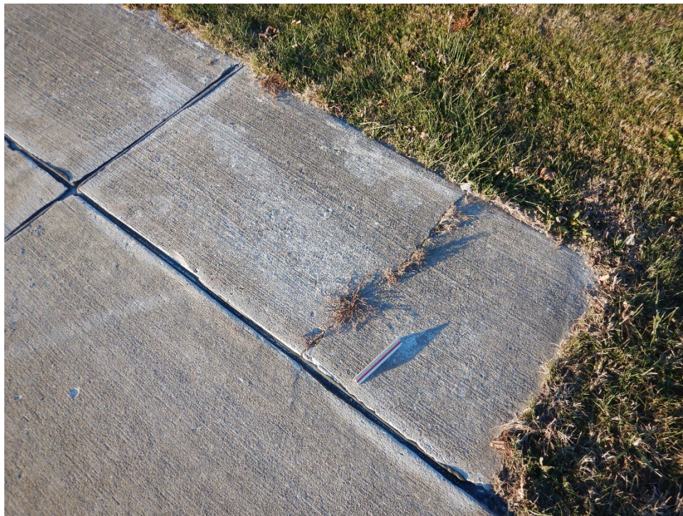
T01CD-01. LTD Cracking (Sample Unit No. 07).
