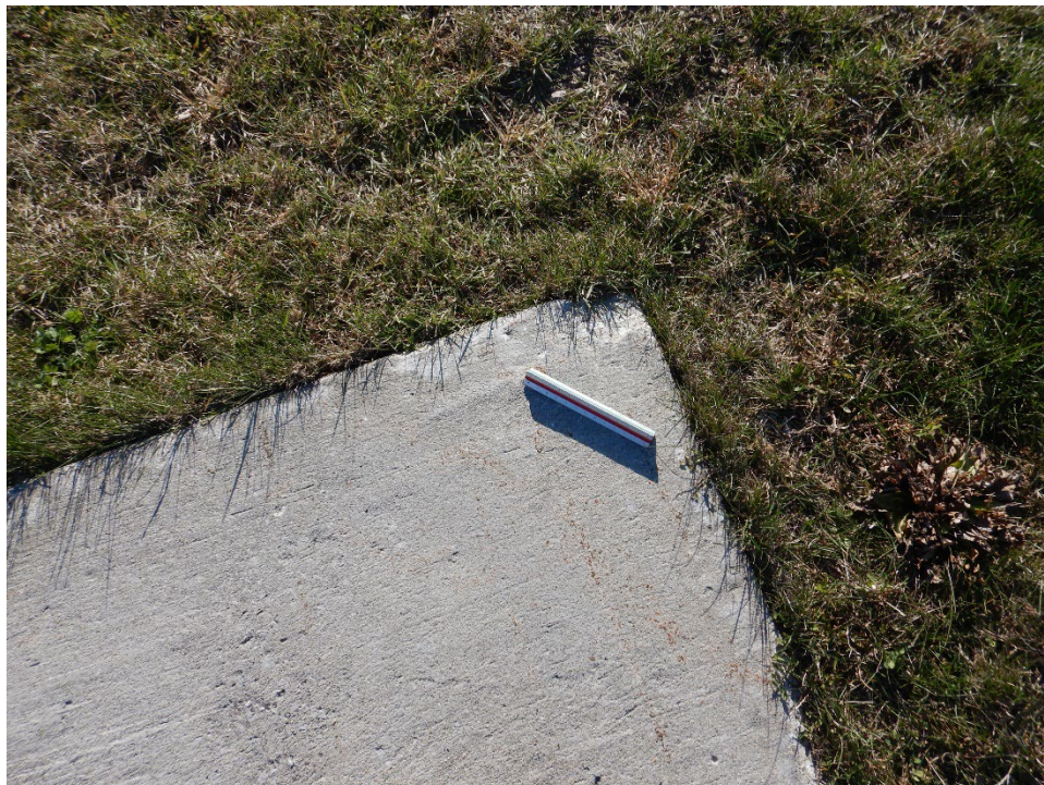
T03CD-01. Corner Spalling (Sample Unit No. 06).
