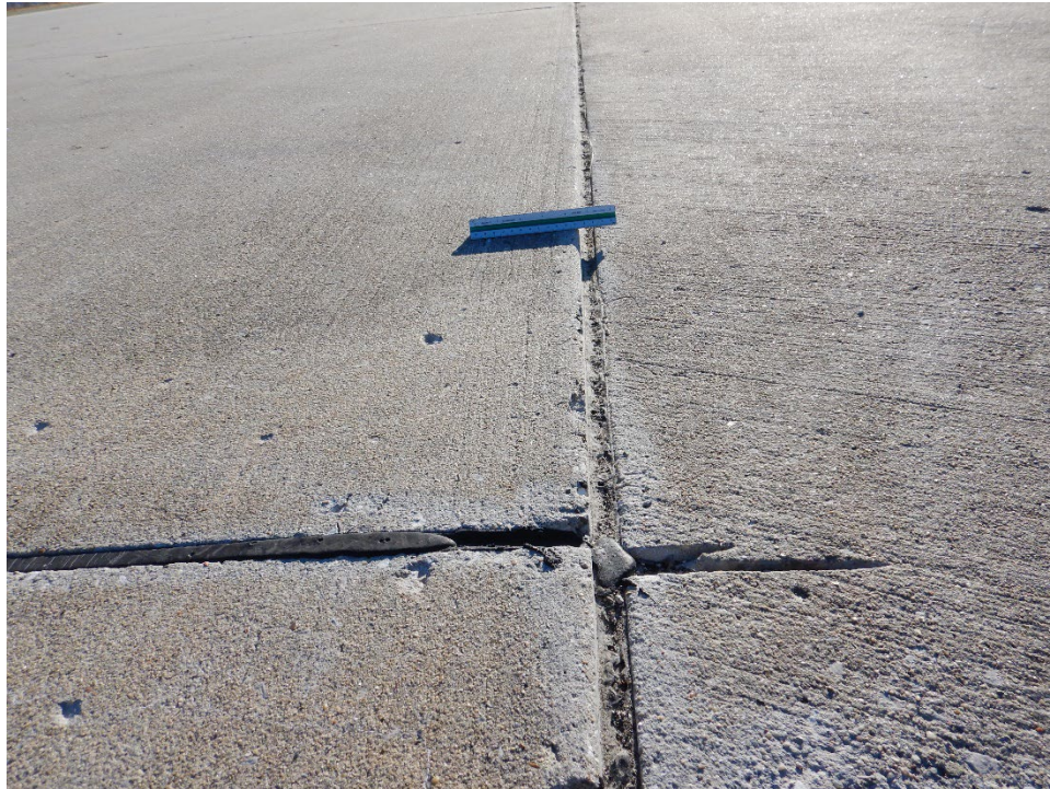
R13CD-01. Faulting (Sample Unit No. 01).
