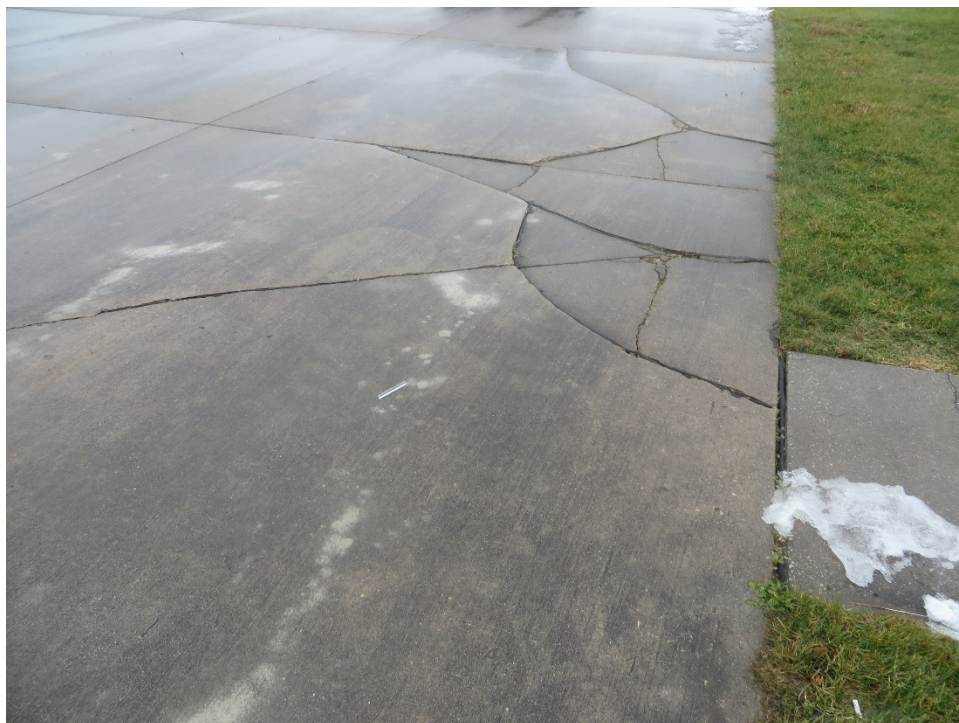
A01CO-01. Shattered Slab (Additional Sample Unit No. 04).
