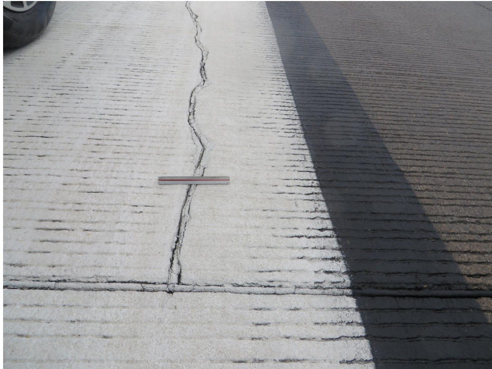
R18CO-01. LTD Cracking (Sample Unit No. 40).
