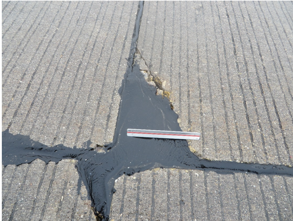
R18CO-01. Corner Spalling (Sample Unit No. 40).
