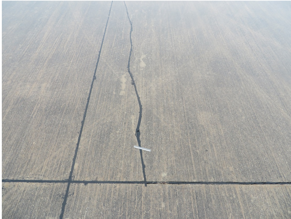
A01CO-01. LTD Cracking (Sample Unit No. 03).
