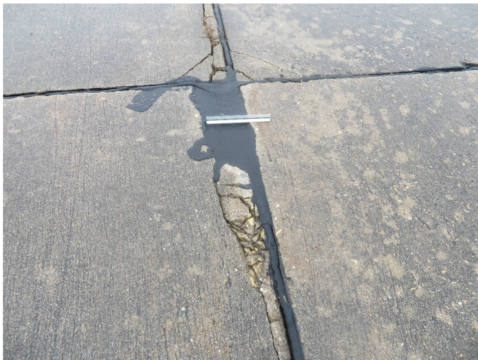
T01CO-01. Joint Spalling (Sample Unit No. 01).
