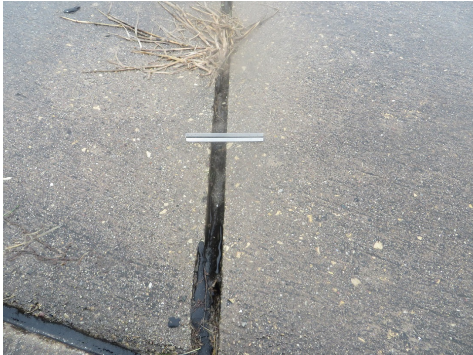
T01CO-01. Joint Seal Damage (Sample Unit No. 03).
