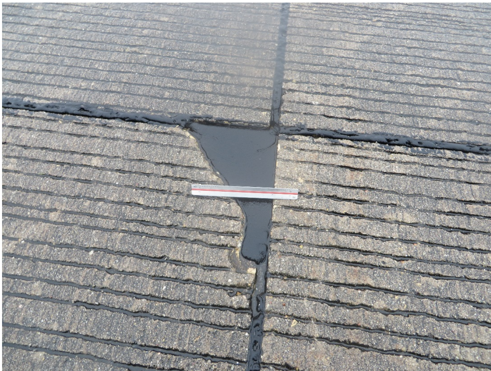
R18CO-01. Corner Spalling (Additional Sample Unit No. 17).
