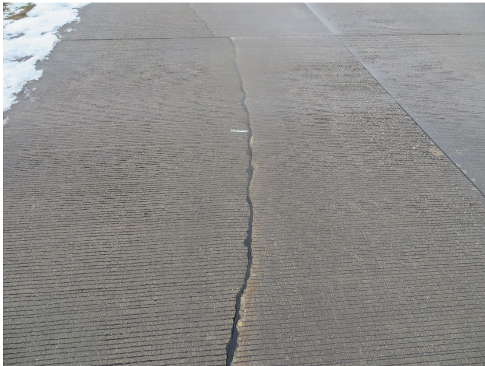
R18CO-01. LTD Cracking (Additional Sample Unit No. 17).
