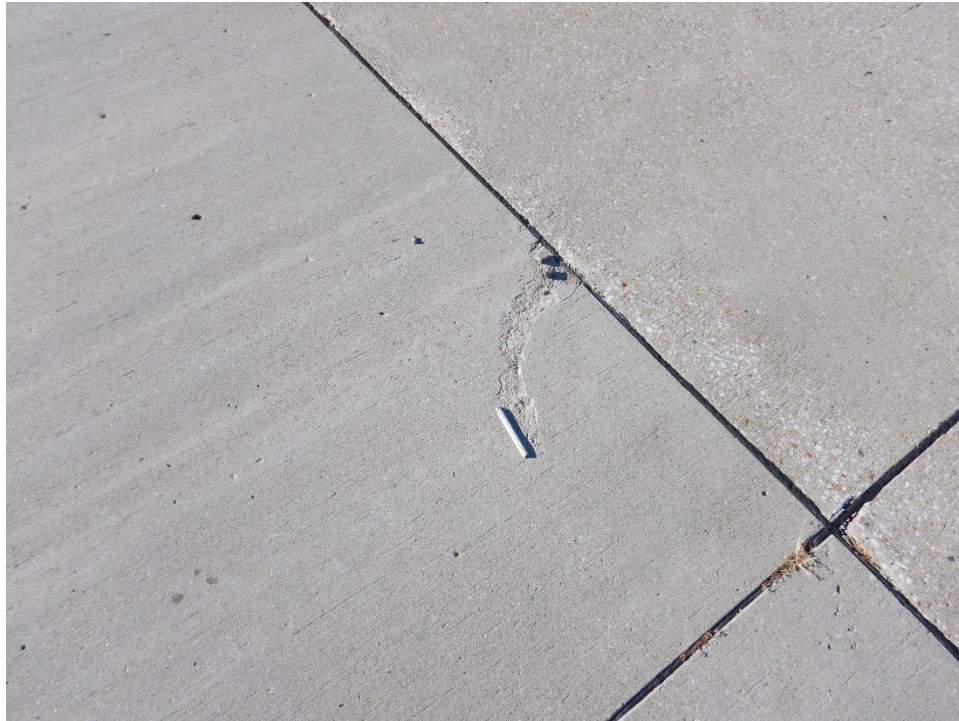
T02CB-03. Joint Spalling (Sample Unit No. 05).
