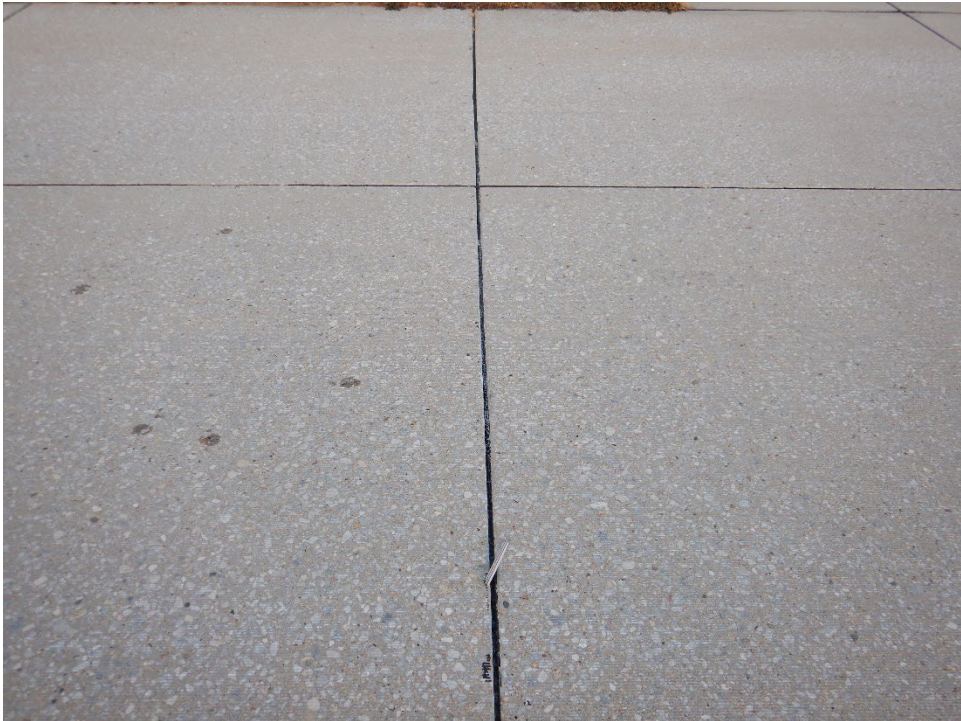
T03CB-01. Joint Seal Damage (Sample Unit No. 03).
