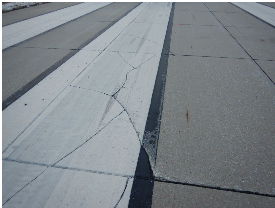
R14CB-01. Shattered Slab (Additional Sample Unit No. 03).
