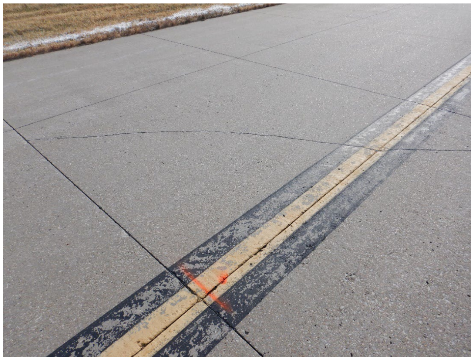
T01CB-01. LTD Cracking (Sample Unit No. 55).
