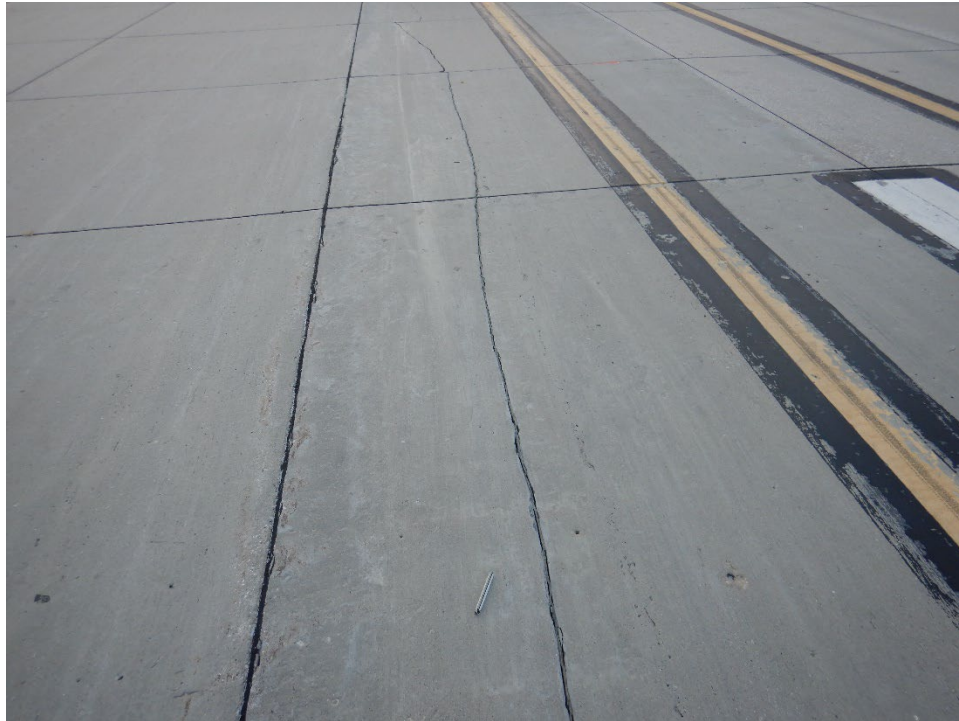
R14CB-01. LTD Cracking (Sample Unit No. 36).
