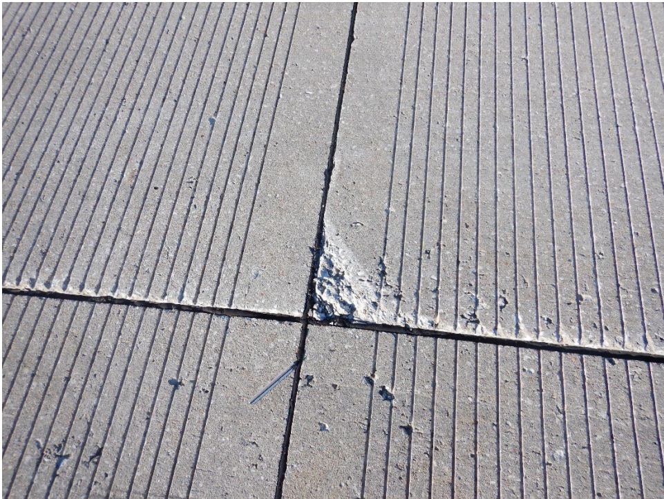
R18CB-01. Corner Spalling (Sample Unit No. 119).
