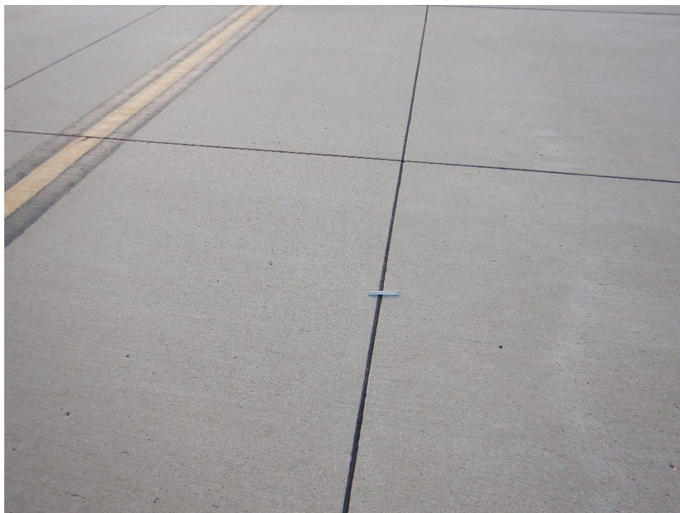
A01CB-01. Joint Seal Damage (Sample Unit No. 23).
