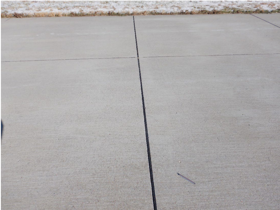
T02CB-02. Joint Seal Damage (Sample Unit No. 02).
