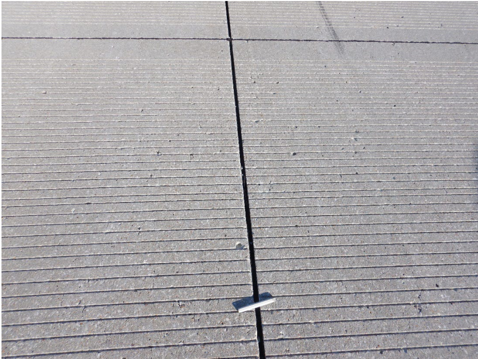
R18CB-01. Joint Seal Damage (Sample Unit No. 99).
