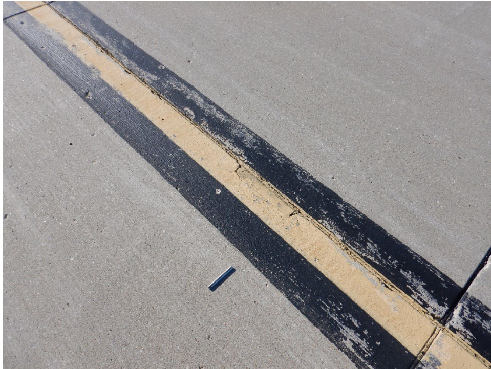
T04CB-03. Small Patching (Sample Unit No. 11).
