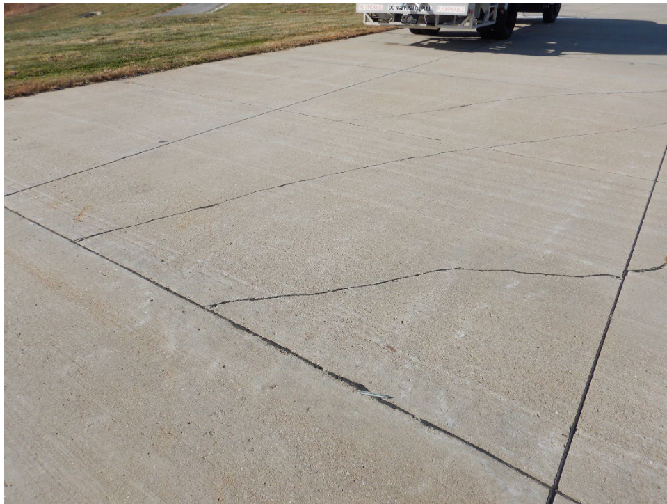
A02CB-01. LTD Cracking (Sample Unit No. 25).
