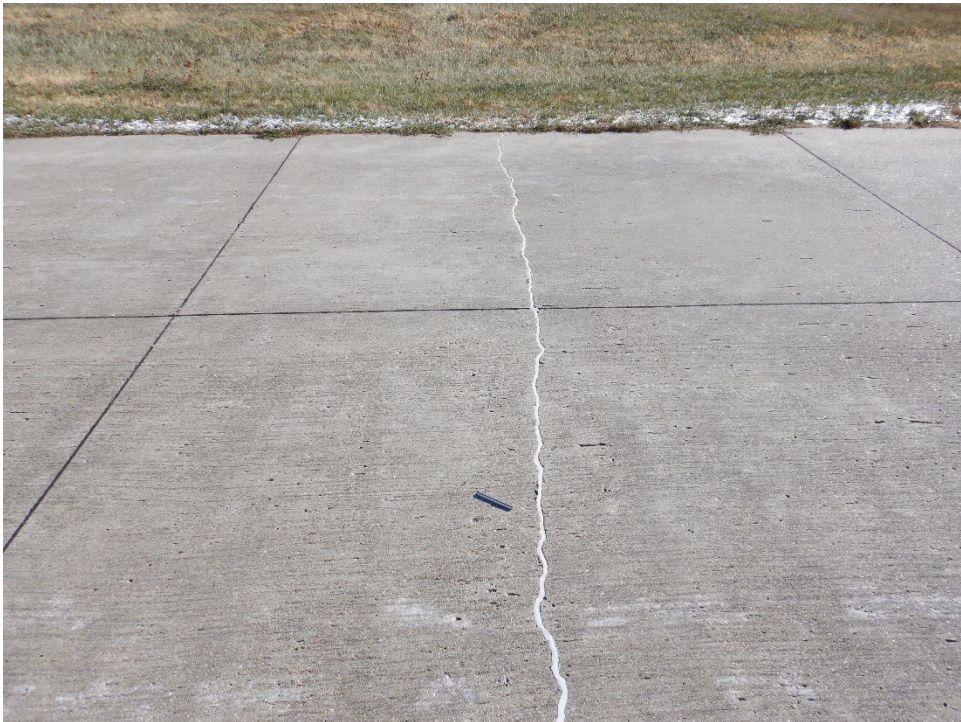
TH01CB-03. LTD Cracking (Sample Unit No. 03).
