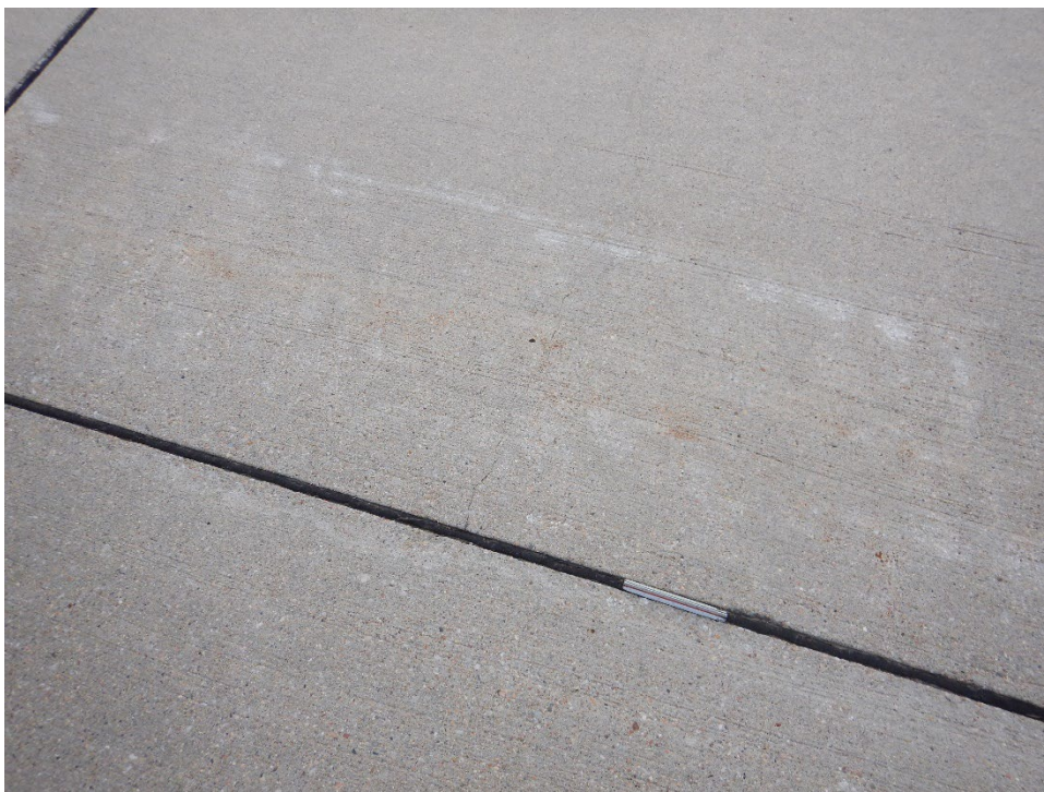
TH01CB-02. Shrinkage Cracking (Sample Unit No. 13).
