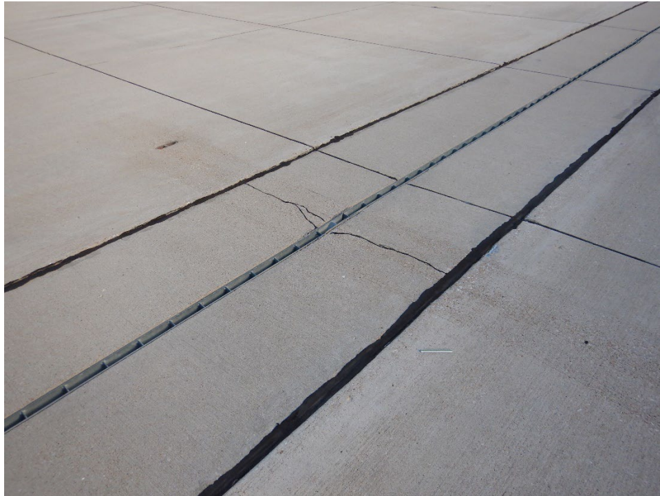
A01CB-01. LTD Cracking (Sample Unit No. 61).
