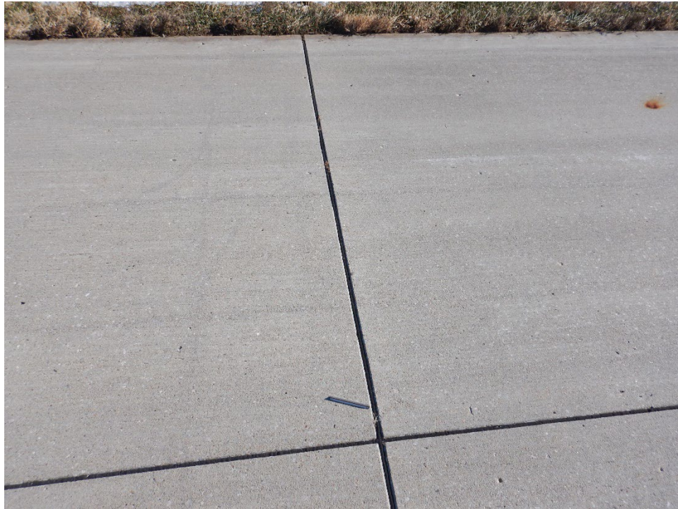
T04CB-02. Joint Seal Damage (Sample Unit No. 08).
