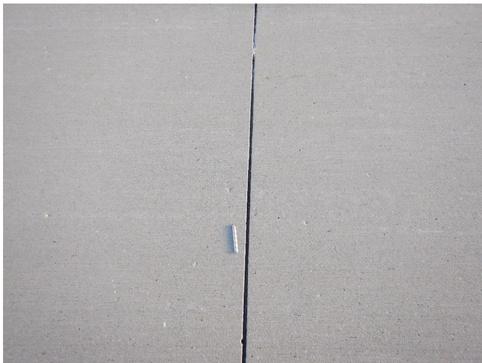
T02CB-01. Joint Seal Damage (Sample Unit No. 24).
