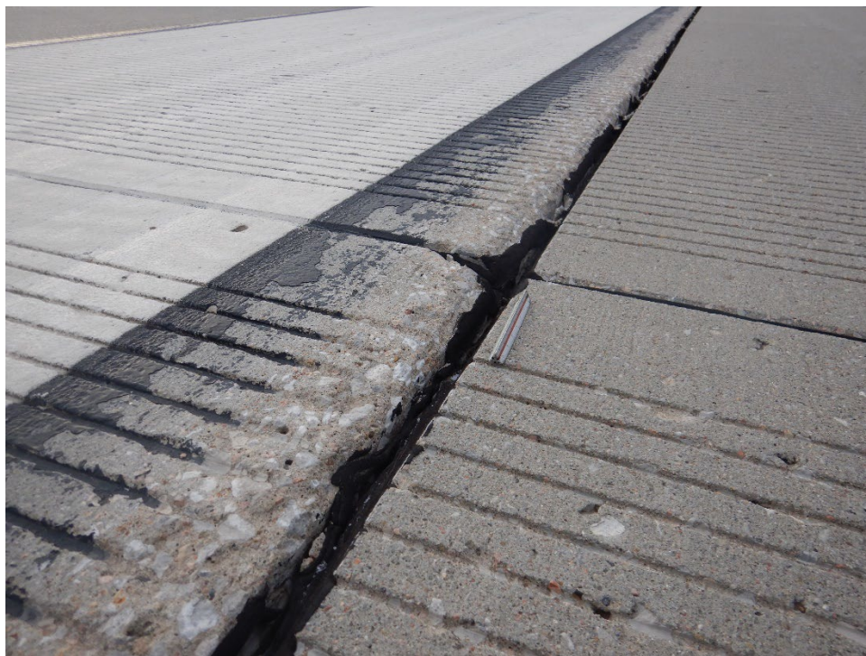
R14CB-02. Faulting (Sample Unit No. 15).
