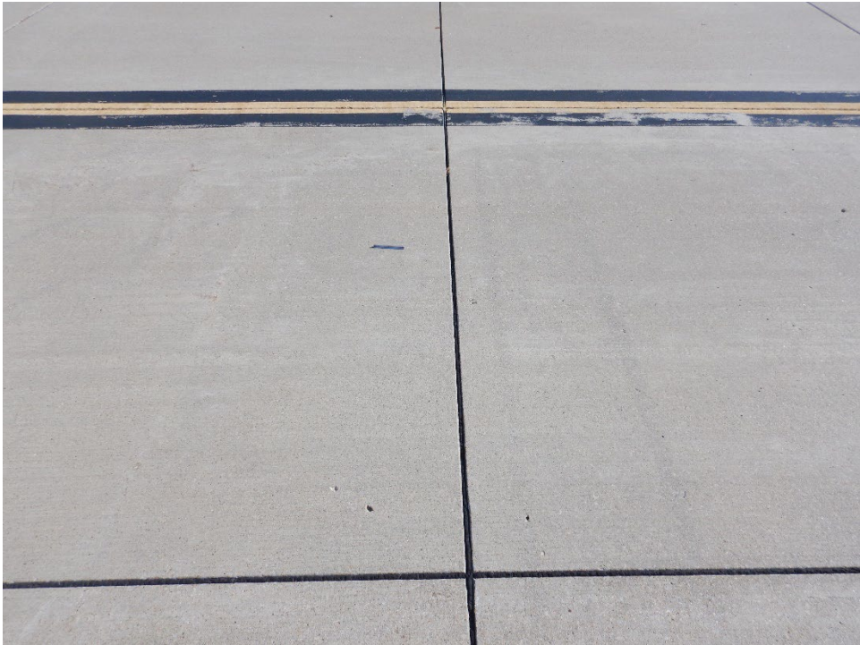
T05CB-01. Joint Seal Damage (Sample Unit No. 12).
