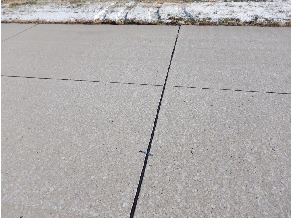
T04CB-01. Joint Seal Damage (Sample Unit No. 09).
