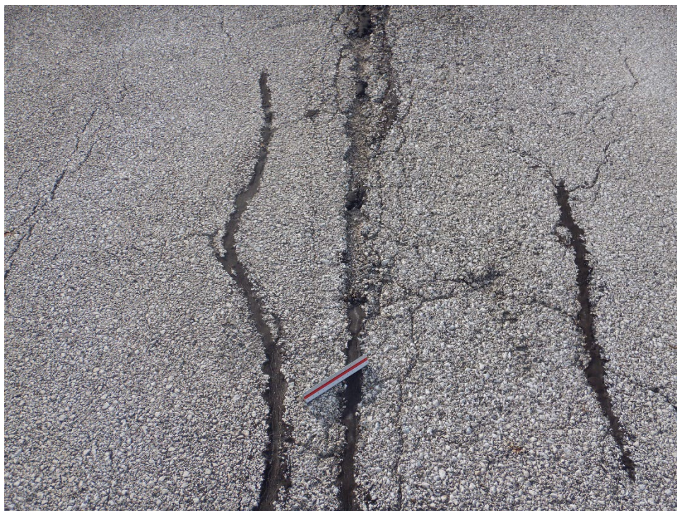
R16CT-02. L&T Cracking (Sample Unit No. 20).
