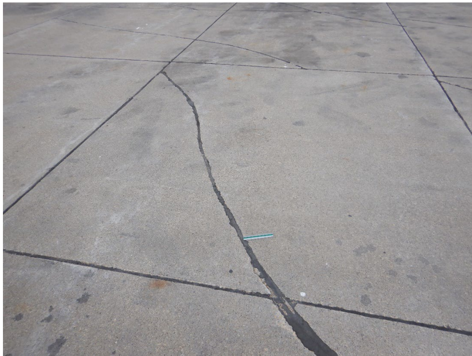
A01CT-01. LTD Cracking (Sample Unit No. 12).
