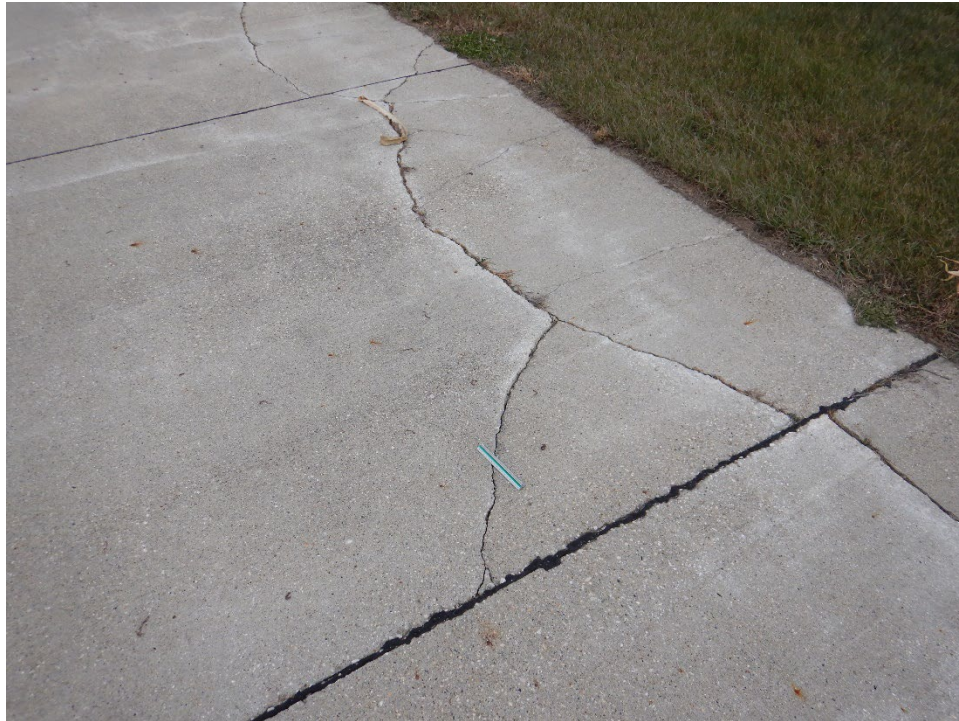
TH01CT-01. Shattered Slab (Sample Unit No. 03).
