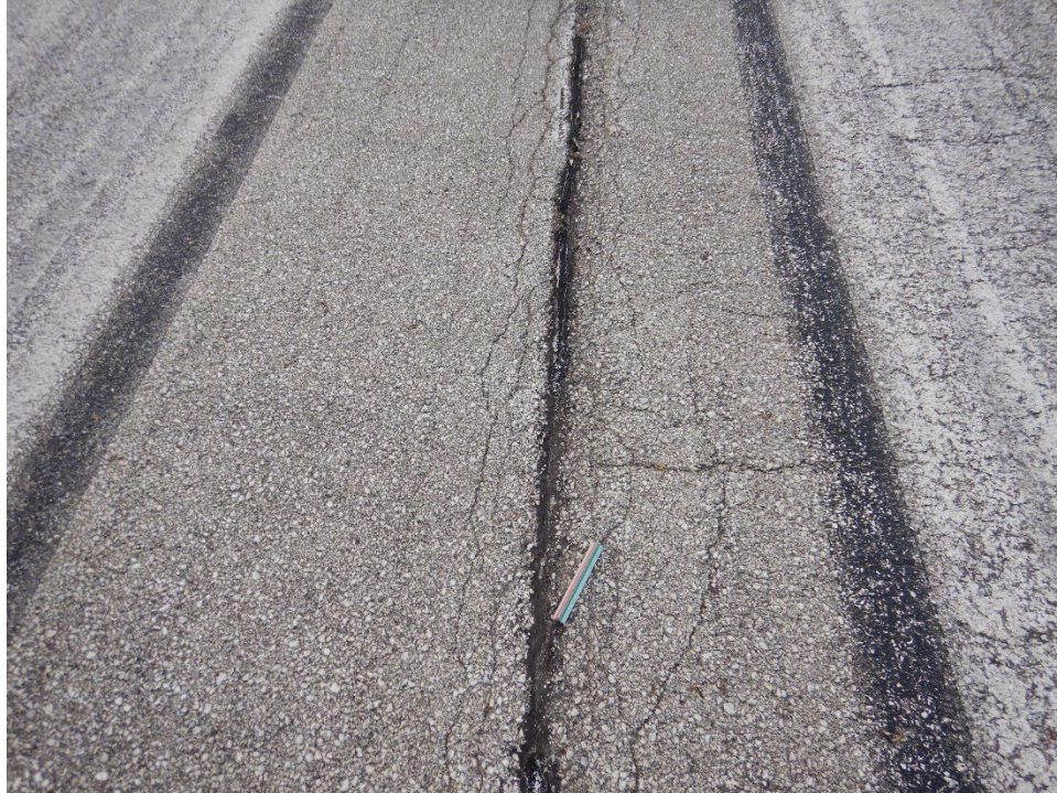
R16CT-03. L&T Cracking (Sample Unit No. 44).
