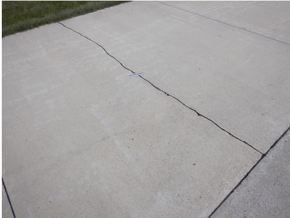
TH01CT-02. LTD Cracking (Sample Unit No. 04).
