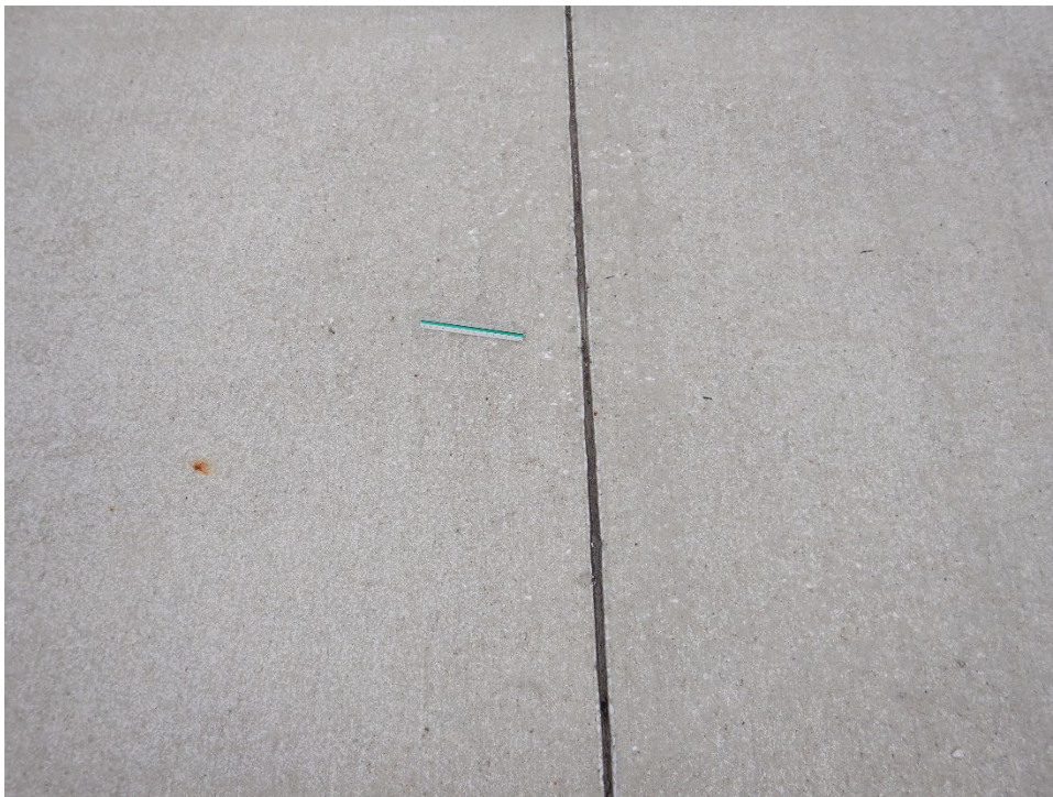
R16CT-04. Joint Seal Damage (Sample Unit No. 04).
