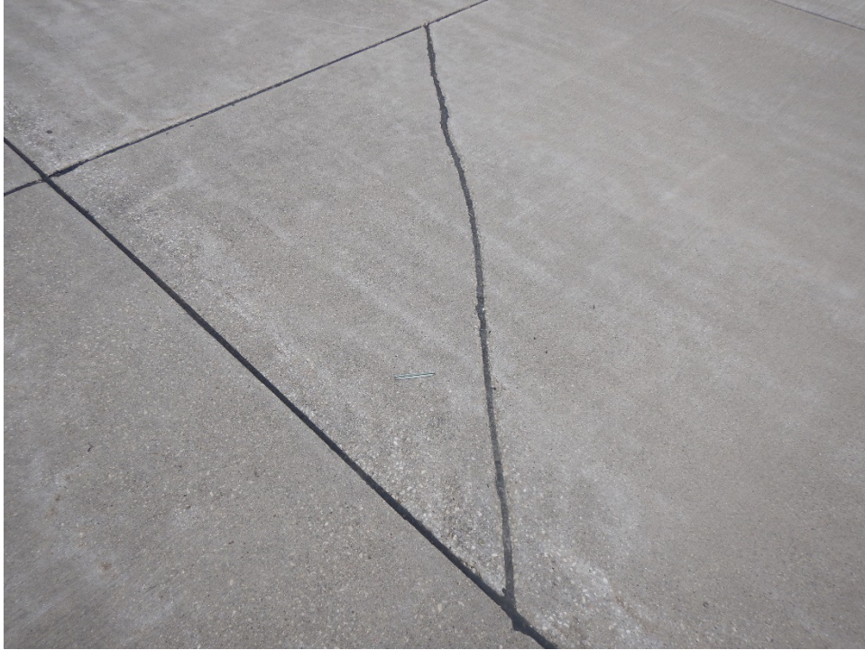
A01DE-03. LTD Cracking (Sample Unit No. 04).
