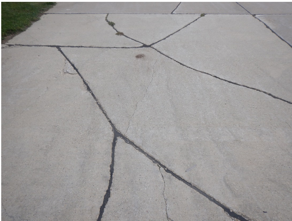
A01DE-03. Shattered Slab (Sample Unit No. 01).
