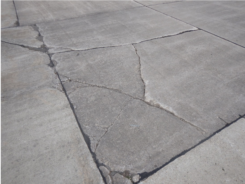
A01DE-04. Shattered Slab (Sample Unit No. 03).
