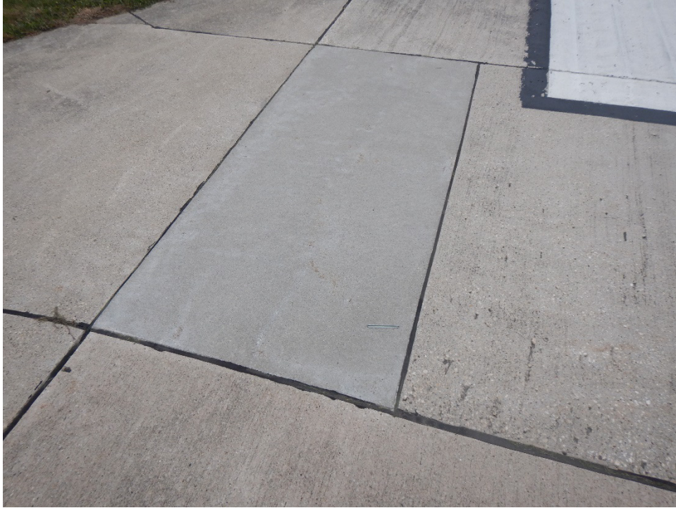
R11DE-02. Large Patching (Sample Unit No. 08).
