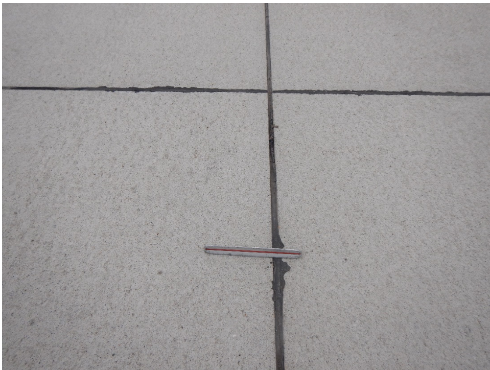
TH02DE-01. Joint Seal Damage (Sample Unit No. 05).
