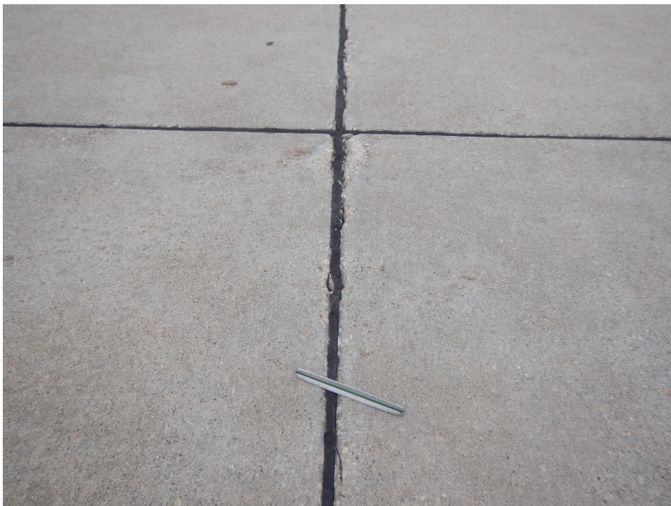
T02DE-01. Joint Seal Damage (Sample Unit No. 05).
