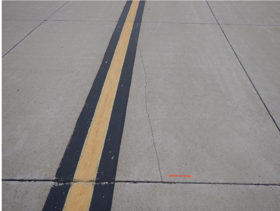
T02DE-01. LTD Cracking (Sample Unit No. 03).
