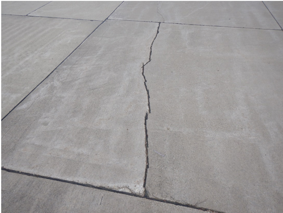
A01DE-04. LTD Cracking (Sample Unit No. 02).
