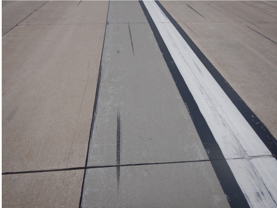
R11DE-01. Large Patching (Sample Unit No. 08).
