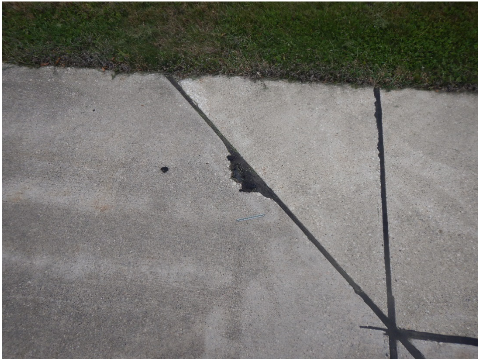
R11DE-03. Small Patching (Sample Unit No. 04).
