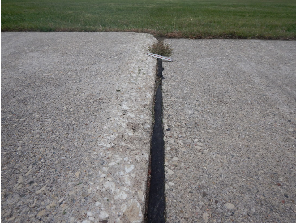
A01DE-04. Faulting (Sample Unit No. 03).
