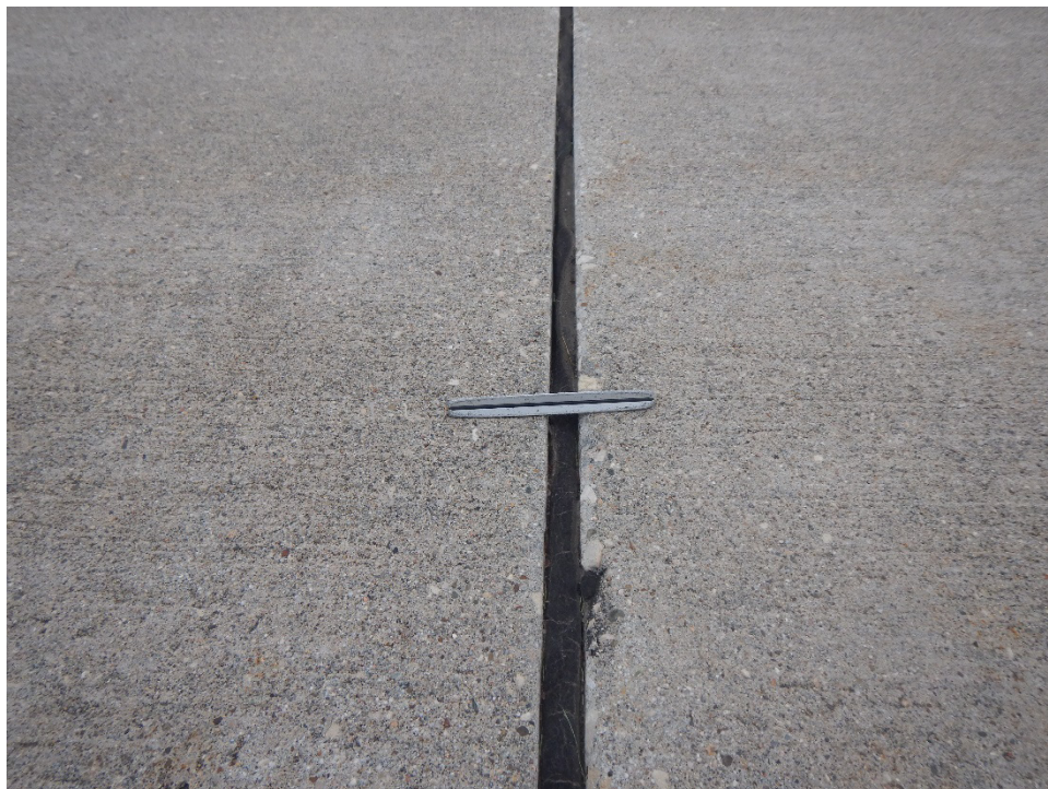
R11DE-01. Joint Seal Damage (Sample Unit No. 12).
