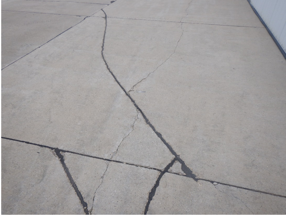
A01DE-01. Shattered Slab (Sample Unit No. 01).
