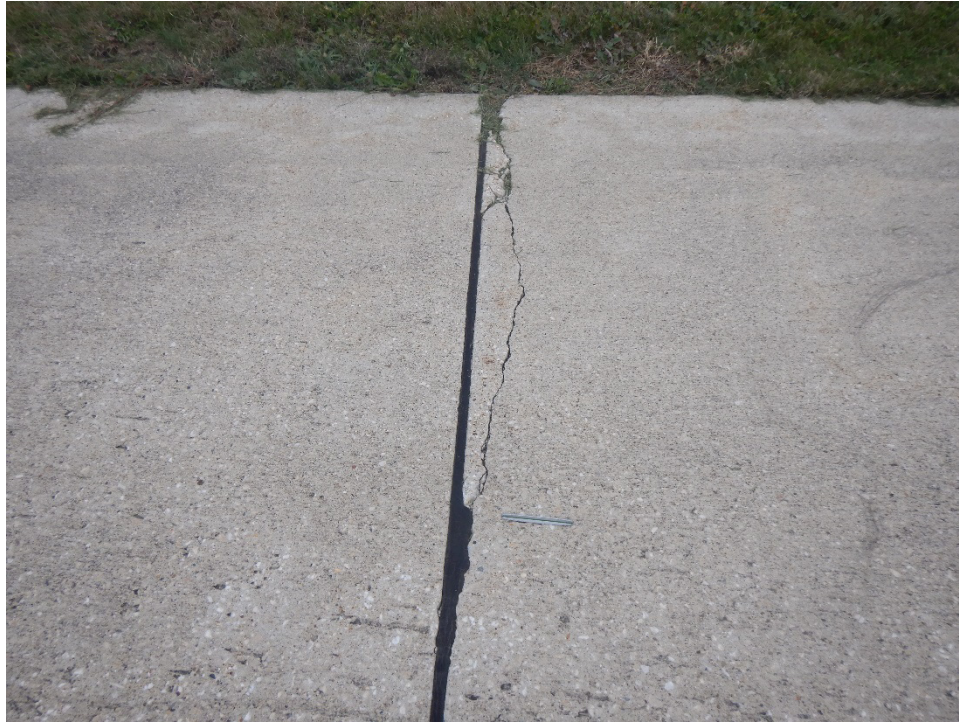
R11DE-02. Joint Spalling (Sample Unit No. 49).
