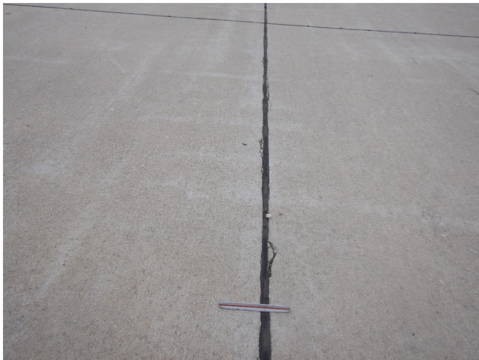
TH01DE-02. Joint Seal Damage (Sample Unit No. 08).
