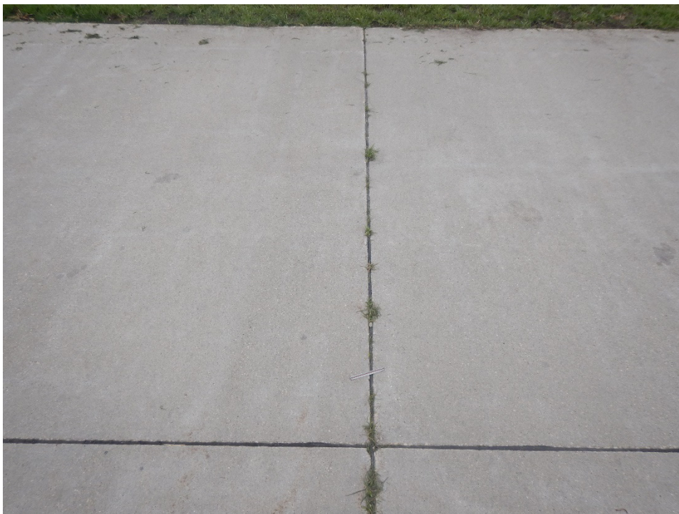
A01DE-06. Joint Seal Damage (Sample Unit No. 09).
