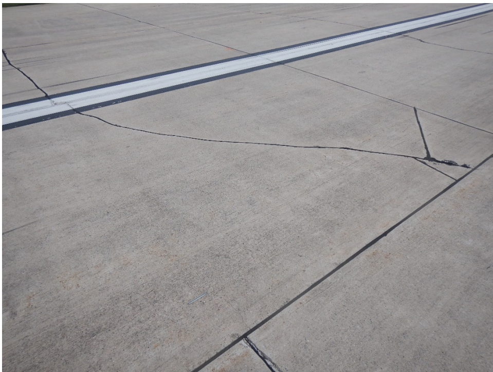
R11DE-02. Shattered Slab (Sample Unit No. 65).
