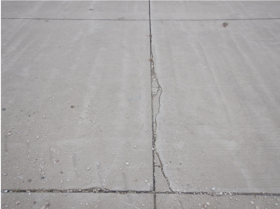
TH01DE-01. Joint Spalling (Sample Unit No. 01).
