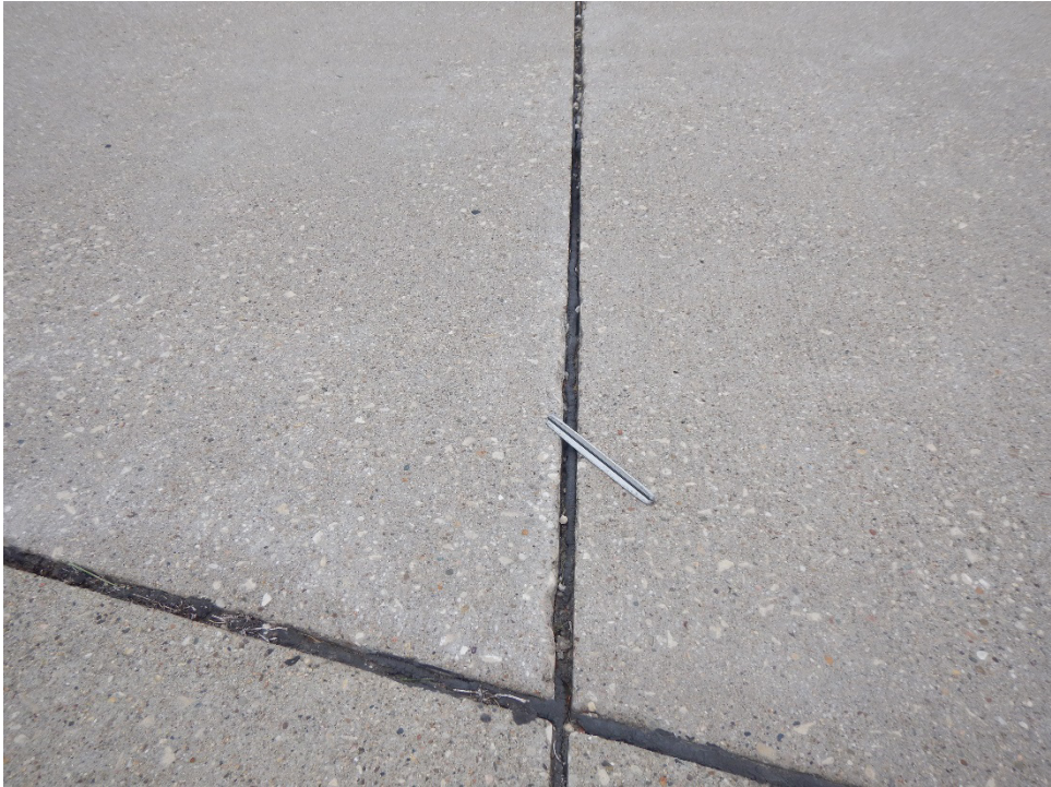
TH01DE-01. Joint Seal Damage (Sample Unit No. 04).
