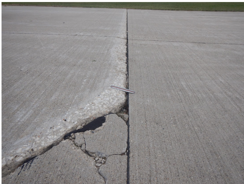
TH01DE-01. Faulting (Sample Unit No. 03).
