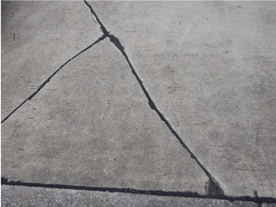
T01DE-01. LTD Cracking (Sample Unit No. 02).
