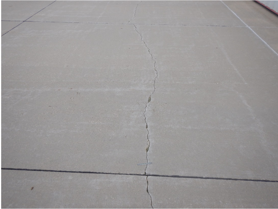
A01DE-06. LTD Cracking (Sample Unit No. 05).
