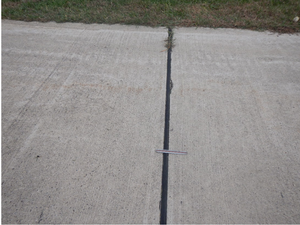
R11DE-05. Joint Seal Damage (Sample Unit No. 02).
