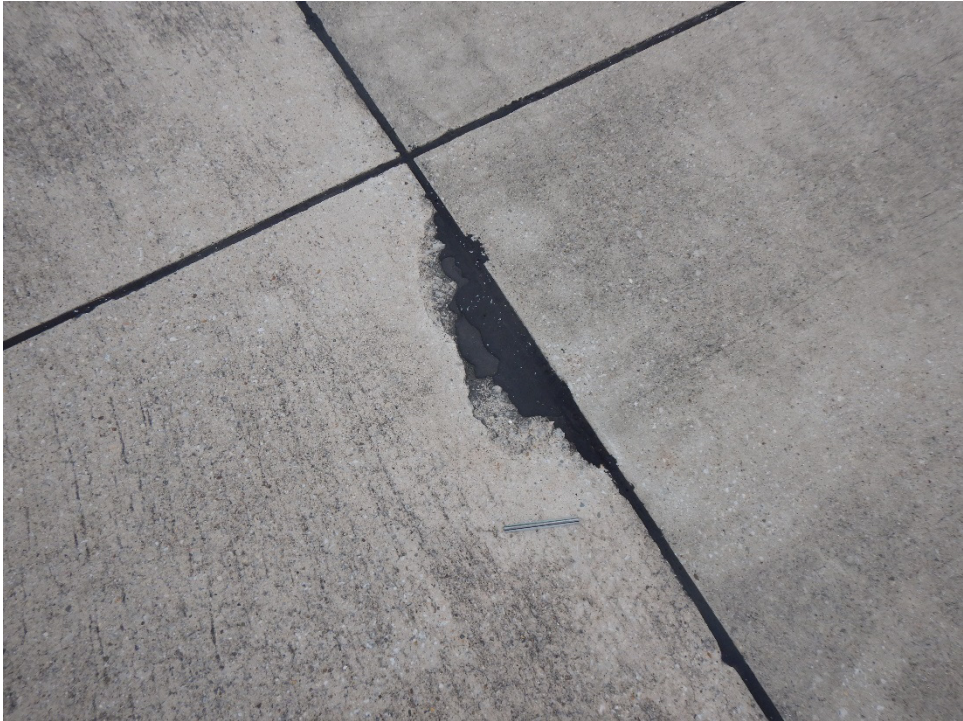
T01DE-01. Joint Spalling (Sample Unit No. 01).
