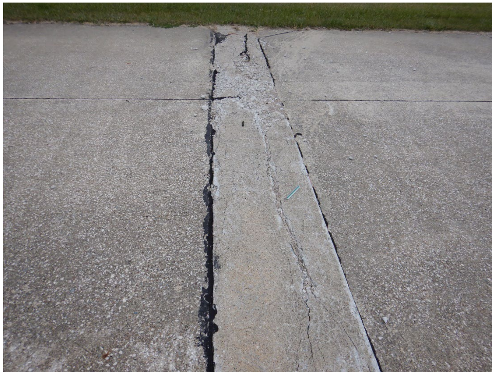
R12DN-04. Large Patching (Additional Sample Unit No. 03).
