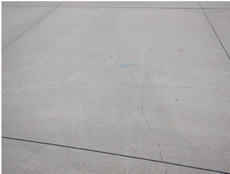
TH01DN-03. LTD Cracking (Sample Unit No. 01).
