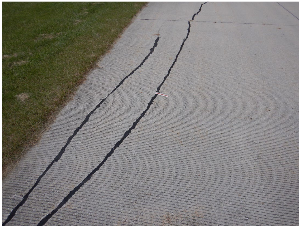
R12DN-01. Shattered Slab (Sample Unit No. 35).
