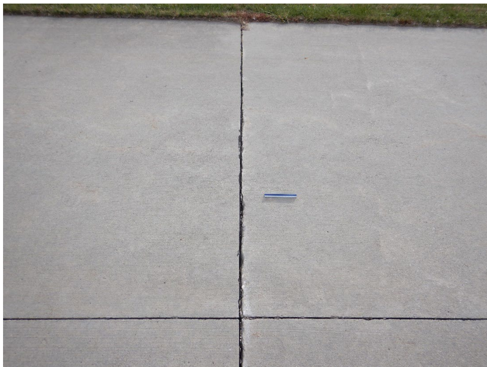
T01DN-04. Joint Seal Damage (Sample Unit No. 01).
