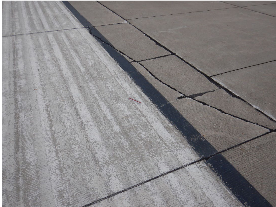
R12DN-02. Shattered Slab (Sample Unit No. 16).
