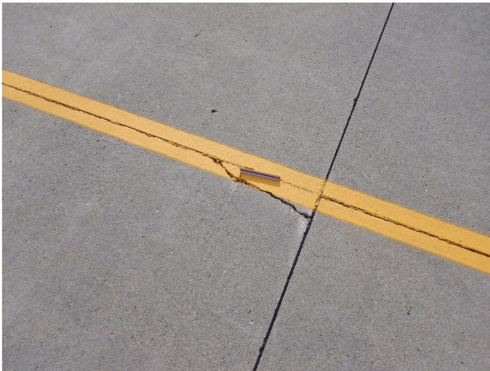
TH01DN-01. Joint Spalling (Sample Unit No. 03).
