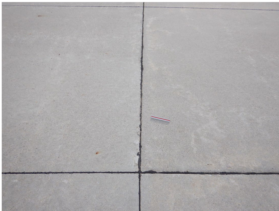
T01DN-01. Joint Seal Damage (Sample Unit No. 01).
