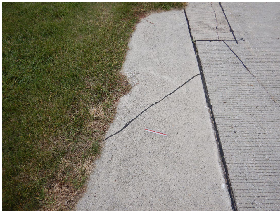
T01DN-06. LTD Cracking (Sample Unit No. 01).
