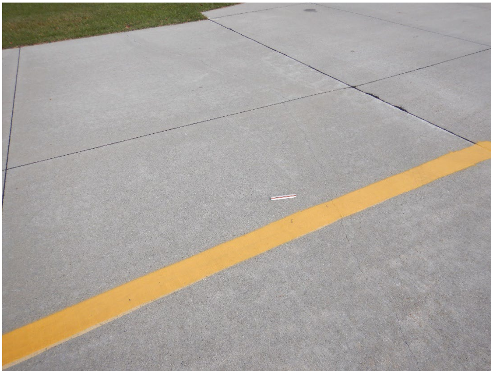
A01DN-01. LTD Cracking (Sample Unit No. 01).
