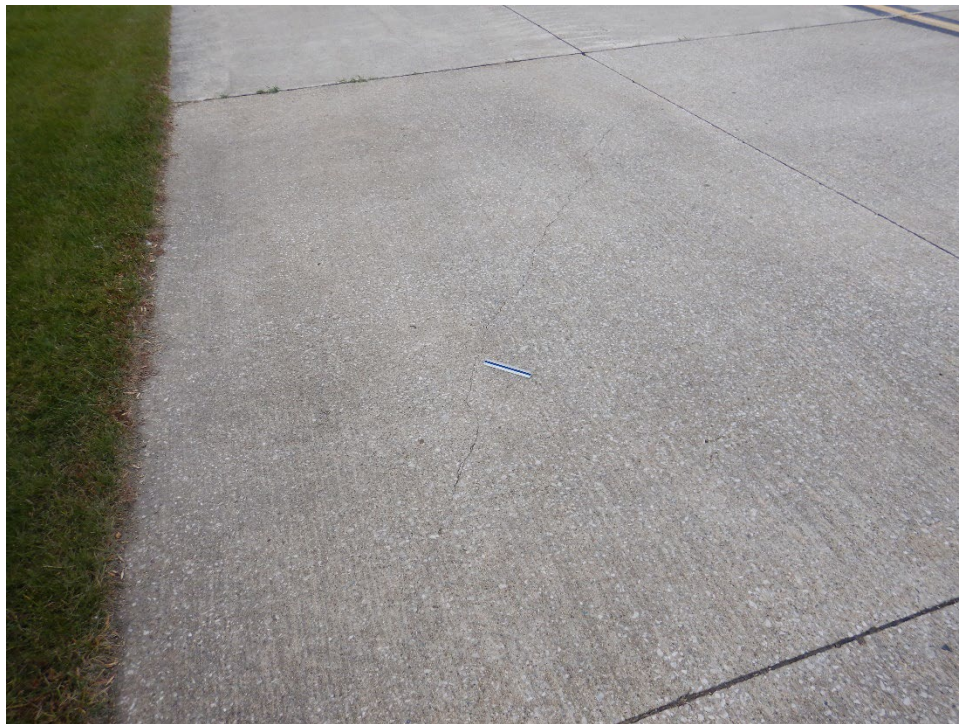
T01DN-05. LTD Cracking (Sample Unit No. 01).
