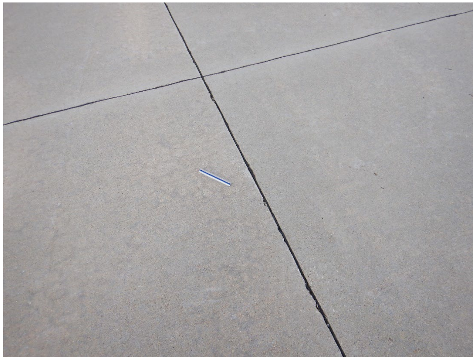
T01DN-02. Joint Seal Damage (Sample Unit No. 01).
