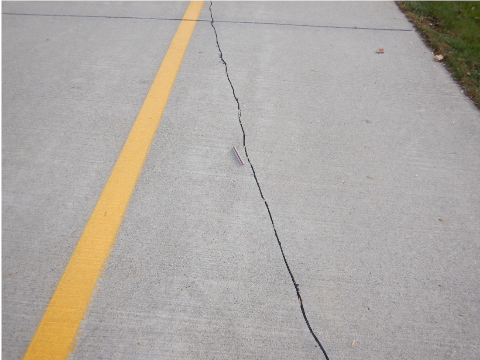
TH01DN-02. LTD Cracking (Sample Unit No. 01).
