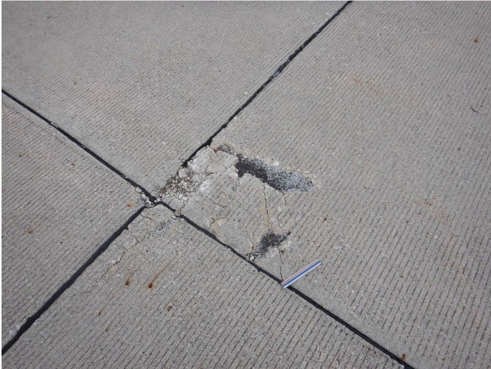
R12DN-01. Corner Spalling (Additional Sample Unit No. 36).
