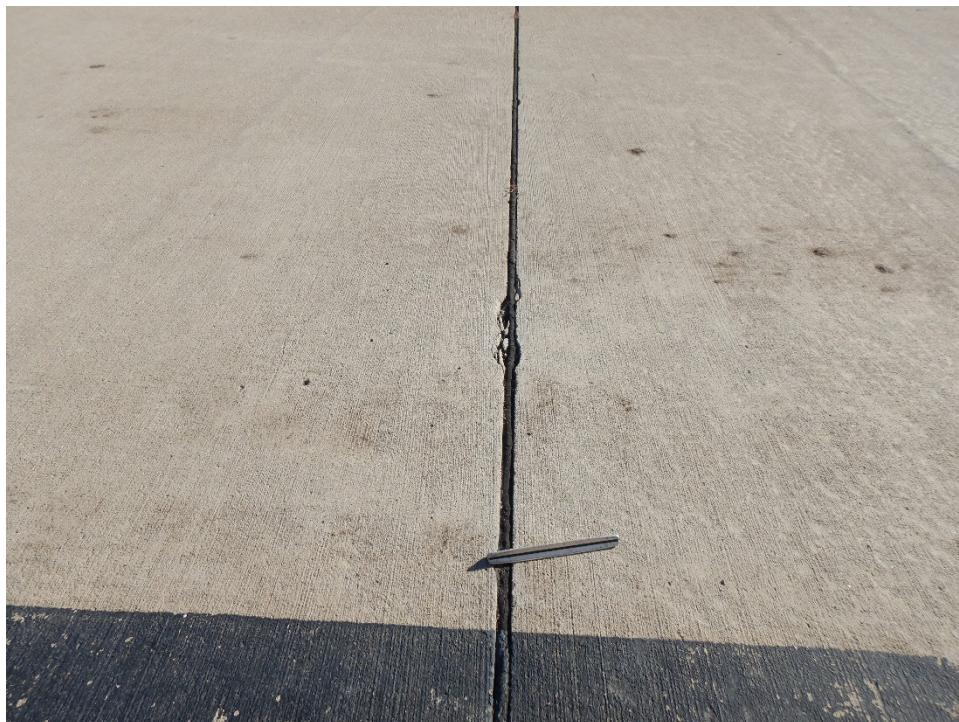
TH01FA-01. Joint Seal Damage (Sample Unit No. 05).
