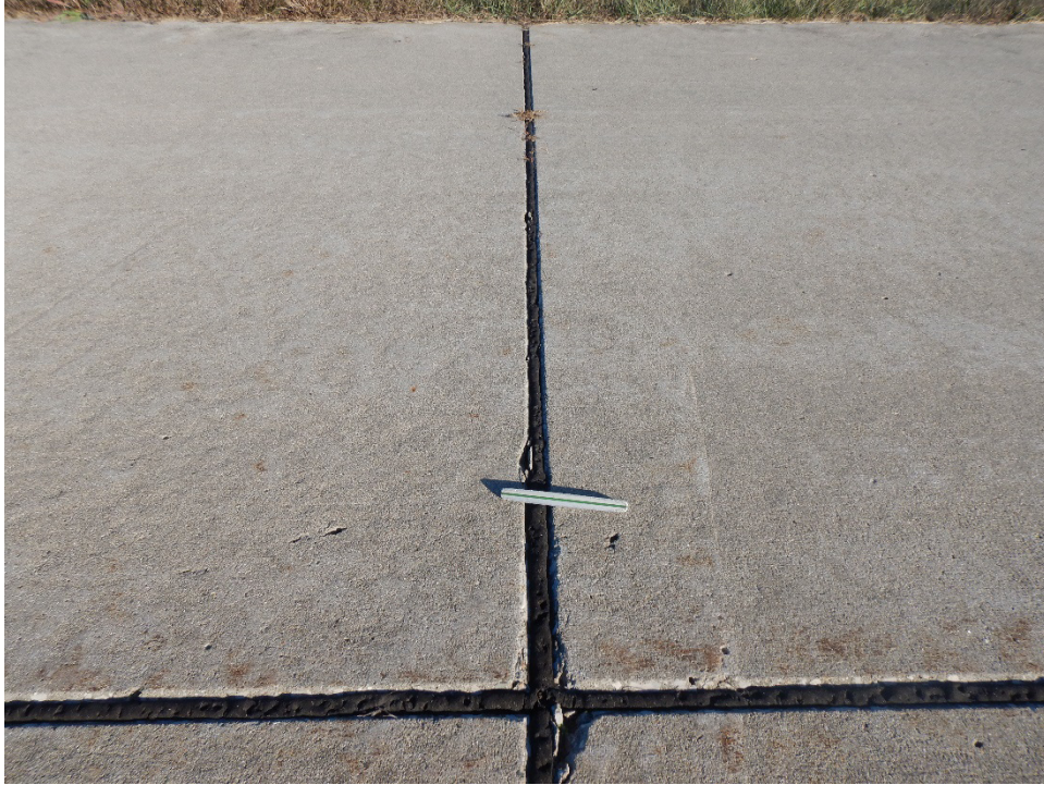
T04FA-01. Joint Seal Damage (Sample Unit No. 04).
