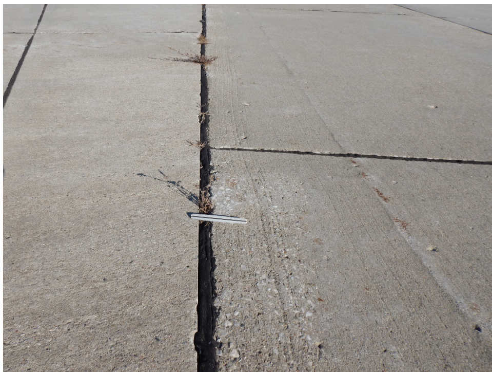
T02FA-01. Joint Seal Damage (Sample Unit No. 05).
