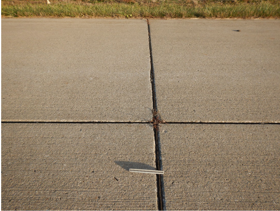
TA1FA-02. Joint Seal Damage (Sample Unit No. 03).
