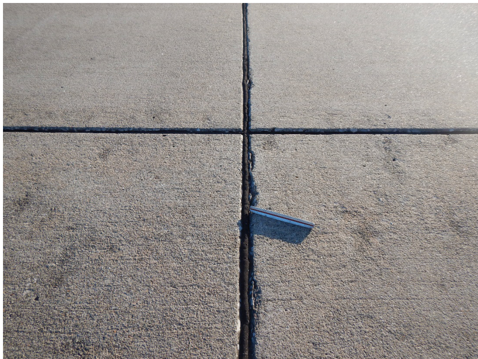
TAF A-01. Joint Seal Damage (Sample Unit No. 57).
