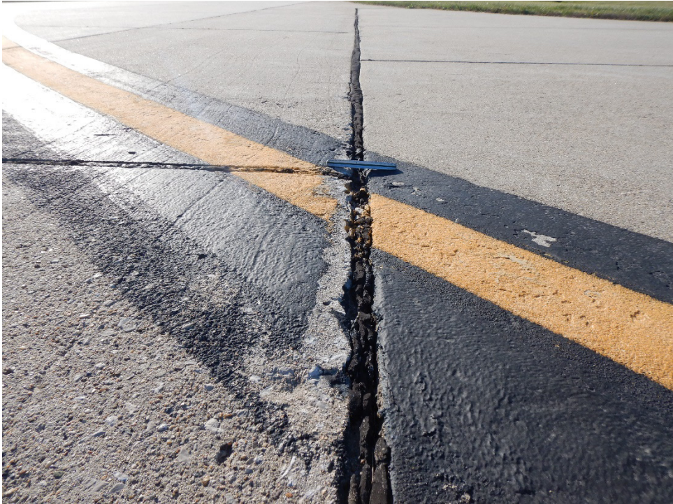
T03FA-01. Faulting (Sample Unit No. 05).
