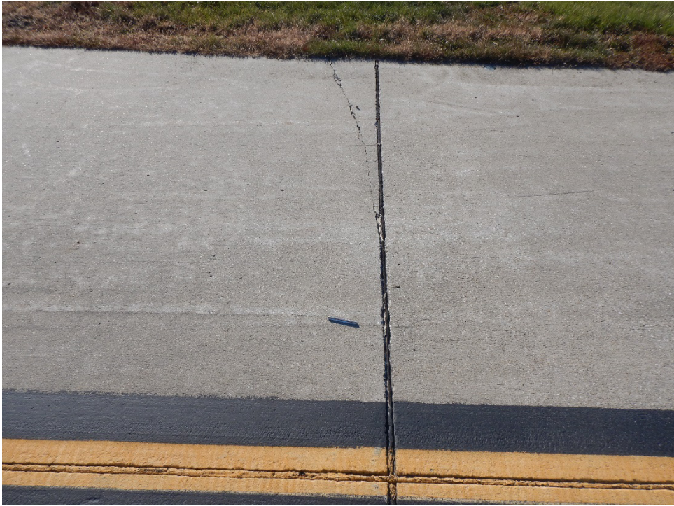
TH01FA-03. LTD Cracking (Sample Unit No. 01).
