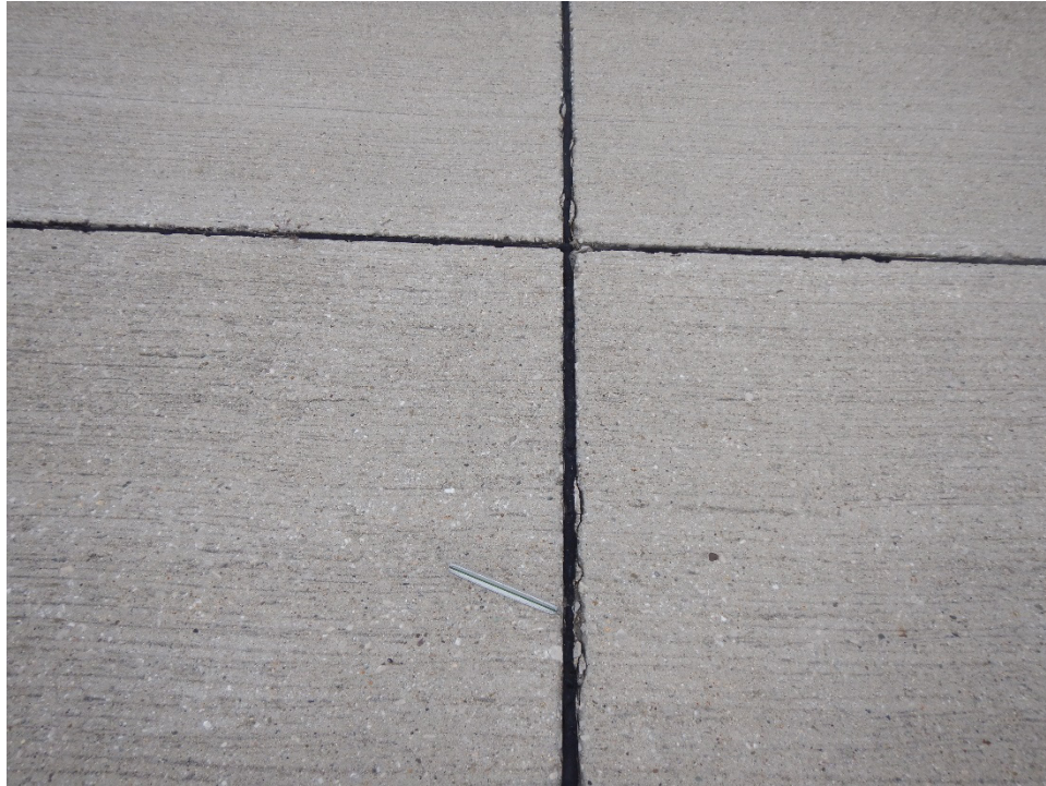
TA3FA-02. Joint Seal Damage (Sample Unit No. 03).
