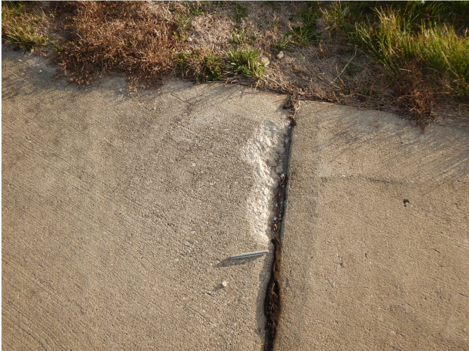
TA1FA-01. Joint Spalling (Sample Unit No. 01).
