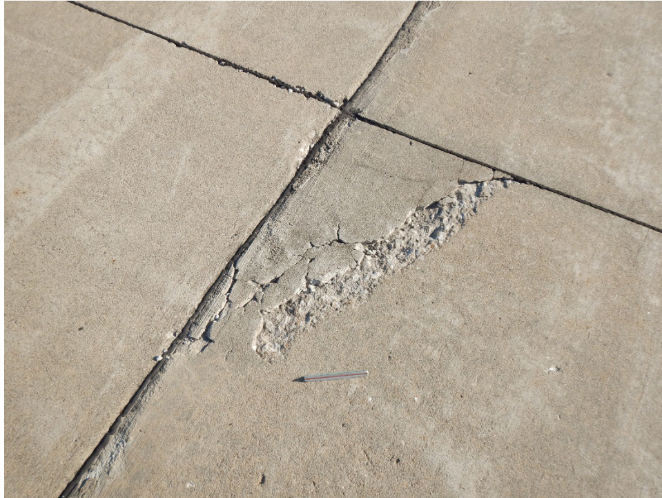
T07FA-01. Corner Spalling (Sample Unit No. 04).
