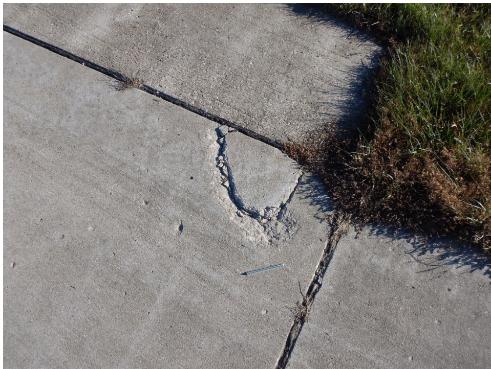
T07FA-02. Joint Spalling (Sample Unit No. 05).
