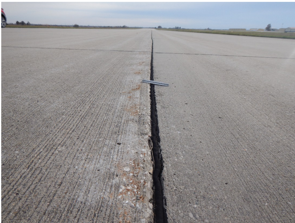
R18FA-01. Faulting (Sample Unit No. 113).
