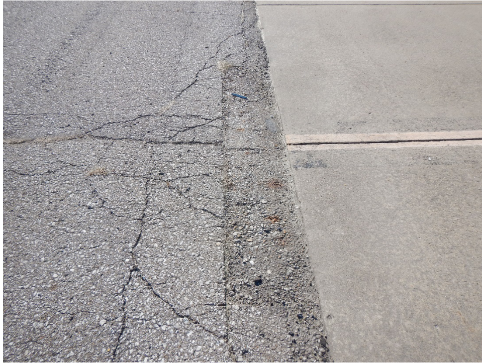
TH01FA-02. Patching (Sample Unit No. 02).
