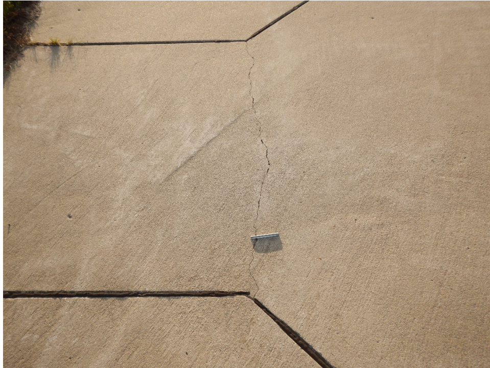
TA1FA-01. LTD Cracking (Sample Unit No. 01).
