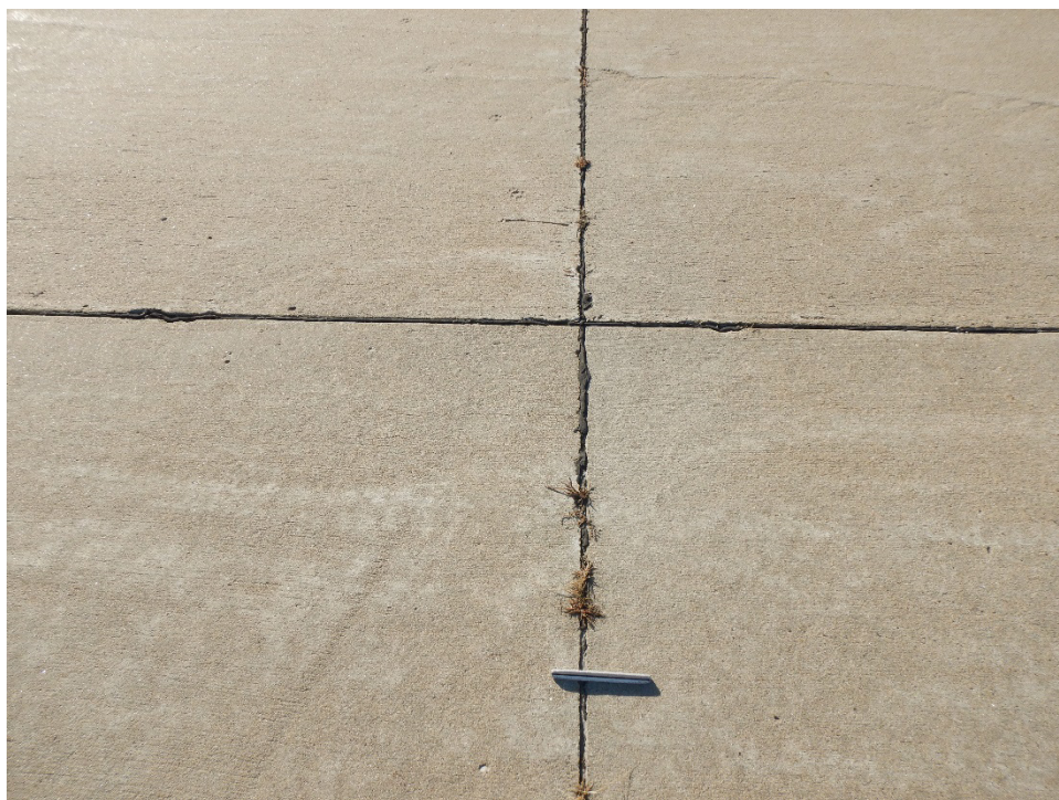
T07FA-01. Joint Seal Damage (Sample Unit No. 02).
