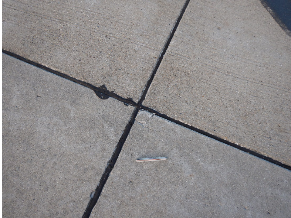
TAF A-01. Corner Spalling (Sample Unit No. 07).
