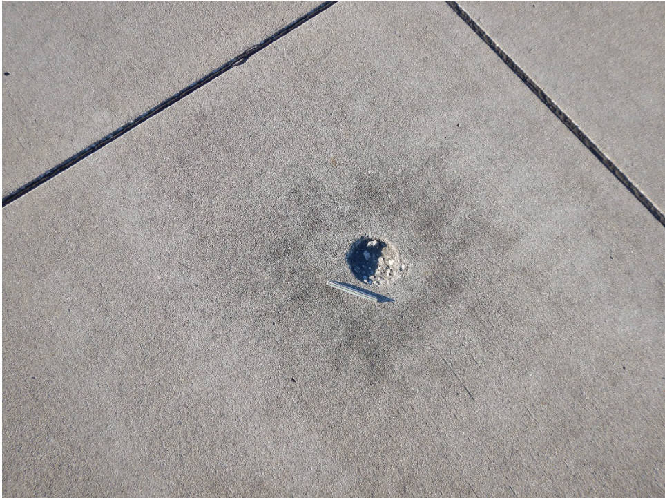
TAF A-02. Small Patching (Sample Unit No. 02).
