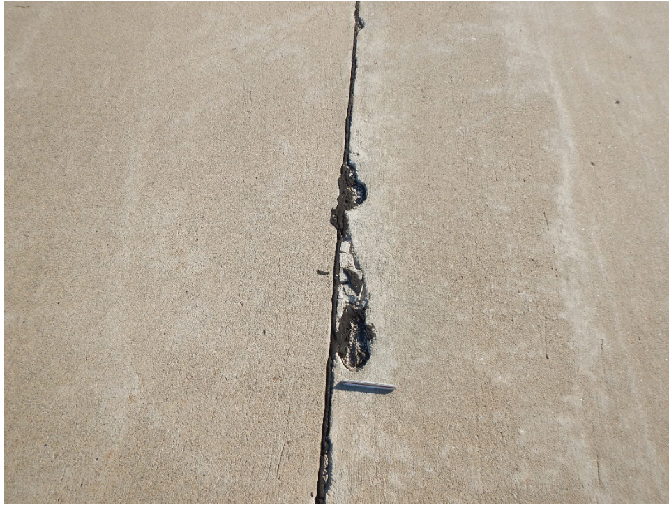
T07FA-01. Joint Spalling (Sample Unit No. 03).
