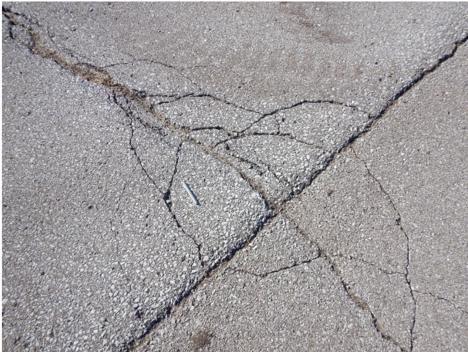
TH01FA-02. Alligator Cracking (Sample Unit No. 01).
