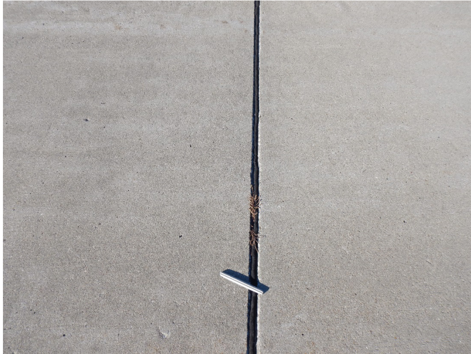
T07FA-02. Joint Seal Damage (Sample Unit No. 02).
