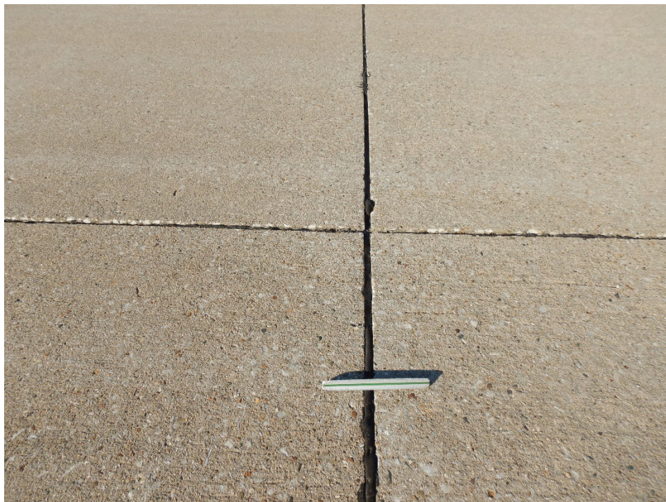
A01FA-02. Joint Seal Damage (Sample Unit No. 19).
