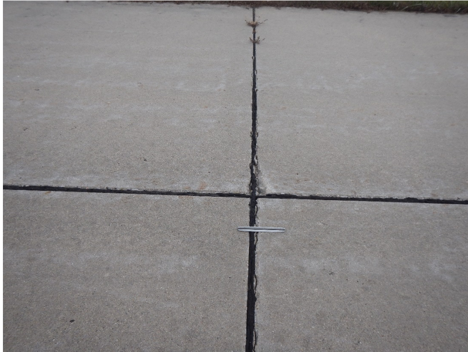
TA3FA-01. Joint Seal Damage (Sample Unit No. 03).
