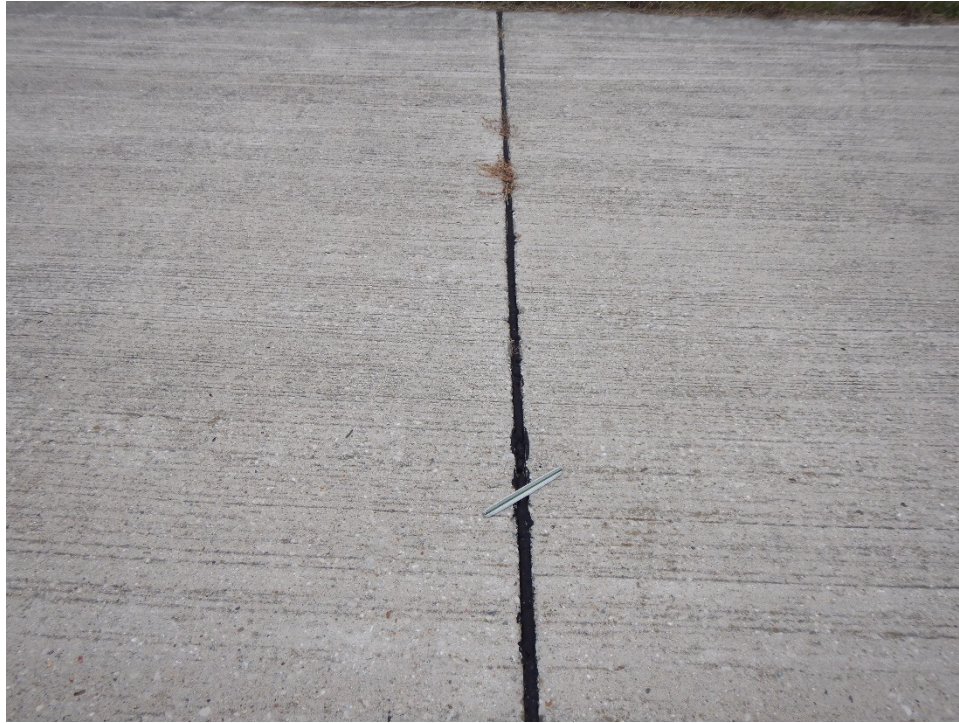
TA2FA-02. Joint Seal Damage (Sample Unit No. 02).
