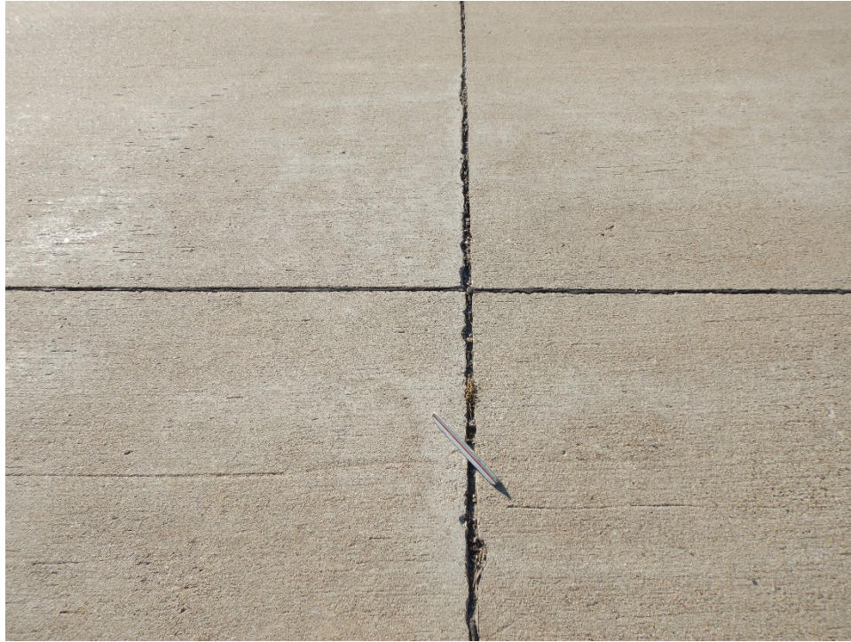
A01FA-01. Joint Seal Damage (Sample Unit No. 02).
