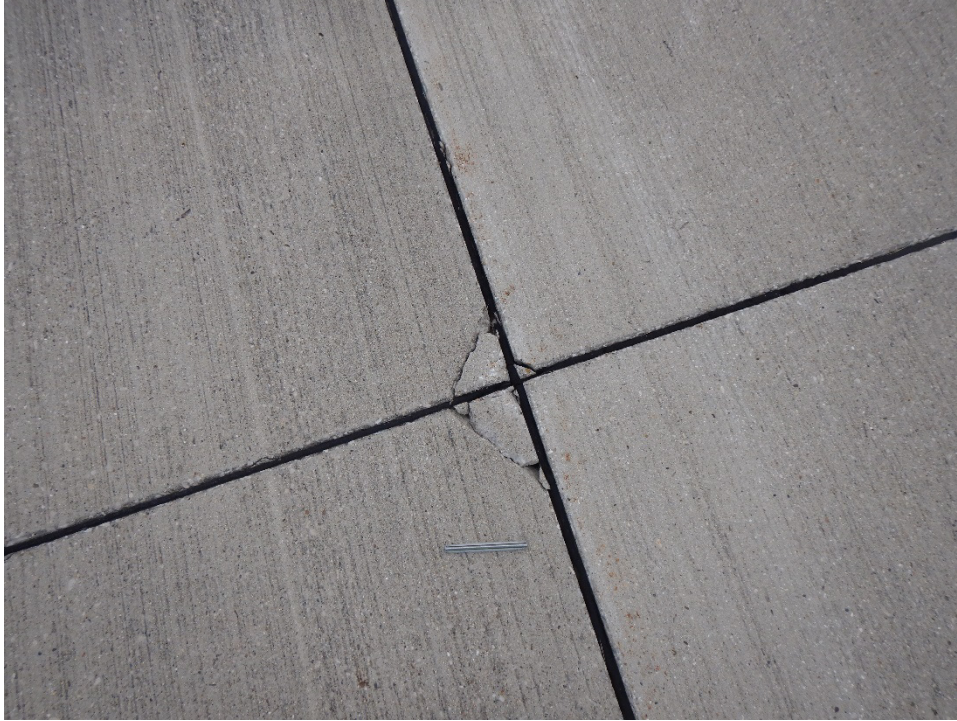
R18FA-01. Corner Spalling (Sample Unit No. 73).
