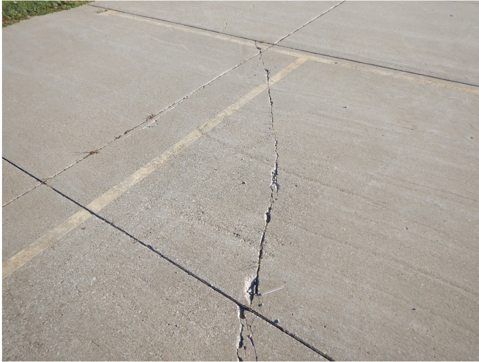
A01FA-02. LTD Cracking (Sample Unit No. 26).
