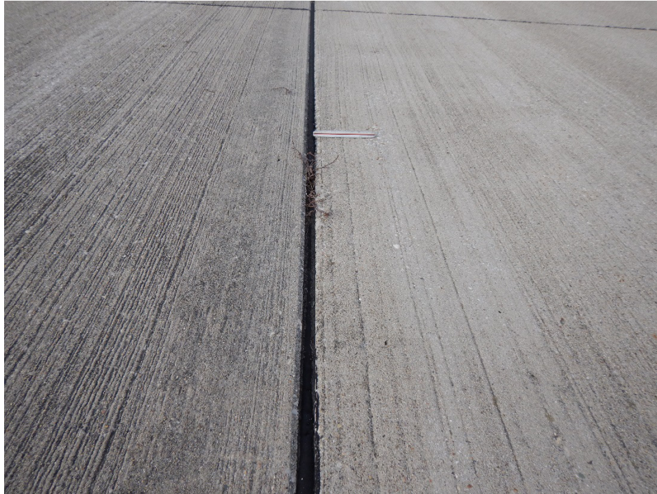
R18FA-01. Joint Seal Damage (Sample Unit No. 103).
