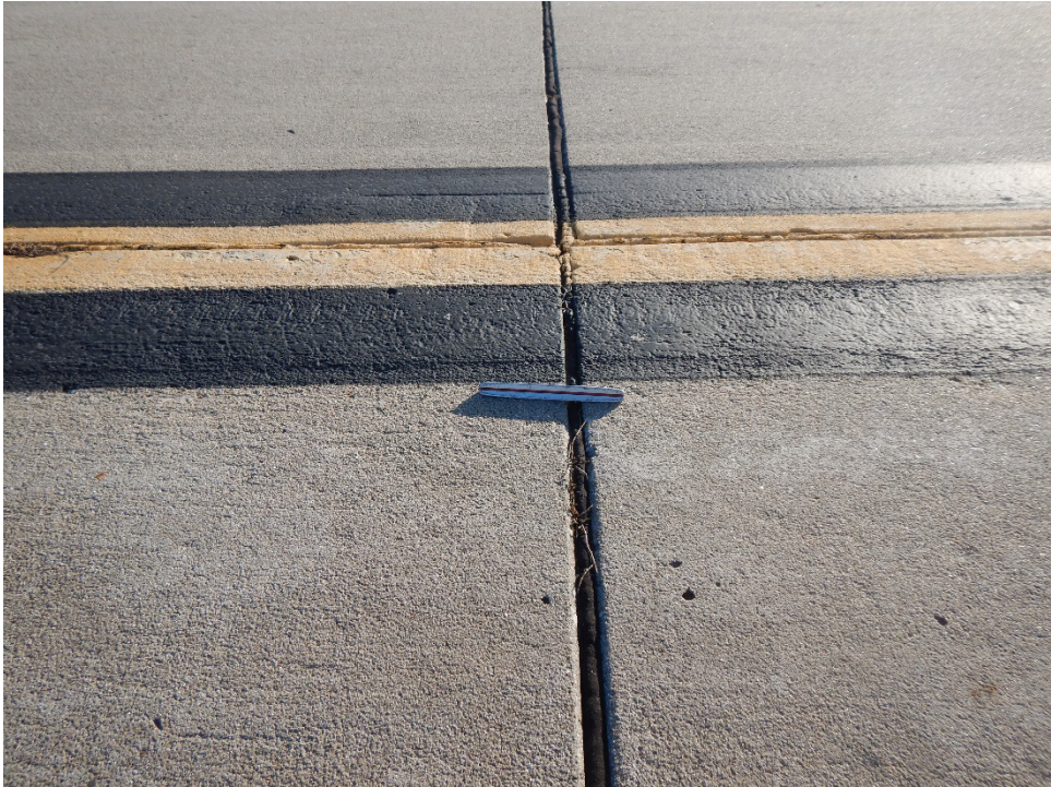
TAF A-02. Joint Seal Damage (Sample Unit No. 10).
