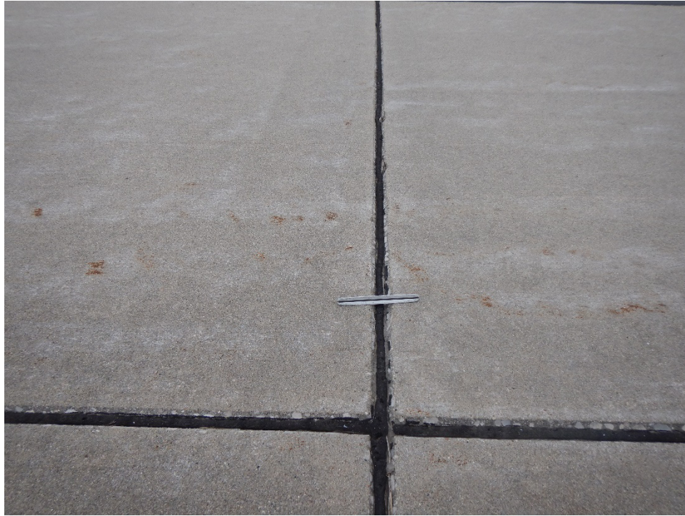
TA2FA-01. Joint Seal Damage (Sample Unit No. 04).
