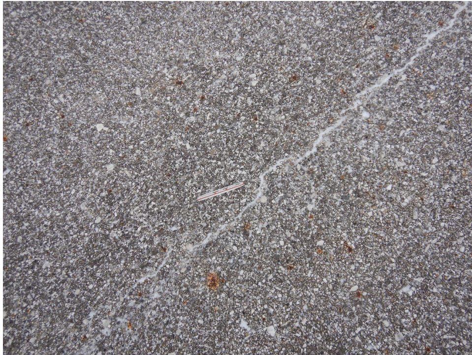
T02FC-01. L&T Cracking (Sample Unit No. 02).
