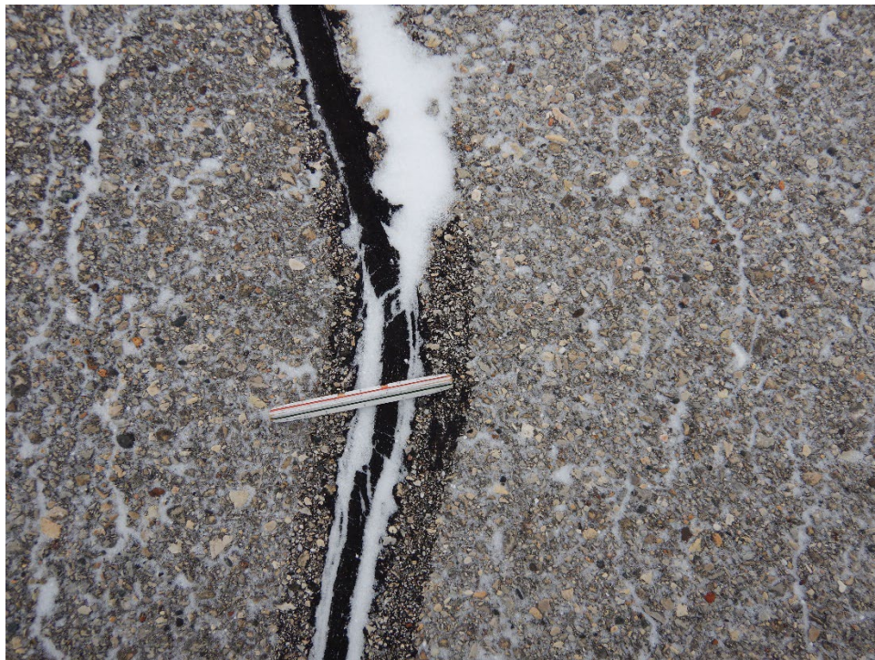
R09FC-04. L&T Cracking (Sample Unit No. 04).
