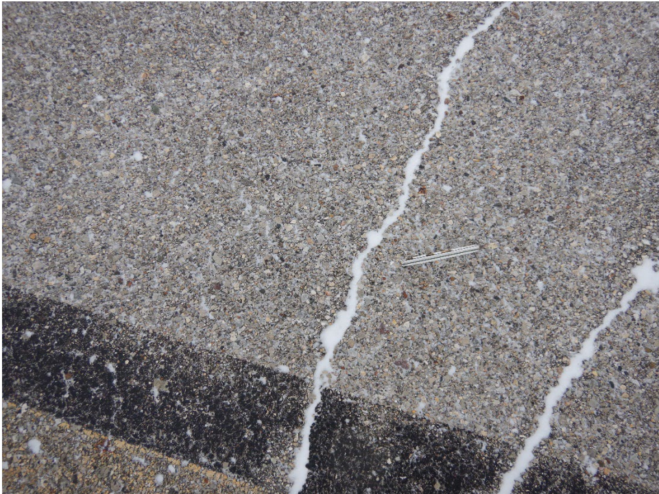
T02FC-03. L&T Cracking (Sample Unit No. 01).
