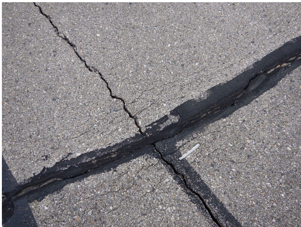
R09FC-02. L&T Cracking (Sample Unit No. 01) (1).
