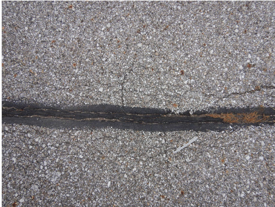
TH01FC-03. L&T Cracking (Sample Unit No. 03).
