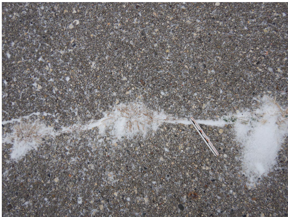
T01FC-02. L&T Cracking (Sample Unit No. 02).
