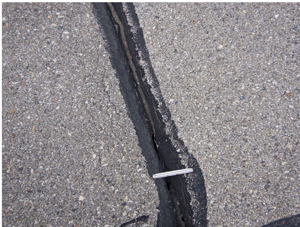
R09FC-01. L&T Cracking (Sample Unit No. 01).
