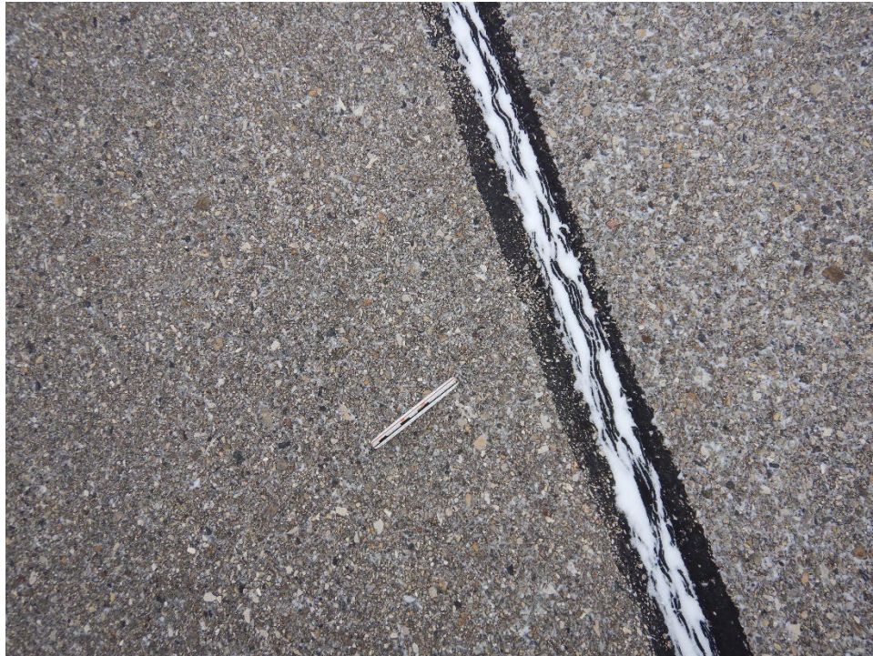
R09FC-03. L&T Cracking (Sample Unit No. 03) (1).
