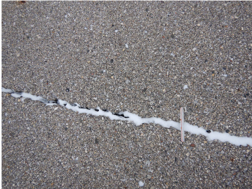
T02FC-02. L&T Cracking (Sample Unit No. 01).
