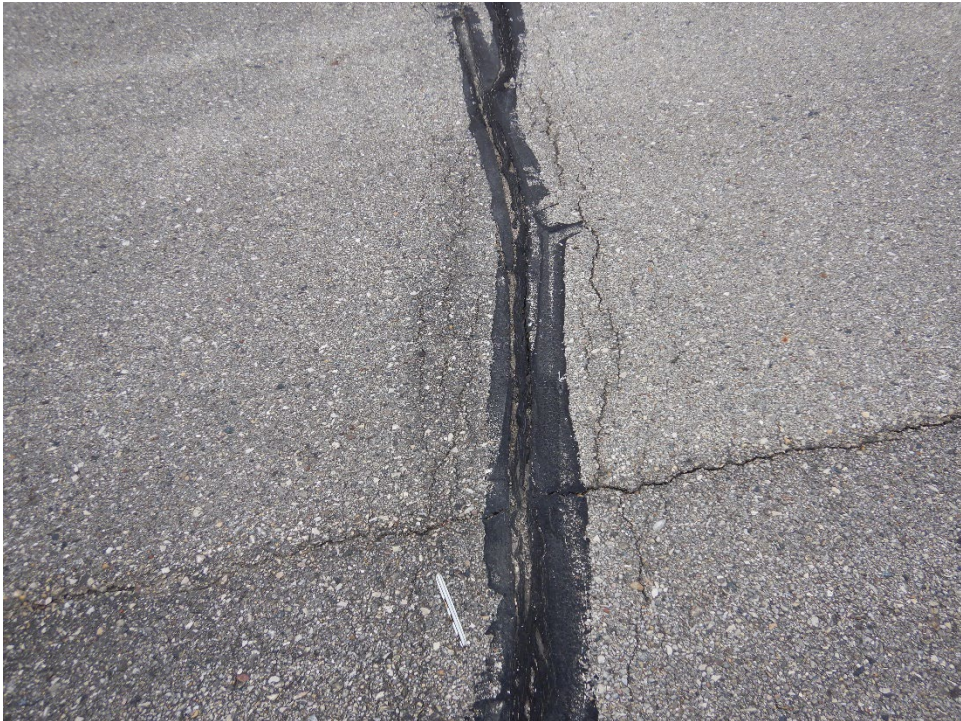
R09FC-02. L&T Cracking (Sample Unit No. 01) (2).
