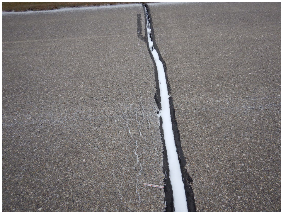
R09FC-03. L&T Cracking (Sample Unit No. 03) (2).
