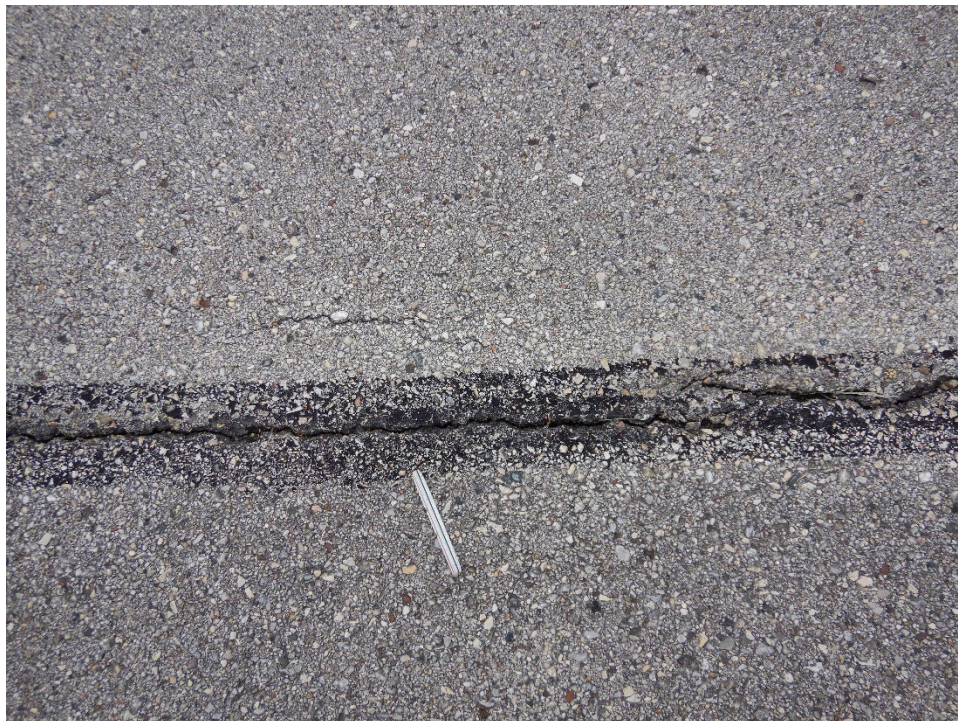
R15FC-01. L&T Cracking (Sample Unit No. 05).
