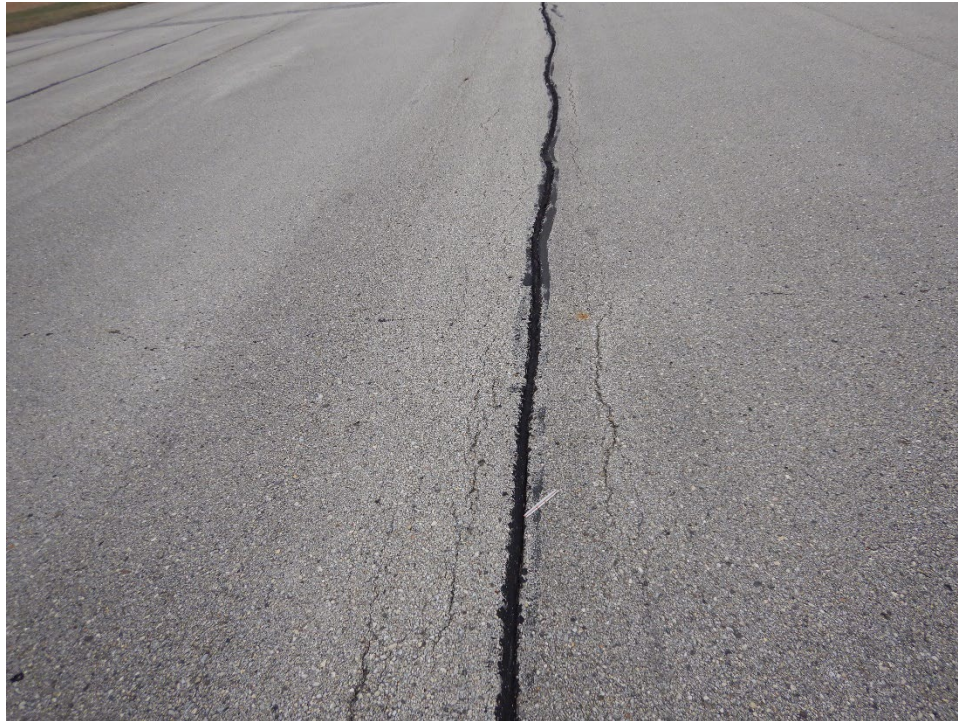
R15FC-01. Alligator Cracking (Sample Unit No. 41).
