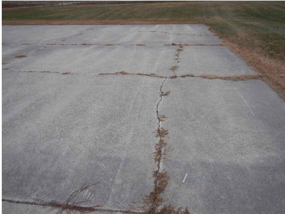
TH01FC-02. Shattered Slab (Sample Unit No. 01).
