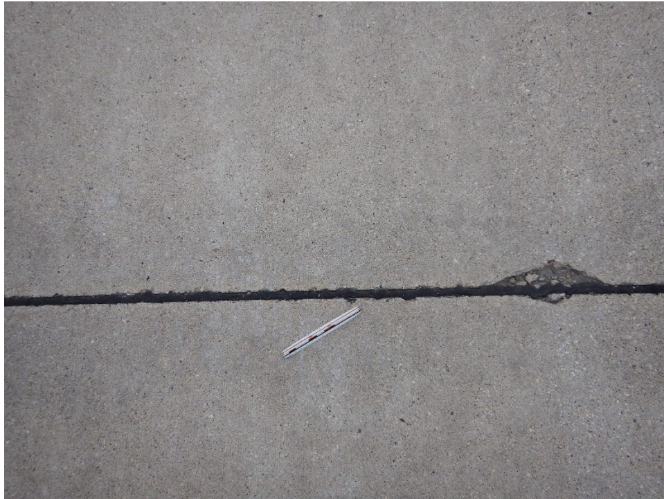
TH01FC-01. Joint Seal Damage (Sample Unit No. 03).
