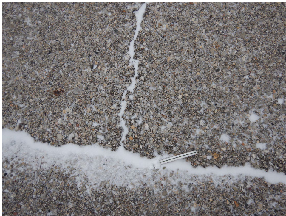
T01FC-01. L&T Cracking (Sample Unit No. 02).
