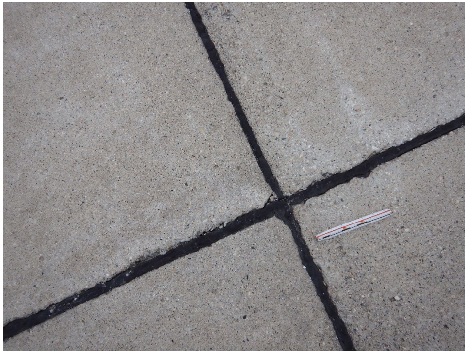
A01FC-01. Joint Seal Damage (Sample Unit No. 05).
