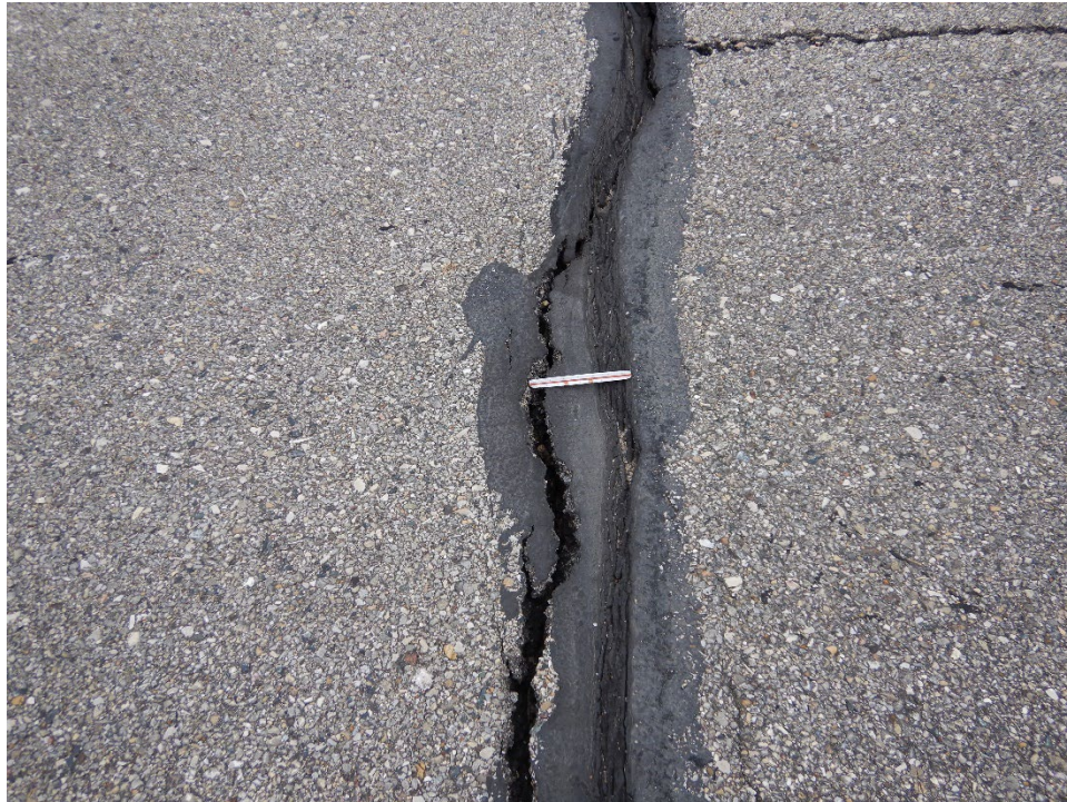
R09FC-01. L&T Cracking (Sample Unit No. 09).
