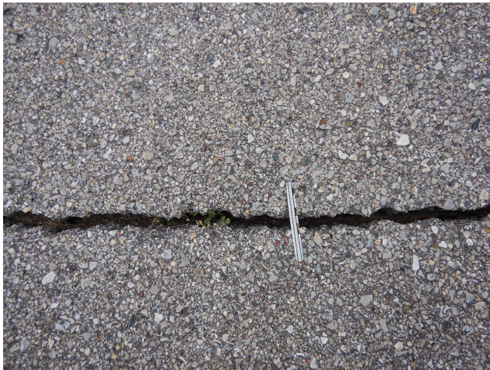
TH01FC-04. L&T Cracking (Sample Unit No. 01).
