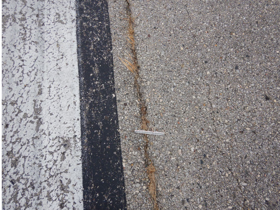
R15FC-02. L&T Cracking (Sample Unit No. 49).
