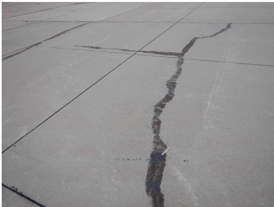
A01FC-02. LTD Cracking (Sample Unit No. 06).
