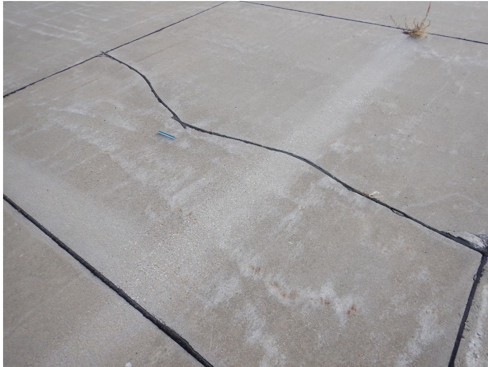
A01GL-04. LTD Cracking (Sample Unit No. 01).
