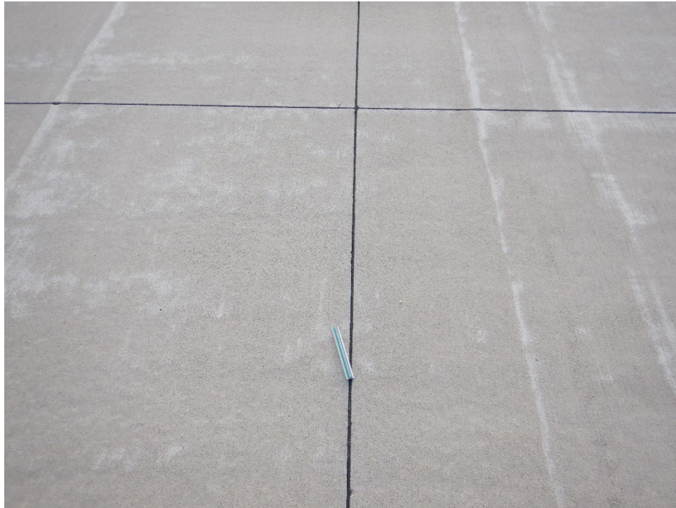
A01GL-06. Joint Seal Damage (Sample Unit No. 01).
