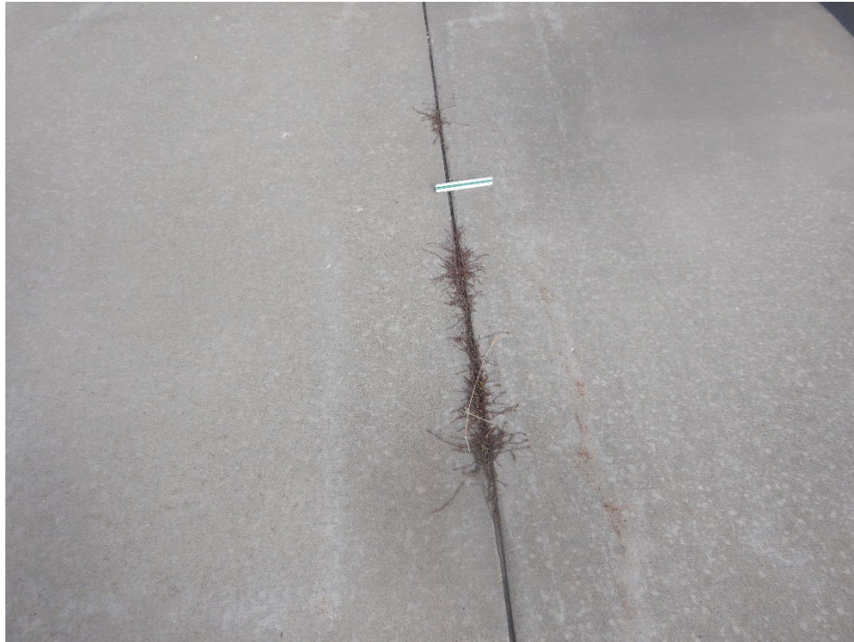
R13GL-05. Joint Seal Damage (Sample Unit No. 05).
