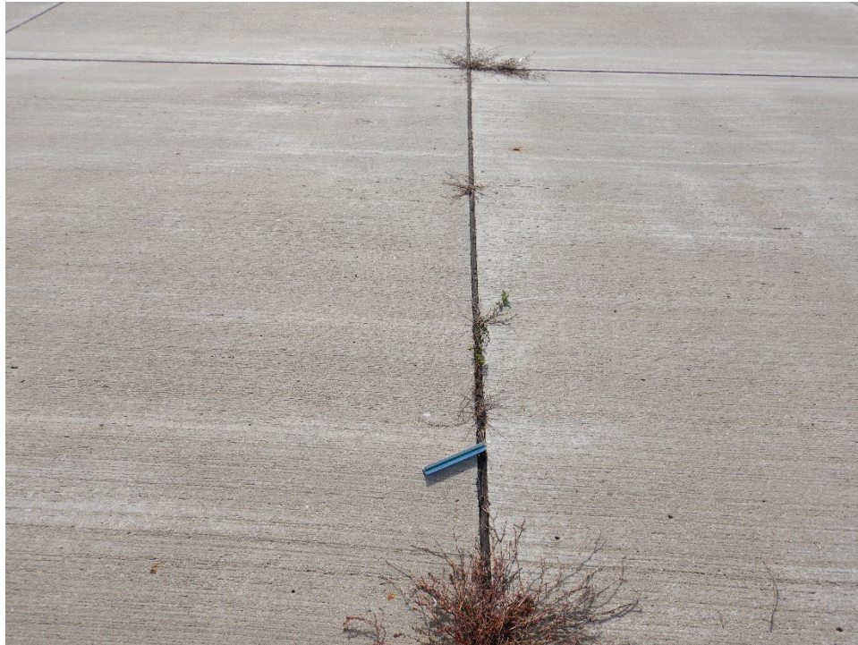
R13GL-03. Joint Seal Damage (Sample Unit No. 02).
