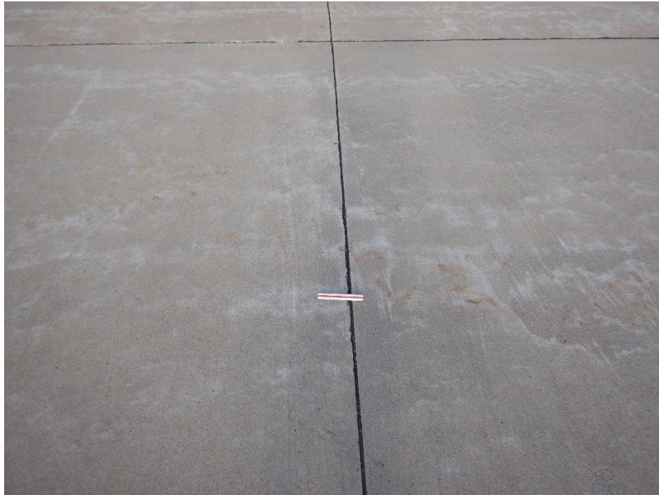
A01GL-05. Joint Seal Damage (Sample Unit No. 03).
