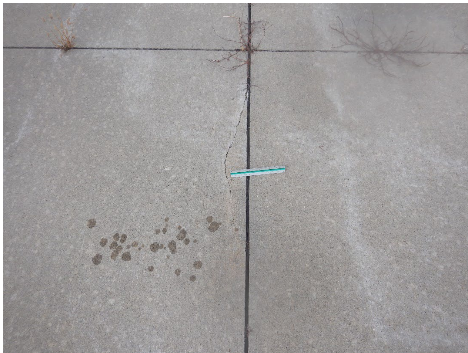
R13GL-05. Joint Spalling (Sample Unit No. 03).
