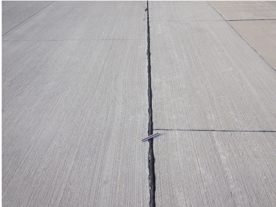
T01GL-01. Joint Seal Damage (Sample Unit No. 20).
