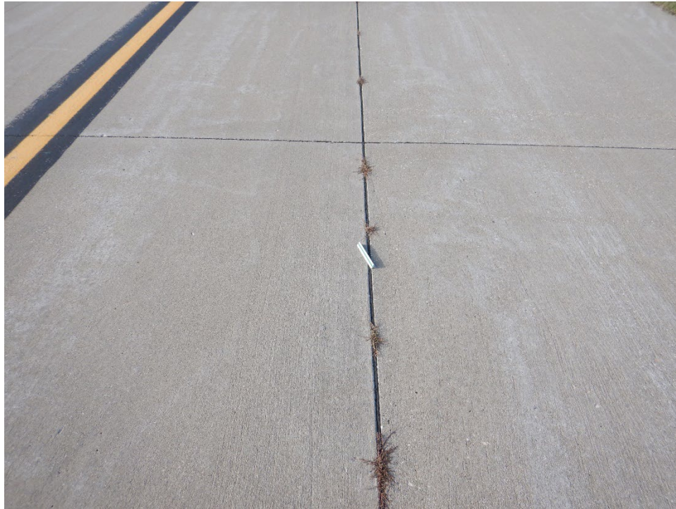
T02GL-01. Joint Seal Damage (Sample Unit No. 01).
