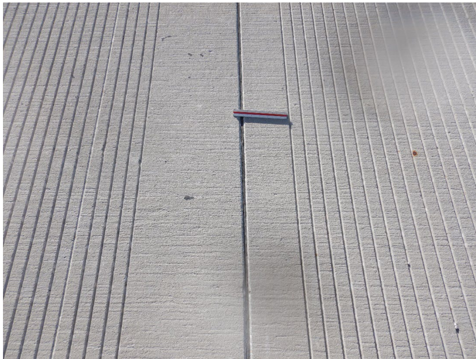
R13GL-01. Joint Seal Damage (Sample Unit No. 95).
