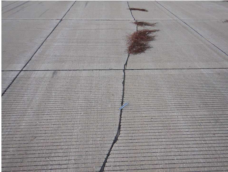
R13GL-02. LTD Cracking (Additional Sample Unit No. 16).
