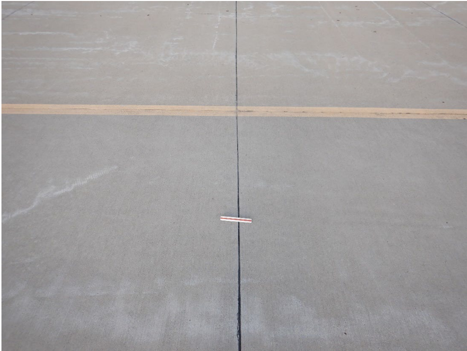
TH01GL-02. Joint Seal Damage (Sample Unit No. 01).
