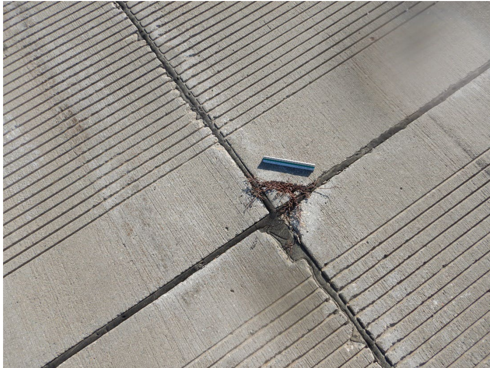
R13GL-02. Corner Spalling (Sample Unit No. 20).
