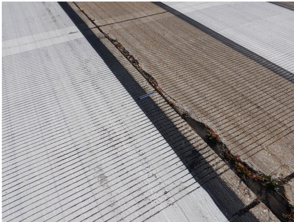
R13GL-02. Joint Spalling (Sample Unit No. 02).
