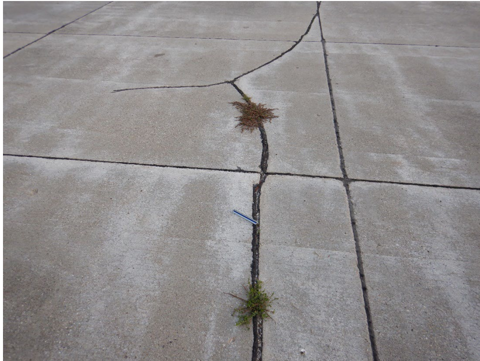
A01GL-03. LTD Cracking (Sample Unit No. 10).
