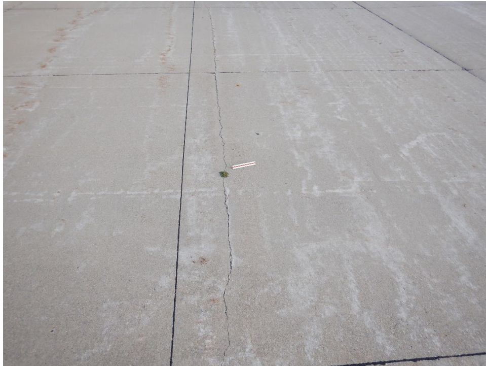
TH01GL-01. LTD Cracking (Sample Unit No. 05).
