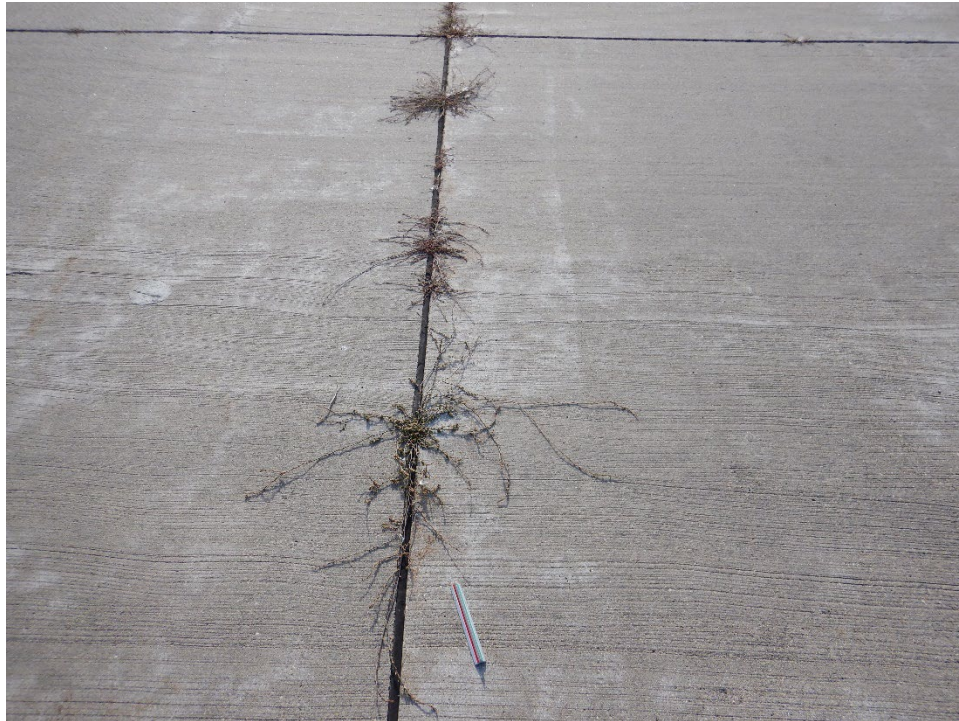
R13GL-04. Joint Seal Damage (Sample Unit No. 01).
