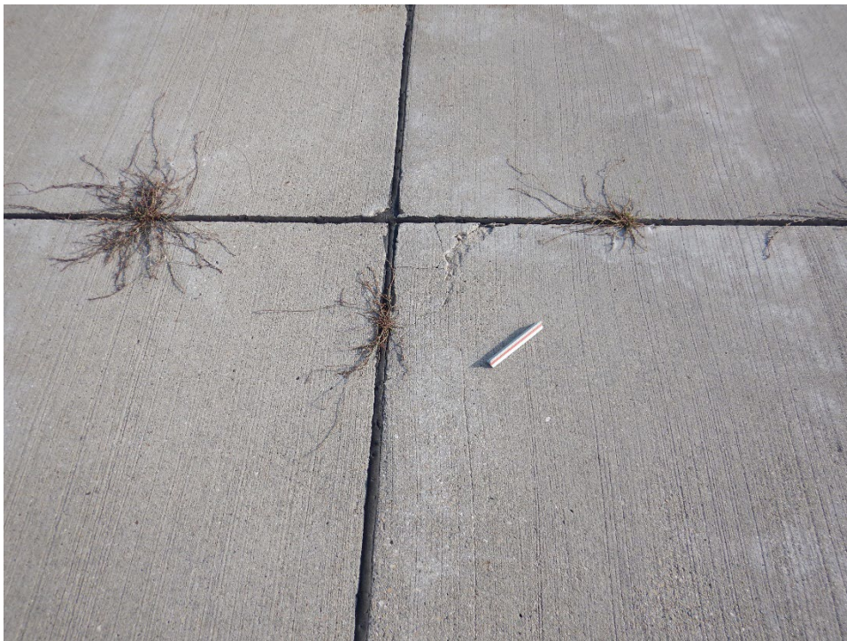
R13GL-04. Corner Spalling (Sample Unit No. 01).
