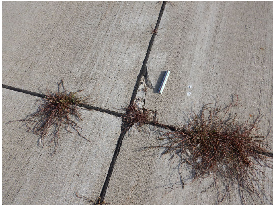
R13GL-03. Joint Spalling (Sample Unit No. 02).
