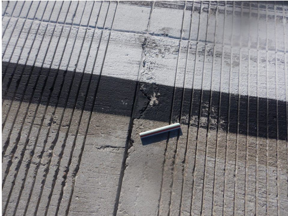
R13GL-01. Joint Spalling (Sample Unit No. 45).
