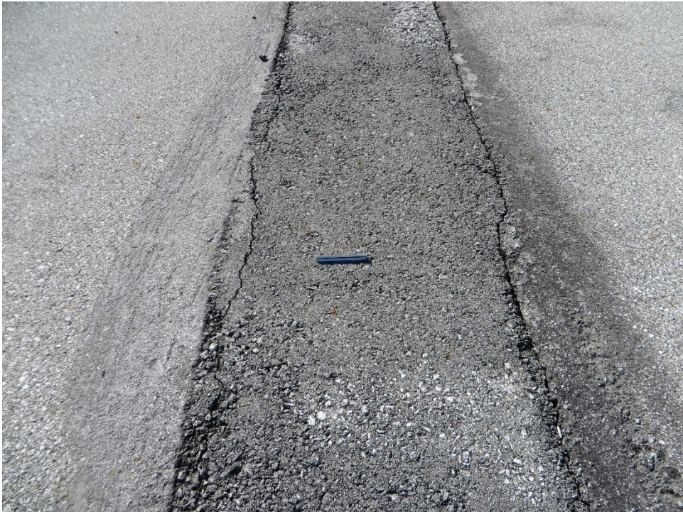
R12IG-03. Patching (Sample Unit No. 01).
