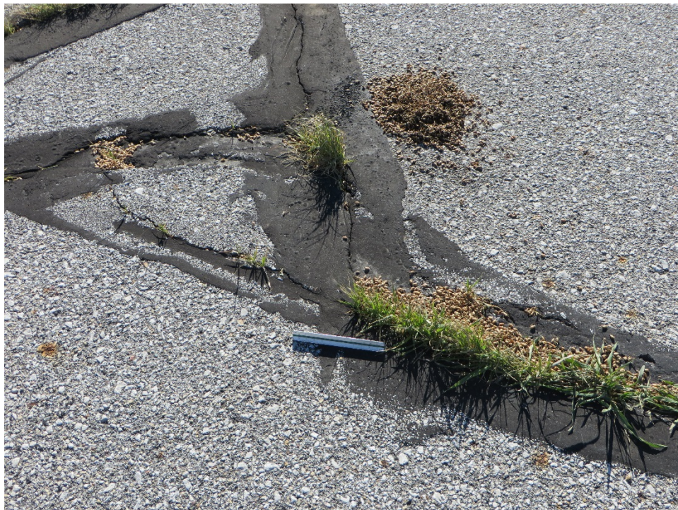
T01IG-01. L&T Cracking (Sample Unit No. 03).
