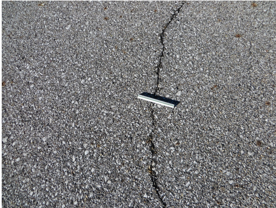
R12IG-02. L&T Cracking (Sample Unit No. 01).
