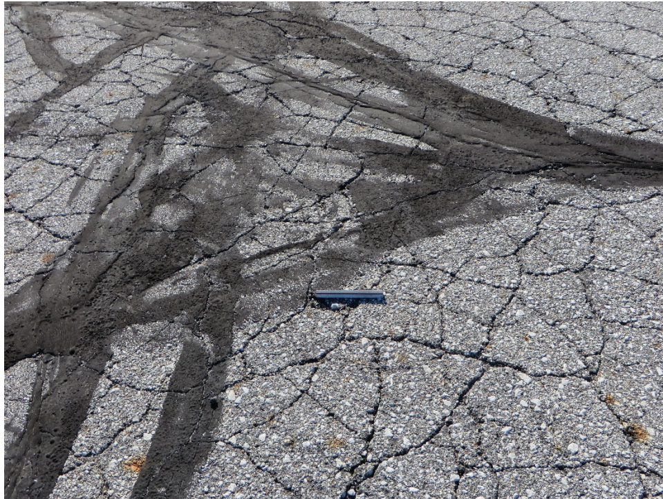
T01IG-01. Alligator Cracking (Sample Unit No. 03).
