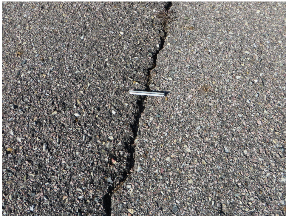
R12IG-01. L&T Cracking (Sample Unit No. 03).
