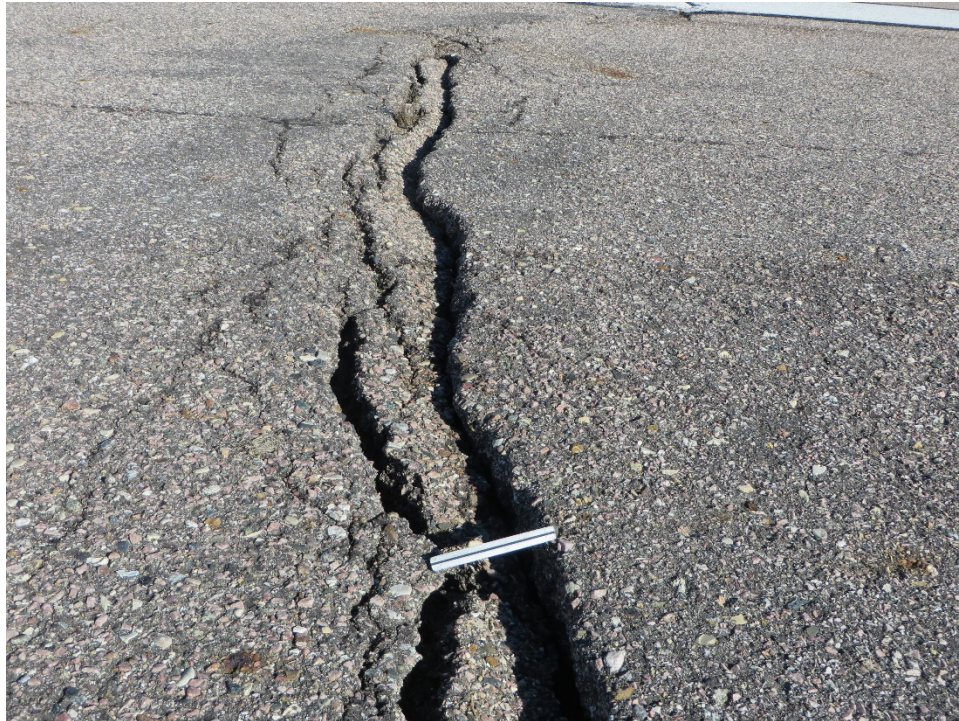
R12IG-01. L&T Cracking (Sample Unit No. 06).
