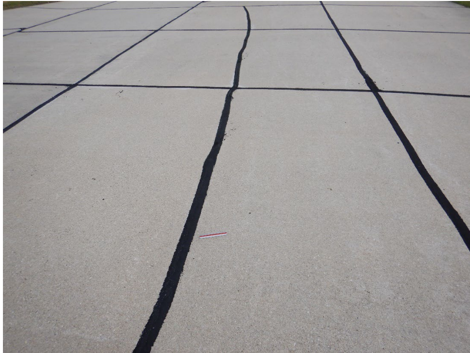
A02JE-01. LTD Cracking (Sample Unit No. 06).
