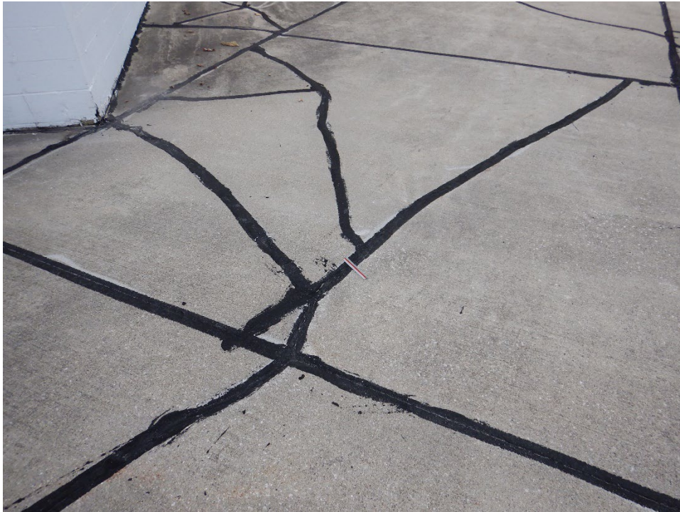
A01JE-03. Shattered Slab (Sample Unit No. 04).
