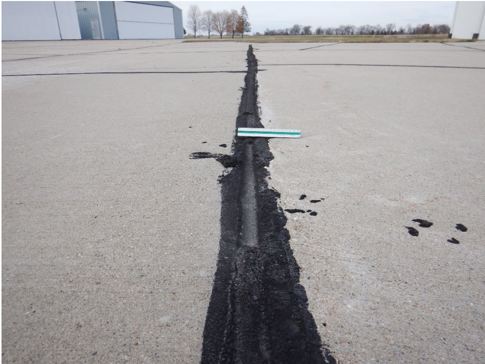
A02JE-02. Faulting (Sample Unit No. 02).
