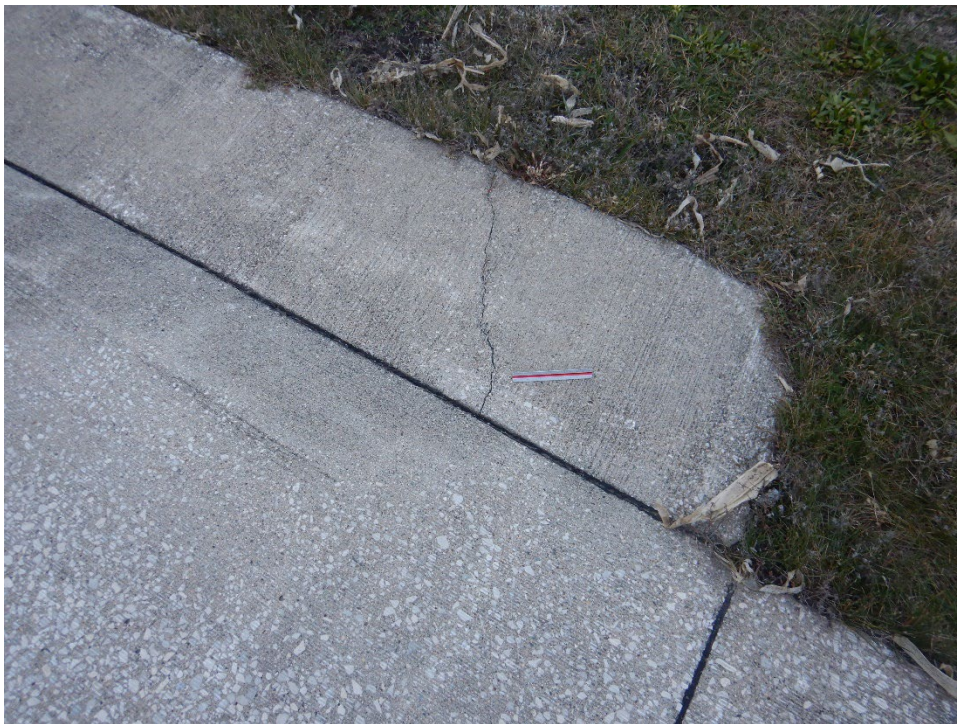
T01JE-01. LTD Cracking (Sample Unit No. 05).
