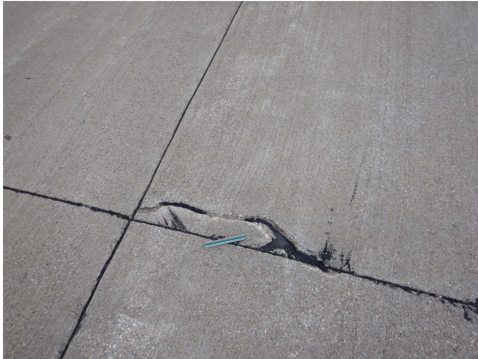
R14JE-03. Joint Spalling (Sample Unit No. 04).
