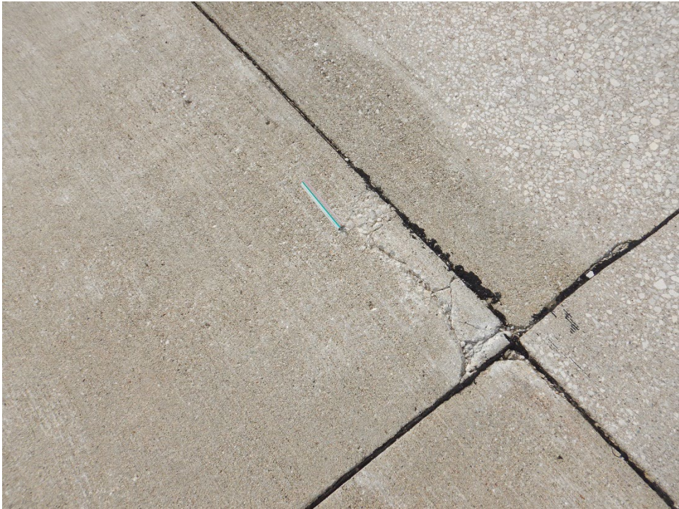
A01JE-01. Joint Spalling (Sample Unit No. 13).
