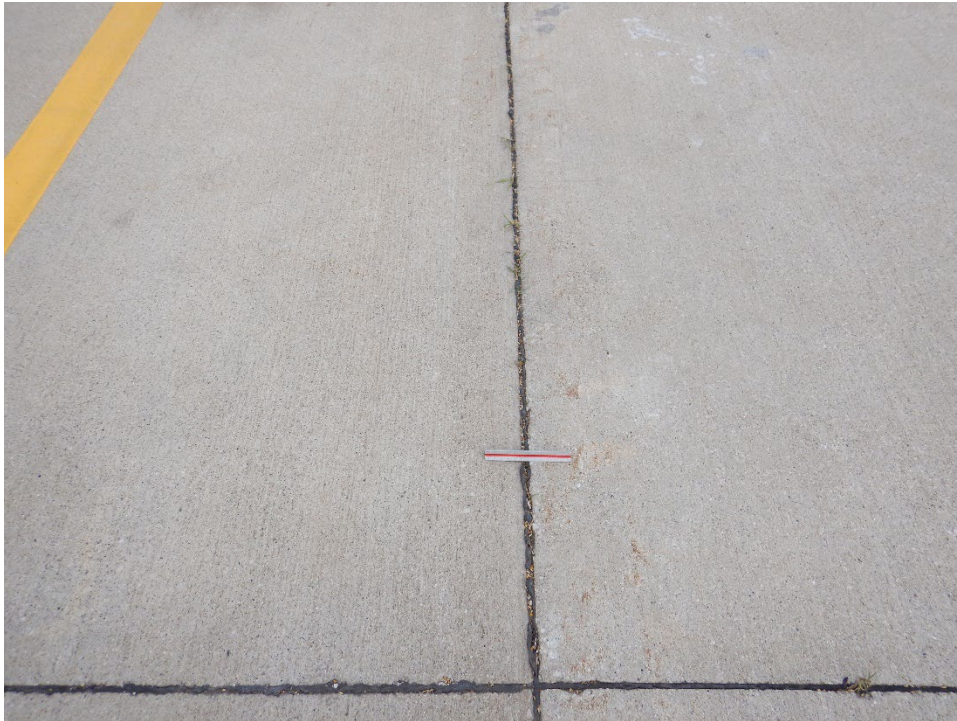
A01JE-02. Joint Seal Damage (Sample Unit No. 04).
