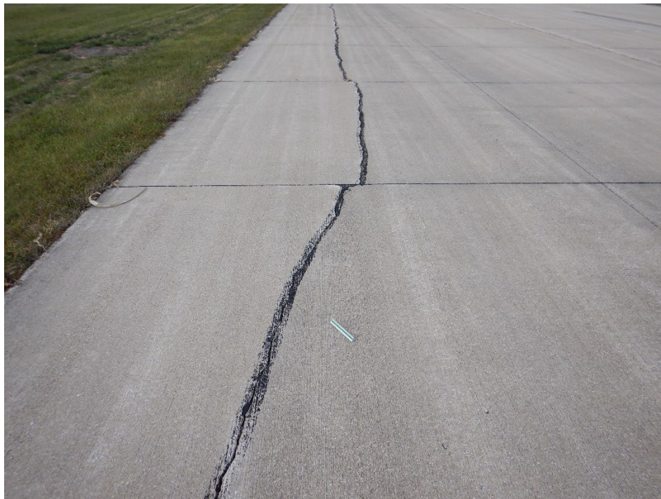
R14JE-01. LTD Cracking (Sample Unit No. 15).
