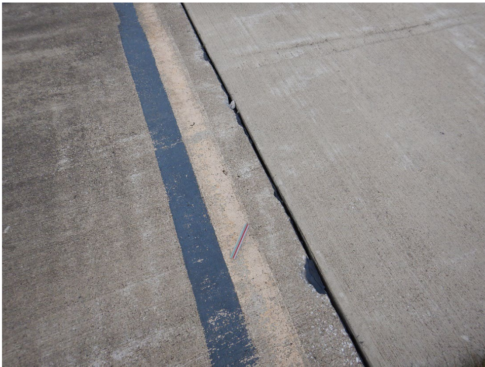
R14JE-02. Joint Spalling (Sample Unit No. 01).
