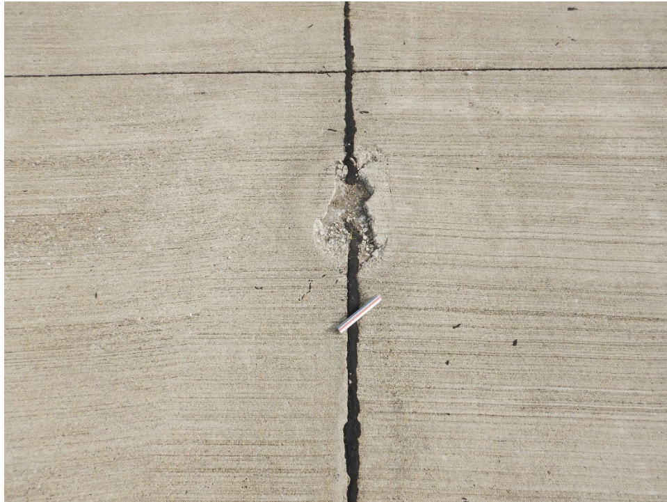
A01JE-01. Joint Spalling (Additional Sample Unit No. 12).
