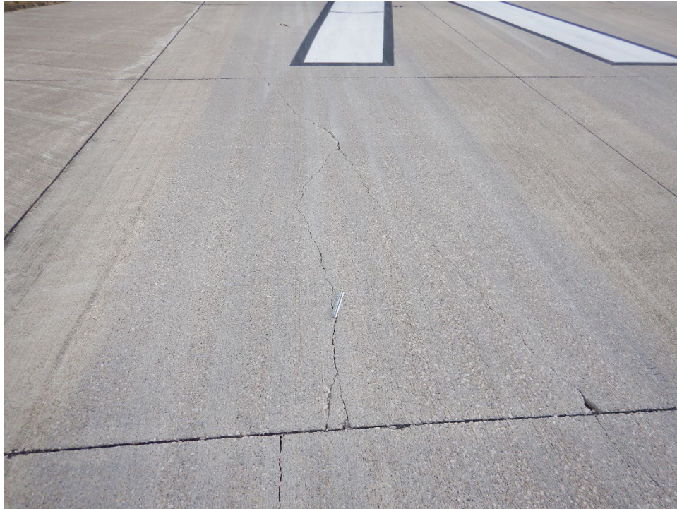
R14JE-02. Shattered Slab (Sample Unit No. 05).
