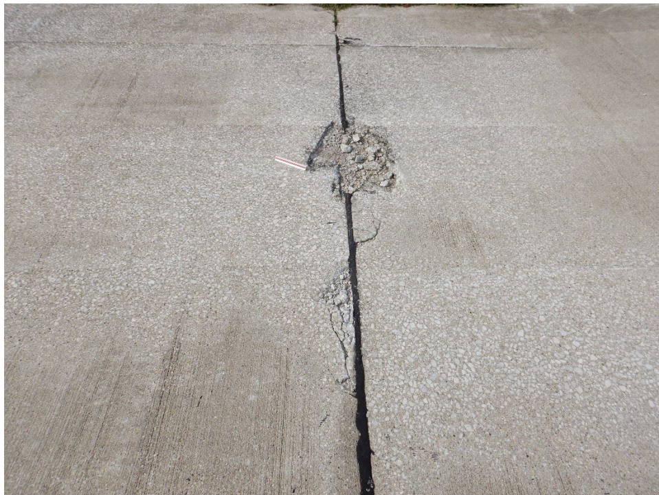
A01JE-01. Joint Spalling (Additional Sample Unit No. 18).
