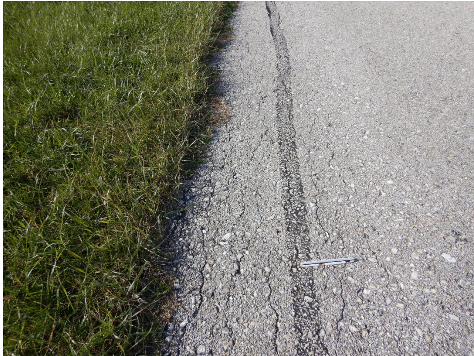
T04MT-01. Alligator Cracking (Sample Unit No. 03).
