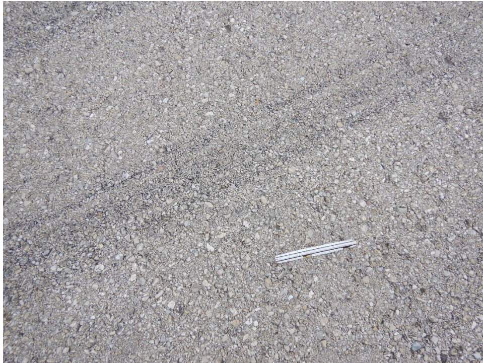
R13MT-01. Weathering (Sample Unit No. 16).
