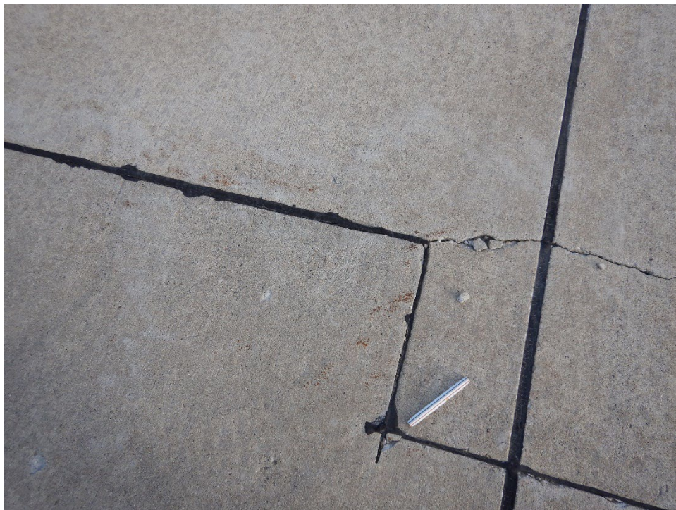
TH01MT-01. Small Patching (Sample Unit No. 11).
