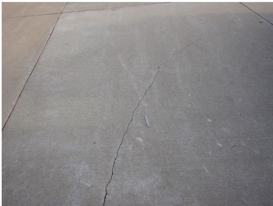
TH01MT-02. LTD Cracking (Sample Unit No. 05).
