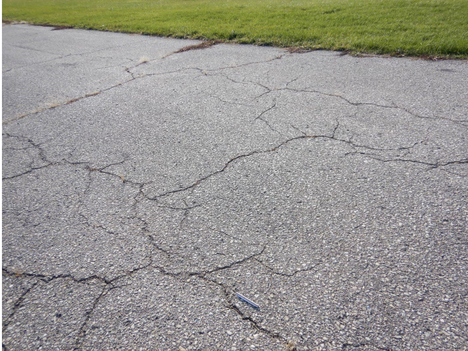
TH02MT-01. Block Cracking (Sample Unit No. 03).
