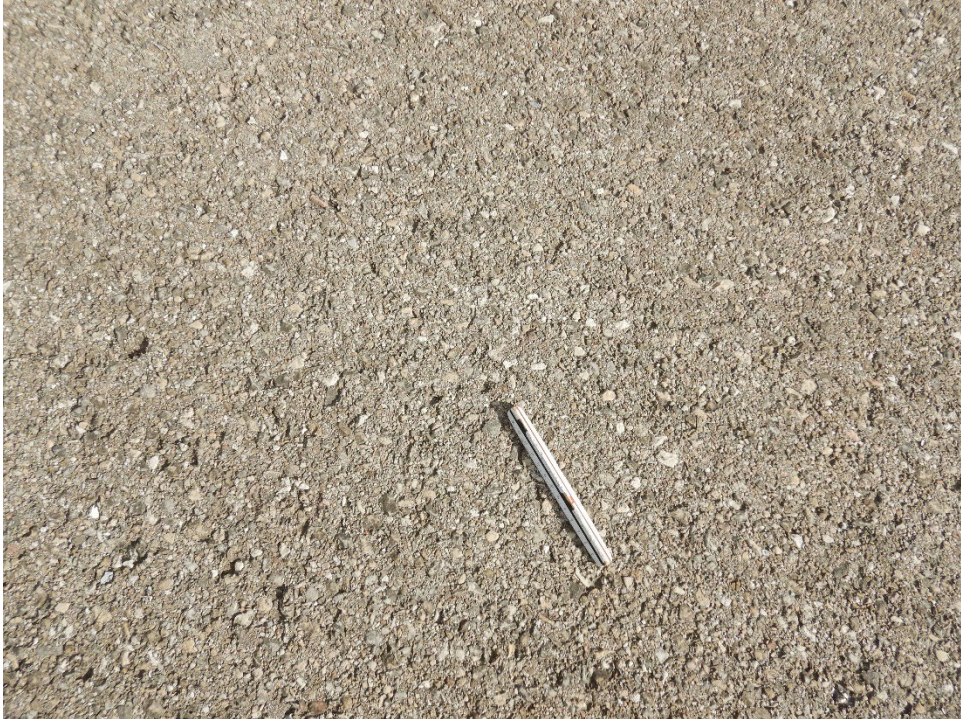
R18MT-04. Weathering (Sample Unit No. 01).
