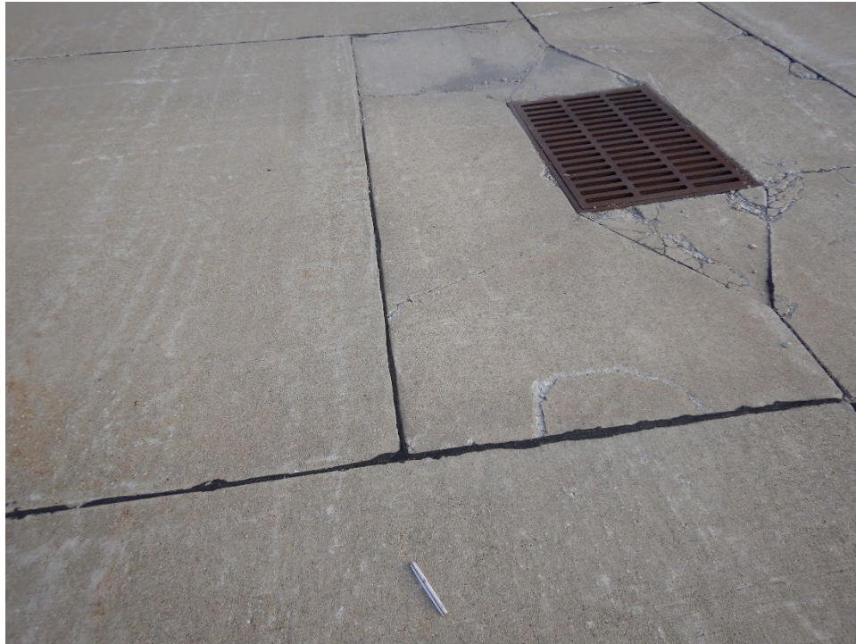
TH01MT-01. Large Patching (Additional Sample Unit No. 07).
