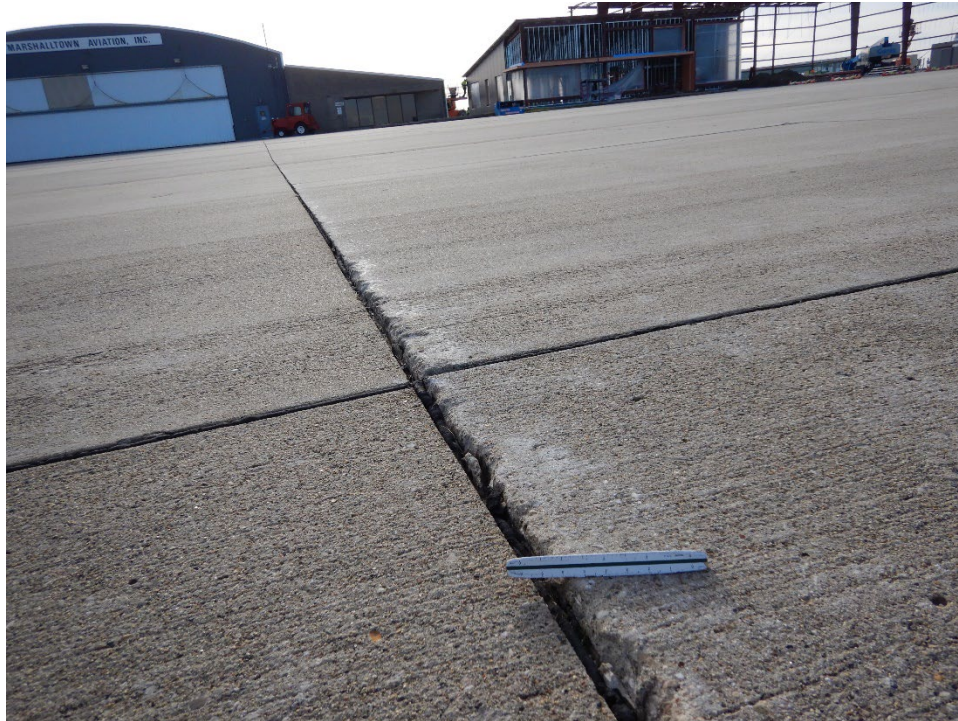
A01MT-01. Faulting (Sample Unit No. 06).
