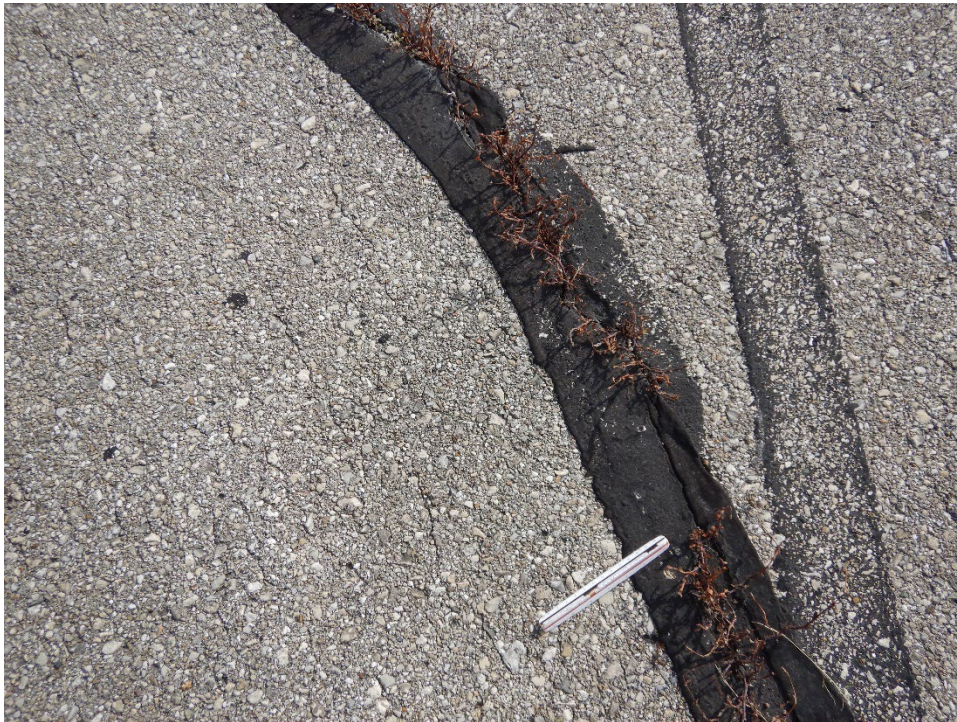
R18MT-01. L&T Cracking (Sample Unit No. 02) (2).
