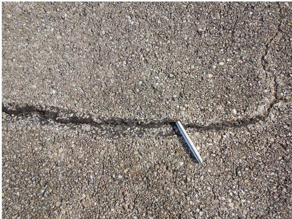
R13MT-04. L&T Cracking (Sample Unit No. 01).
