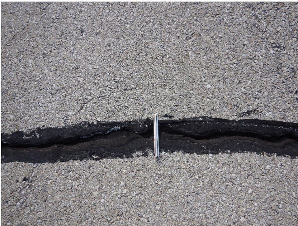
T02MT-01. L&T Cracking (Sample Unit No. 05).
