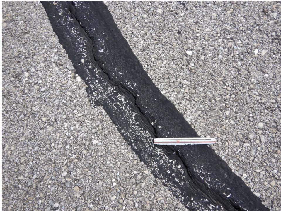
R18MT-03. L&T Cracking (Sample Unit No. 01).
