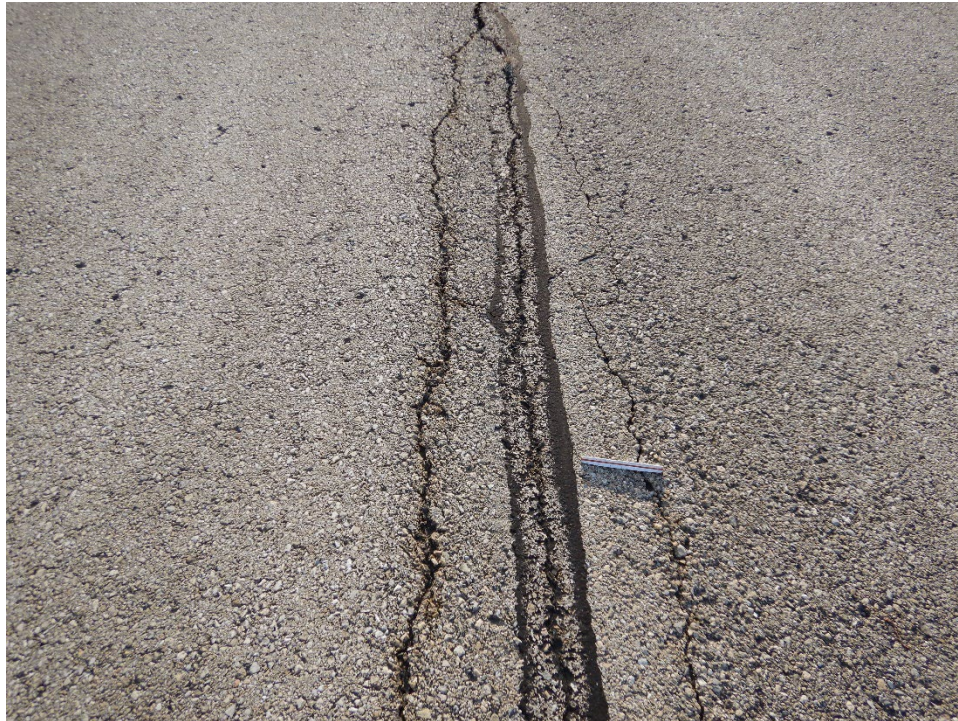
R13MT-02. Alligator Cracking (Sample Unit No. 75).
