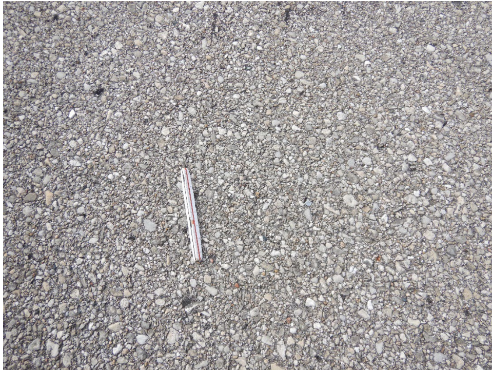
R18MT-02. Weathering (Sample Unit No. 03).
