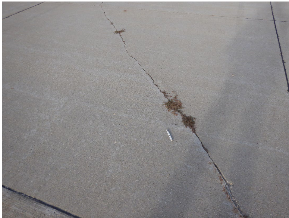
A02MT-01. LTD Cracking (Sample Unit No. 10).
