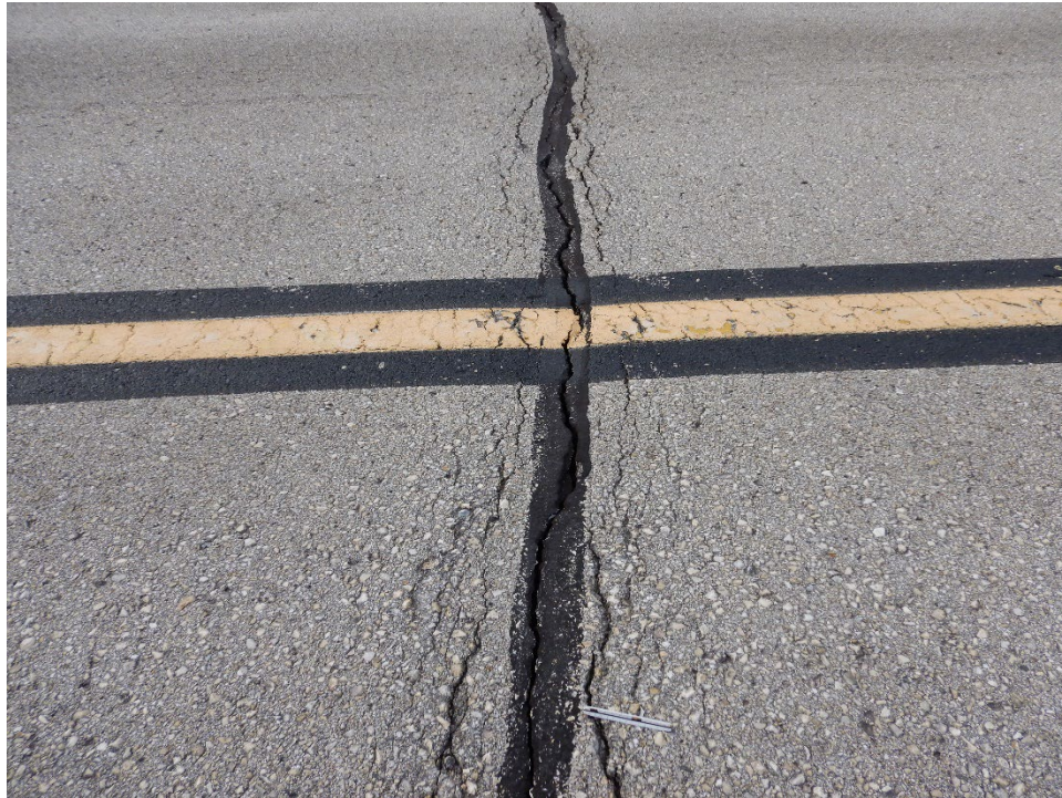
T03MT-01. L&T Cracking (Sample Unit No. 08).
