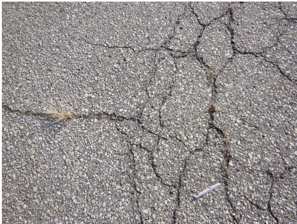
TH02MT-01. Alligator Cracking (Sample Unit No. 03).
