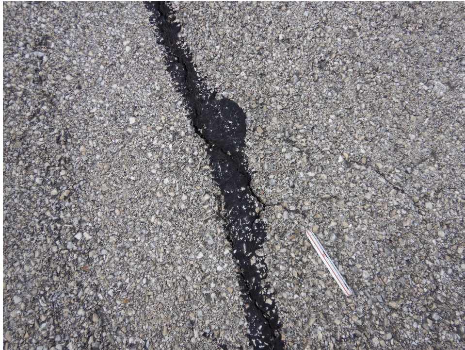
R13MT-03. L&T Cracking (Sample Unit No. 02).
