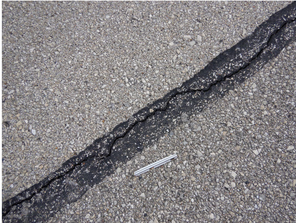
R18MT-02. L&T Cracking (Sample Unit No. 03).
