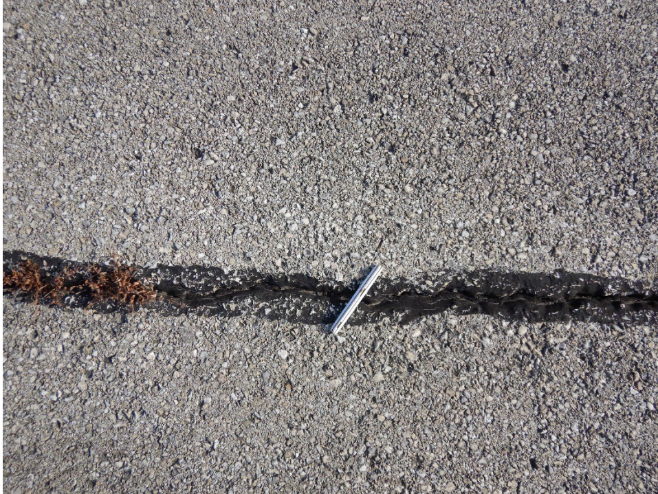
T02MT-02. L&T Cracking (Sample Unit No. 01).
