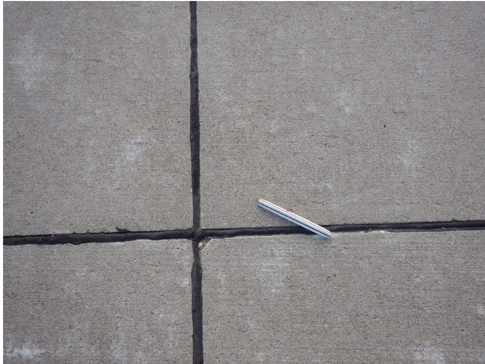
A03MT-01. Joint Seal Damage (Sample Unit No. 02).
