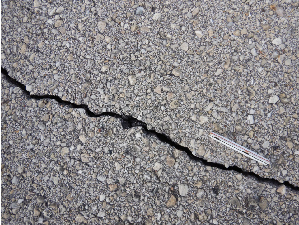
T03MT-01. L&T Cracking (Sample Unit No. 03).
