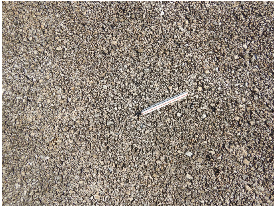
R13MT-04. Weathering (Sample Unit No. 01).
