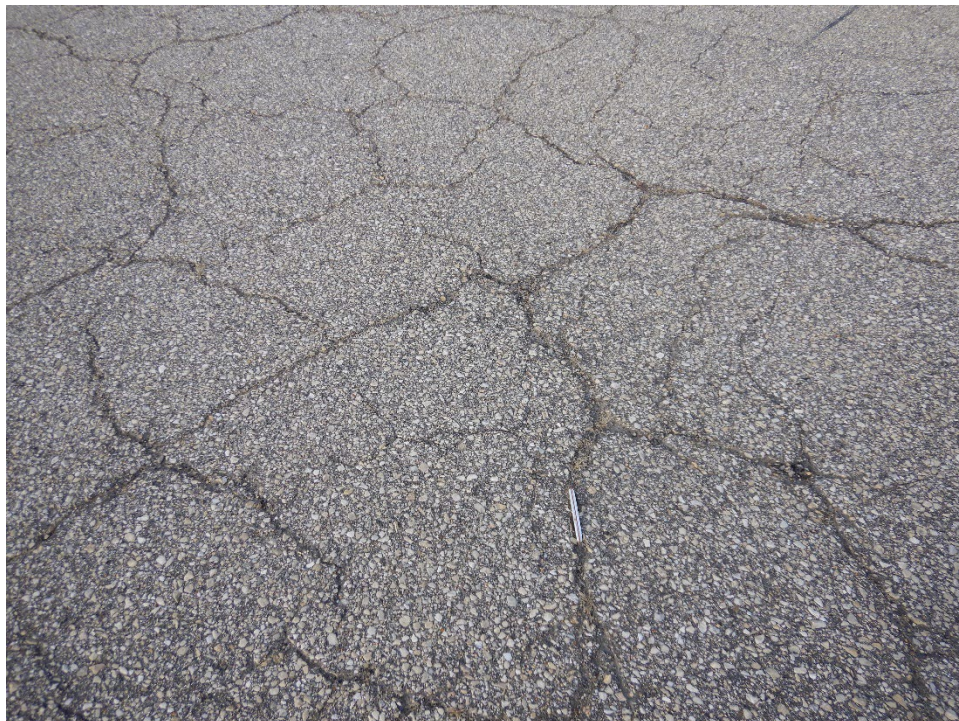
A02MT-02. Block Cracking (Sample Unit No. 02).
