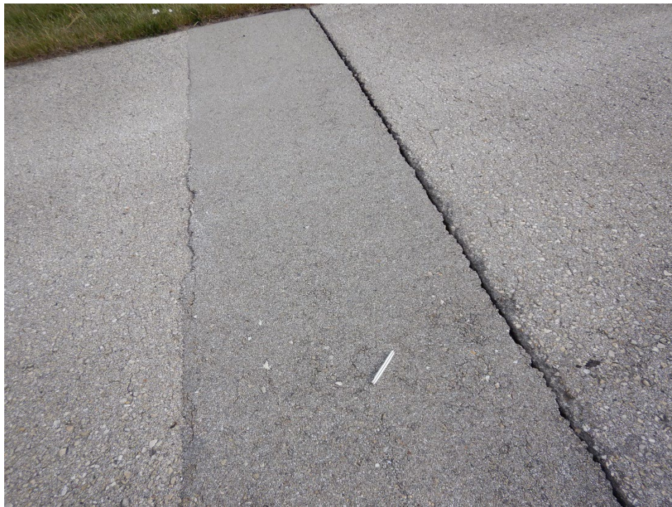
T03MT-01. Patching (Sample Unit No. 03).
