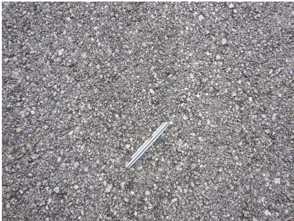
R18MT-03. Weathering (Sample Unit No. 01).
