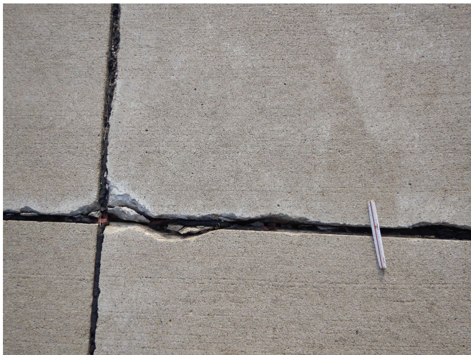
A01MT-01. Joint Seal Damage (Sample Unit No. 11).
