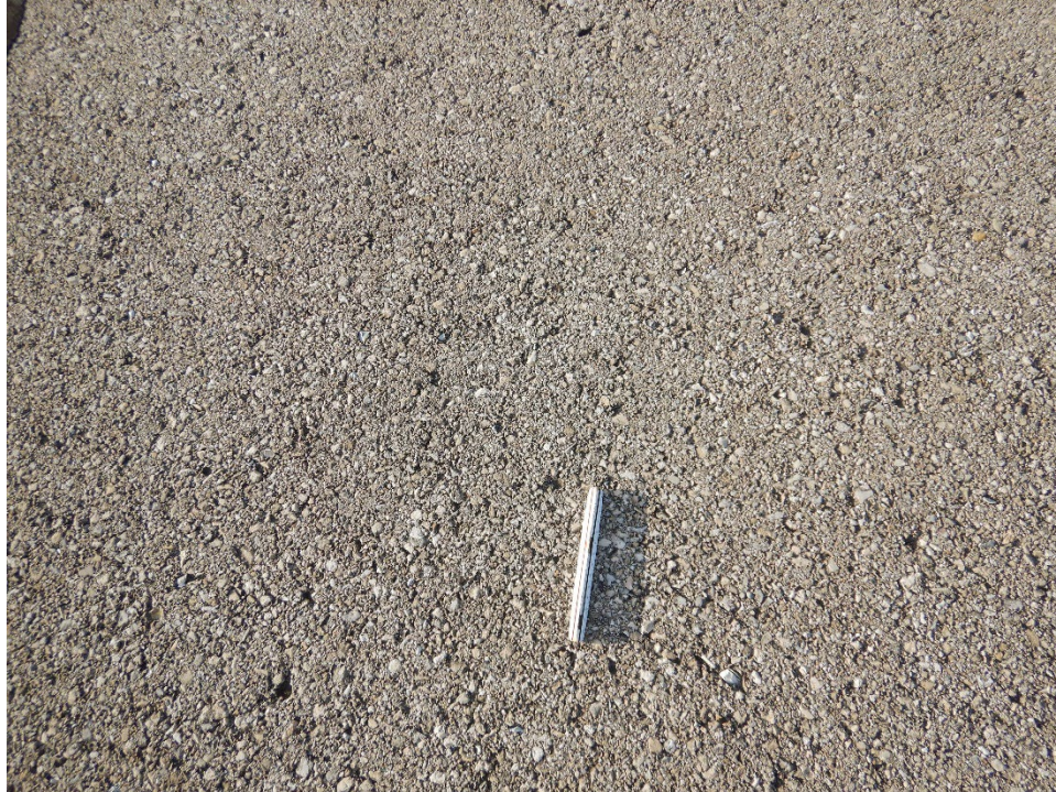
R13MT-02. Weathering (Sample Unit No. 75).
