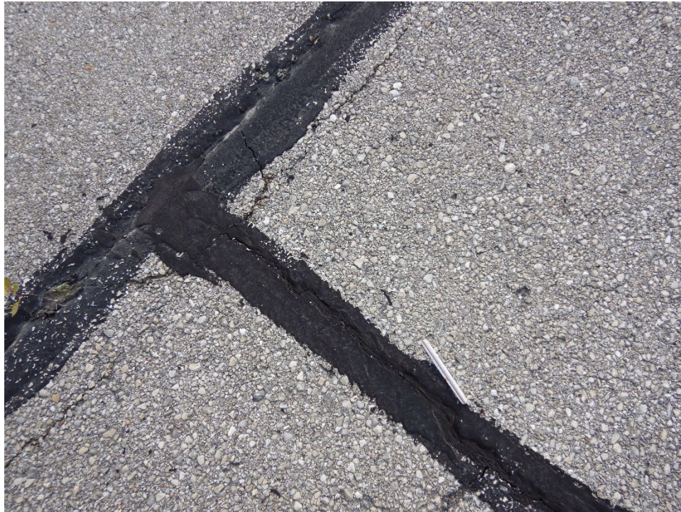
T03MT-02. L&T Cracking (Sample Unit No. 01).
