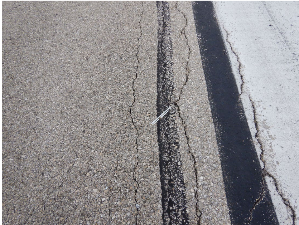
R13MT-01. Alligator Cracking (Sample Unit No. 03).
