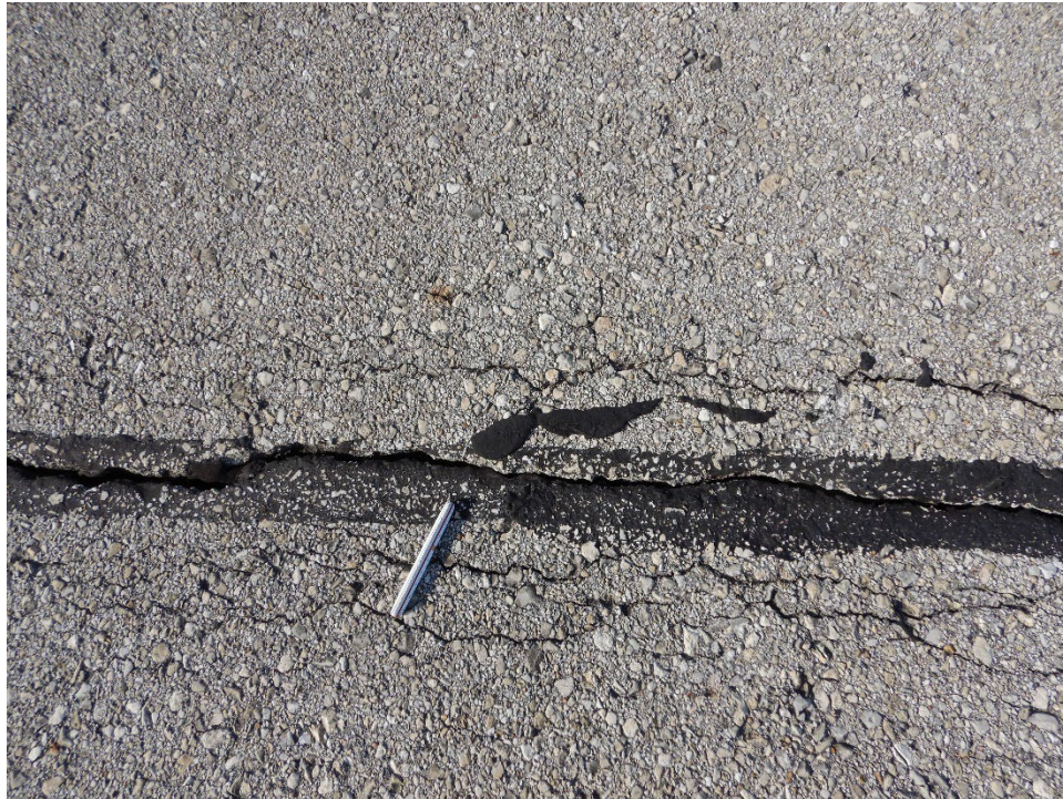
T04MT-01. L&T Cracking (Sample Unit No. 11).
