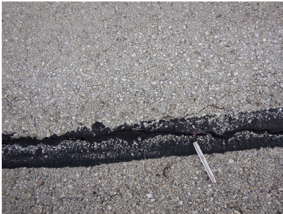
R13MT-01. L&T Cracking (Sample Unit No. 16).
