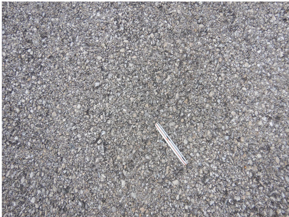
R13MT-03. Weathering (Sample Unit No. 02).
