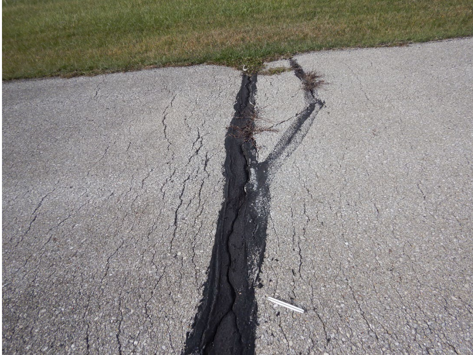
R18MT-01. L&T Cracking (Sample Unit No. 02) (1).
