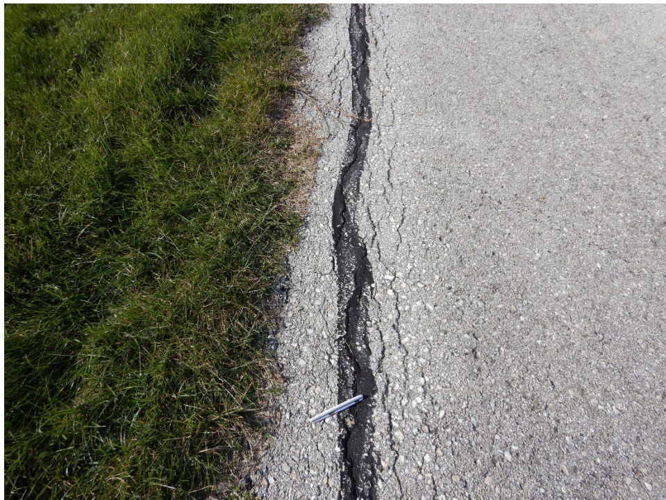
T04MT-01. Alligator Cracking (Sample Unit No. 11).
