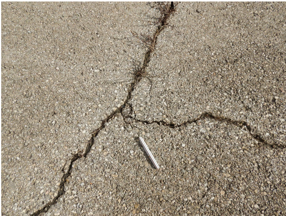
R18MT-04. L&T Cracking (Sample Unit No. 01).
