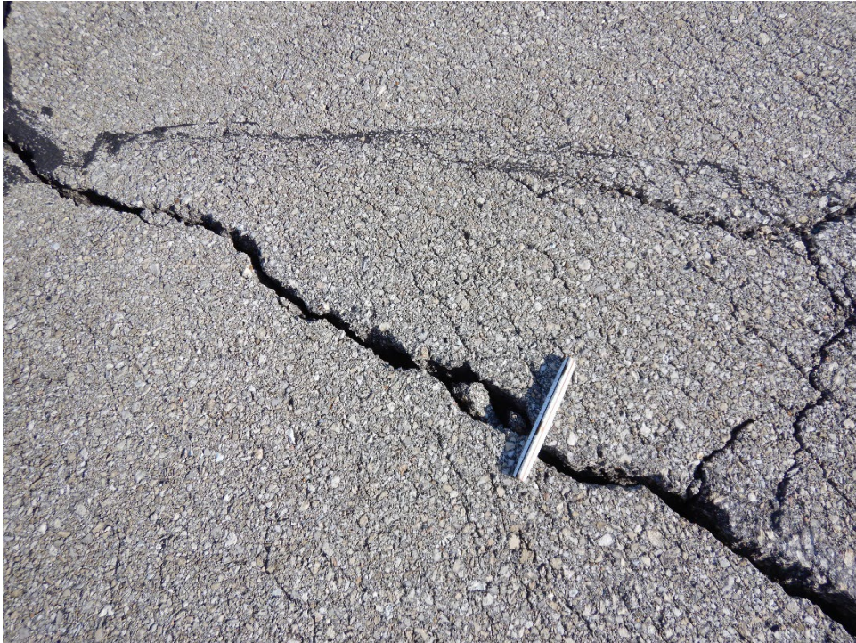
T03MT-03. L&T Cracking (Sample Unit No. 06).
