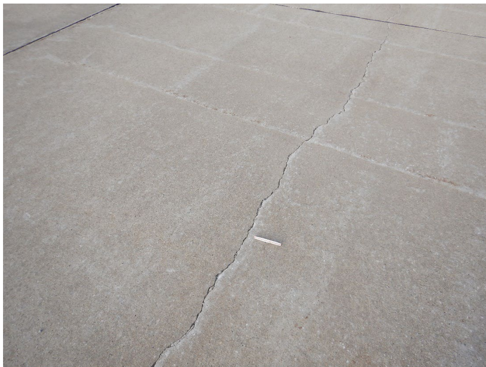
TH01MT-01. LTD Cracking (Additional Sample Unit No. 07).
