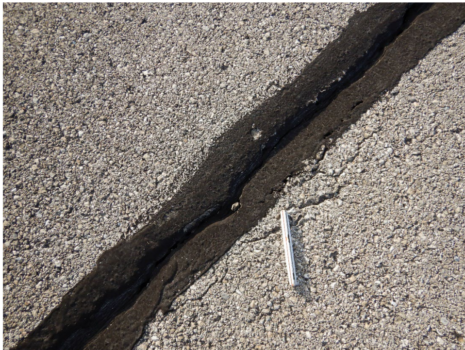
R13MT-02. L&T Cracking (Sample Unit No. 75).
