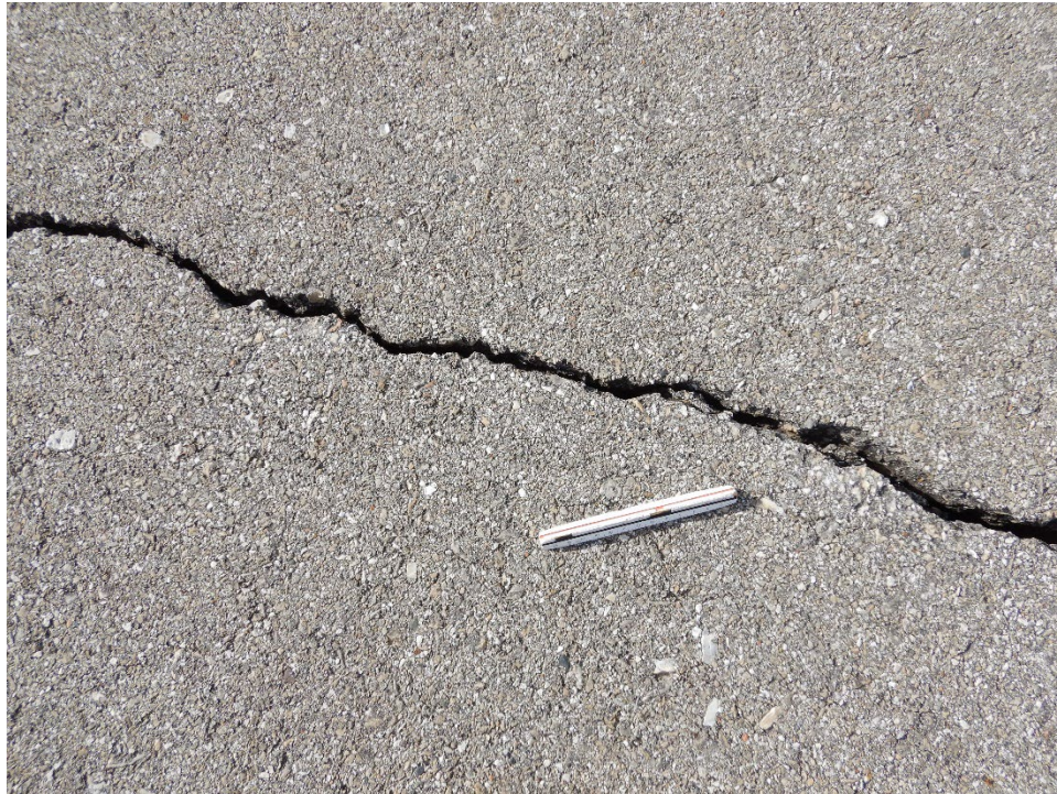
T01MT-01. L&T Cracking (Sample Unit No. 02).
