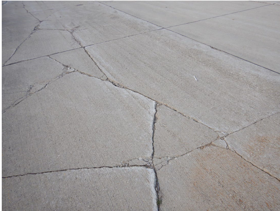
A01MT-01. Shattered Slab (Additional Sample Unit No. 23).
