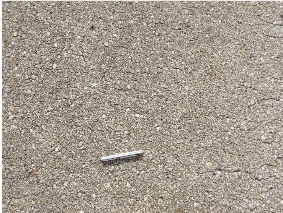
R18MT-01. Weathering (Sample Unit No. 02).
