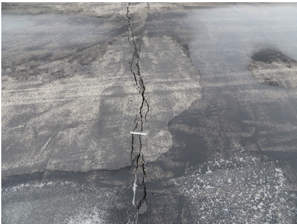
R09MD-03. L&T Cracking (Sample Unit No. 03).
