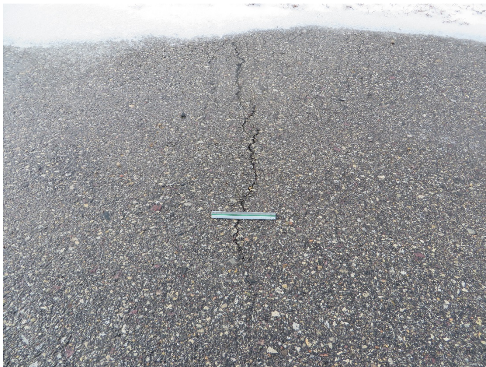
T01MD-01. L&T Cracking (Sample Unit No. 02).
