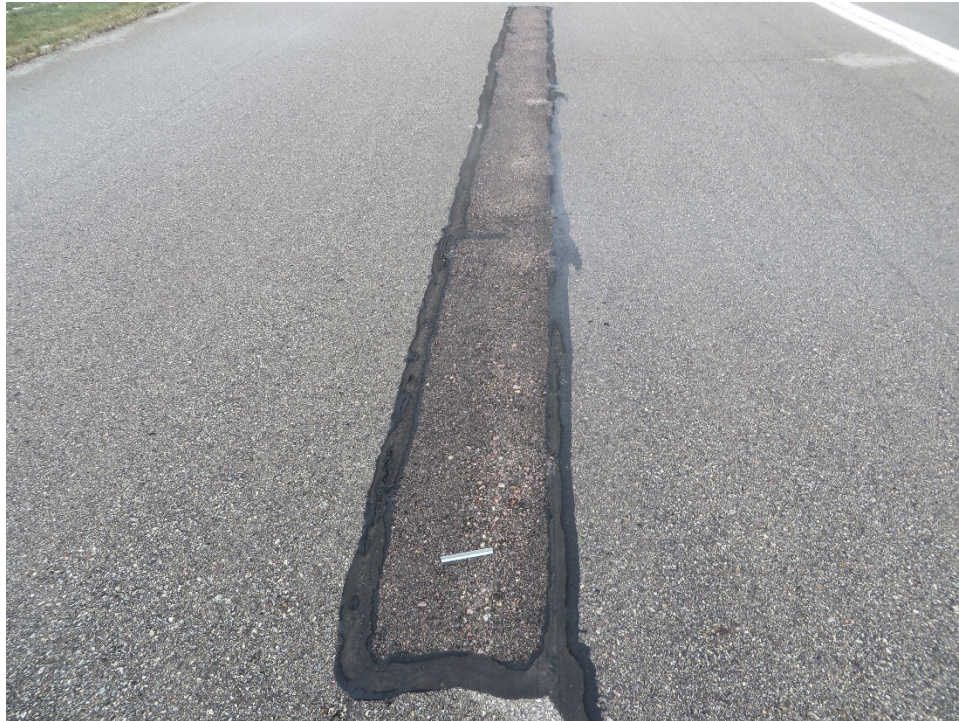
R09MD-01. Patching (Sample Unit No. 07).
