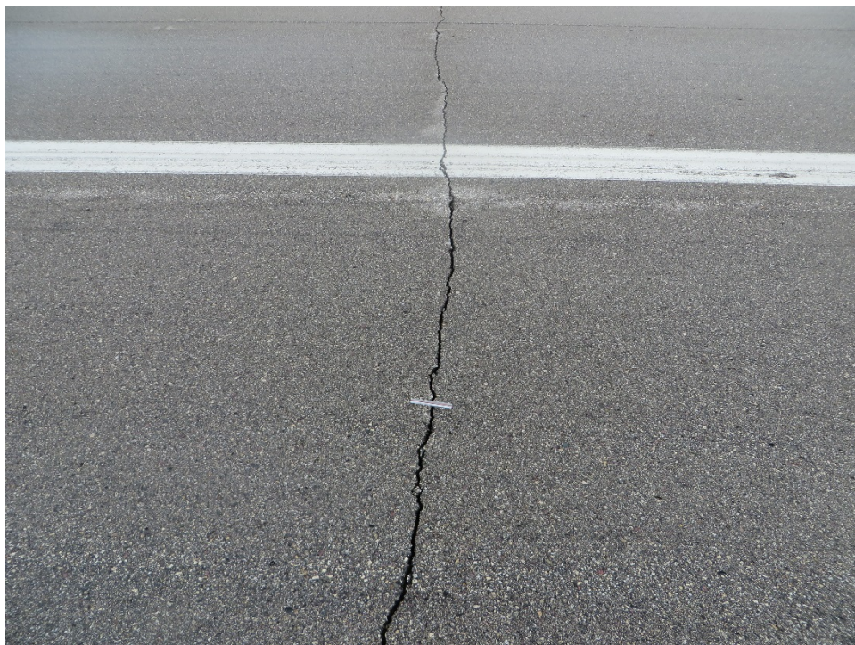
R09MD-01. L&T Cracking (Sample Unit No. 07).
