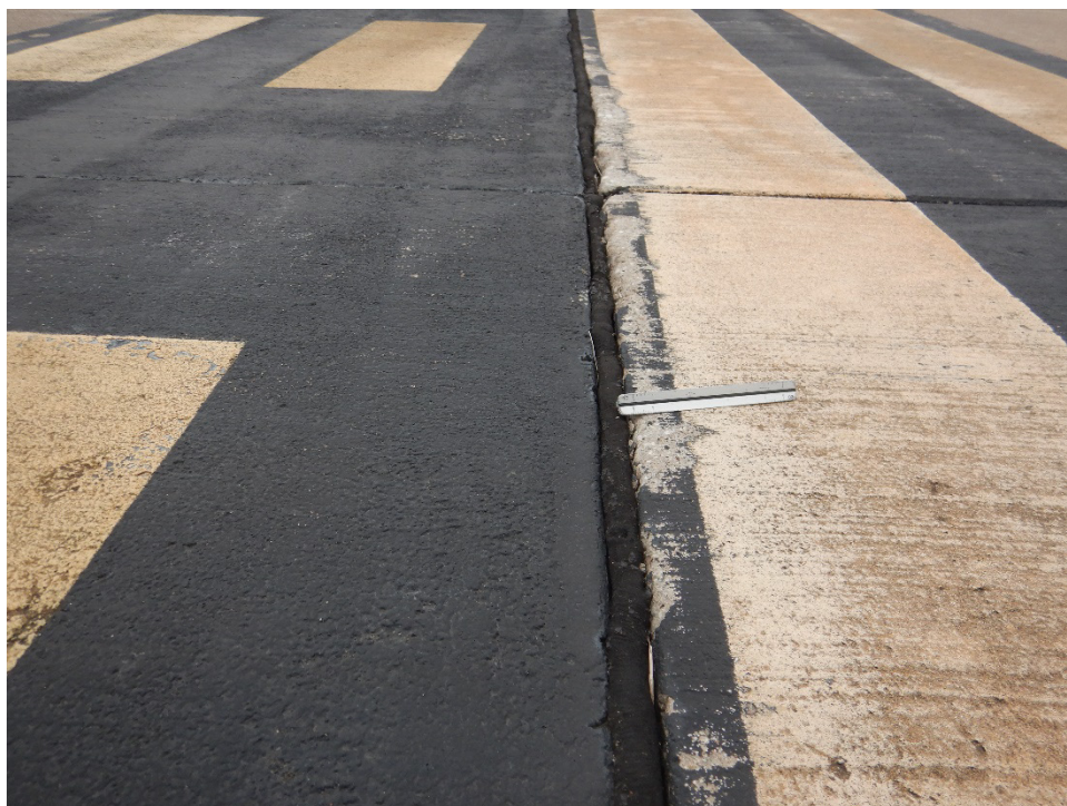
TBMU-04. Faulting (Sample Unit No. 06).
