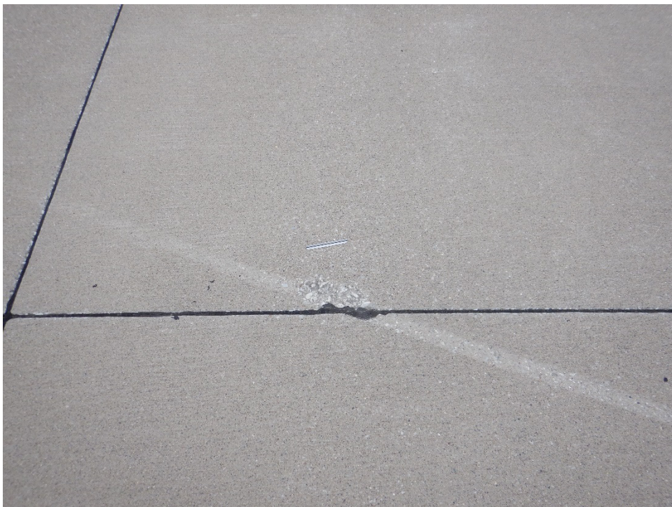
TA1MU-02. Joint Spalling (Sample Unit No. 04).
