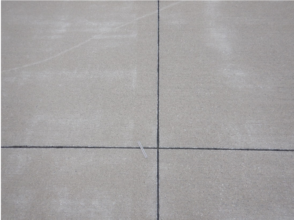
TAMU-05. Joint Seal Damage (Sample Unit No. 04).
