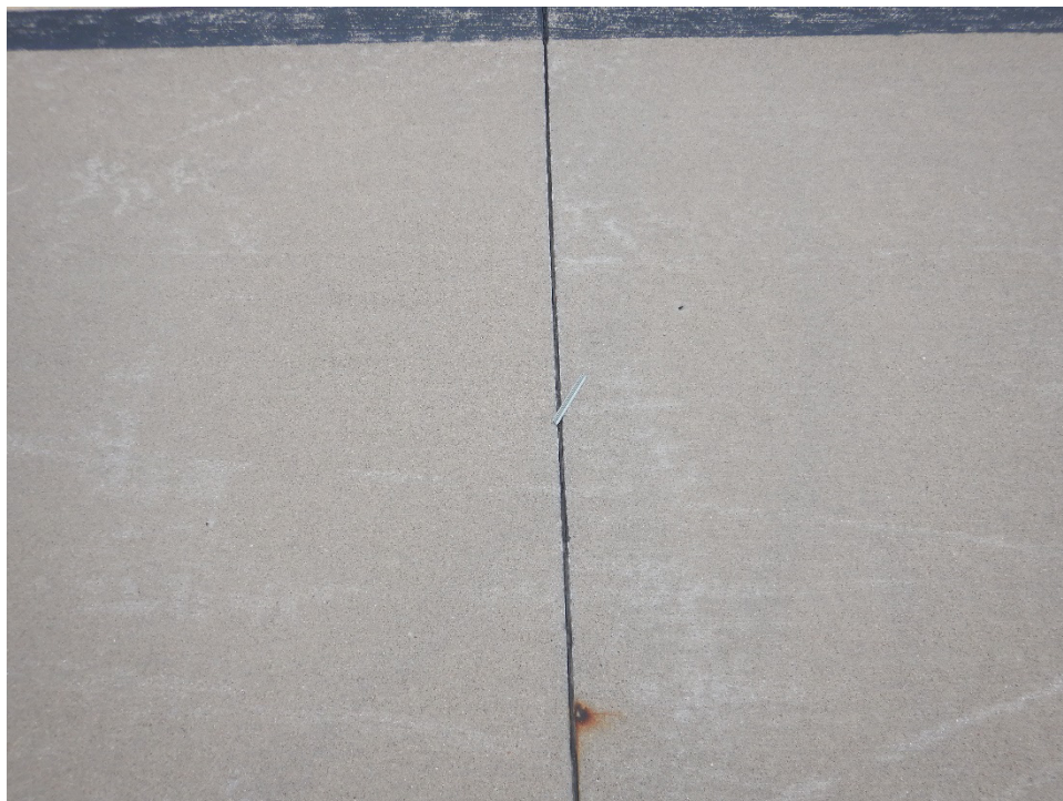
TAMU-01. Joint Seal Damage (Sample Unit No. 04).
