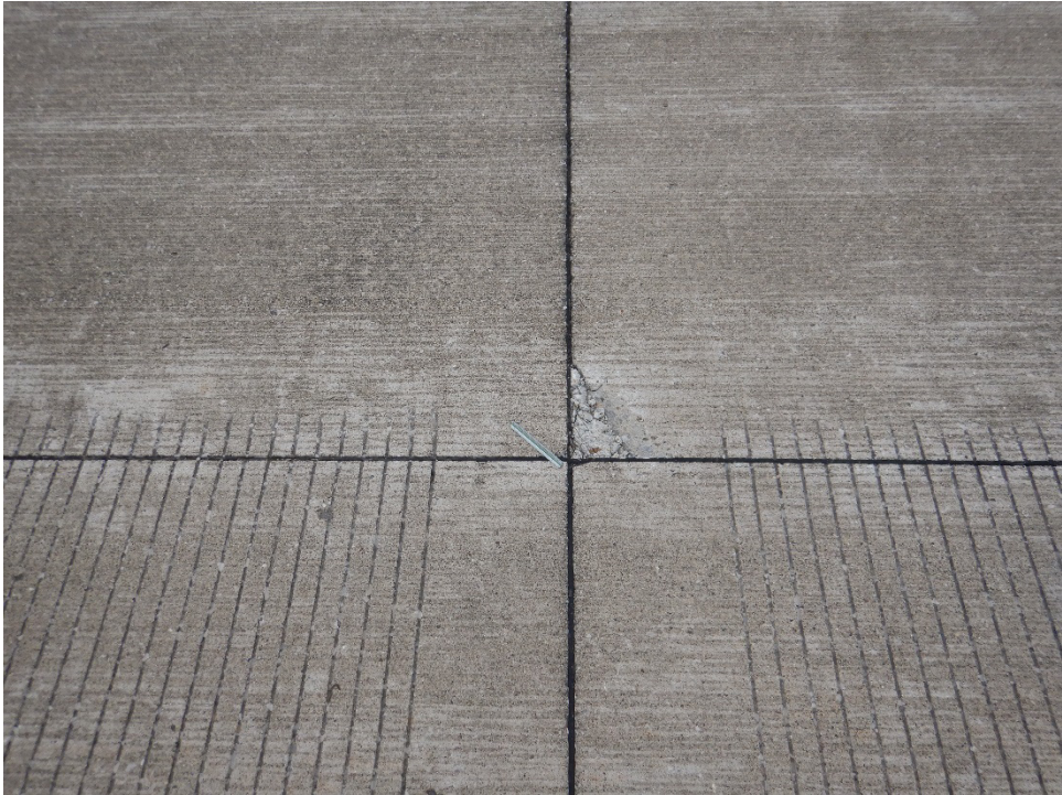
R12MU-01. Corner Spalling (Sample Unit No. 29).
