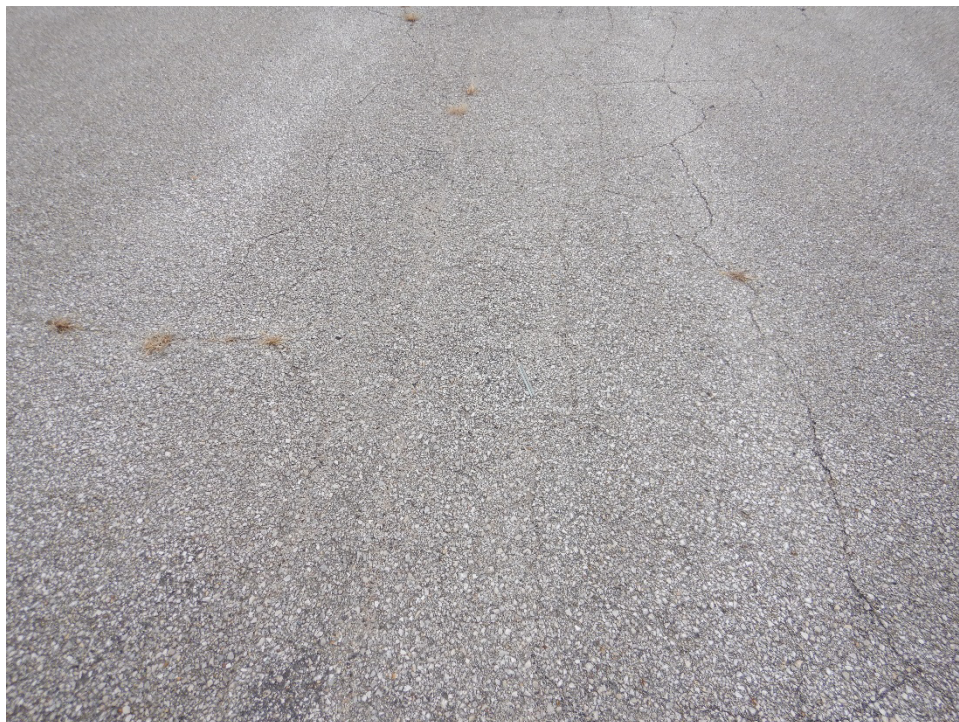
TH01MU-02. Alligator Cracking (Sample Unit No. 02).
