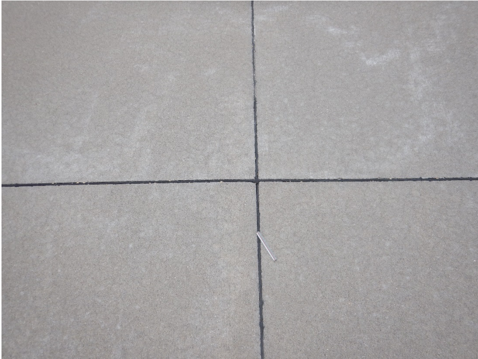
A01MU-02. Joint Seal Damage (Sample Unit No. 02).
