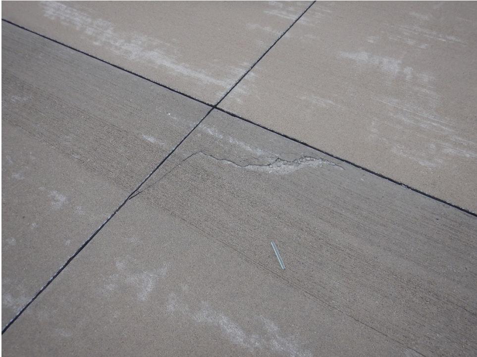
TCMU-01. Joint Spalling (Sample Unit No. 04).
