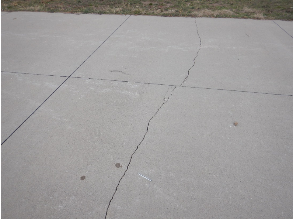
TH01MU-03. LTD Cracking (Sample Unit No. 10).
