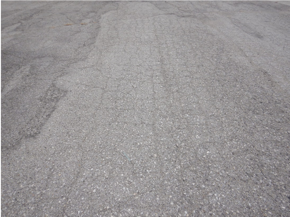
TH01MU-01. Alligator Cracking (Sample Unit No. 01).
