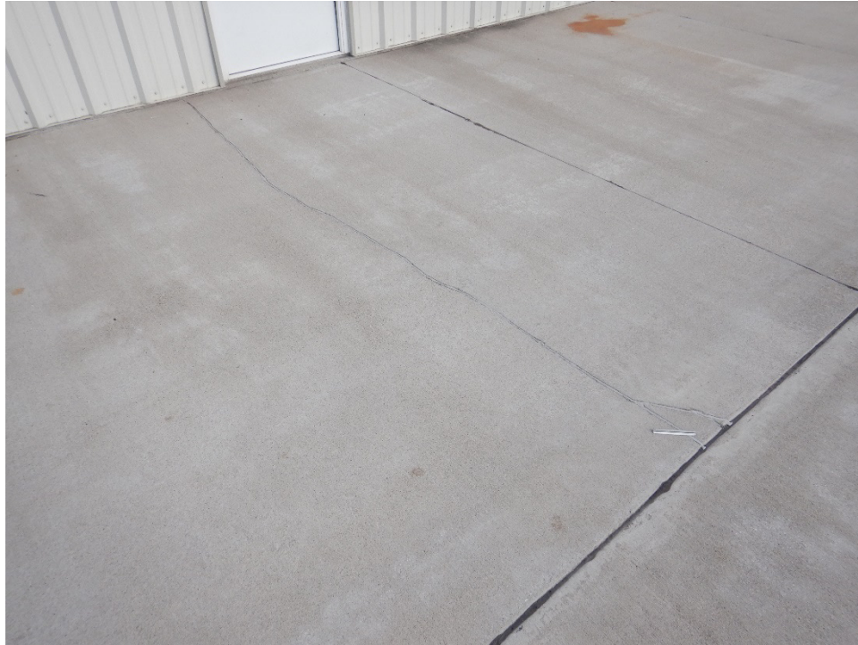
TH01MU-04. LTD Cracking (Sample Unit No. 04).
