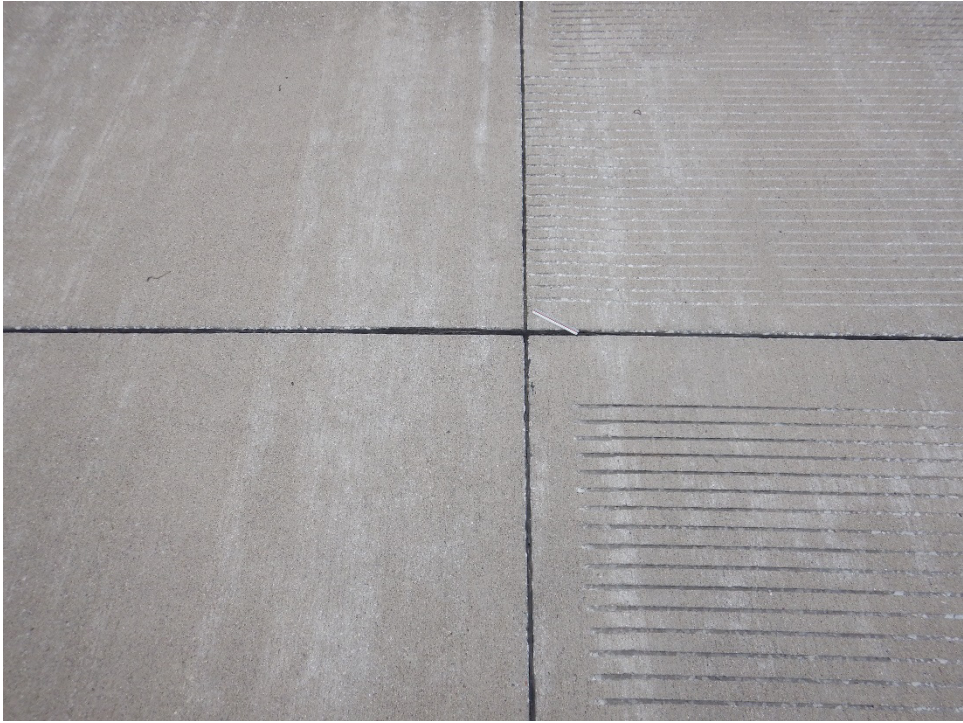
R06MU-01. Joint Seal Damage (Sample Unit No. 142).
