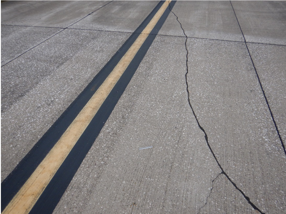
TBMU-02. LTD Cracking (Sample Unit No. 31).
