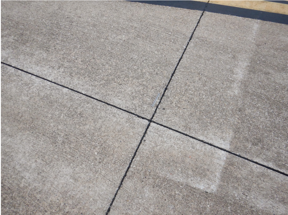
TBMU-03. Joint Seal Damage (Sample Unit No. 03).
