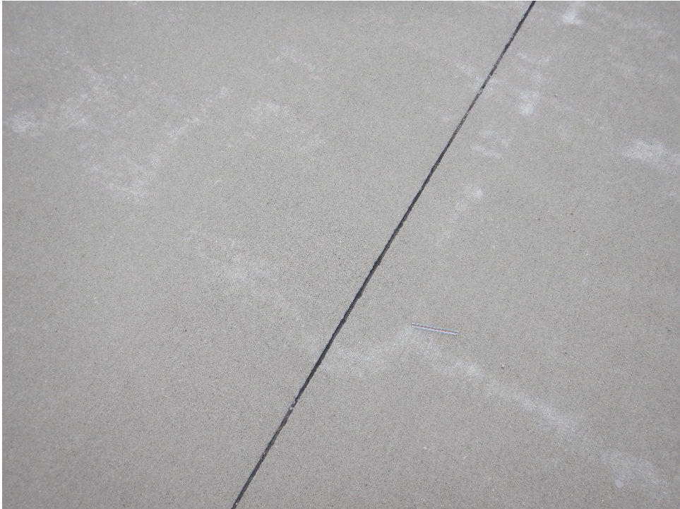
TH01MU-03. Joint Seal Damage (Sample Unit No. 08).
