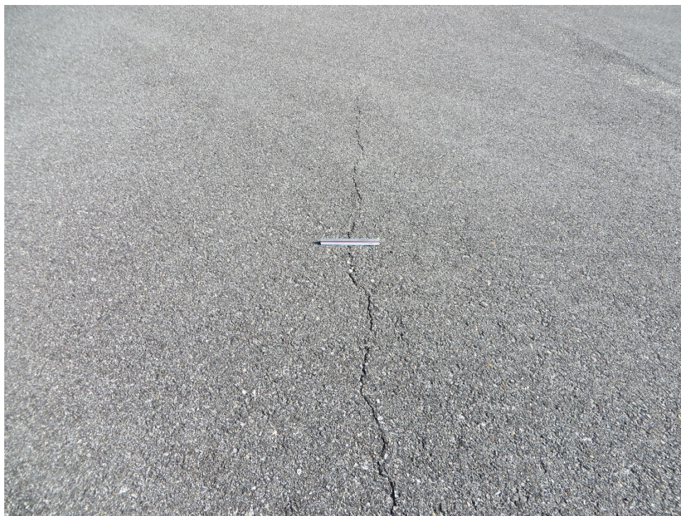
A01NH-01. L&T Cracking (Sample Unit No. 09).
