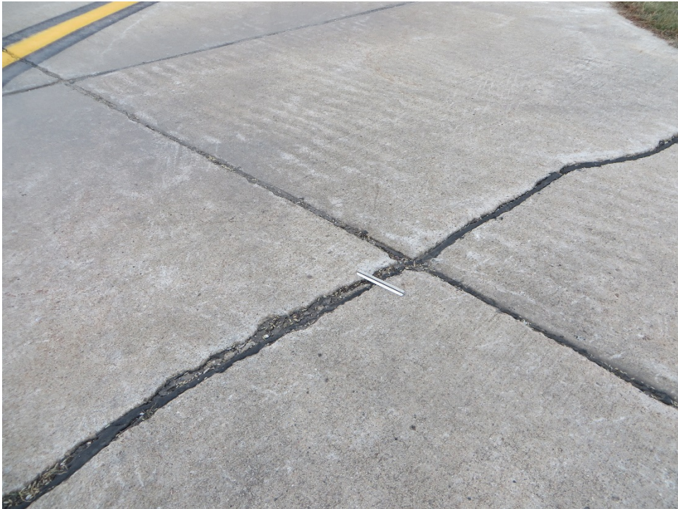
T02OS-02. LTD Cracking (Sample Unit No. 03).
