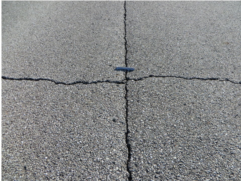
R17OS-02. Joint Reflection Cracking (Sample Unit No. 03).
