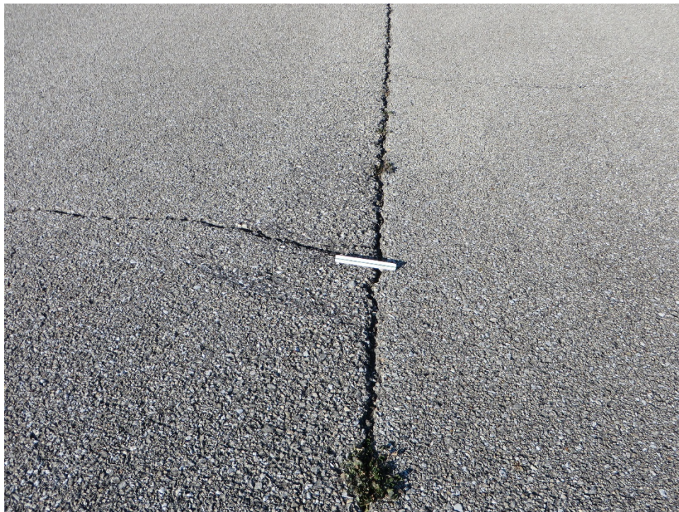
R17OS-01. L&T Cracking (Sample Unit No. 28).
