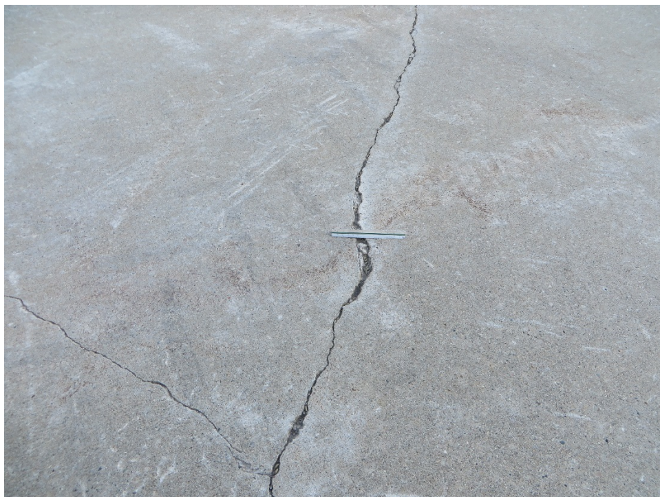
A01OS-02. LTD Cracking (Sample Unit No. 02).
