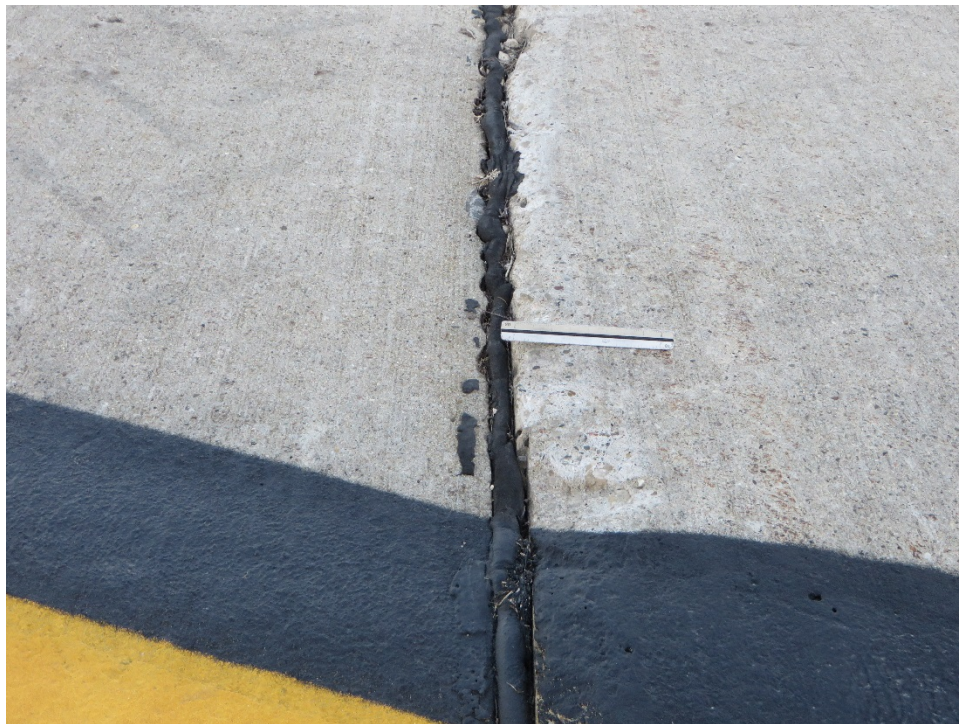
T02OS-02. Faulting (Sample Unit No. 03).
