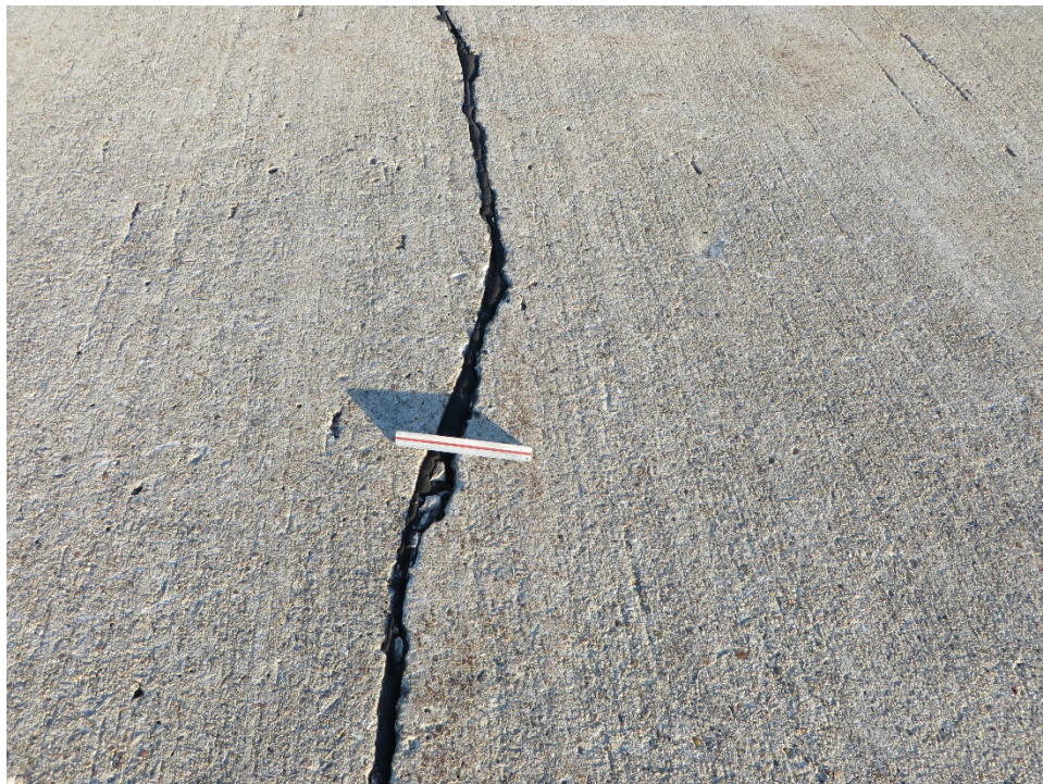
T01OS-01. LTD Cracking (Sample Unit No. 01).
