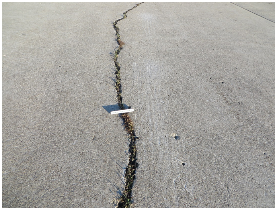
A01OS-01. LTD Cracking (Sample Unit No. 03).
