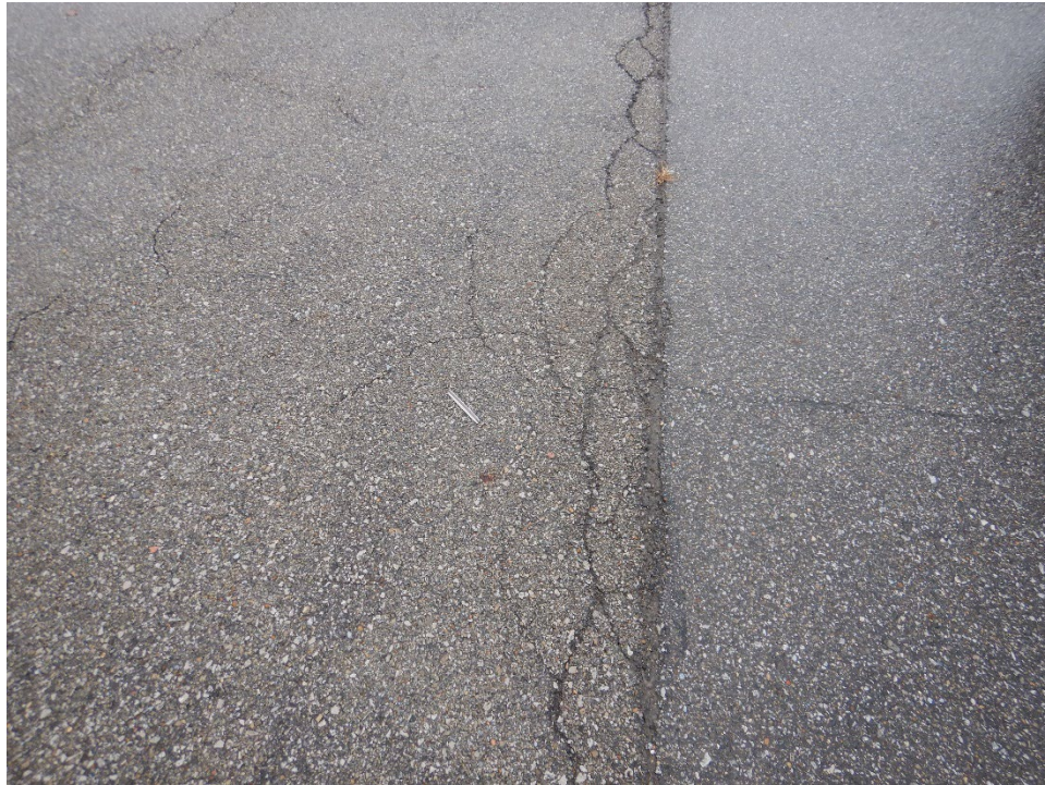
A02OT-04. Alligator Cracking (Sample Unit No. 01).
