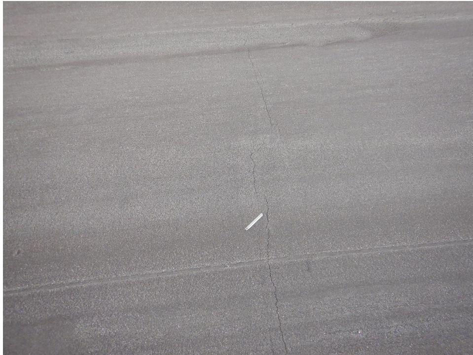
R04OT-02. Joint Reflection Cracking (Sample Unit No. 65).
