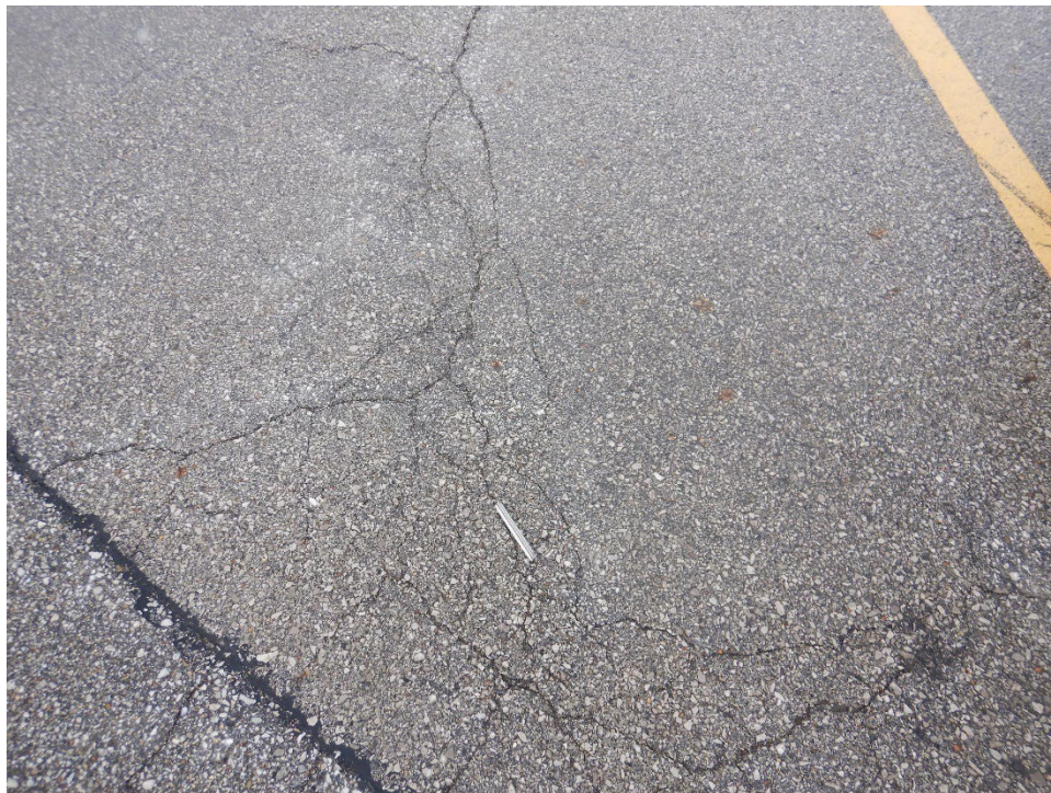
TAOT-02. Alligator Cracking (Sample Unit No. 01).
