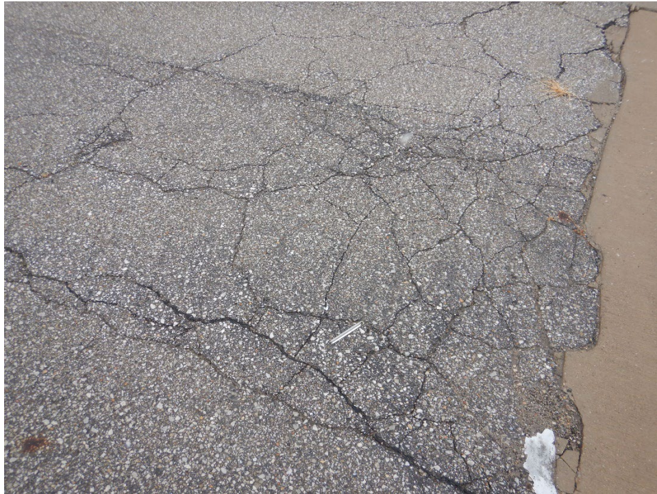
A01OT-05. Alligator Cracking (Sample Unit No. 01).
