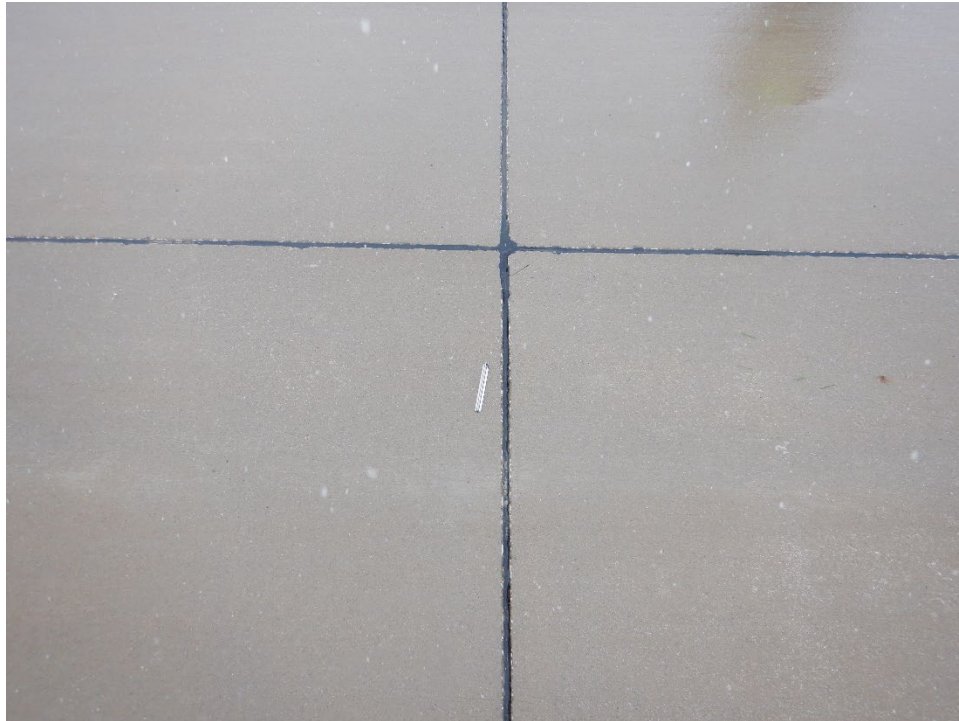
TAOT-07. Joint Seal Damage (Sample Unit No. 16).
