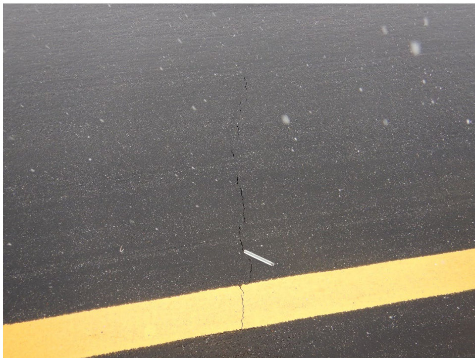
TBOT-04. L&T Cracking (Sample Unit No. 05).
