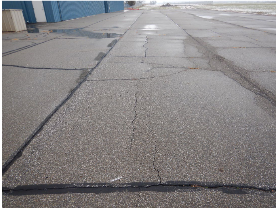
A02OT-03. L&T Cracking (Sample Unit No. 01).
