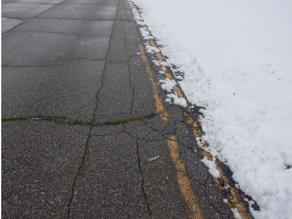
TAOT-06. Alligator Cracking (Sample Unit No. 14).
