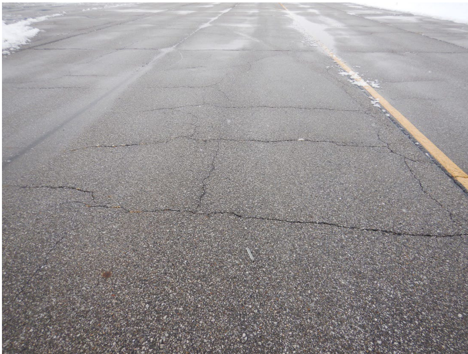
TAOT-06. Block Cracking (Sample Unit No. 06).
