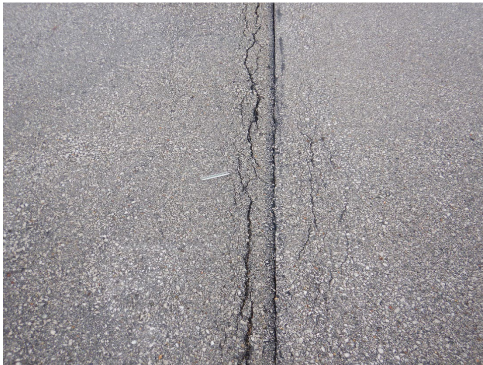
TAOT-04. L&T Cracking (Sample Unit No. 01).
