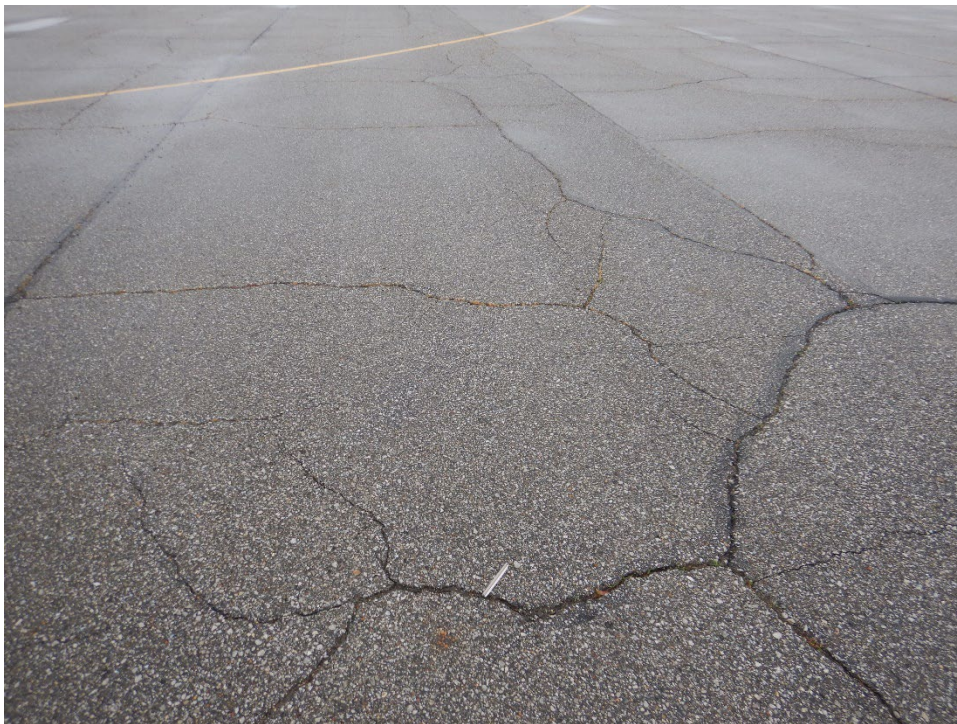
A01OT-02. Block Cracking (Sample Unit No. 06).
