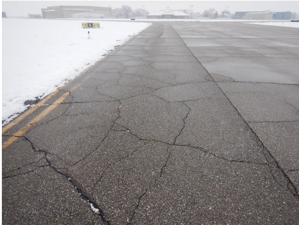
TBOT-01. Block Cracking (Sample Unit No. 02).
