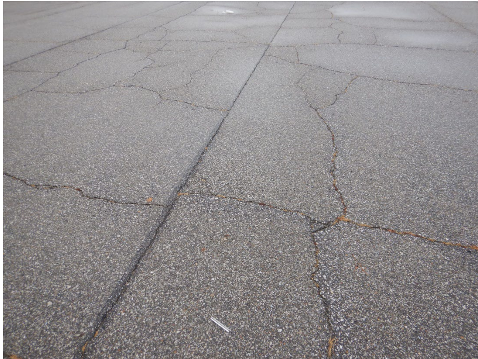
A02OT-01. Block Cracking (Sample Unit No. 09).
