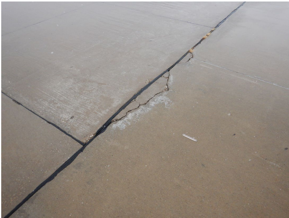
A01OT-08. Joint Spalling (Additional Sample Unit No. 13).
