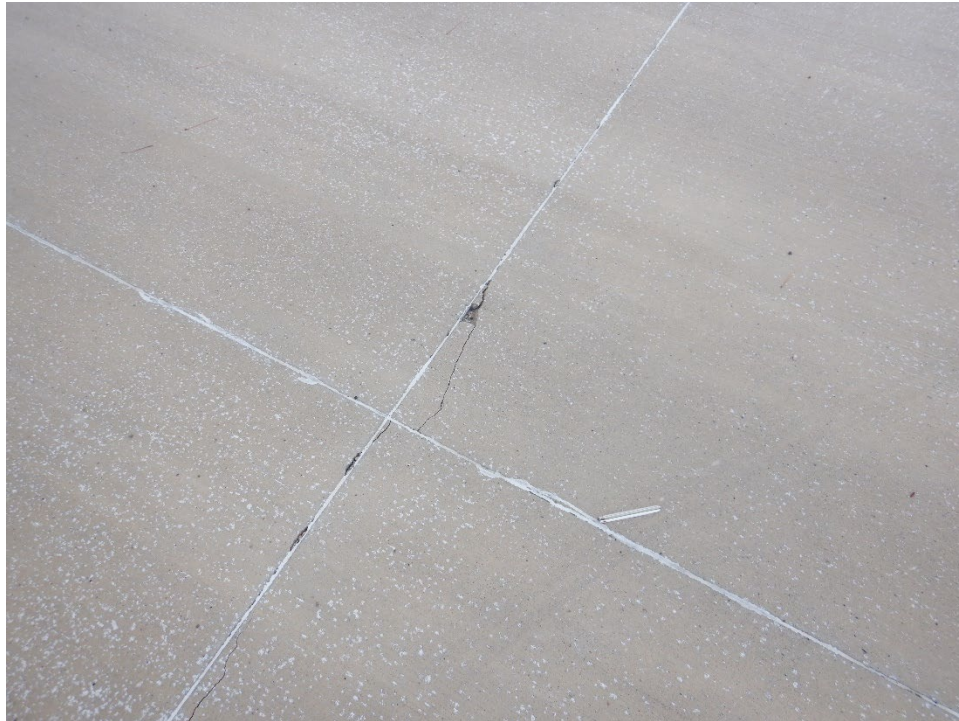
A01OT-03. Joint Spalling (Sample Unit No. 05).
