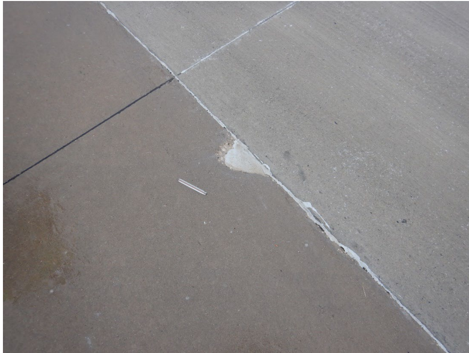
A01OT-07. Joint Spalling (Sample Unit No. 04).
