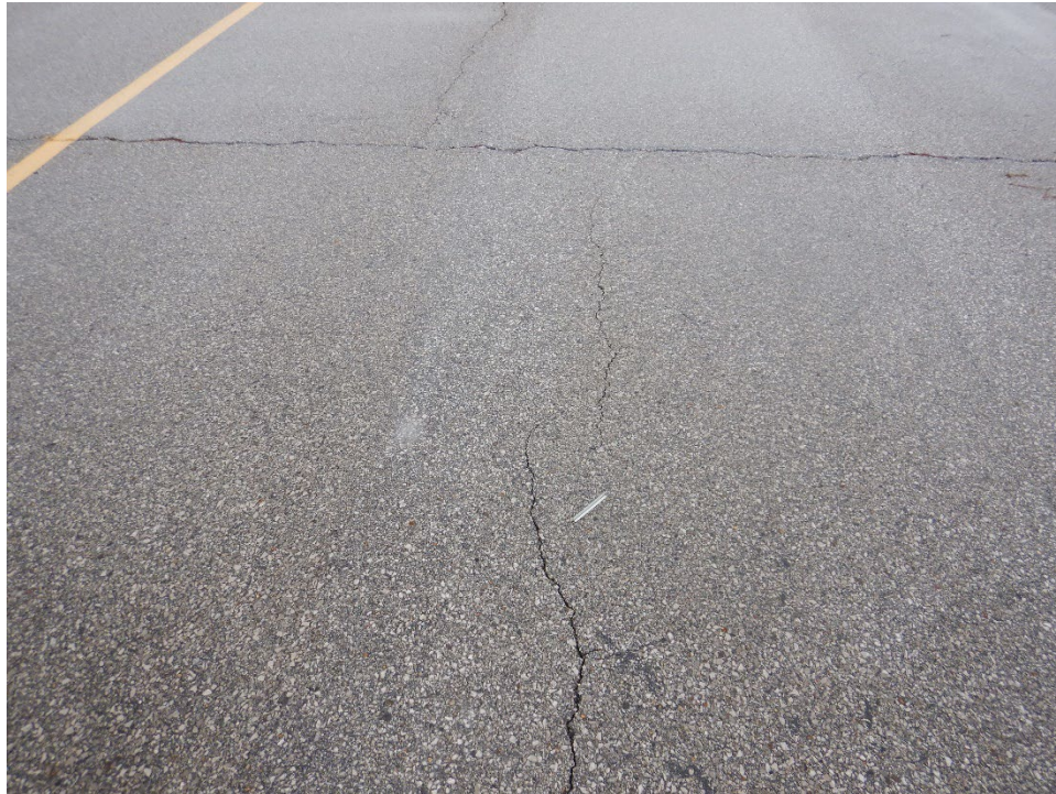
TAOT-02. L&T Cracking (Sample Unit No. 01).
