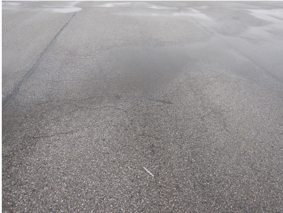
A02OT-02. Alligator Cracking (Sample Unit No. 04).
