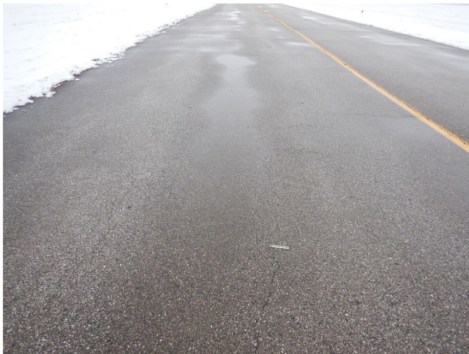
TAOT-03. Rutting (Sample Unit No. 11).
