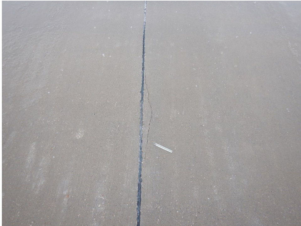
TAOT-08. Joint Spalling (Sample Unit No. 02).
