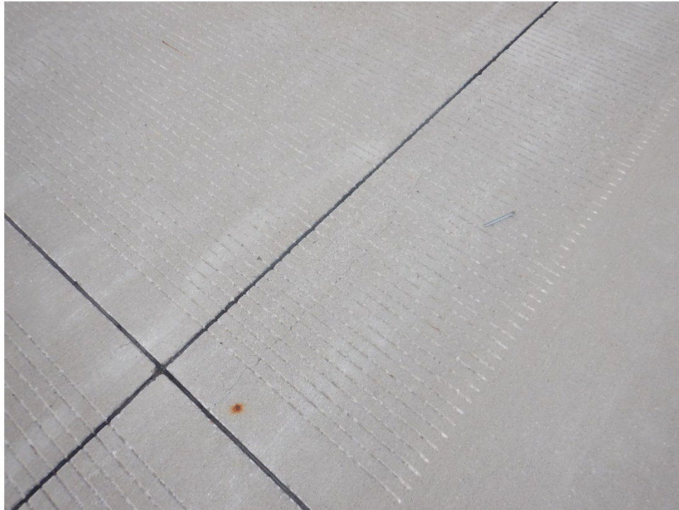
R13OT-01. Joint Spalling (Sample Unit No. 183).
