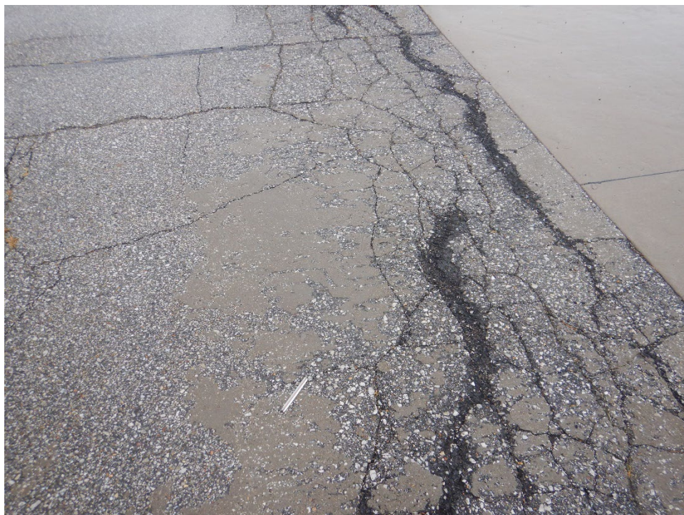
A01OT-01. Alligator Cracking (Sample Unit No. 02).
