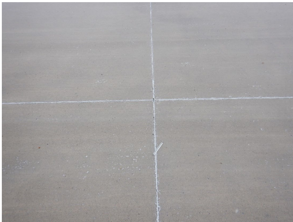
A01OT-03. Joint Seal Damage (Sample Unit No. 10).
