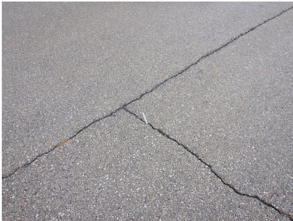
A02OT-04. L&T Cracking (Sample Unit No. 01).
