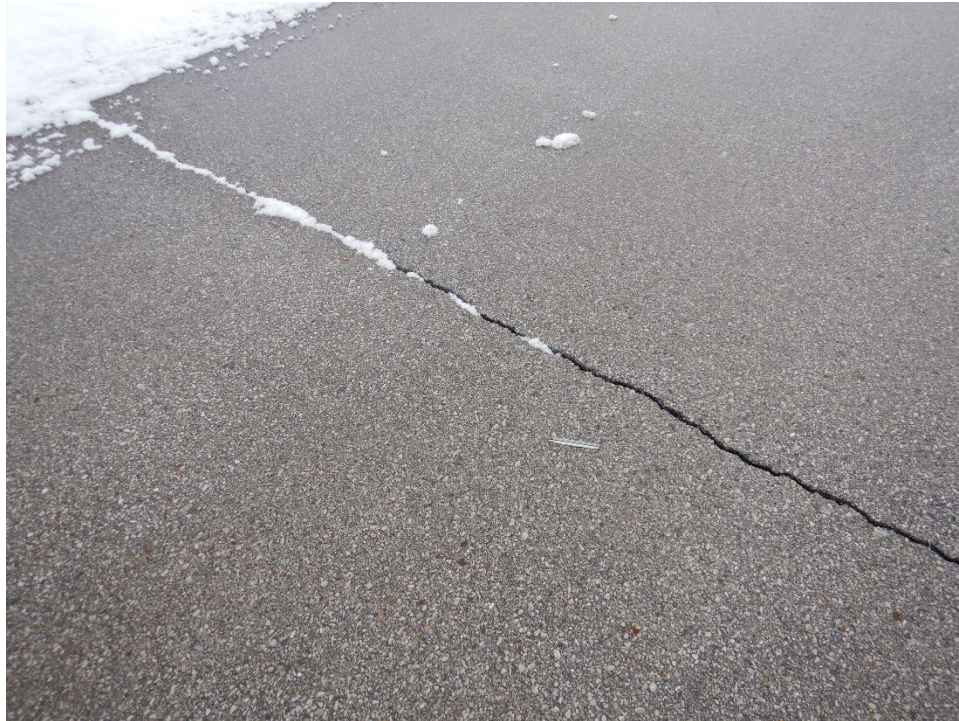
TAOT-01. L&T Cracking (Sample Unit No. 04).
