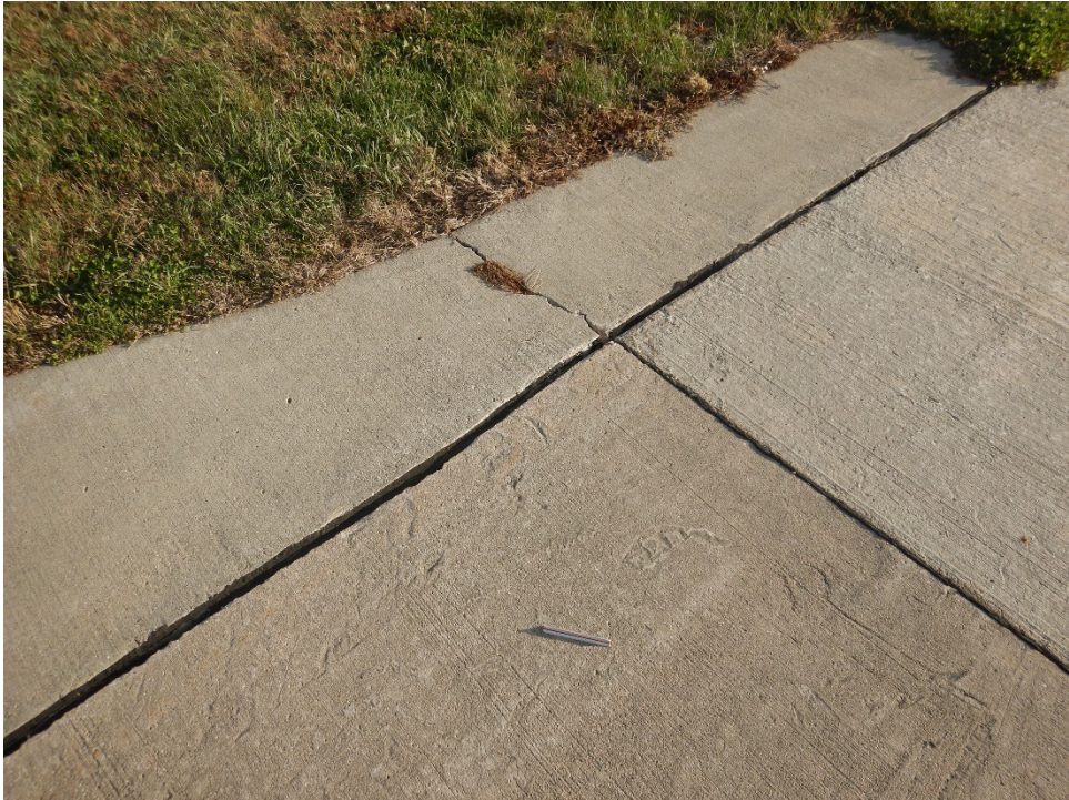
TH02PR-03. LTD Cracking (Sample Unit No. 01).
