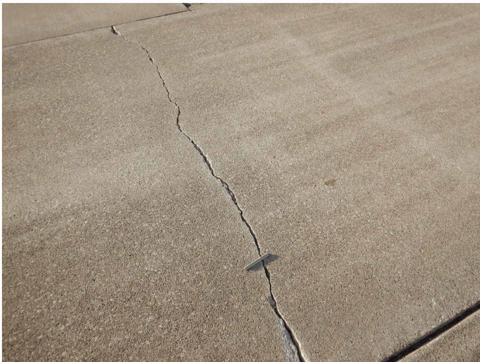
TH02PR-01. LTD Cracking (Sample Unit No. 01).
