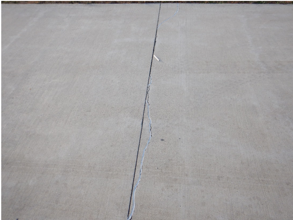
TH01PR-01. Joint Spalling (Sample Unit No. 04).
