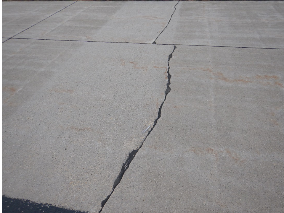
T01PR-01. LTD Cracking (Sample Unit No. 01).
