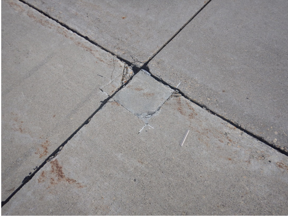
T02PR-01. Small Patching (Sample Unit No. 28).
