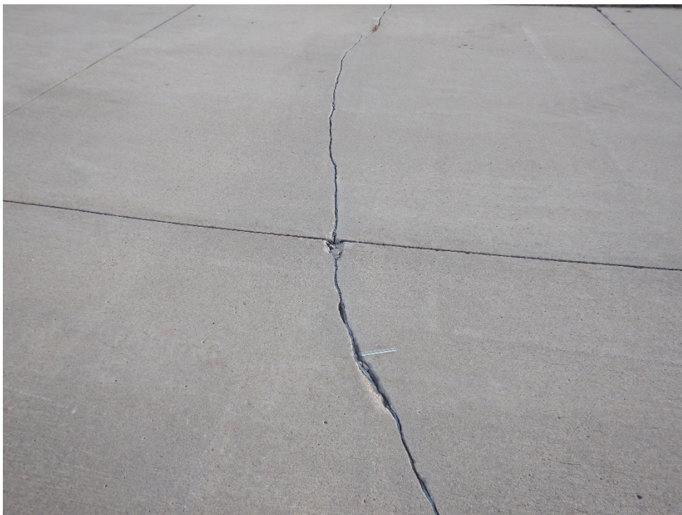
TH01PR-02. LTD Cracking (Sample Unit No. 01).
