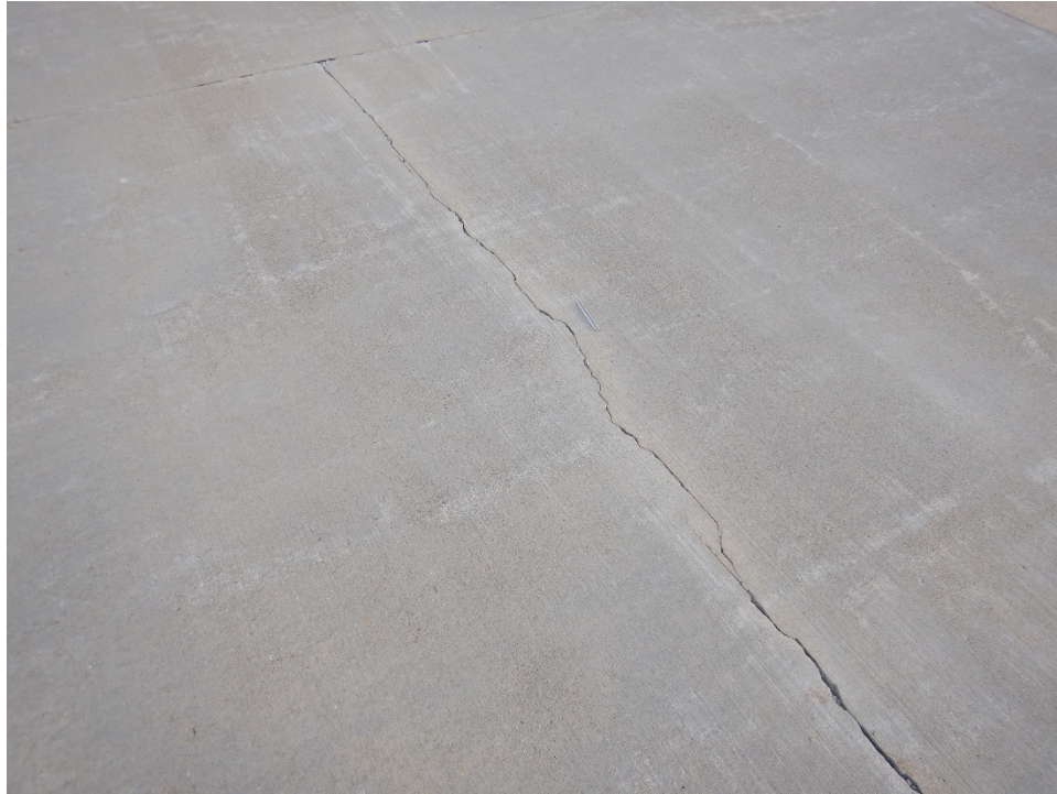
A01PR-01. LTD Cracking (Sample Unit No. 05).
