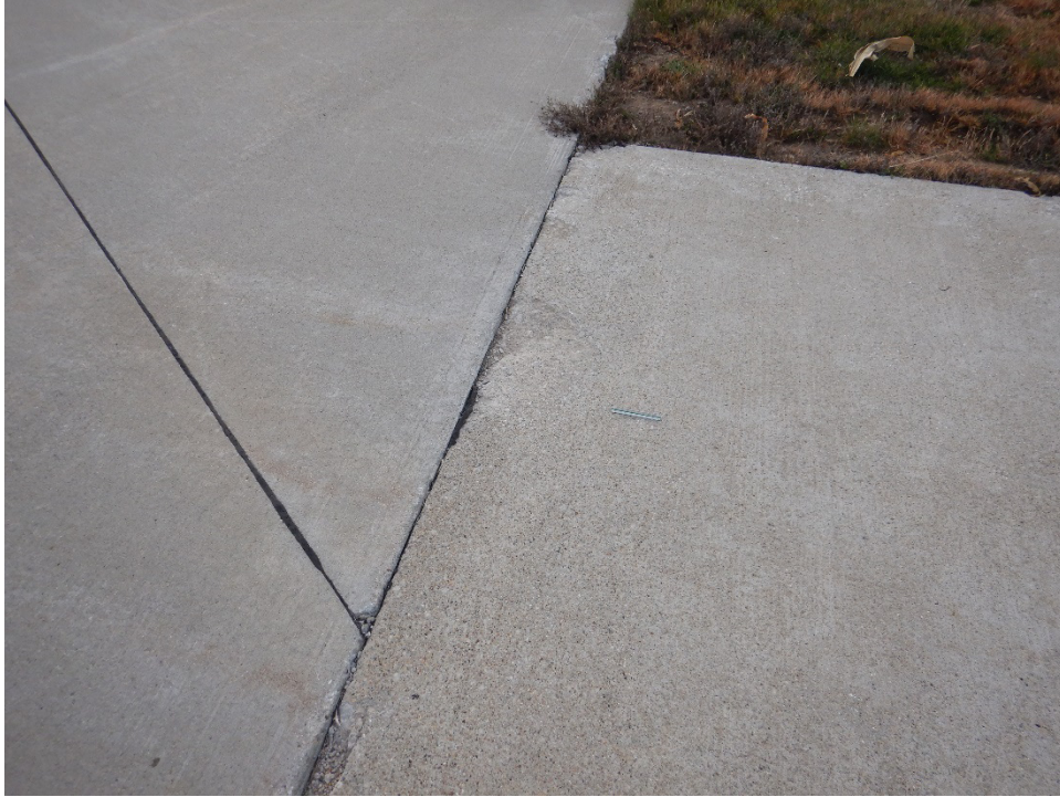
T01PR-02. Joint Spalling (Sample Unit No. 03).
