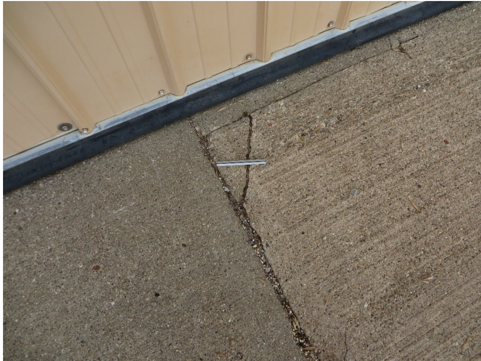
A01RR-02. Corner Spalling (Sample Unit No. 02).
