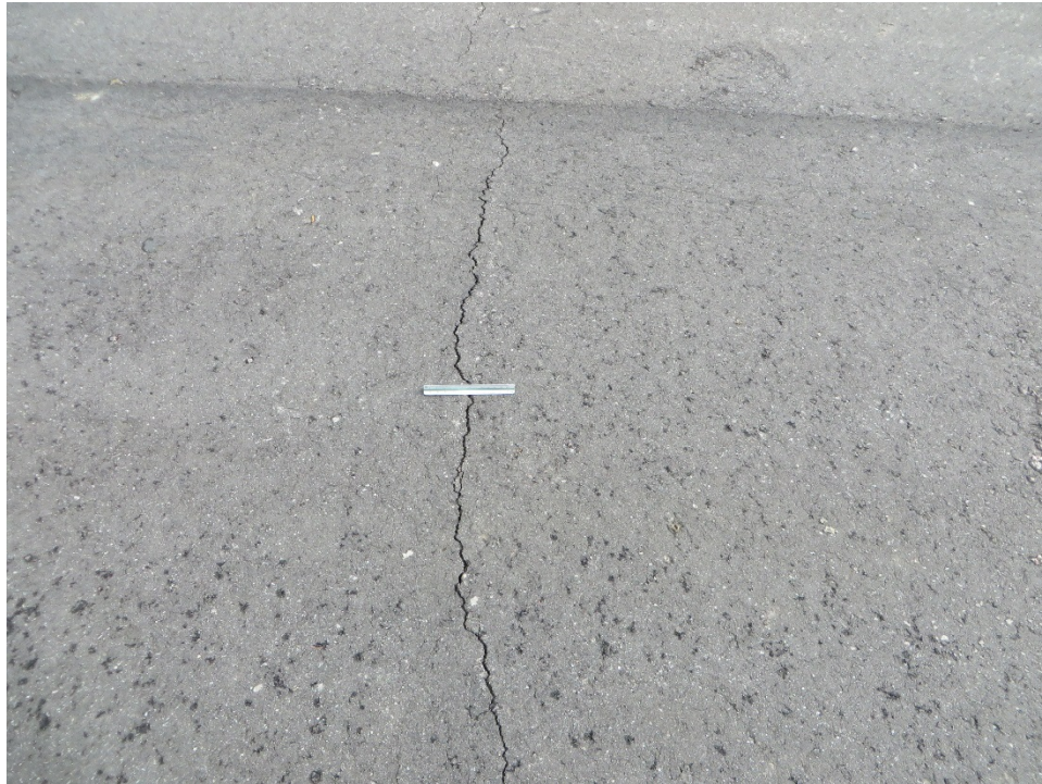
R16RR-03. L&T Cracking (Sample Unit No. 01).
