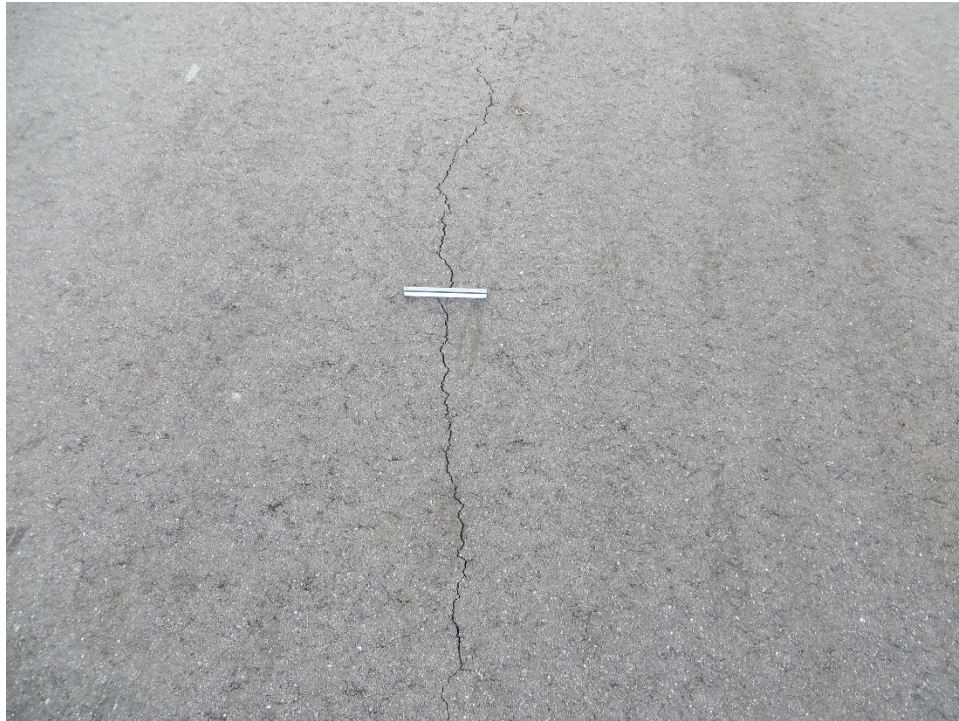
R16RR-01. L&T Cracking (Sample Unit No. 01).
