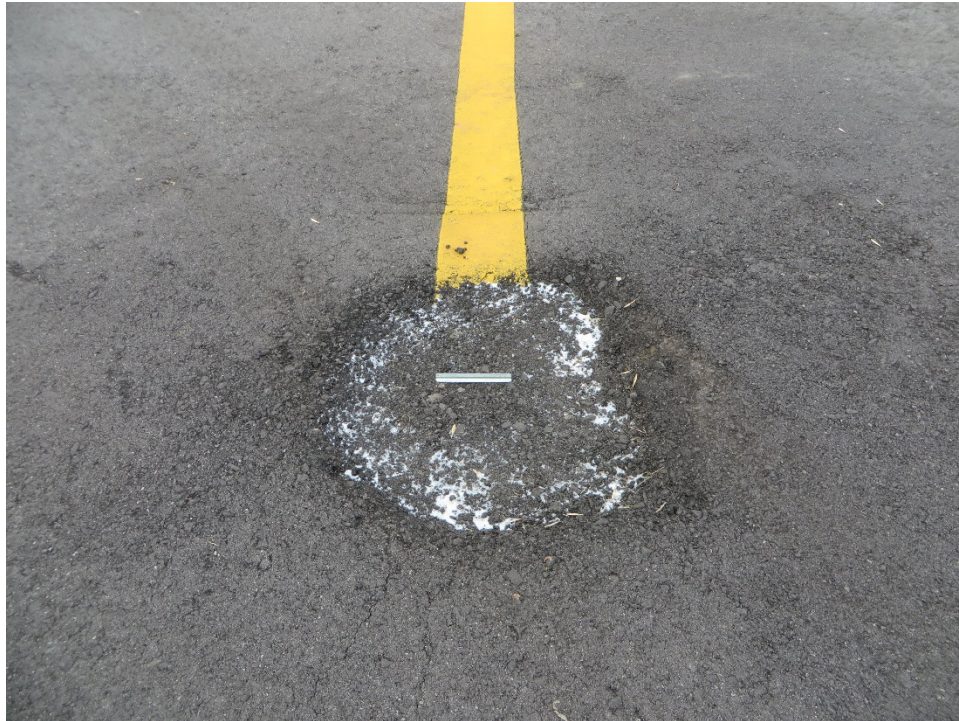
A01RR-01. Raveling (Sample Unit No. 03).
