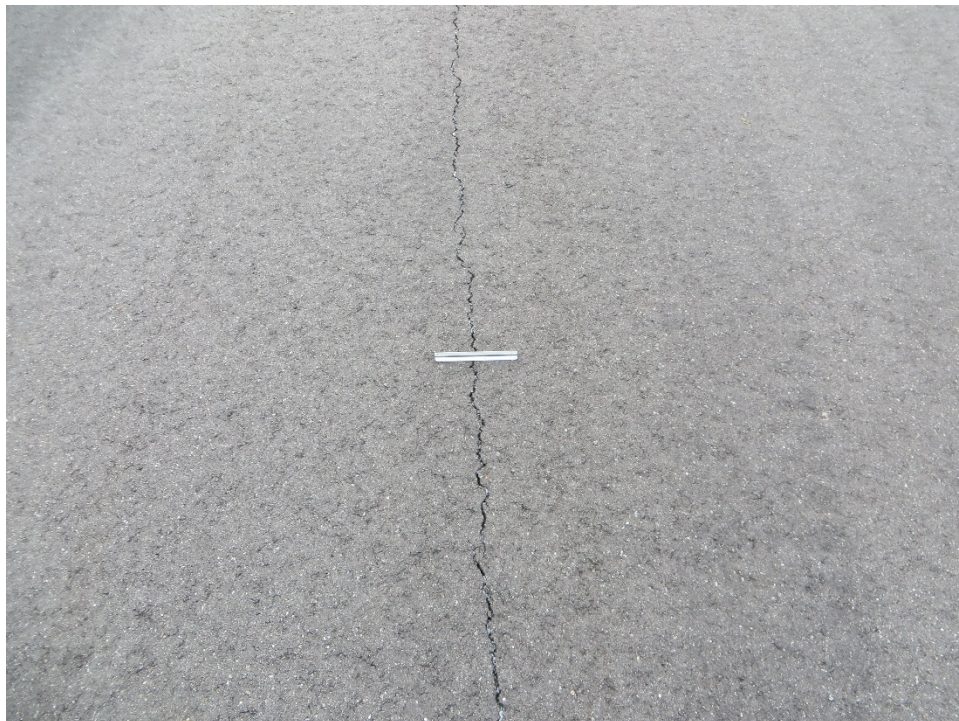
R16RR-02. L&T Cracking (Sample Unit No. 12).
