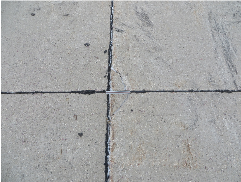
A01RR-03. Corner Spalling (Sample Unit No. 05).
