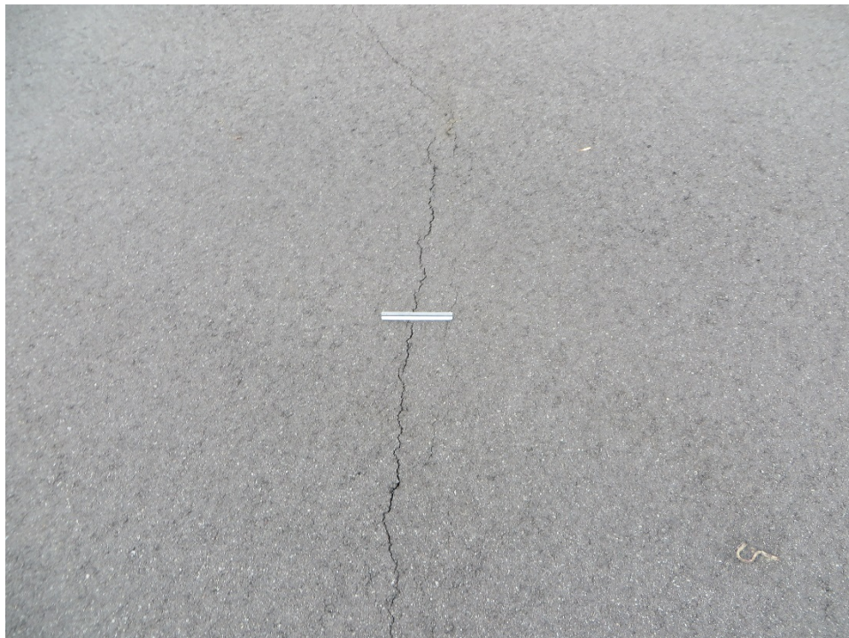
A01RR-01. L&T Cracking (Sample Unit No. 01).
