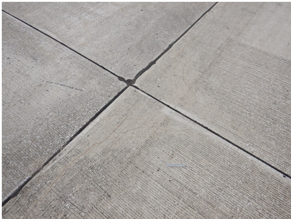
R04SH-01. ASR (Sample Unit No. 34).
