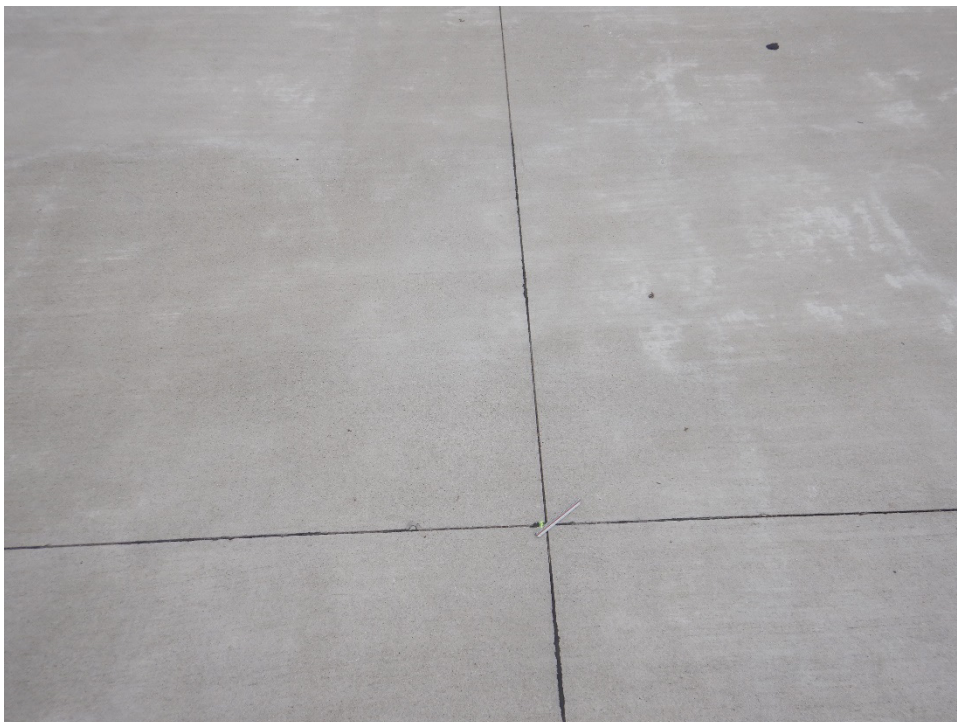
TH01SH-05. Joint Seal Damage (Sample Unit No. 01).
