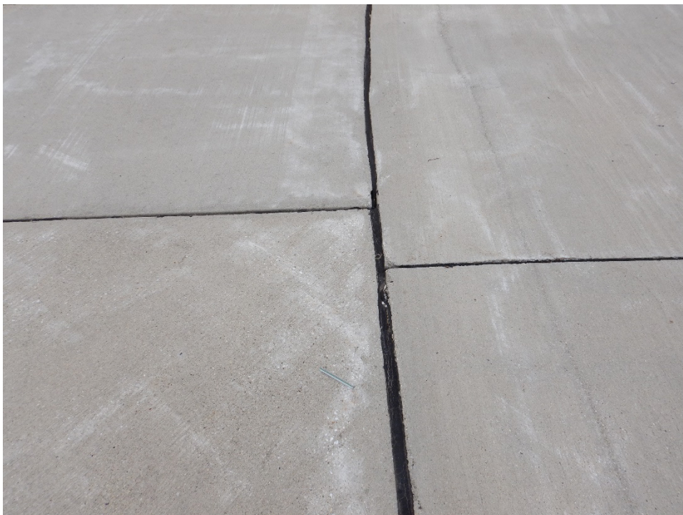
T03SH-01. Joint Seal Damage (Sample Unit No. 16).
