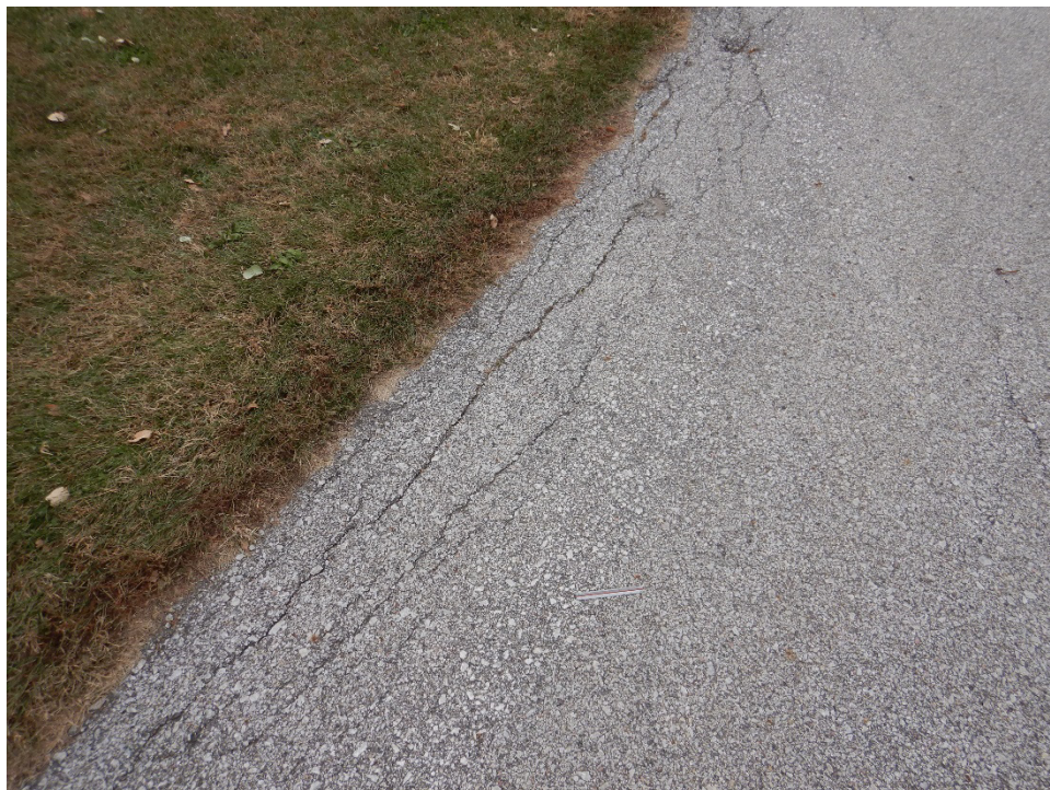
TH01SH-04. Alligator Cracking (Sample Unit No. 01).
