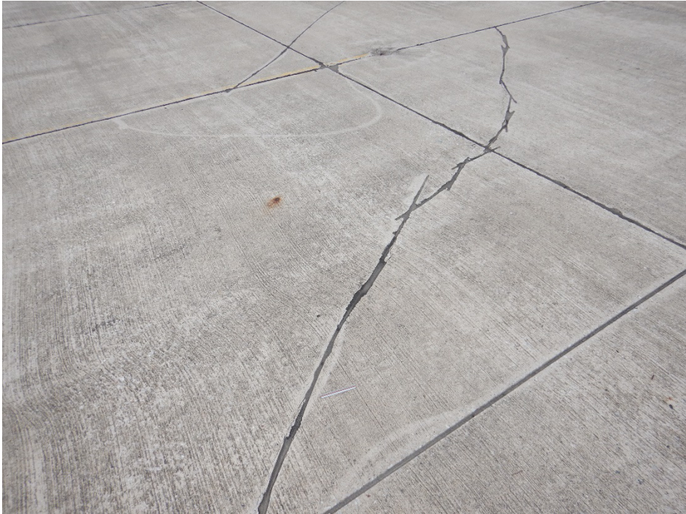
A02SH-01. LTD Cracking (Sample Unit No. 03).
