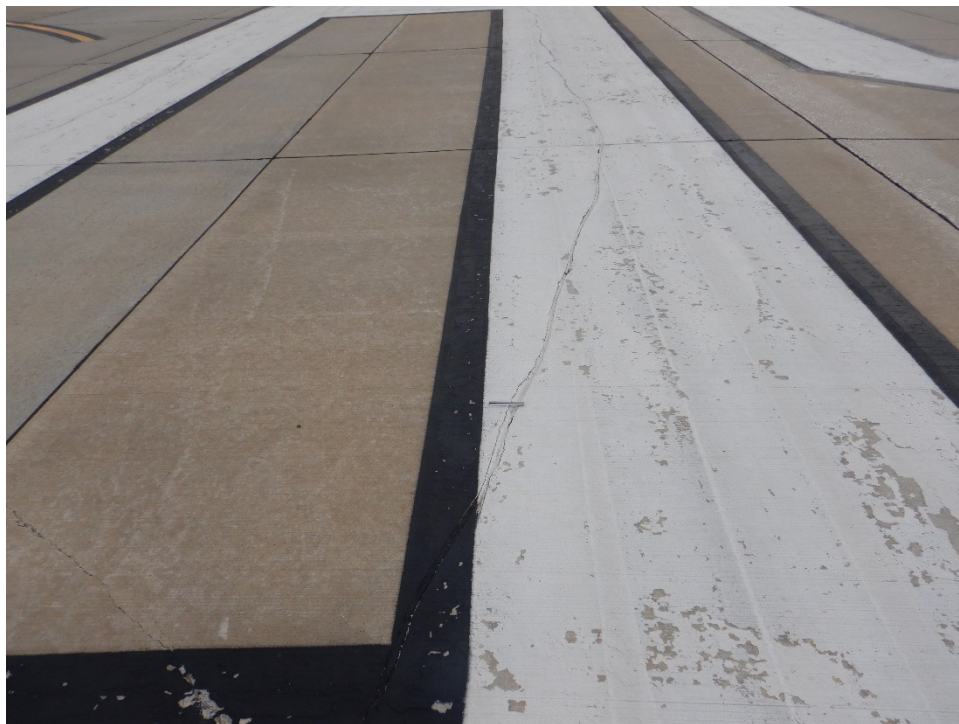
R12SH-04. LTD Cracking (Sample Unit No. 03).
