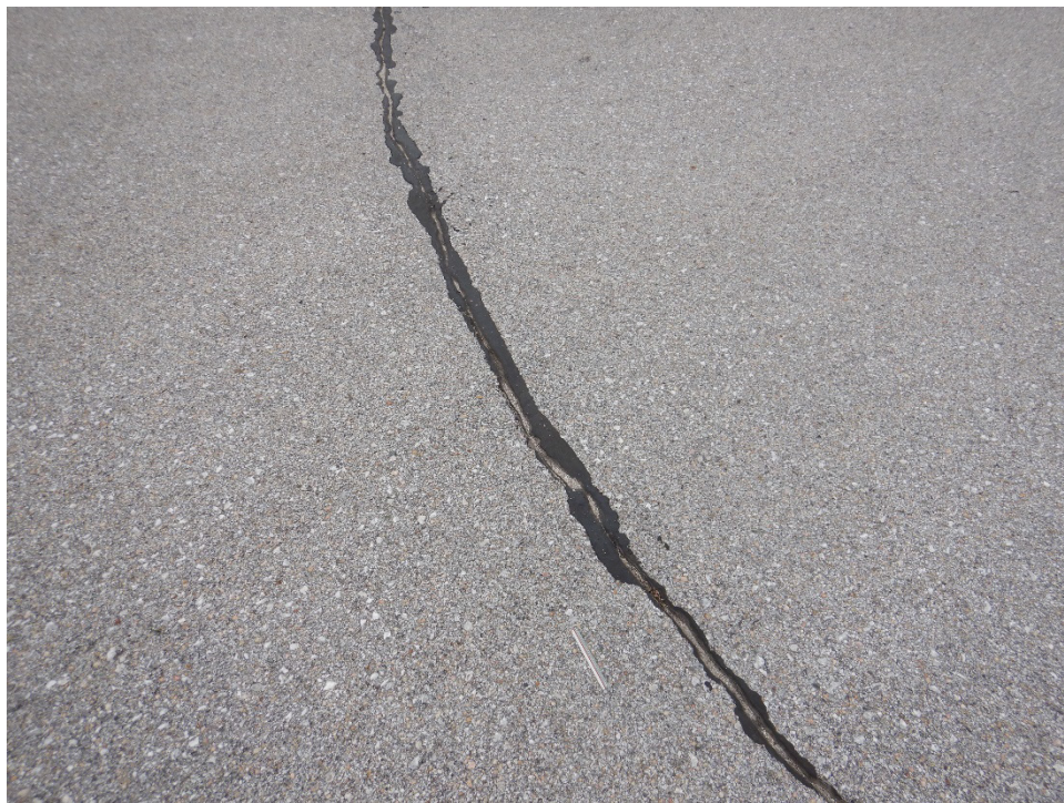
TH01SH-01. L&T Cracking (Sample Unit No. 01).
