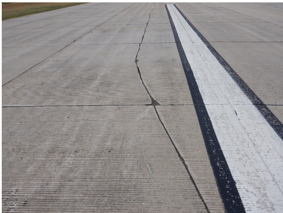
R04SH-02. LTD Cracking (Sample Unit No. 11).
