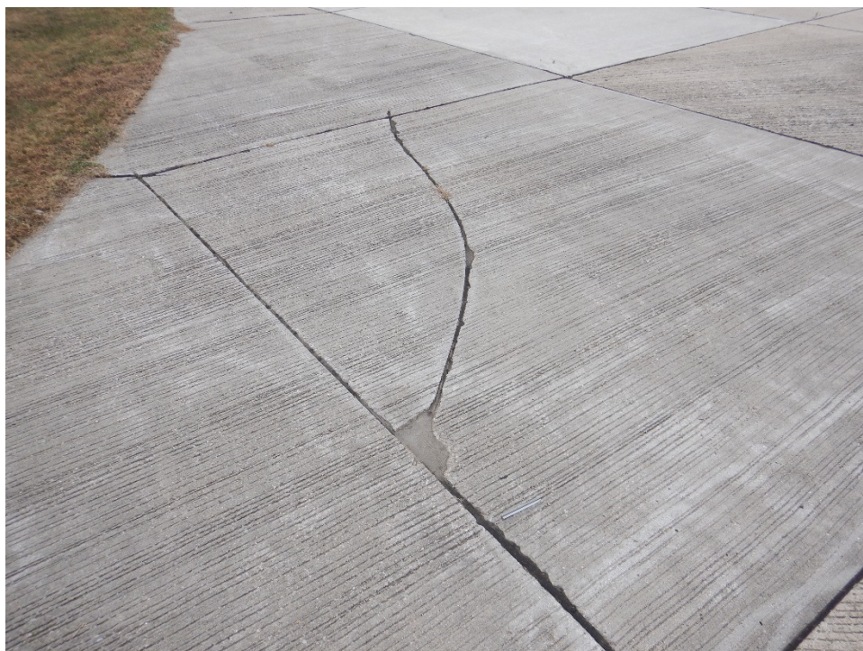
R12SH-03. LTD Cracking (Sample Unit No. 05).
