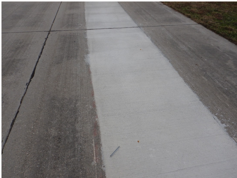
R12SH-01. Large Patching (Sample Unit No. 15).
