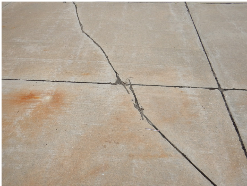
A02SH-03. LTD Cracking (Sample Unit No. 10).
