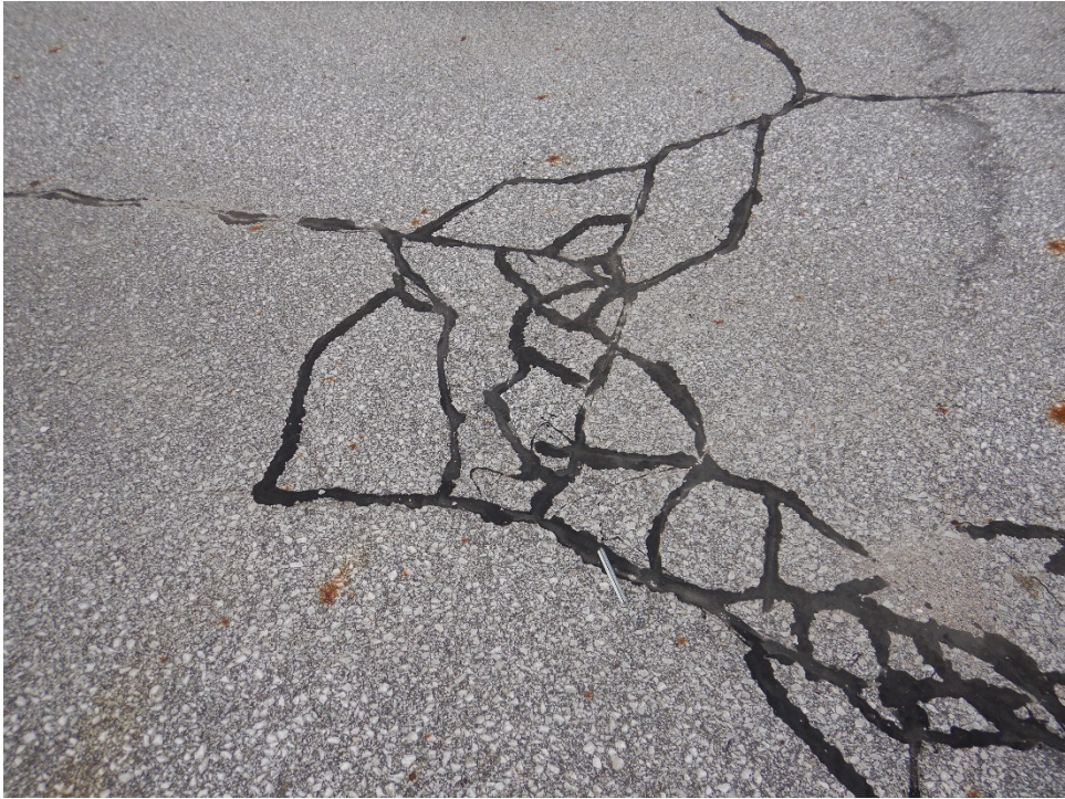
TH01SH-03. Alligator Cracking (Sample Unit No. 01).
