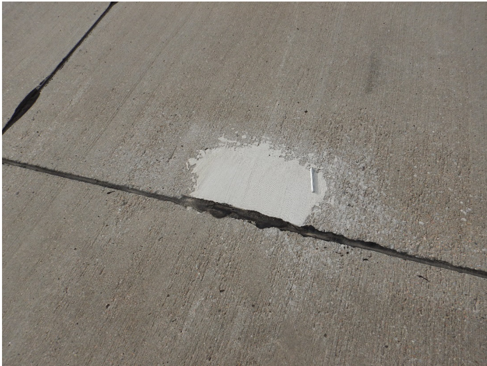
T01SH-01. Small Patching (Sample Unit No. 05).
