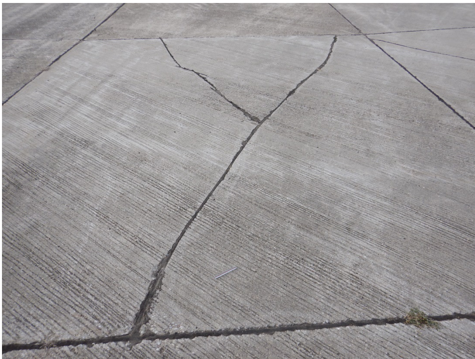
R12SH-02. LTD Cracking (Sample Unit No. 03).
