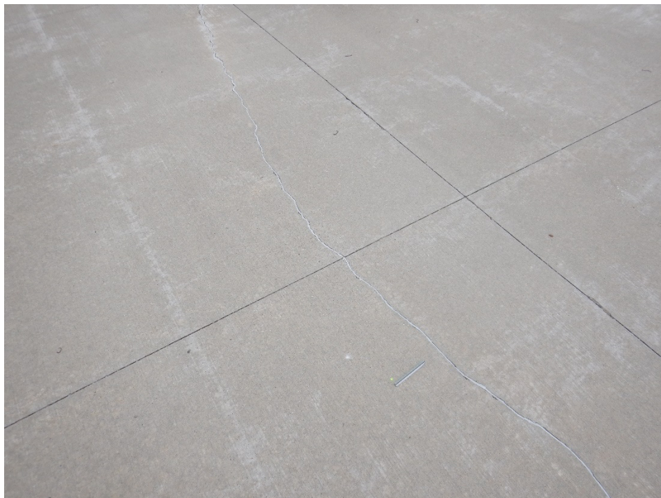
TH01SH-02. LTD Cracking (Sample Unit No. 02).
