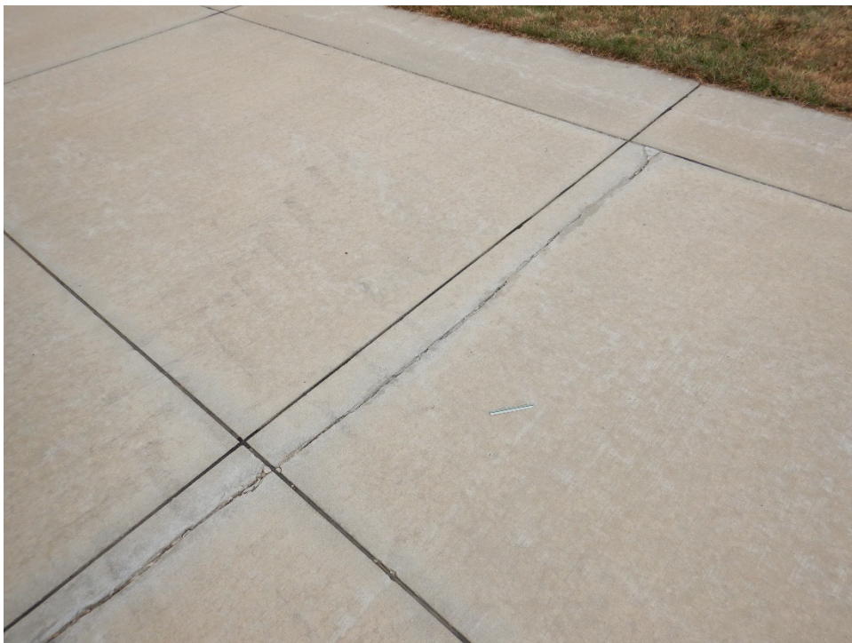
T03SH-02. Joint Spalling (Sample Unit No. 26).
