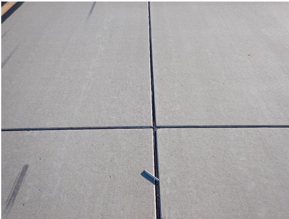
R17SX-01. Faulting (Sample Unit No. 27).
