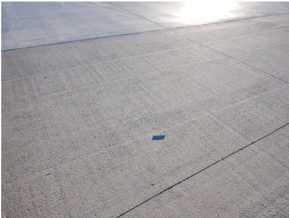
A01SX-03. Shattered Slab (Sample Unit No. 01).
