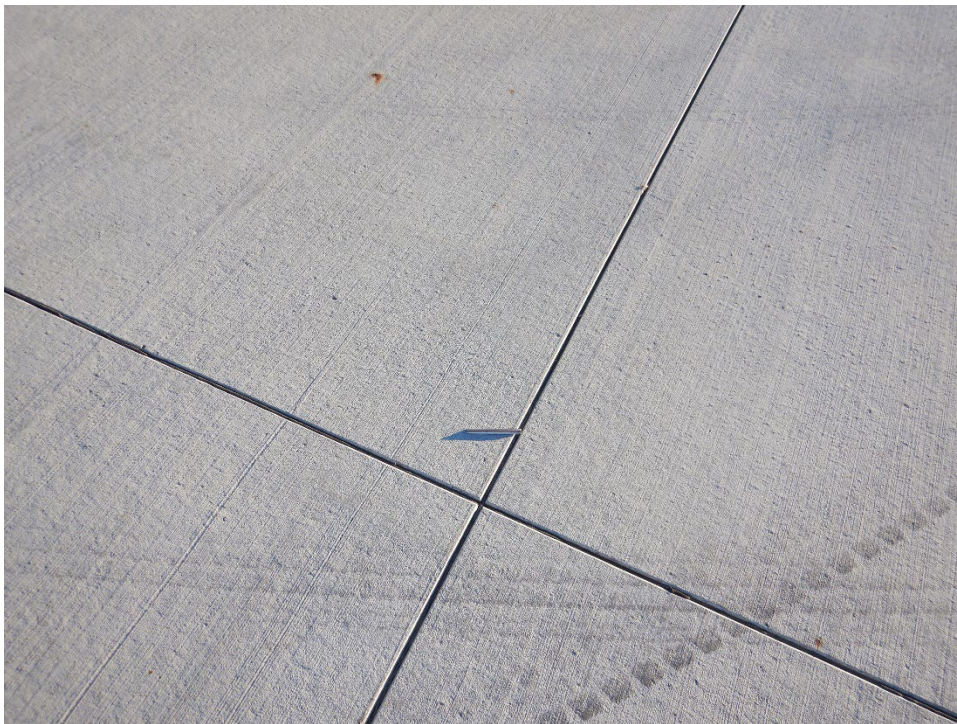
A01SX-02. Joint Seal Damage (Sample Unit No. 05).
