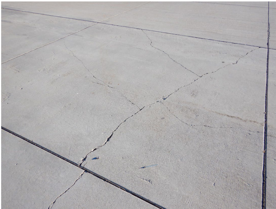
A01SX-01. Shattered Slab (Additional Sample Unit No. 41).
