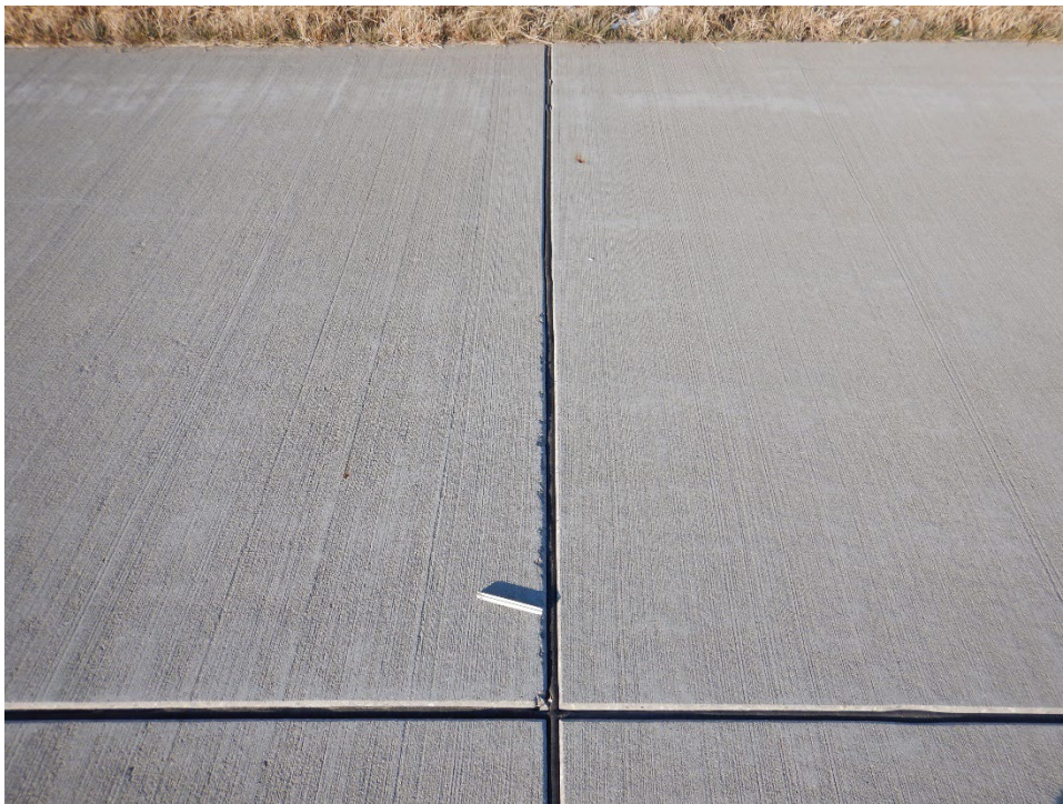
T02SX-04. Joint Seal Damage (Sample Unit No. 01).
