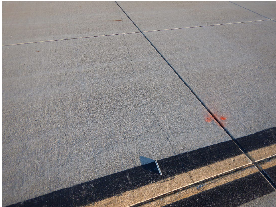
T02SX-01. LTD Cracking (Sample Unit No. 02).
