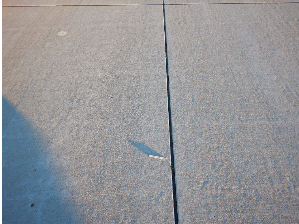
T01SX-01. Joint Seal Damage (Sample Unit No. 06).
