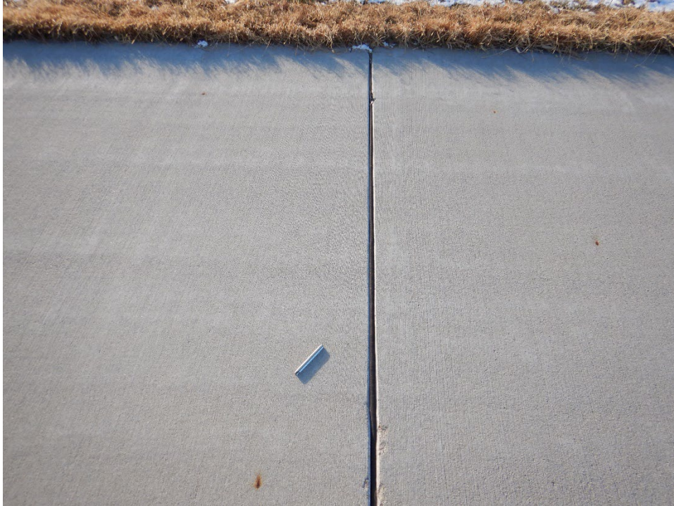
T01SX-02. Joint Seal Damage (Sample Unit No. 02).
