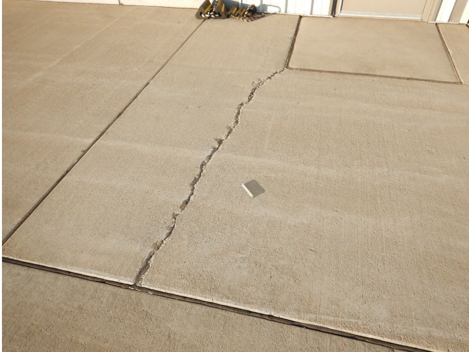
A01SX-01. LTD Cracking (Sample Unit No. 56).
