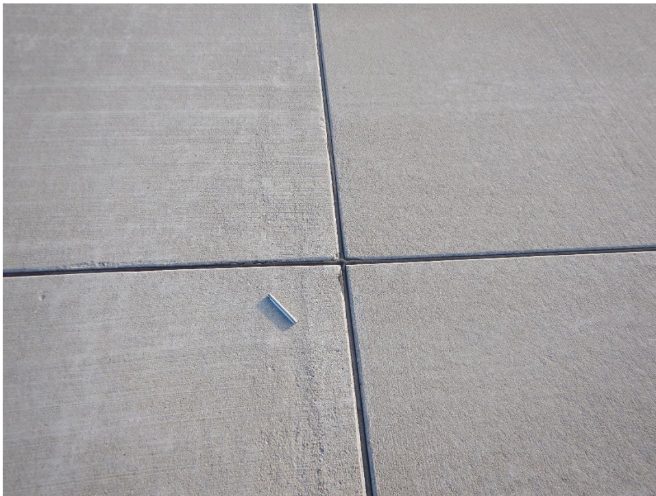
T02SX-03. Joint Seal Damage (Sample Unit No. 01).
