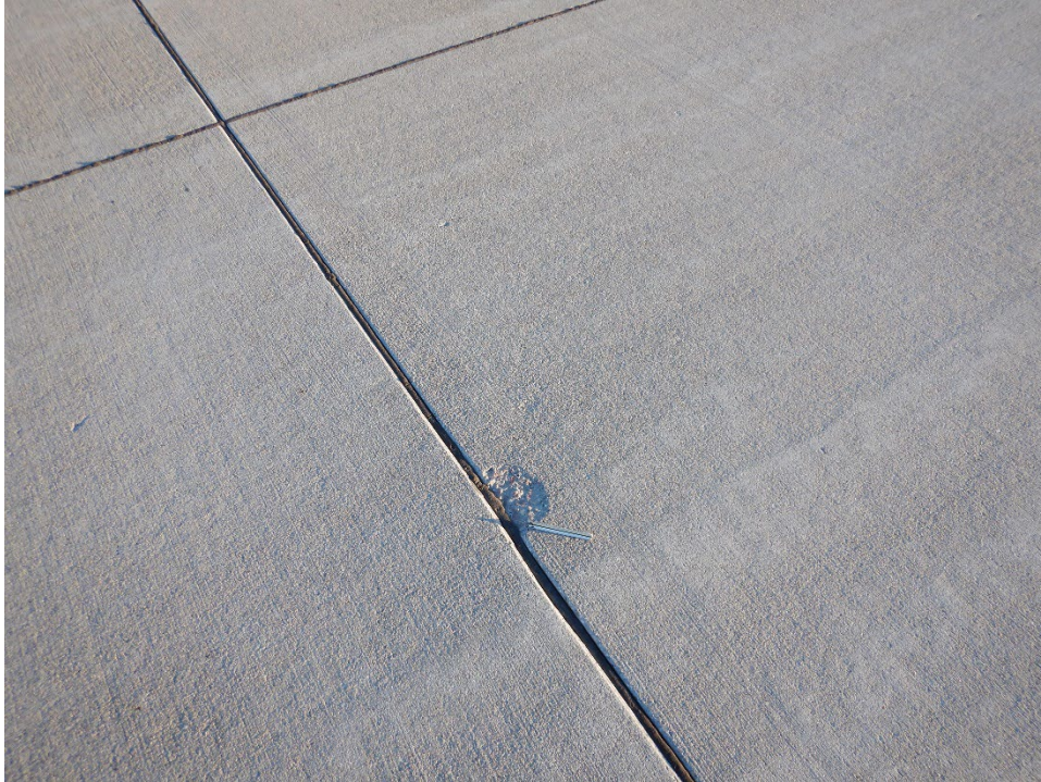
T02SX-02. Joint Spalling (Sample Unit No. 02).
