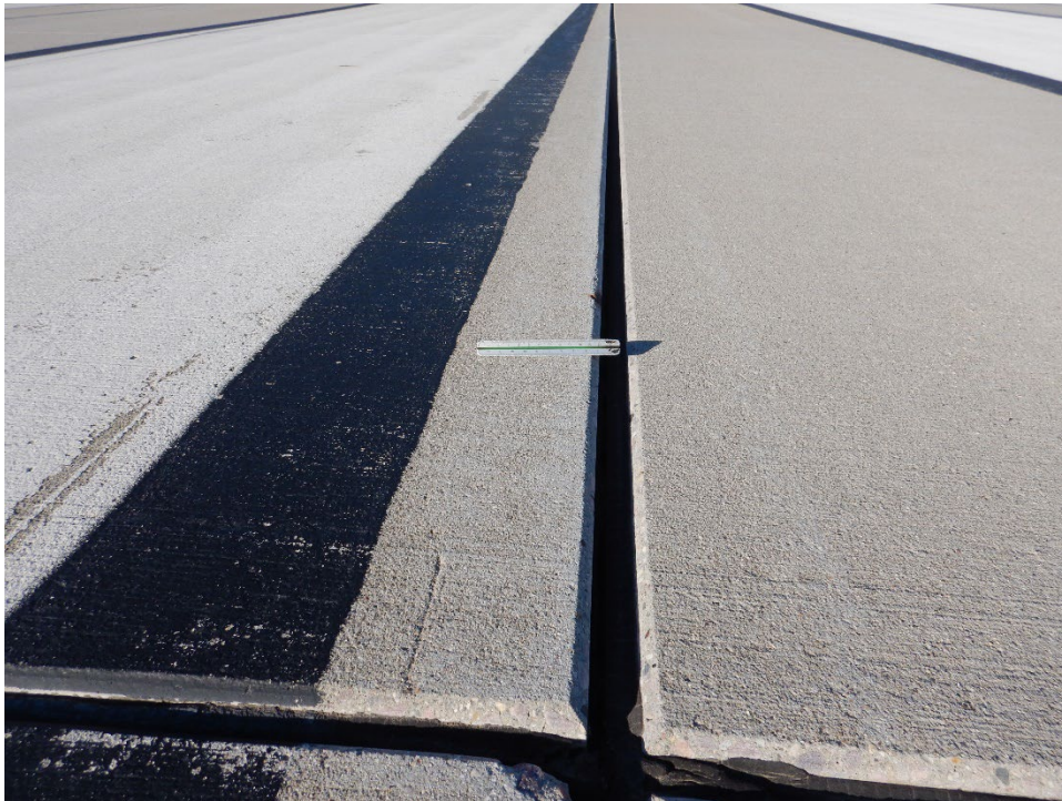
R17SX-02. Faulting (Sample Unit No. 03).
