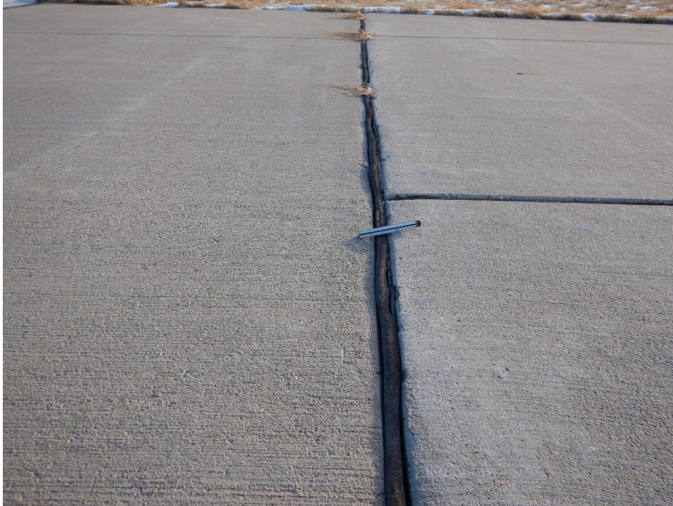
T02SX-03. Faulting (Sample Unit No. 01).
