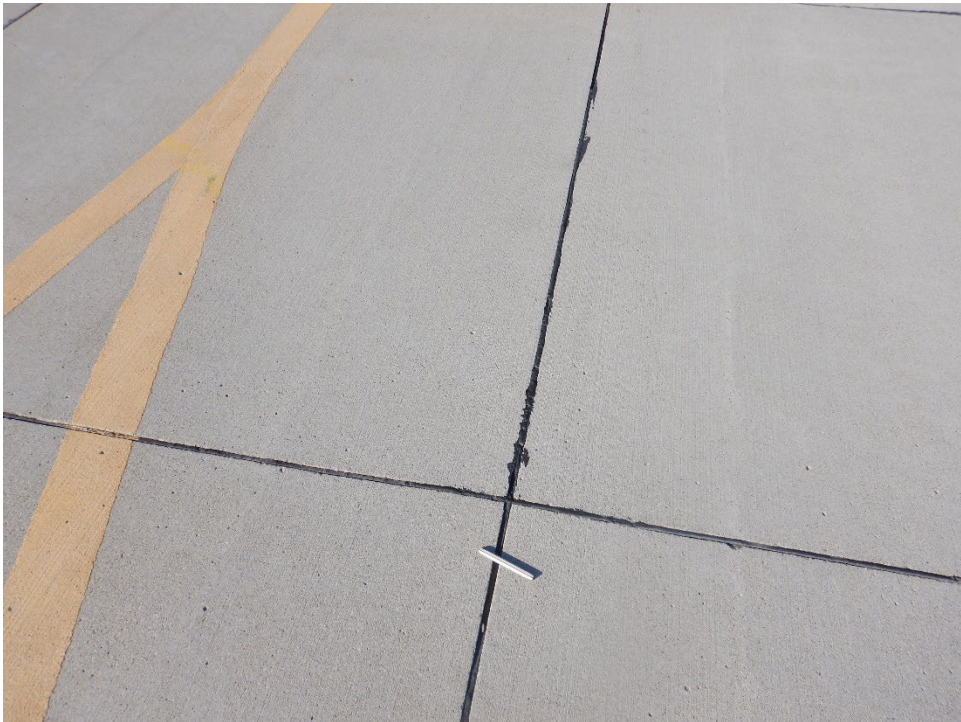
TH01SP-01. Joint Seal Damage (Sample Unit No. 01).
