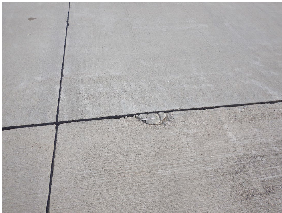
A01SP-03. Joint Spalling (Sample Unit No. 05).
