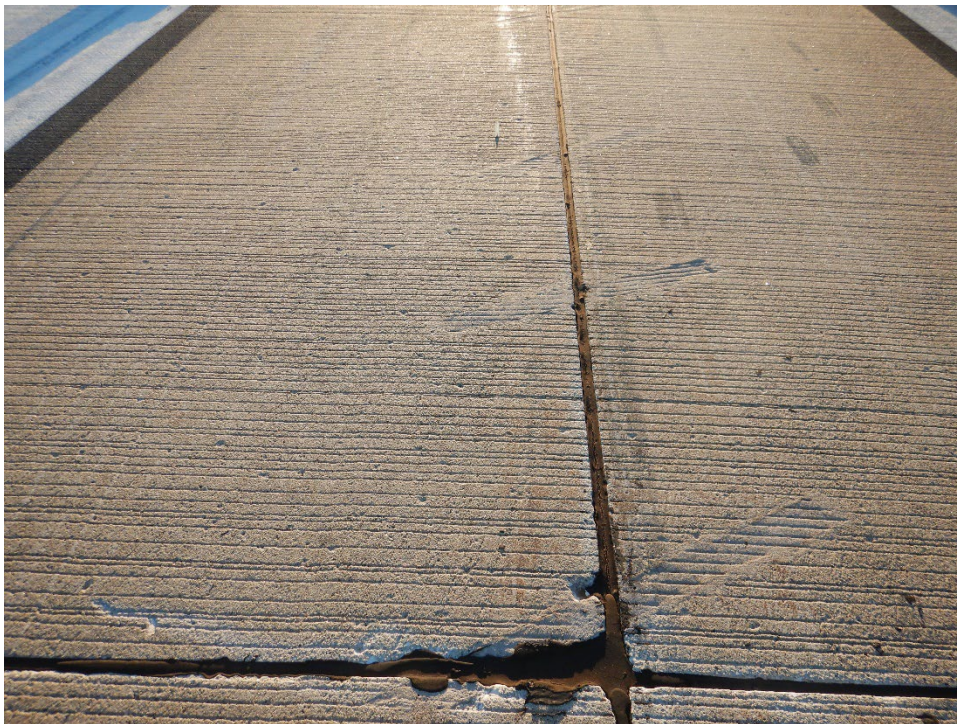
R12SP-01. Small Patching (Sample Unit No. 223).
