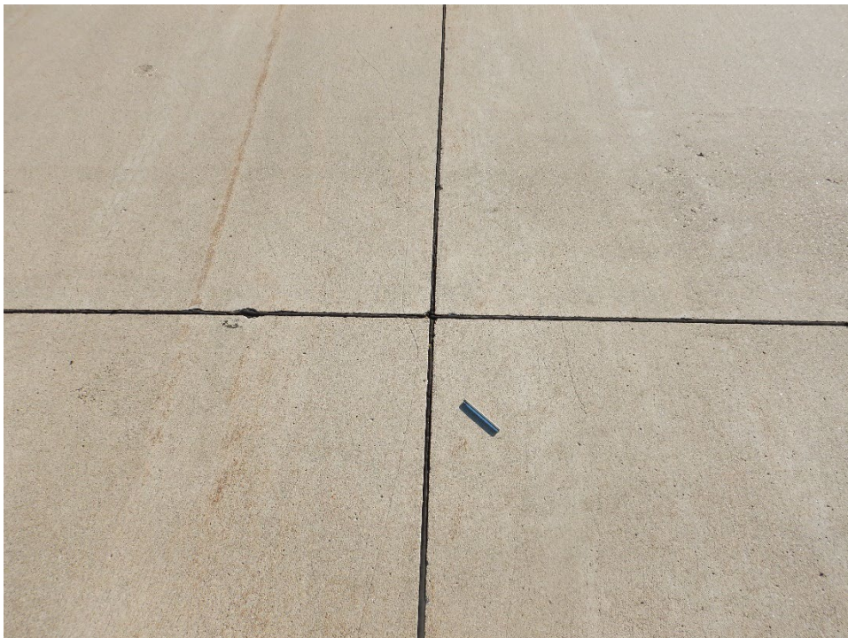
TCSP-03. Joint Seal Damage (Sample Unit No. 03).
