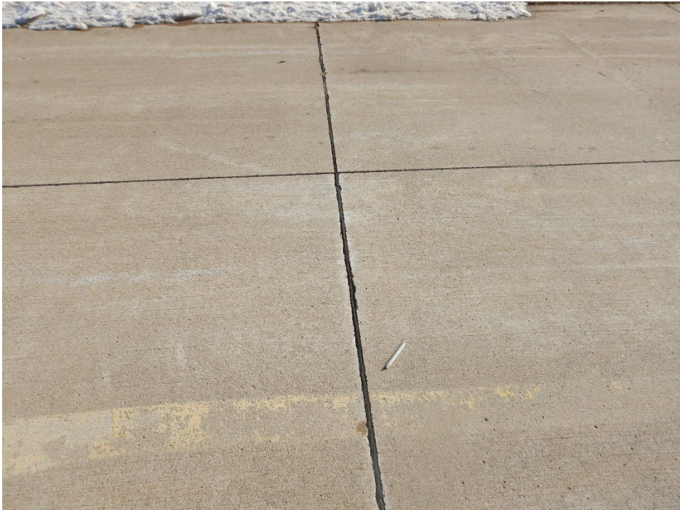
TH01SP-03. Joint Seal Damage (Sample Unit No. 02).
