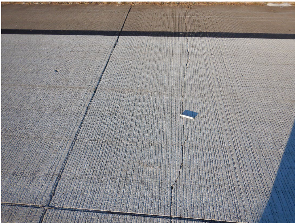
R18SP-01. LTD Cracking (Additional Sample Unit No. 22).
