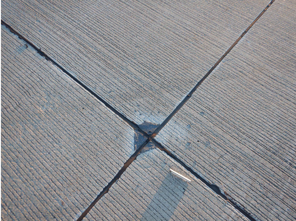
R12SP-01. Small Patching (Sample Unit No. 43).
