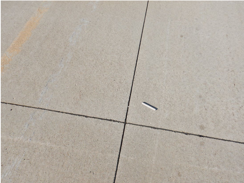
TH01SP-02. Joint Seal Damage (Sample Unit No. 02).
