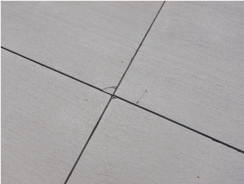
A01SP-01. Corner Spalling (Sample Unit No. 05).
