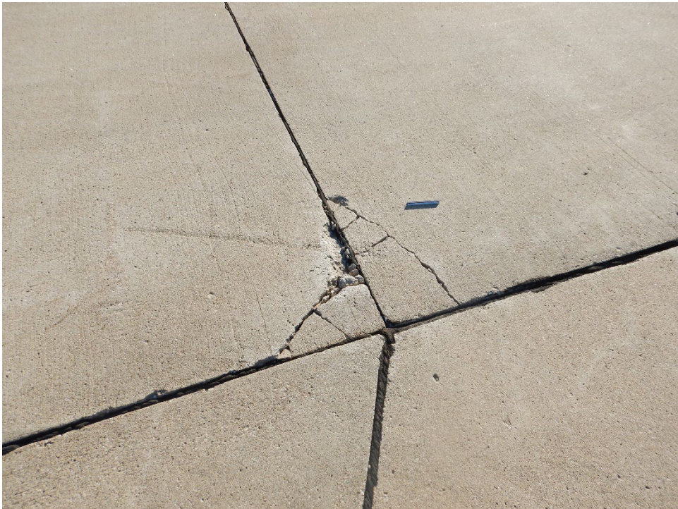
TASP-01. Corner Spalling (Sample Unit No. 02).
