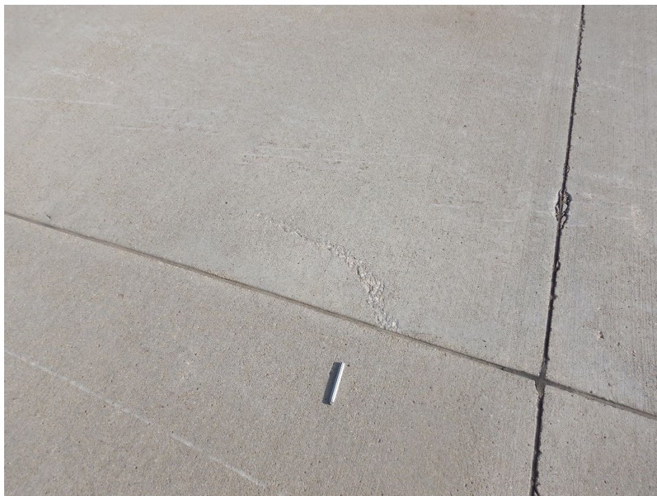
A01SP-06. Joint Spalling (Sample Unit No. 02).
