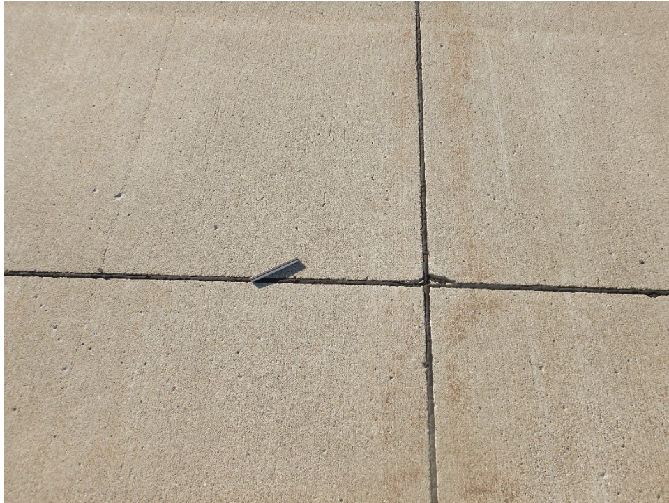
TASP-01. Joint Seal Damage (Sample Unit No. 16).
