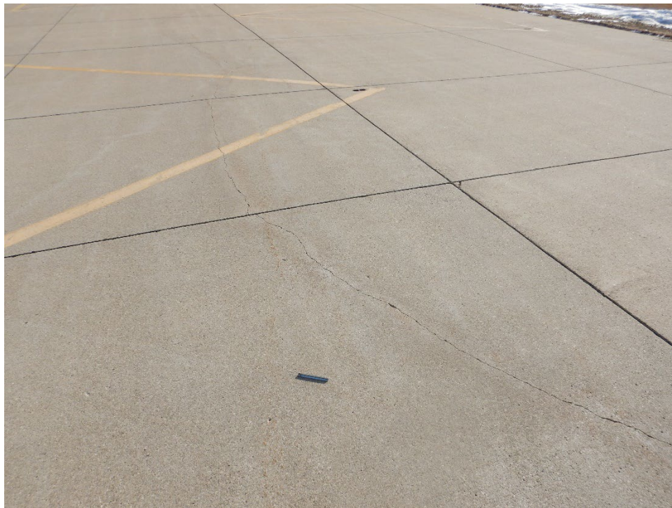
A01SP-04. LTD Cracking (Sample Unit No. 04).
