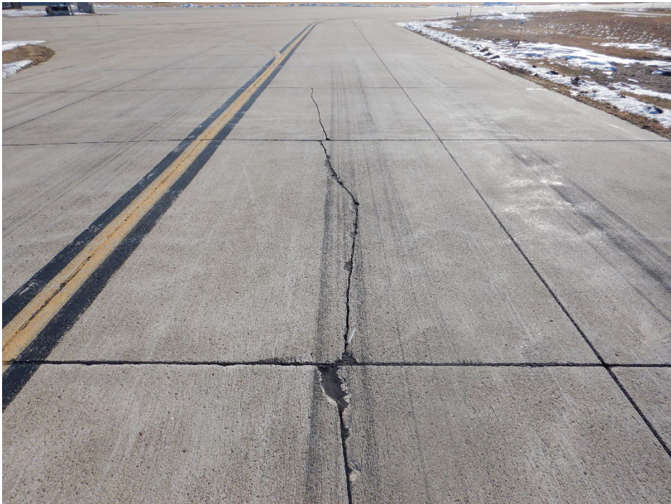
TCSP-01. LTD Cracking (Sample Unit No. 04).
