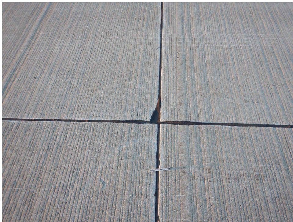
R12SP-01. Corner Spalling (Sample Unit No. 23).
