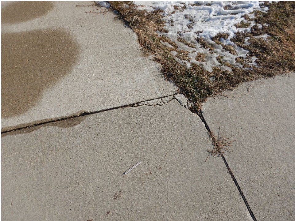
TH01SP-02. Corner Spalling (Sample Unit No. 04).
