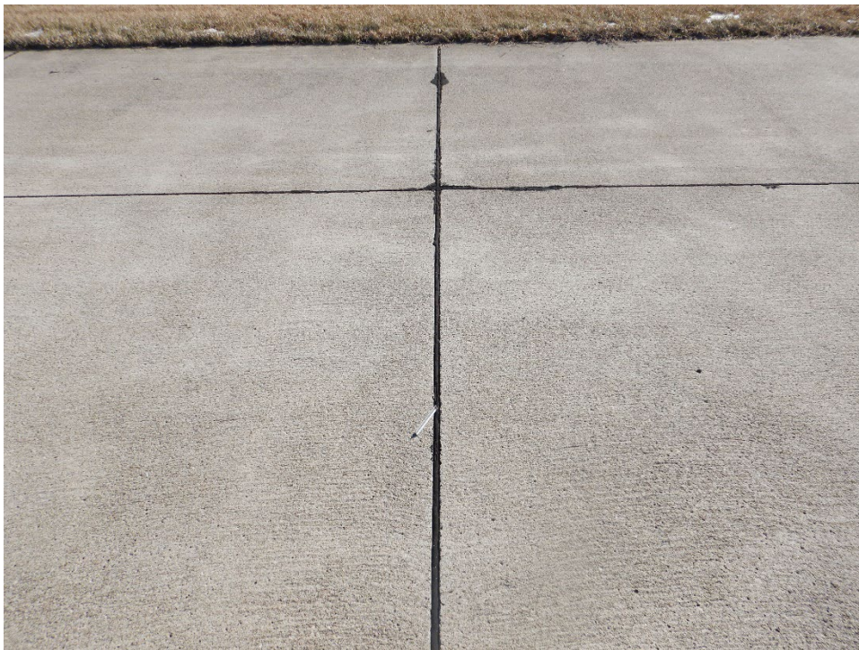
TC2SP-01. Joint Seal Damage (Sample Unit No. 03).
