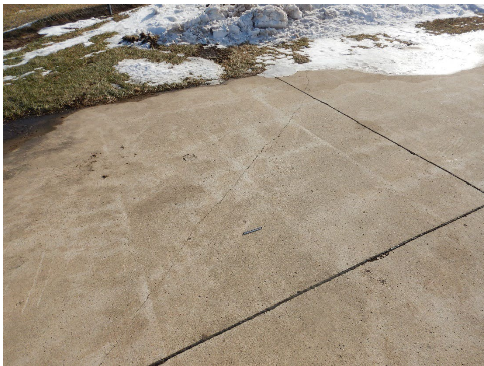
A01SP-05. LTD Cracking (Sample Unit No. 05).
