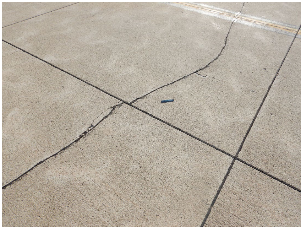
TCSP-02. LTD Cracking (Sample Unit No. 05).
