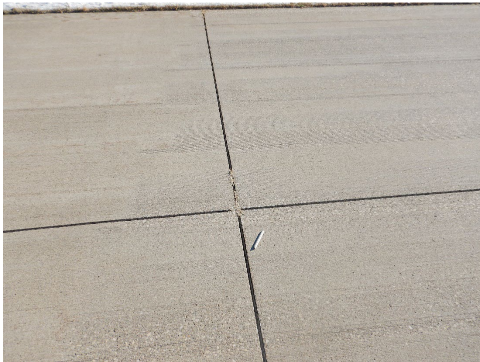
TESP-01. Joint Seal Damage (Sample Unit No. 02).
