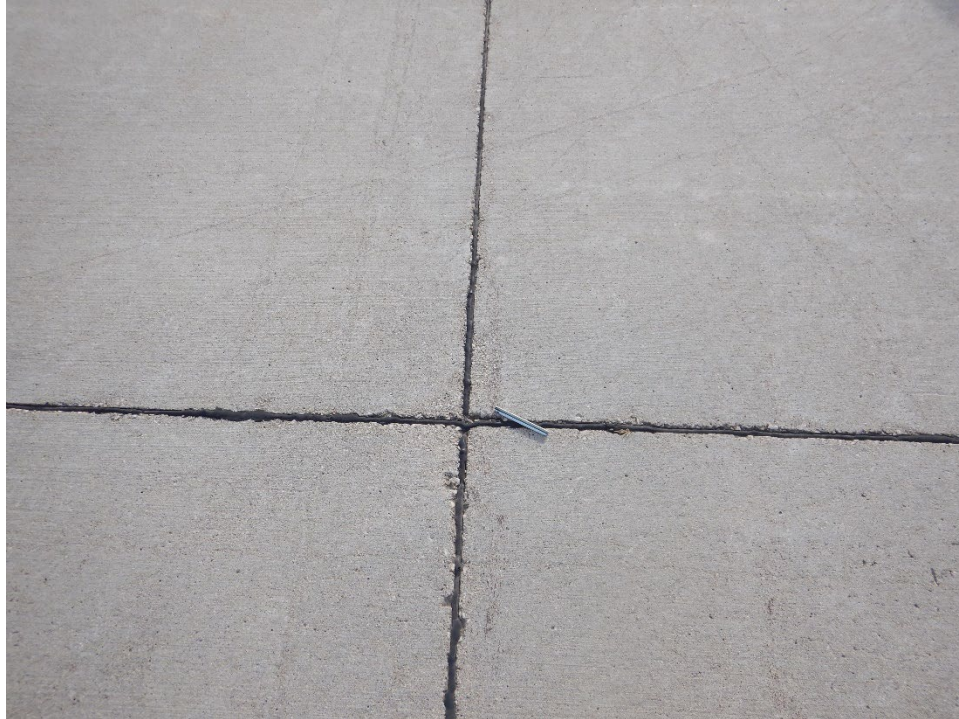
TH01SP-04. Joint Seal Damage (Sample Unit No. 02).
