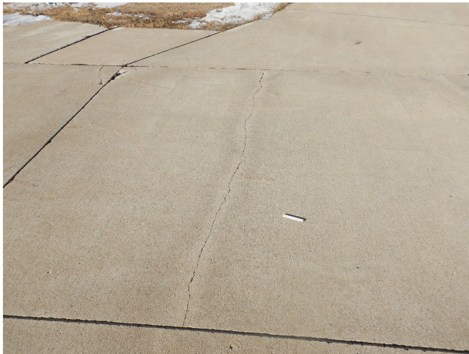
TASP-01. LTD Cracking (Additional Sample Unit No. 01).
