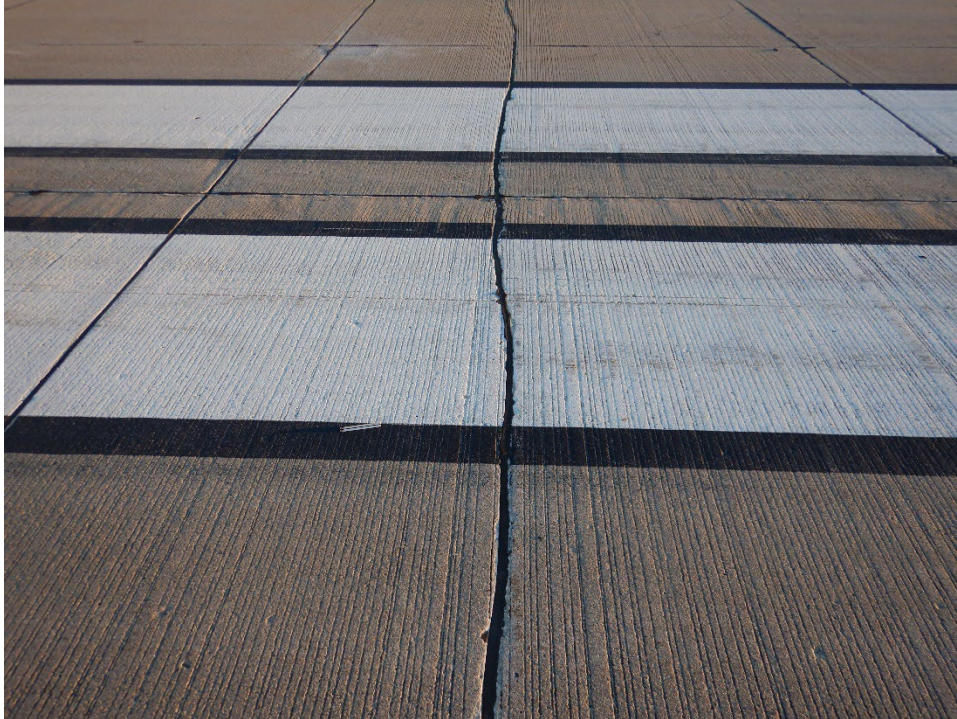
R12SP-01. LTD Cracking (Sample Unit No. 83).
