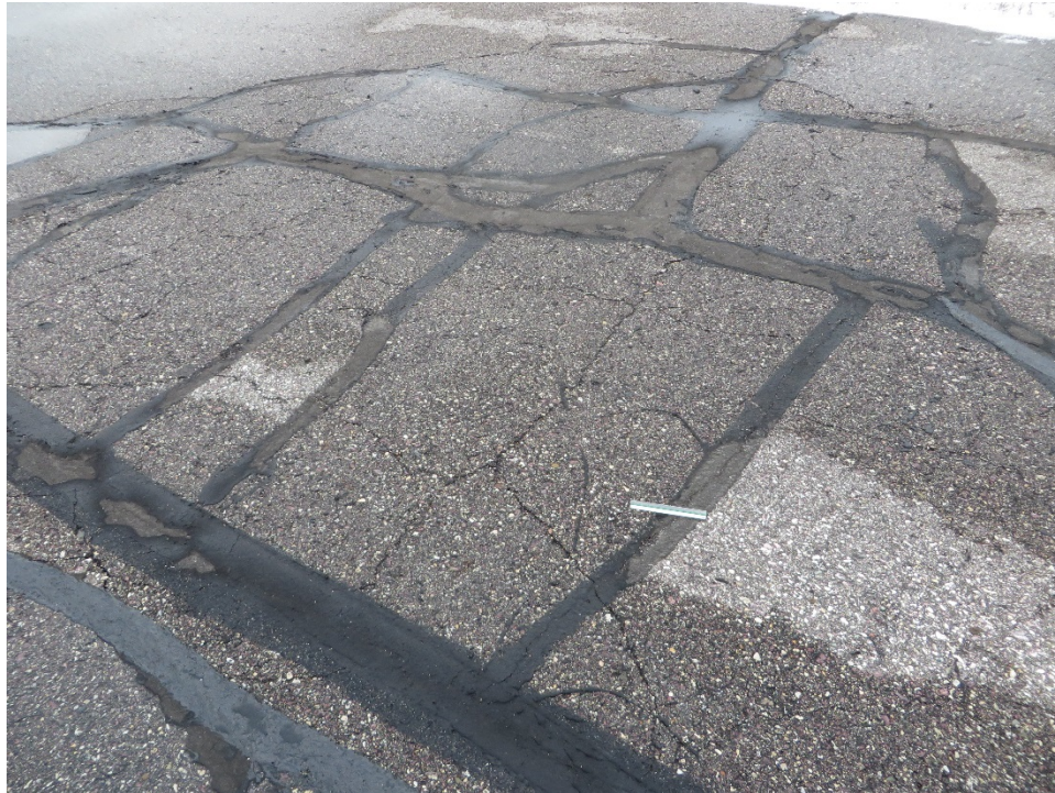
R165I-01. Alligator Cracking (Sample Unit No. 25).
