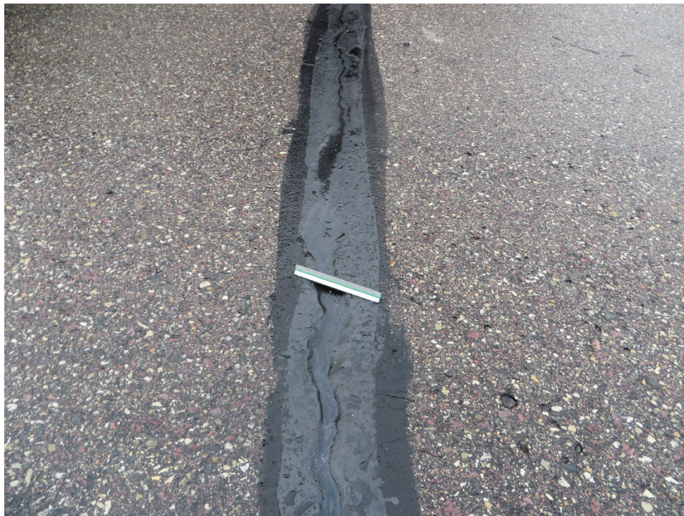
R165I-01. L&T Cracking (Sample Unit No. 02).
