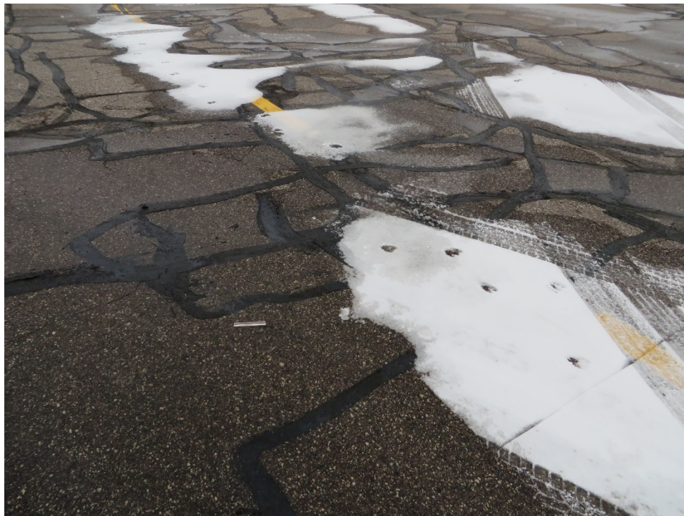
T015I-01. Block Cracking (Sample Unit No. 02).
