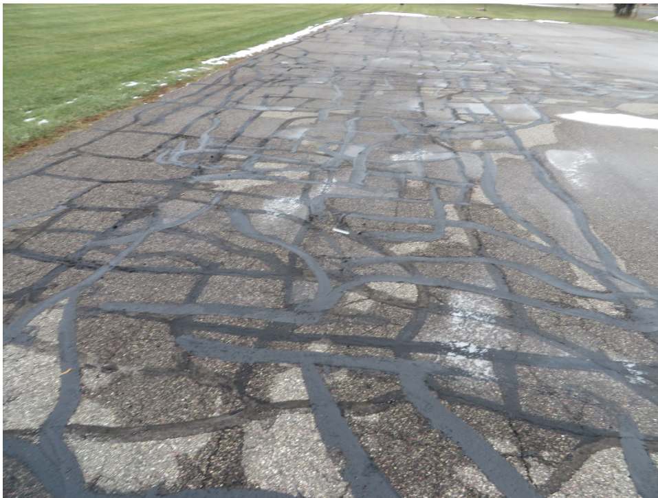
A015I-01. Alligator Cracking (Sample Unit No. 02).
