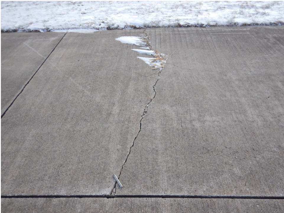
T02SL-01. LTD Cracking (Sample Unit No. 08).
