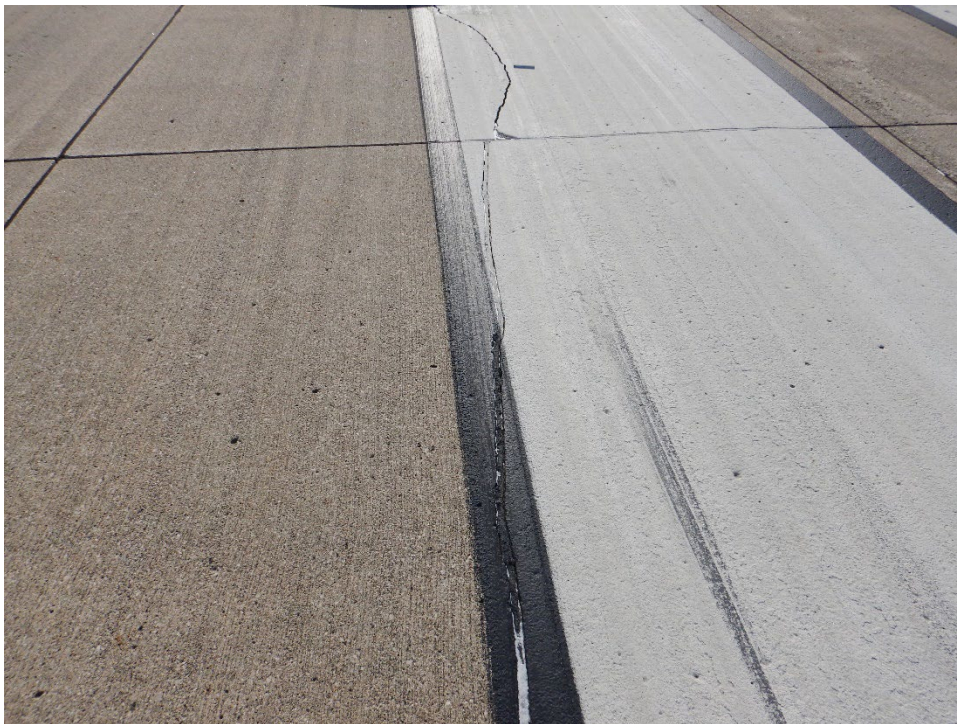
R17SL-01. LTD Cracking (Sample Unit No. 03).
