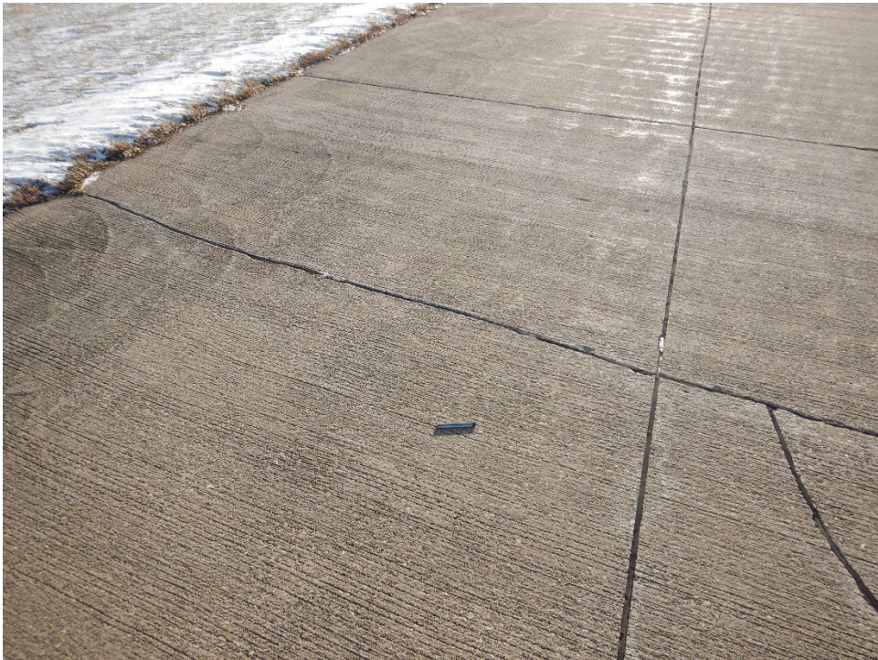
T01SL-01. LTD Cracking (Sample Unit No. 05).
