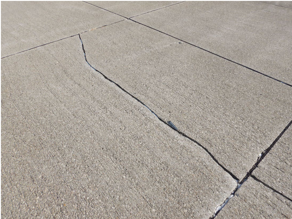
T01SL-02. LTD Cracking (Sample Unit No. 07).
