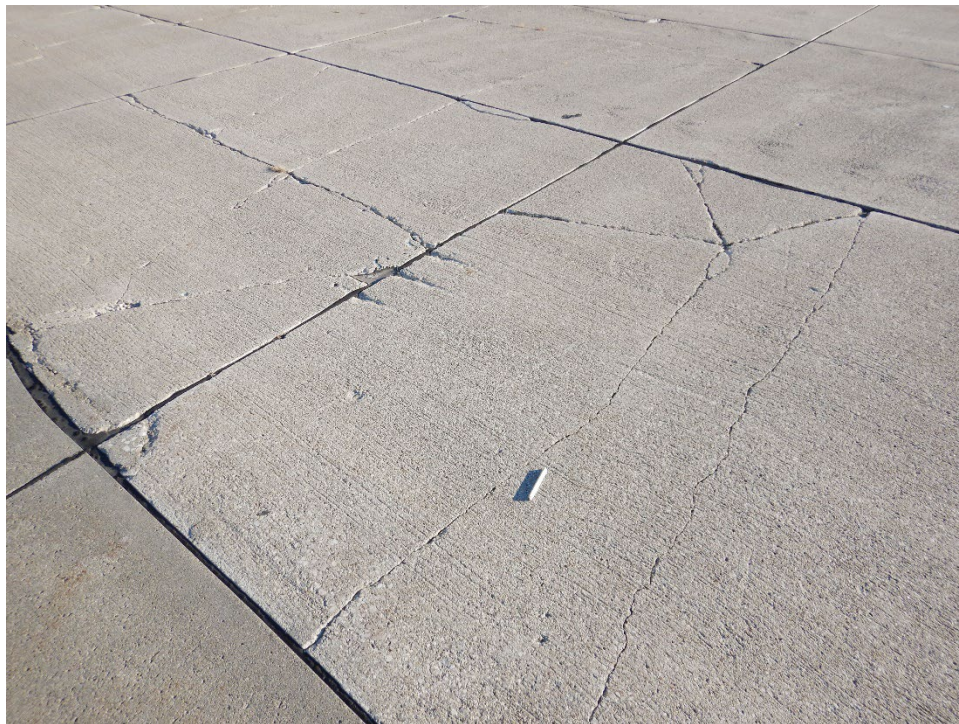
A01SL-02. Shattered Slab (Sample Unit No. 07).
