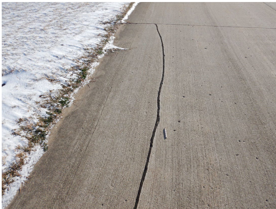
R17SL-02. LTD Cracking (Sample Unit No. 06).
