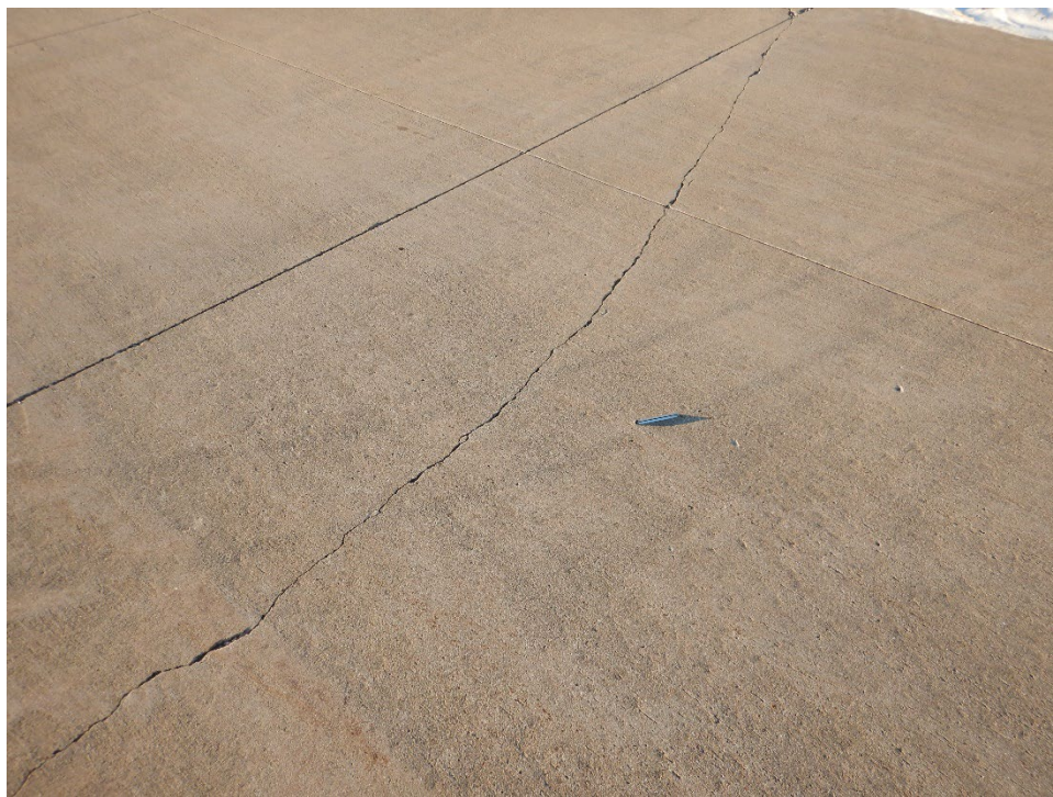
TH01SL-02. LTD Cracking (Sample Unit No. 01).
