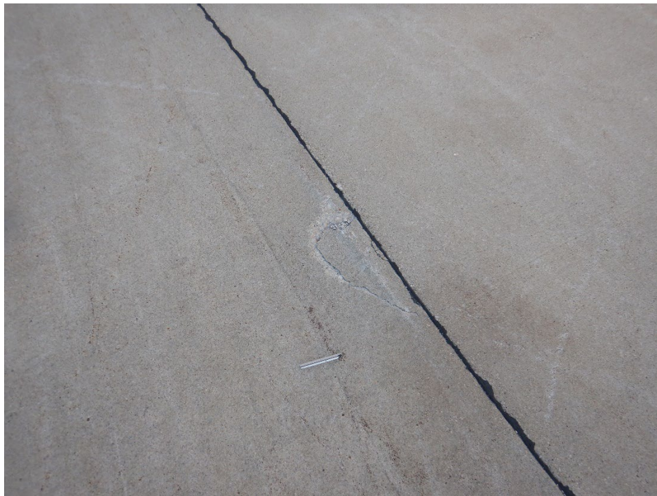
TH01SL-03. Joint Spalling (Sample Unit No. 01).
