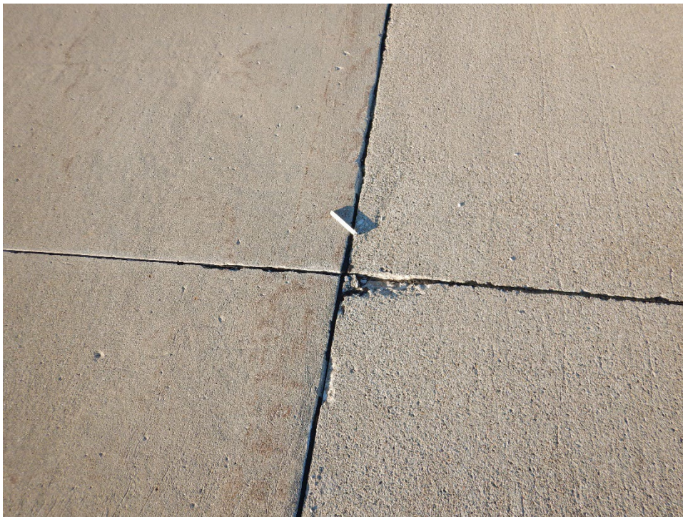
TH01SL-01. Joint Spalling (Sample Unit No. 10).
