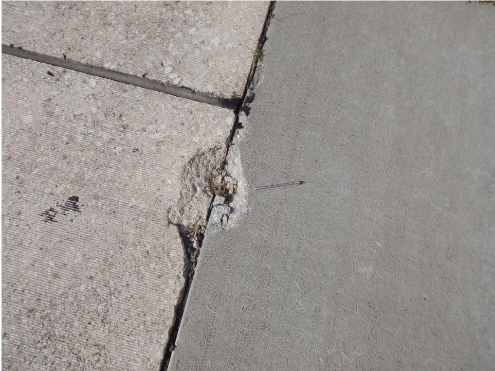
T01TI-02. Joint Spalling (Sample Unit No. 01).
