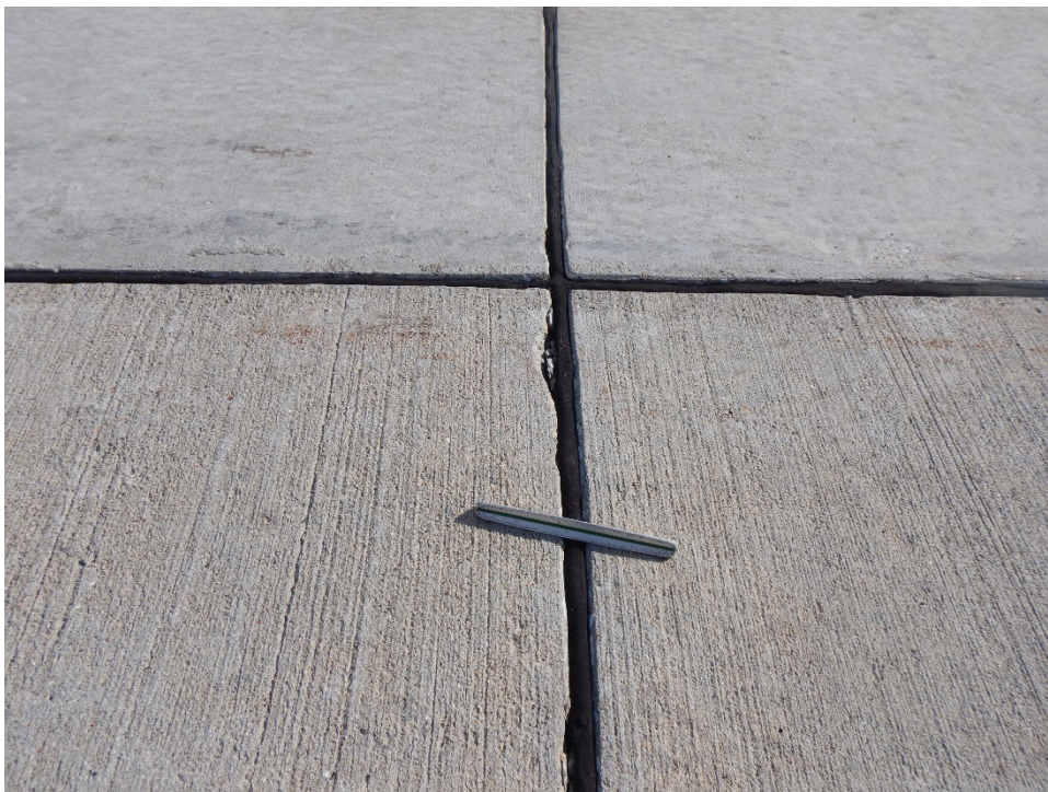
T01TI-02. Joint Seal Damage (Sample Unit No. 03).
