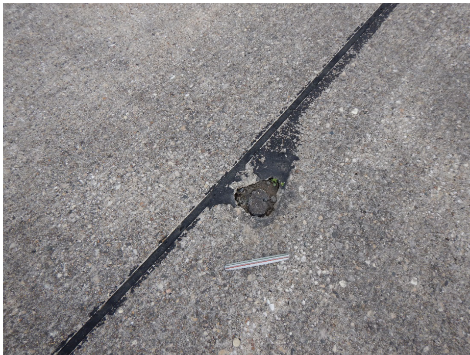
R11TI-01. Joint Spalling (Sample Unit No. 35).
