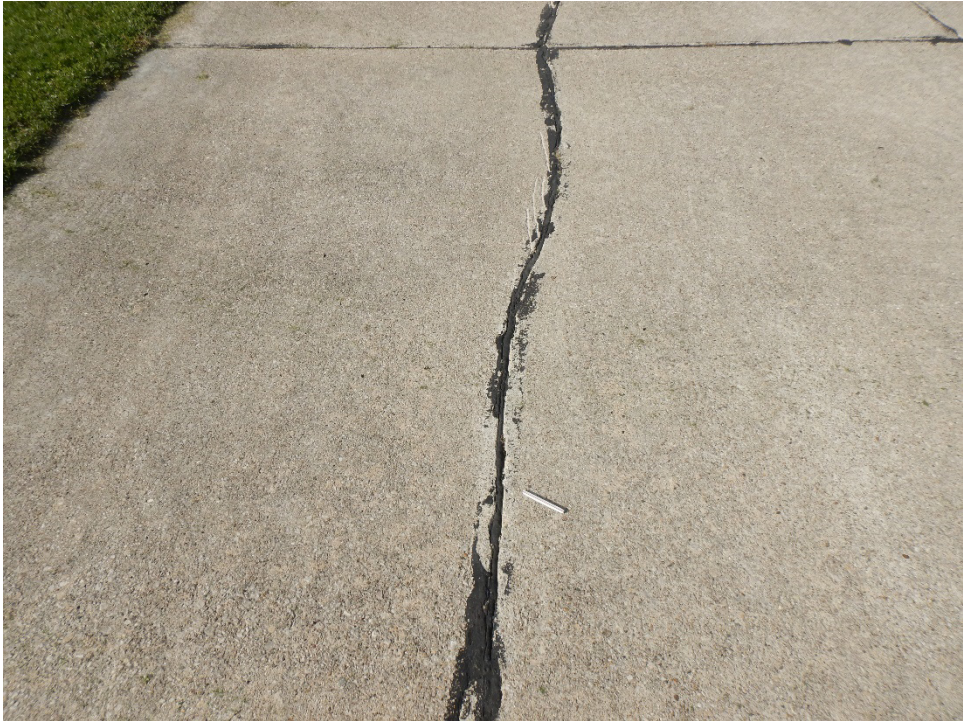
A01TI-01. LTD Cracking (Sample Unit No. 03).
