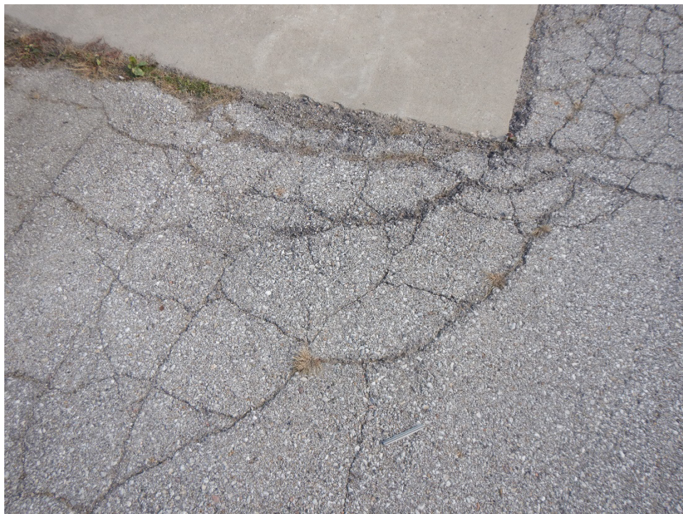
TH01TI-01. Alligator Cracking (Sample Unit No. 02).
