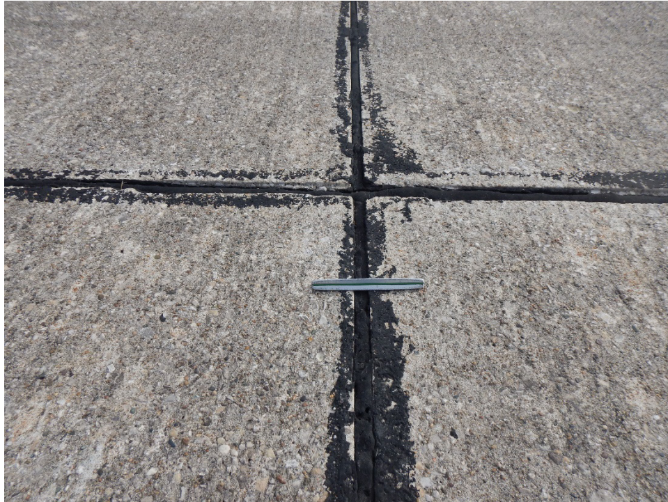
R11TI-01. Joint Seal Damage (Sample Unit No. 15).
