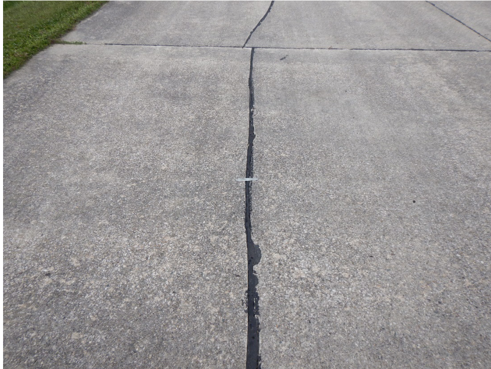
R11TI-01. LTD Cracking (Sample Unit No. 45).
