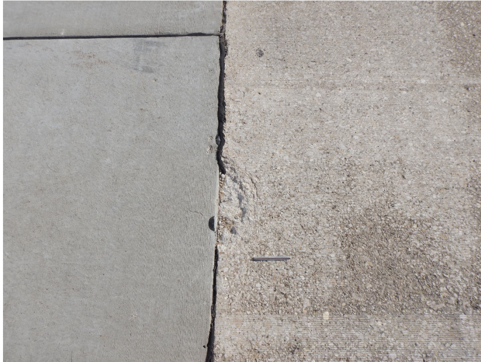
T01TI-03. Joint Spalling (Sample Unit No. 01).
