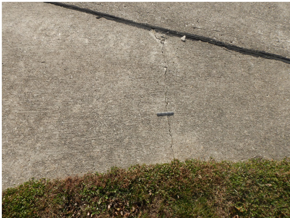
T01TI-03. LTD Cracking (Sample Unit No. 01).
