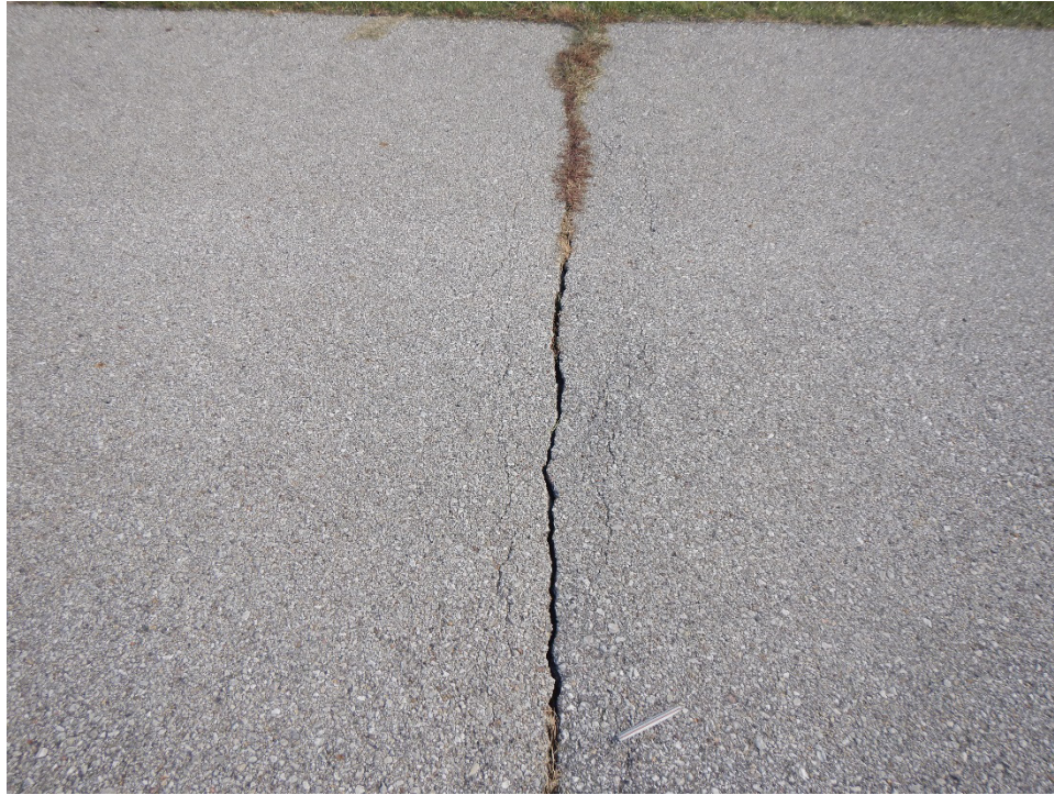
TH01TI-01. L&T Cracking (Sample Unit No. 01).
