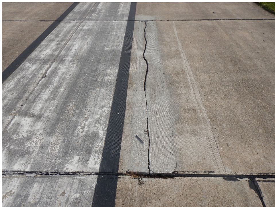
R11TI-01. Large Patching (Sample Unit No. 05).
