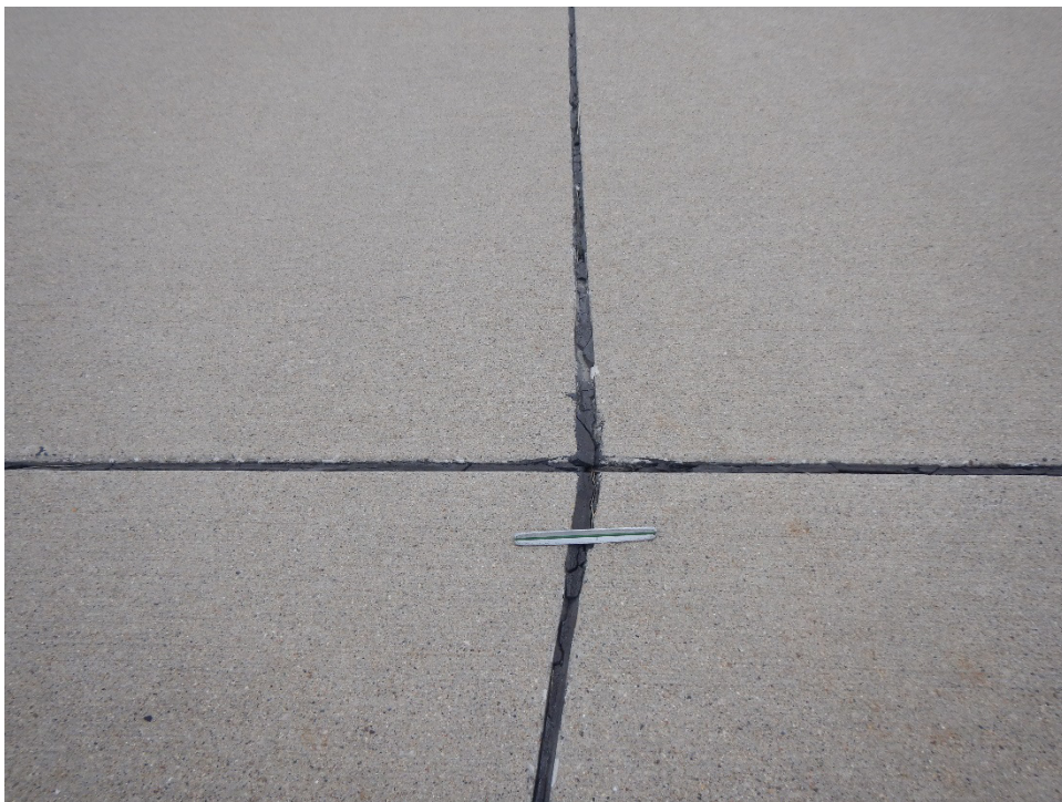
T03VI-01. Joint Seal Damage (Sample Unit No. 02).
