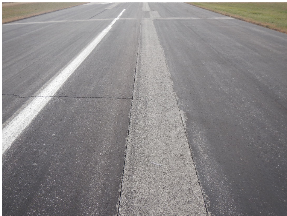
R16VI-02. Patching (Sample Unit No. 13).
