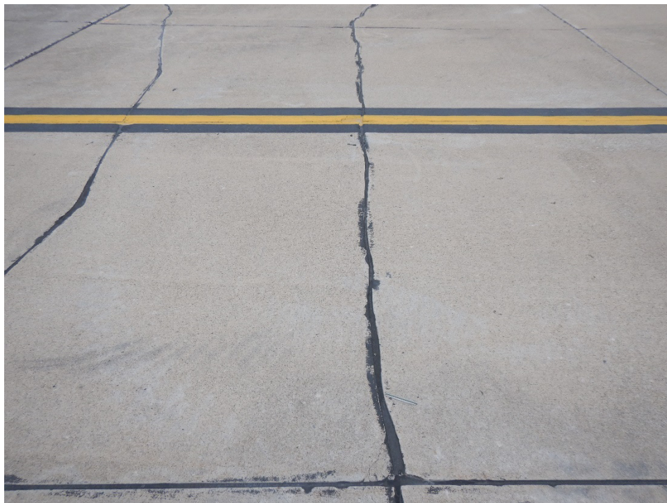
T02VI-01. LTD Cracking (Sample Unit No. 08).
