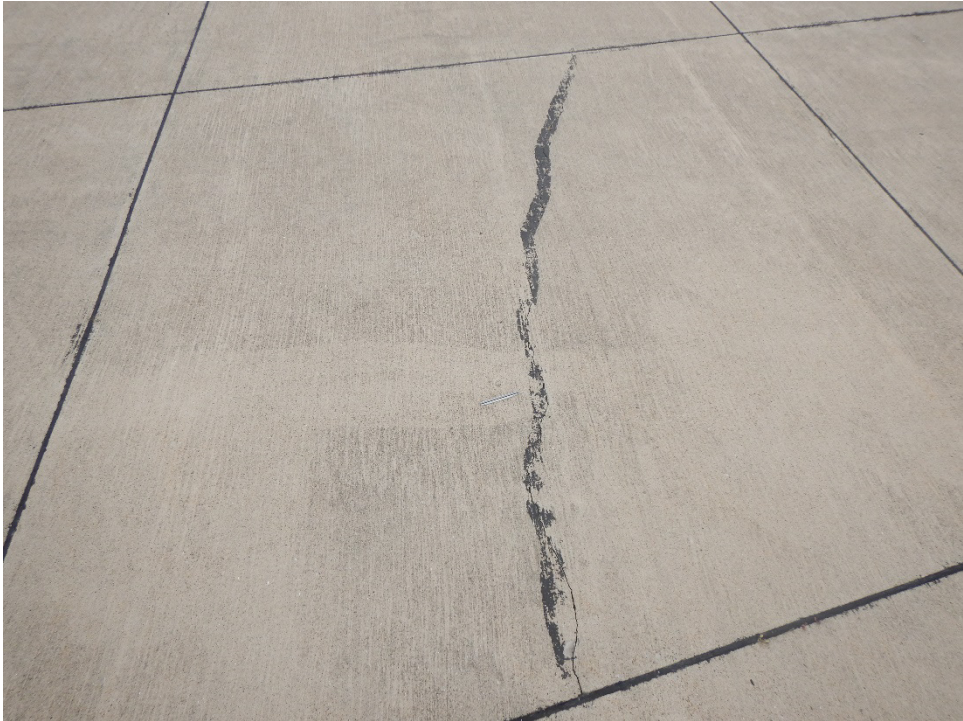
A01VI-03. LTD Cracking (Sample Unit No. 02).
