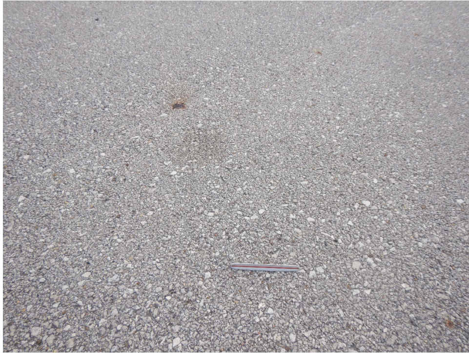
A01VI-02. Weathering (Sample Unit No. 08).
