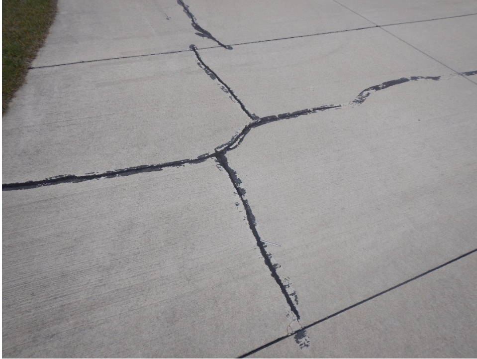
TH01VI-02. Shattered Slab (Sample Unit No. 04).
