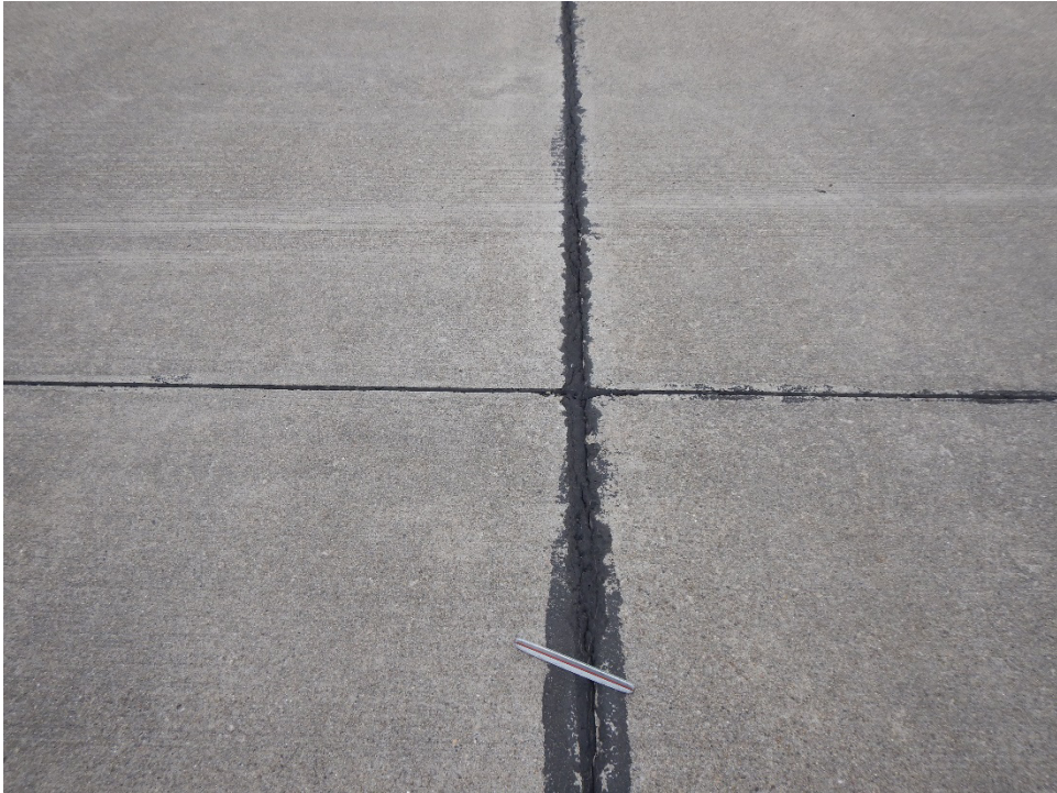
TH01VI-04. Joint Seal Damage (Sample Unit No. 02).
