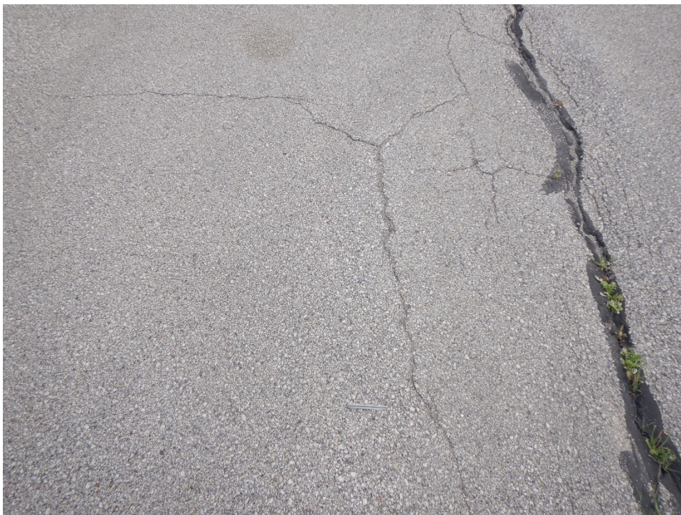
A01VI-05. L&T Cracking (Sample Unit No. 01).
