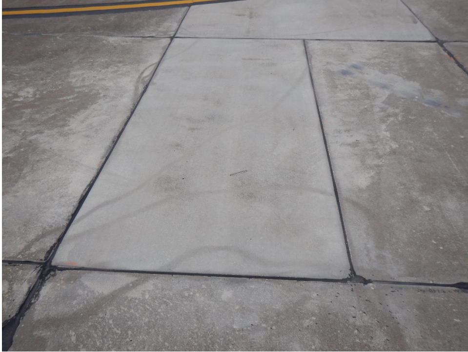
R09VI-01. Large Patching (Sample Unit No. 106).
