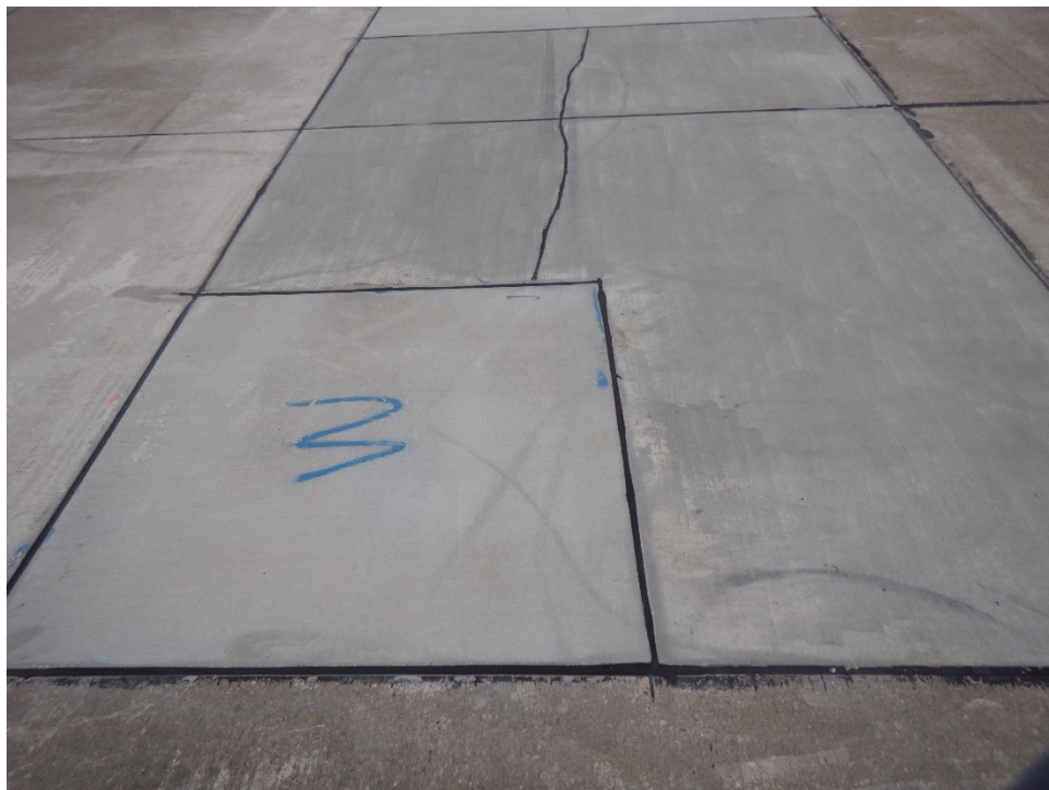
R09VI-01. LTD Cracking (Sample Unit No. 032).
