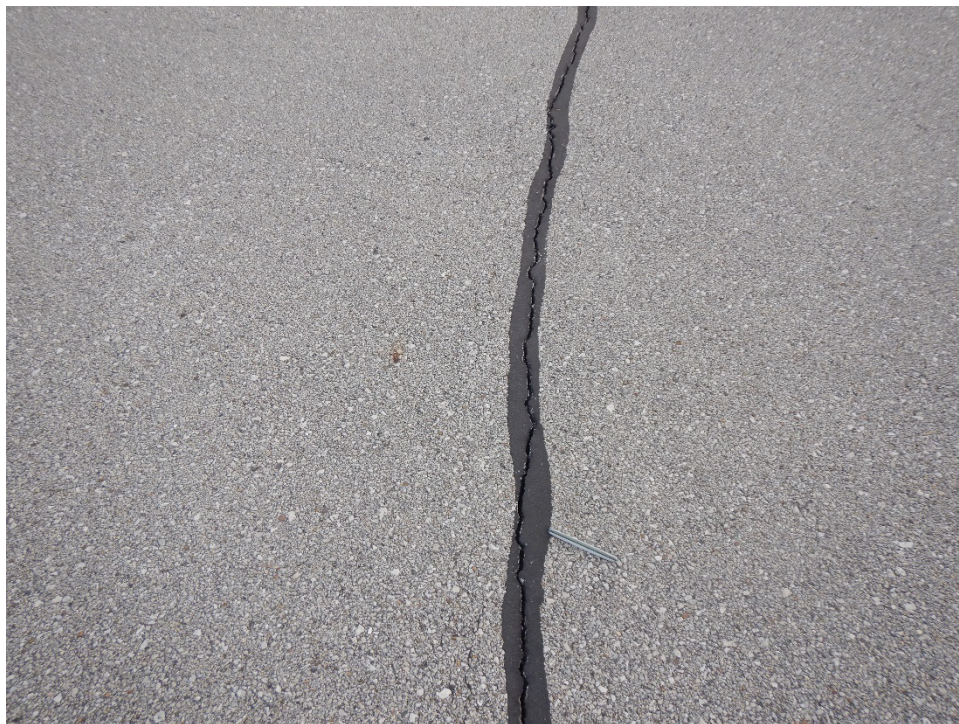
T01VI-01. L&T Cracking (Sample Unit No. 01).
