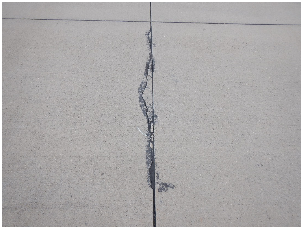
A01VI-04. Joint Spalling (Sample Unit No. 02).
