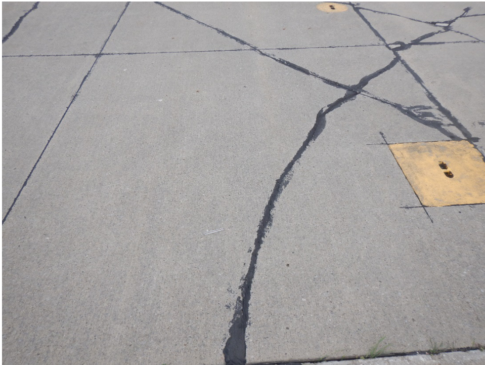
A01VI-01. Shattered Slab (Sample Unit No. 01).
