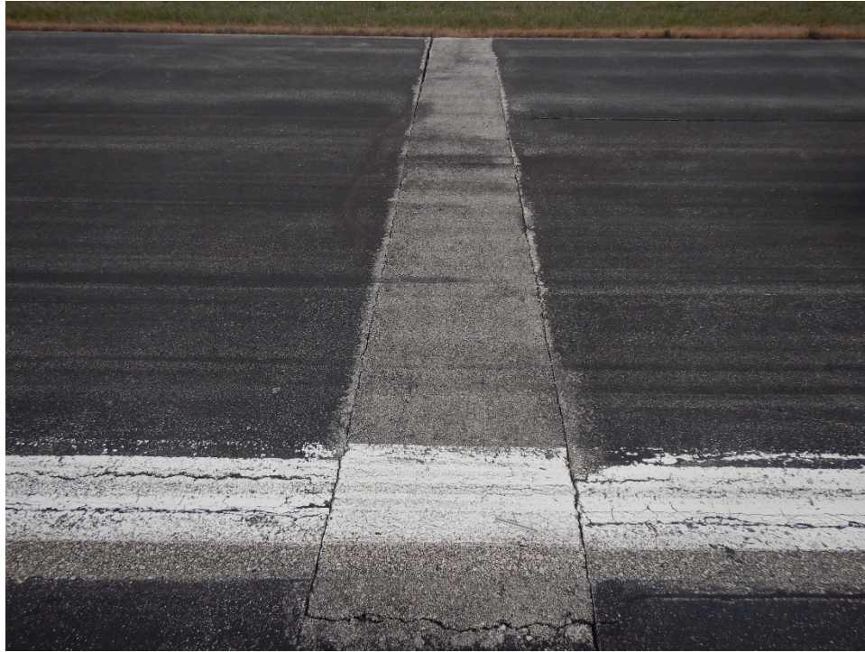
R16VI-01. Patching (Sample Unit No. 05).
