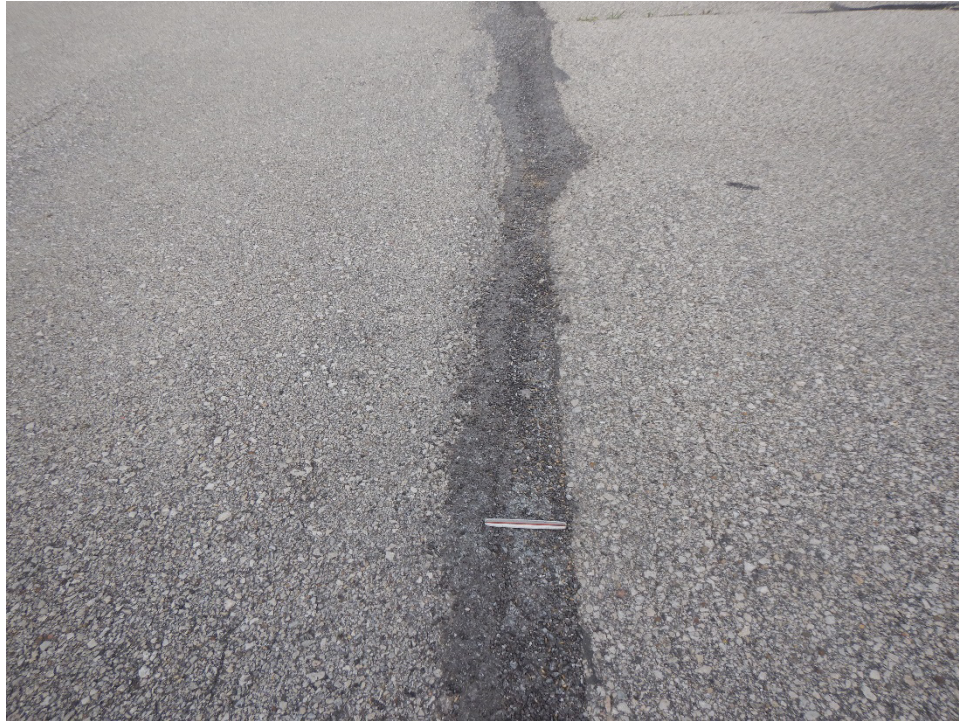
A01VI-02. Patching (Additional Sample Unit No. 01).
