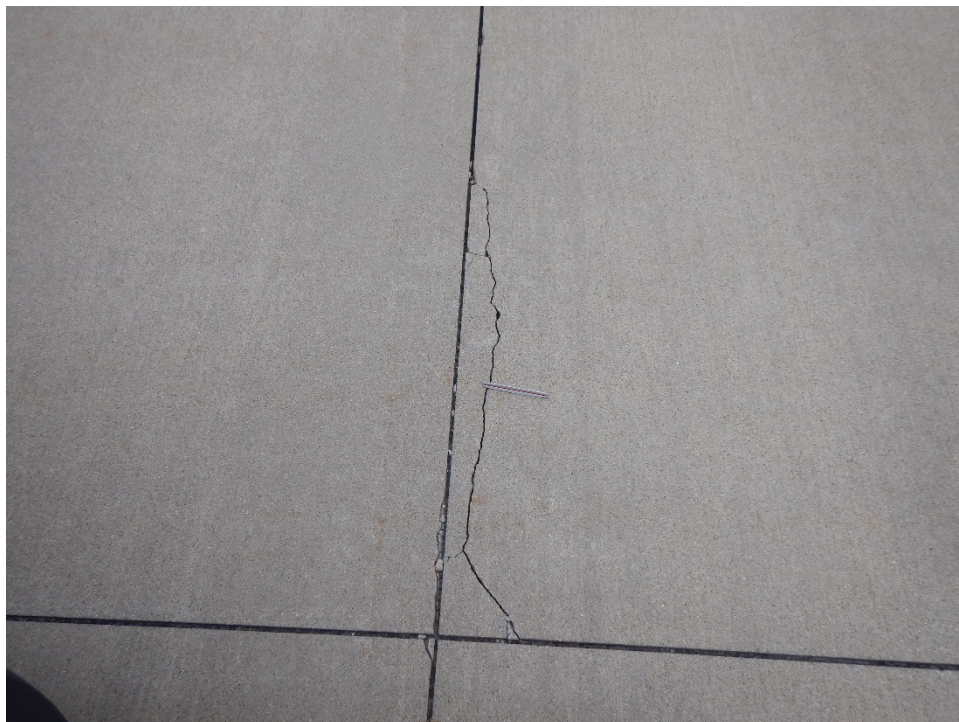
TH01VI-01. Joint Spalling (Sample Unit No. 02).
