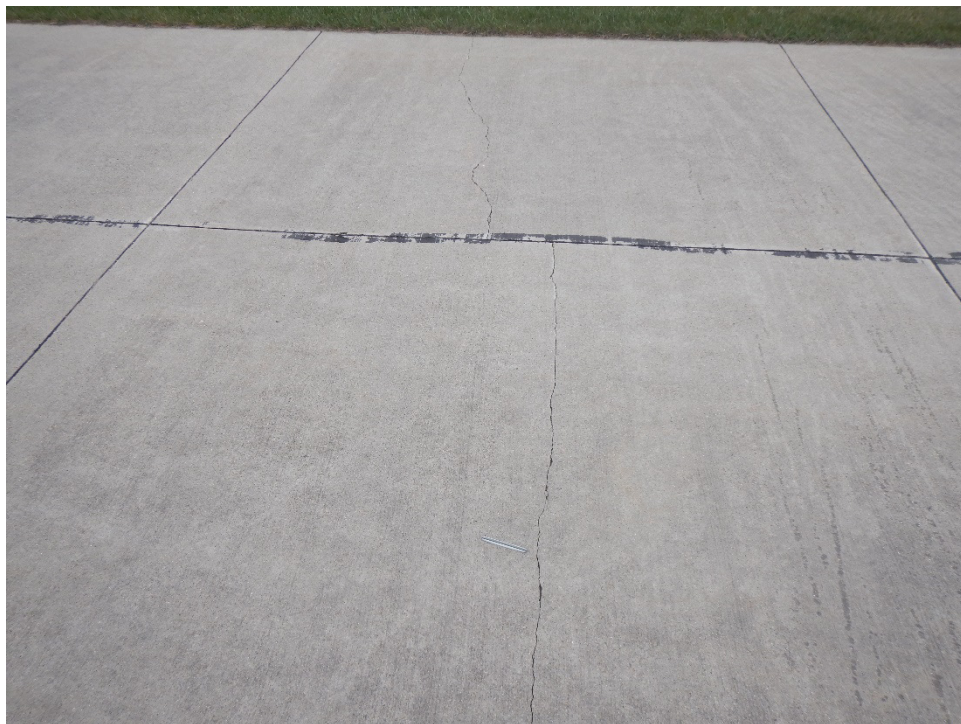
TH01VI-03. LTD Cracking (Sample Unit No. 02).
