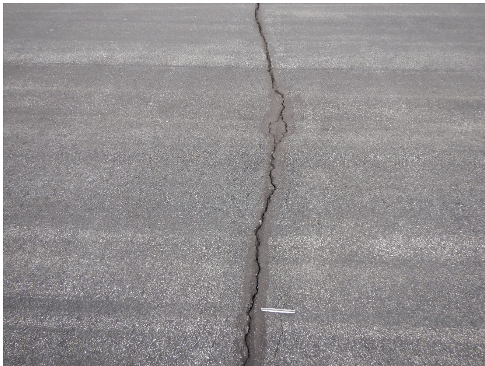
R16VI-01. L&T Cracking (Sample Unit No. 02).
