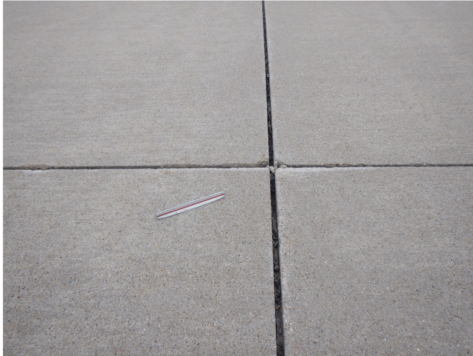
TH01VI-01. Joint Seal Damage (Sample Unit No. 02).
