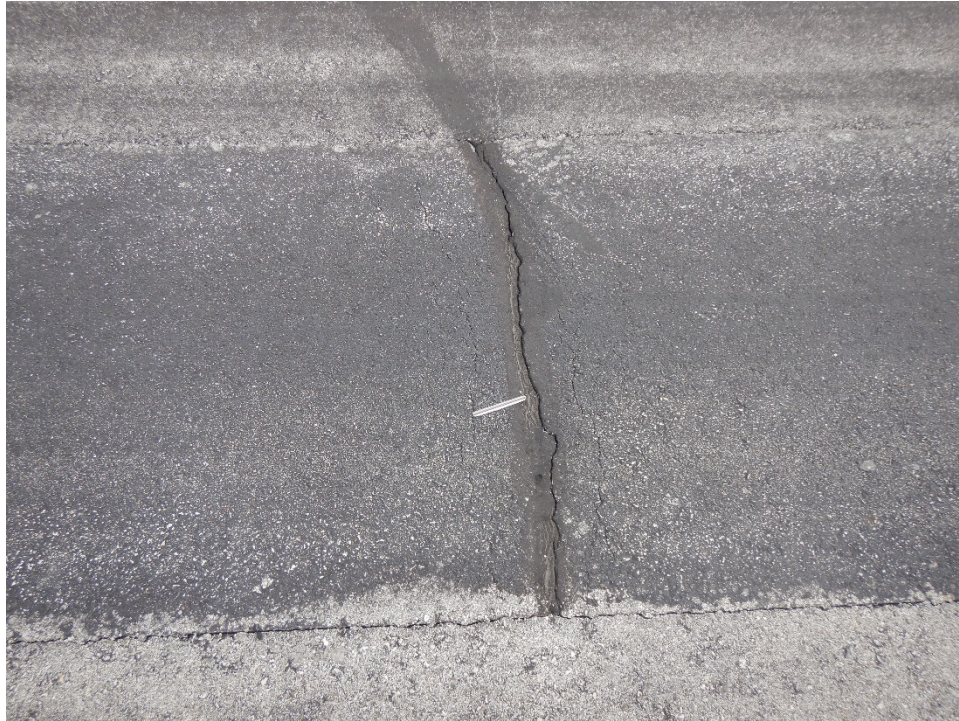
R16VI-02. L&T Cracking (Sample Unit No. 07).
