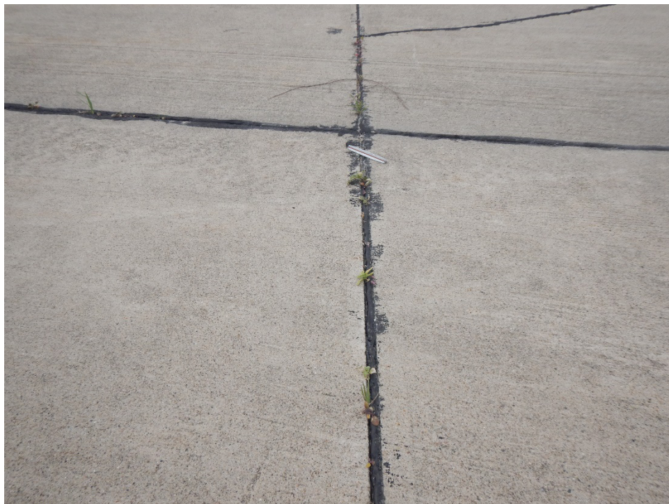
A01VI-03. Joint Seal Damage (Sample Unit No. 02).
