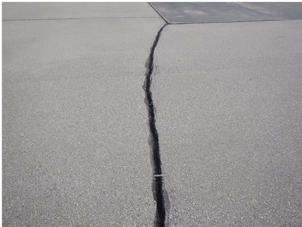
A01VI-02. L&T Cracking (Sample Unit No. 07).
