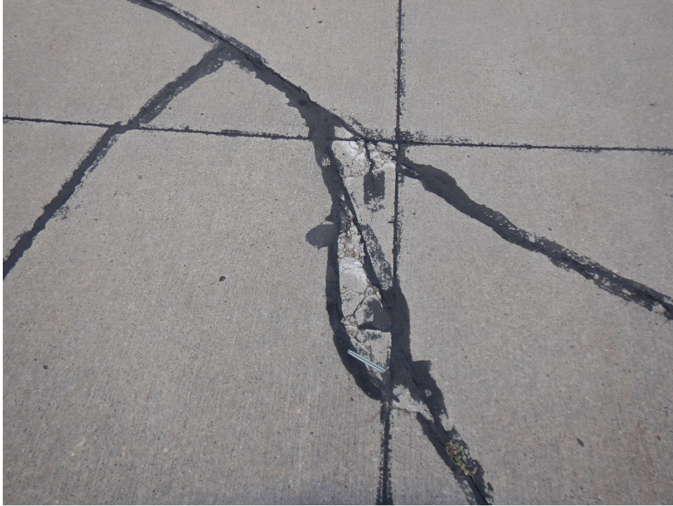
A01VI-01. Joint Spalling (Sample Unit No. 01).
