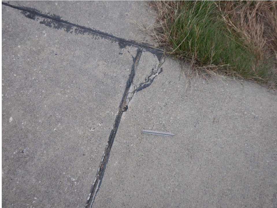
T03VI-01. Joint Spalling (Sample Unit No. 01).
