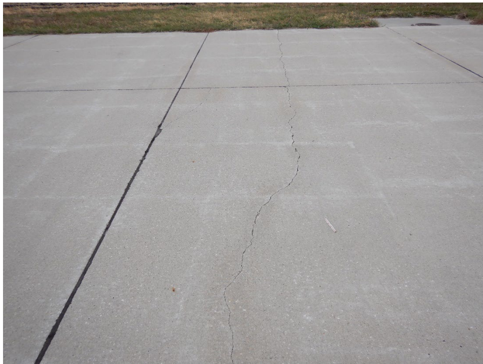
A01WC-04. LTD Cracking (Sample Unit No. 04).
