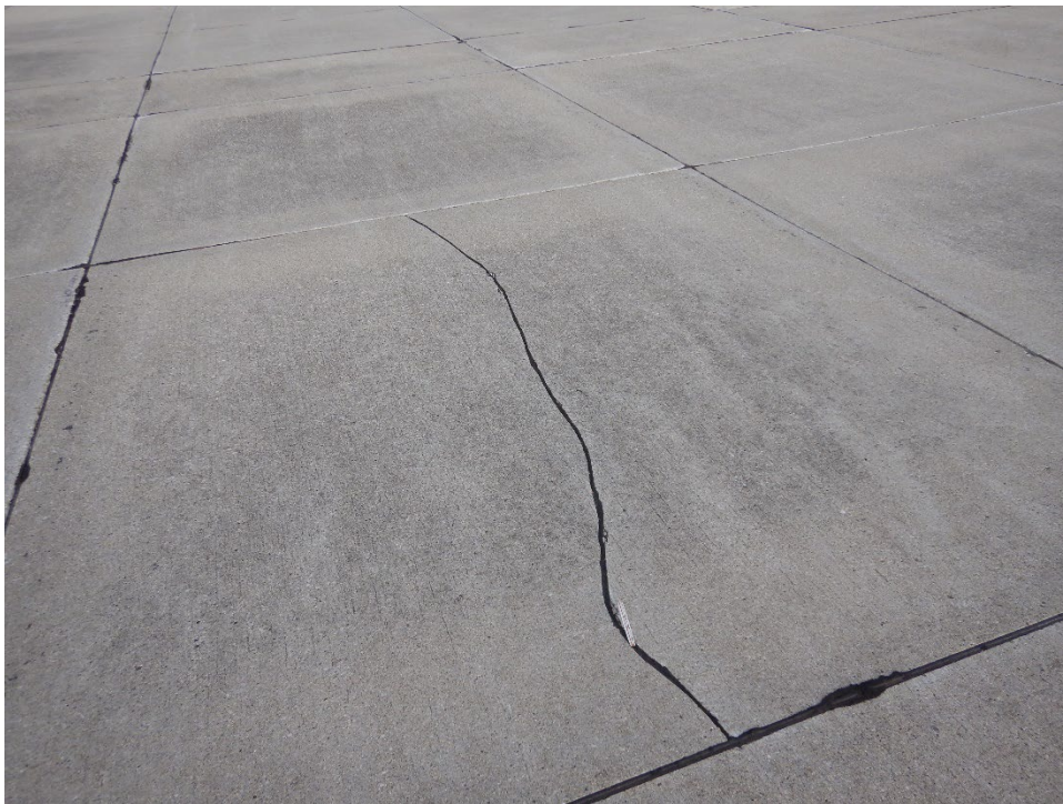
A01WC-02. LTD Cracking (Sample Unit No. 13).
