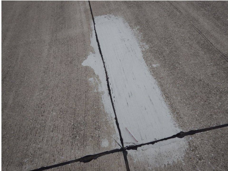
T03WC-01. Small Patching (Sample Unit No. 11).
