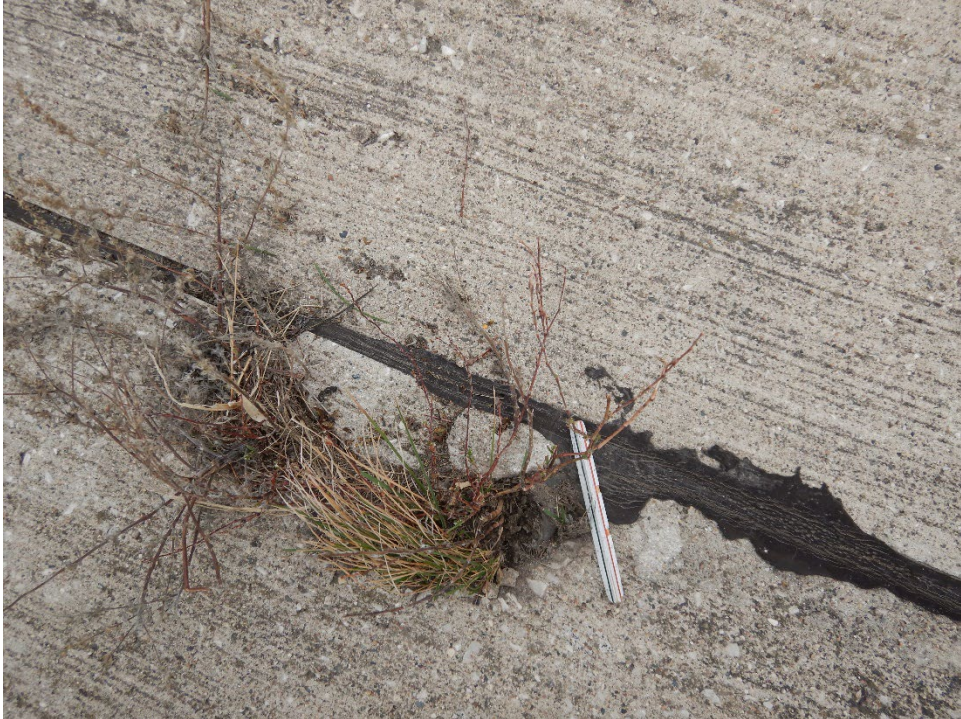
T04WC-01. Joint Spalling (Sample Unit No. 10).
