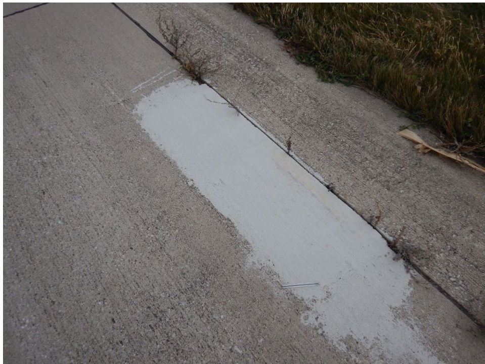
T01WC-02. Small Patching (Sample Unit No. 16).
