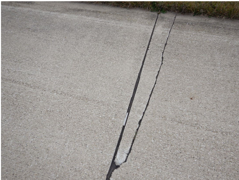
R14WC-01. Joint Spalling (Sample Unit No. 61).
