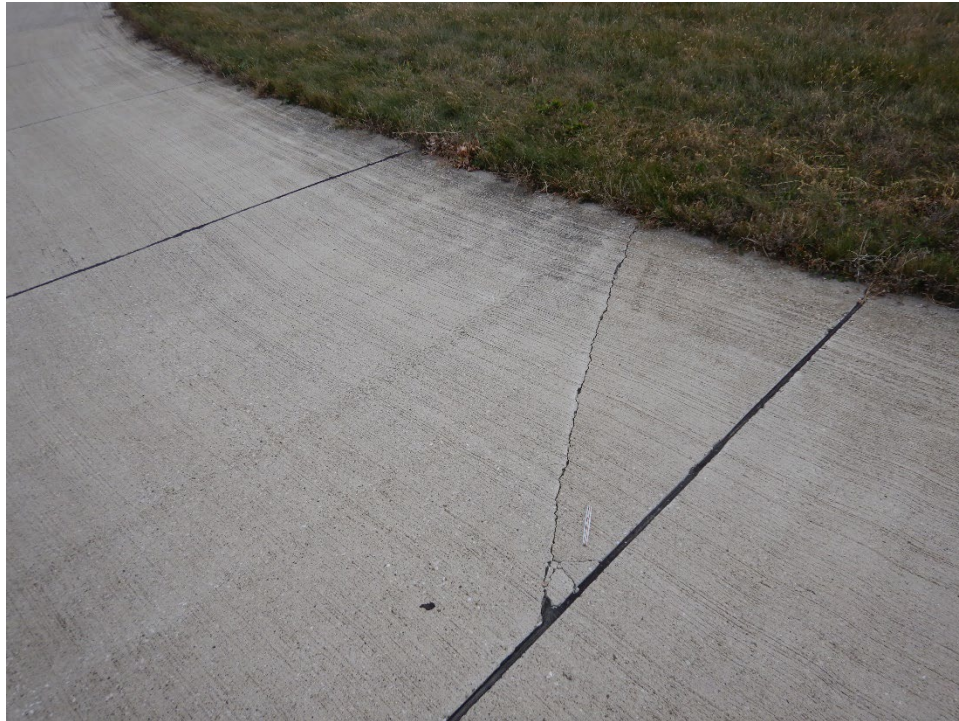
T01WC-02. LTD Cracking (Sample Unit No. 02).
