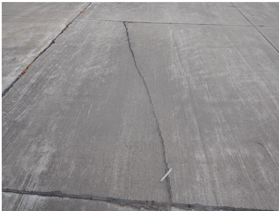
A01WC-03. LTD Cracking (Sample Unit No. 02).
