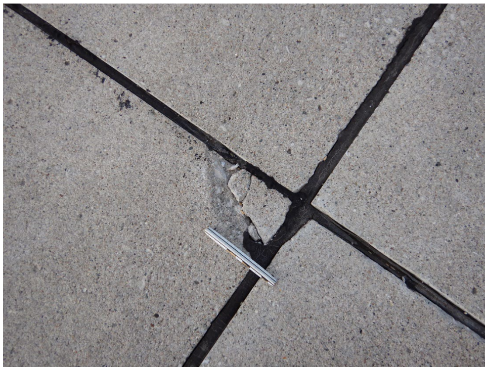
A01WC-01. Corner Spalling (Sample Unit No. 09).
