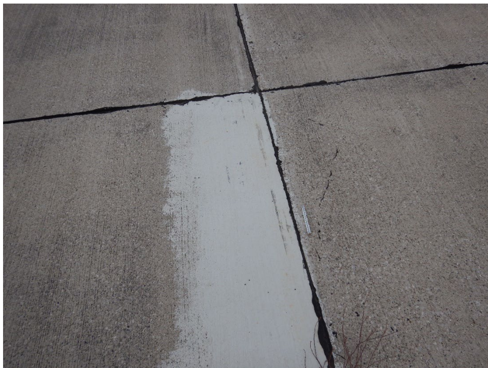
R05WC-01. Small Patching (Sample Unit No. 01).
