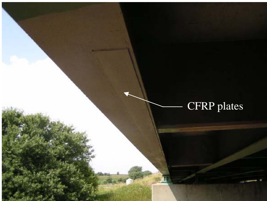
(e) Bottom of bottom flange of Girder 6 in the east end span
