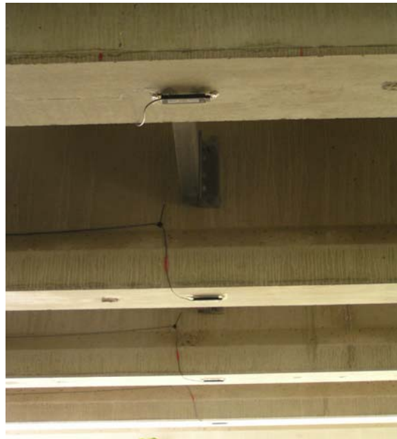
Figure 24. Overall View of the Long-Term Monitoring System (Peak Strain Sensors)
