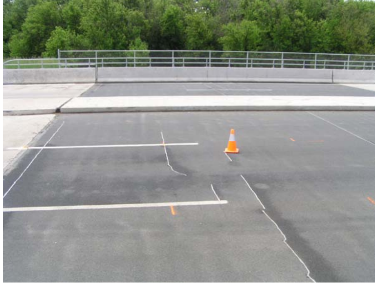
Figure 54. Transverse Cracks in North Traffic
