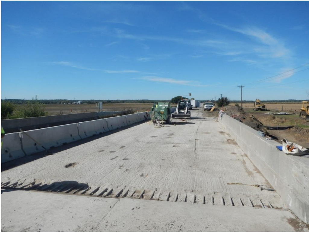
Figure E1. Overall view of IA92 deck, westbound lanes during Oct. 7, 2013 site visit.
