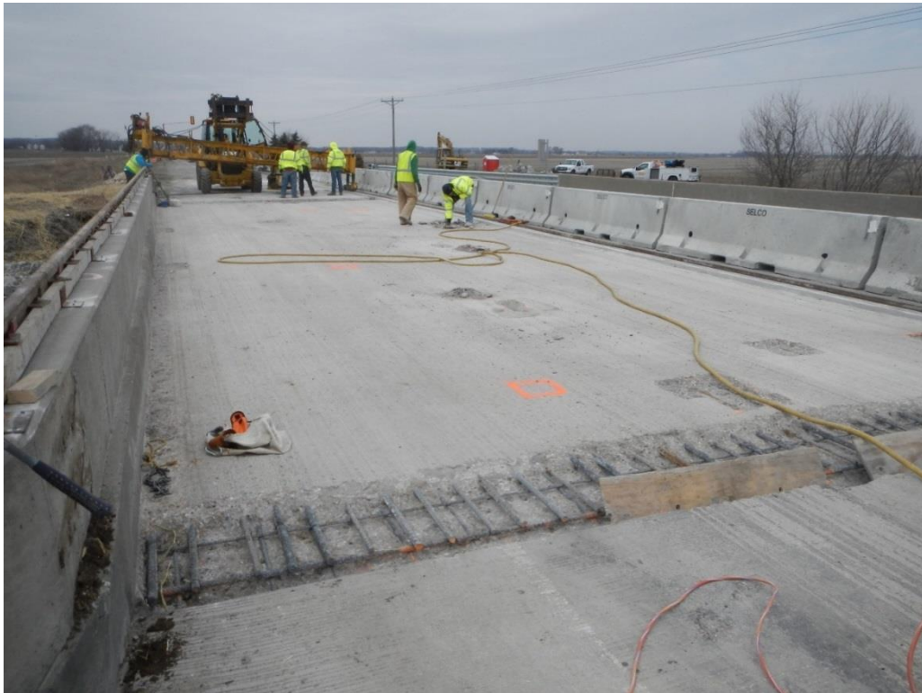
Figure E5. Overall view of IA92 deck, eastbound lanes during April 2, 2014 site visit.
