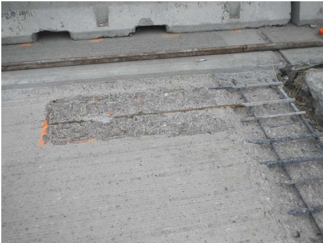
Figure E8. Deck repair location extending from deeper repair at end joint in eastbound lanes of IA 92 deck.
