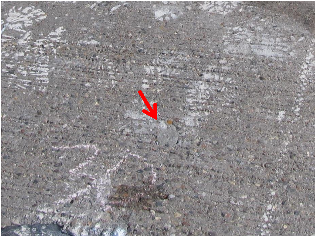
Figure 3.3. Patched rail anchor hole at west end of westbound lanes.
