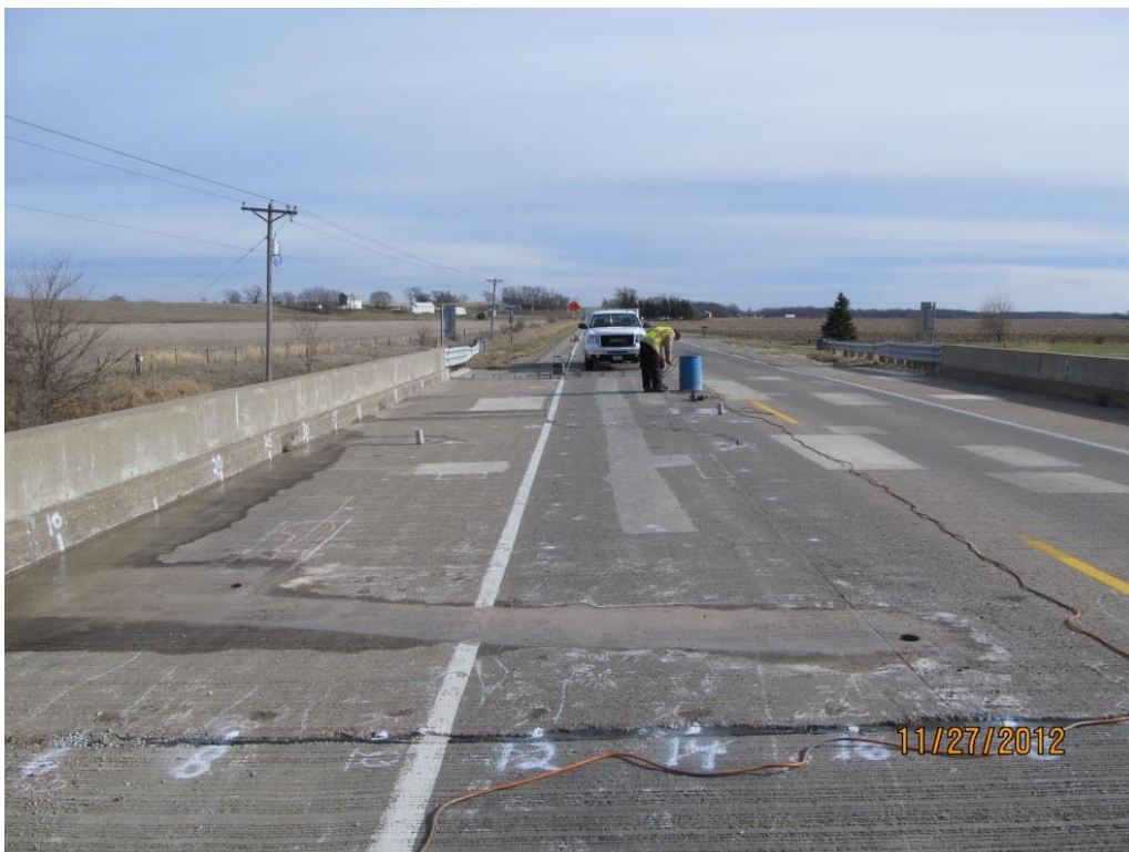
Figure 3.2. Overall view of westbound lane of bridge, looking east. Chalk lines indicate cracks and delaminations identified by survey.
