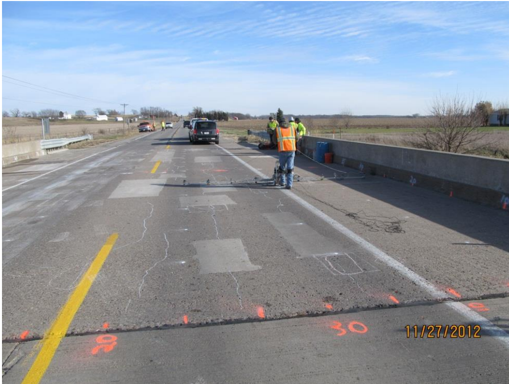
Figure 3.1. Overall view of eastbound lane of bridge, looking east. Chalk lines indicate cracks and delaminations identified by survey.
