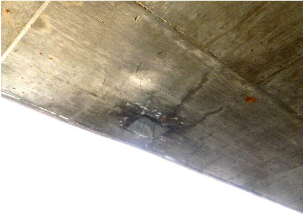
Figure 3.8. Moisture staining on deck underside surrounding drain penetration.
