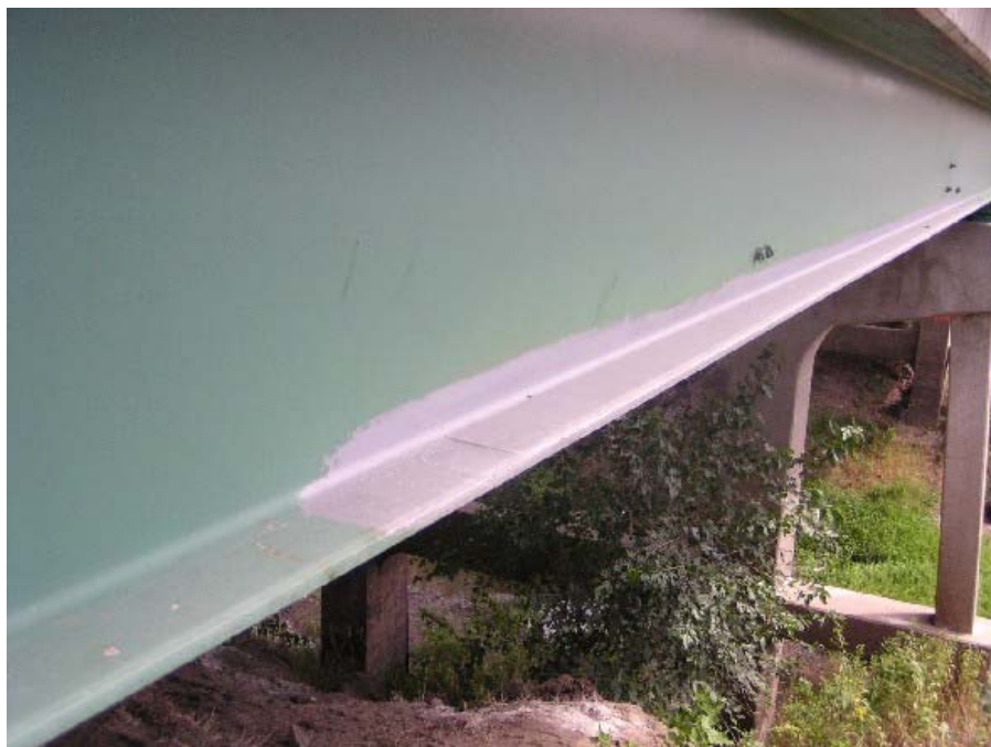
b. Top of bottom flange of Beam 6 in the west end span
