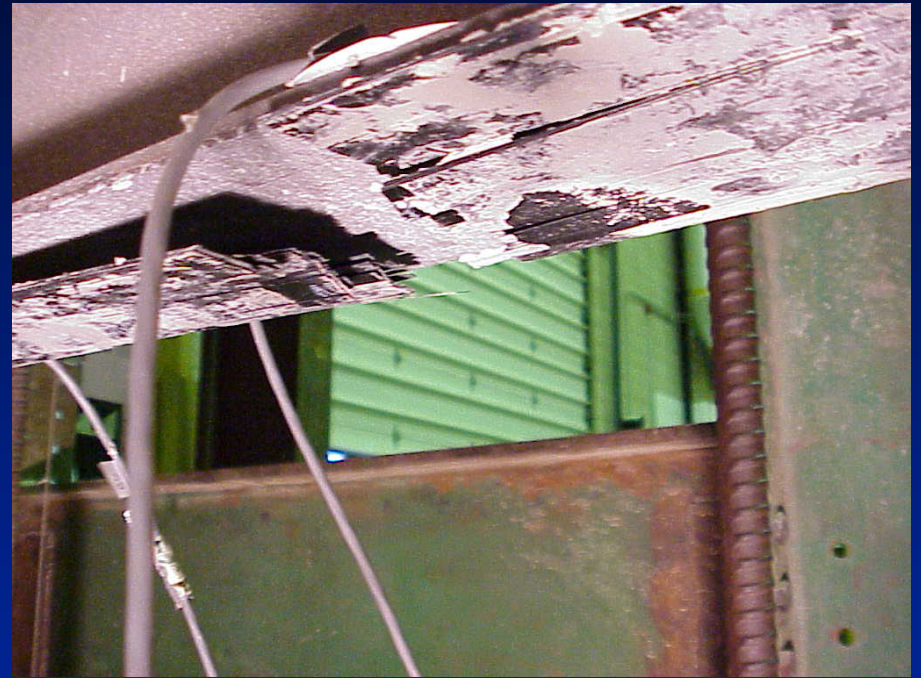
CFRP plate rupture
