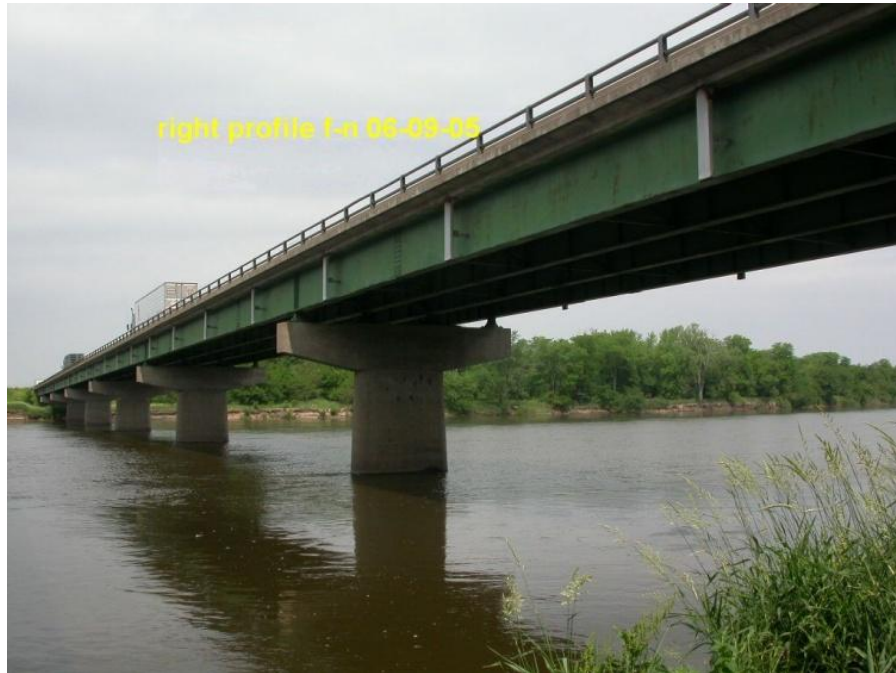
Figure 2. Profile of one of the twin I-80 Bridges over the Cedar River.
