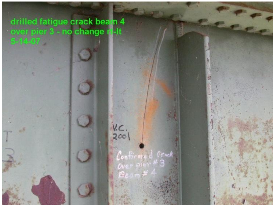
Figure 6. Fracture of web on Girder 4 at Pier 3 of the eastbound I-80 Bridge over the Cedar River. In 1981, a 20" long fracture was found which was initiated at the top of the bearing stiffener at the pier
