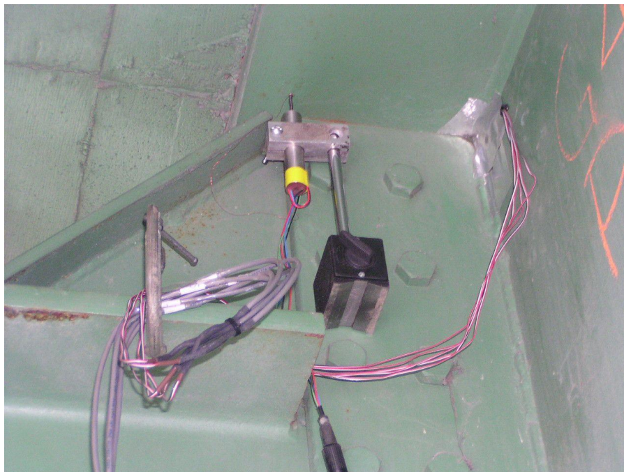
Figure 11. Displacement sensor (same location as Figure 10) to measure girder top flange tipping (vertical displacement also referred to as tilt in this report) relative to bearing stiffener. Similar set-up was used at all four girders at Pier 3.
