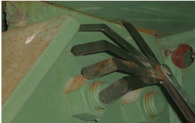
Figure 20. Feeler gage inserted between top of bearing stiffener and Girder 4 top flange at Pier 6. Note the corrosion between the interfaces and also note the retrofit hole that had been previously drilled to arrest a fatigue crack in the girder web.
