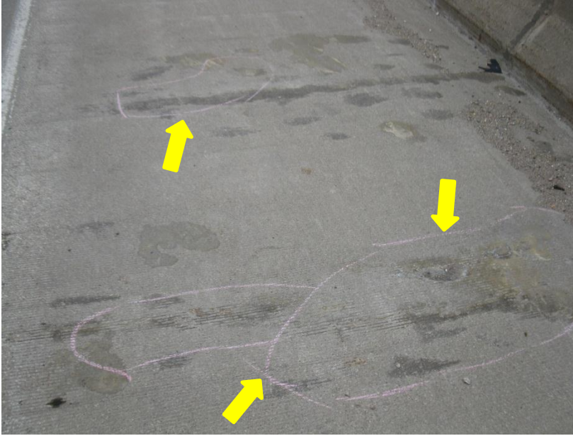
Figure 2.10. Delamination in shoulder (highlighted in chalk). Note epoxy injection resin on the surface.
