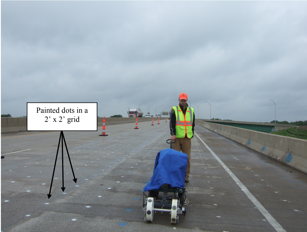
Figure 2: Photograph showing test grid layout for BDS-IEtesting on a 1 ft grid with impacts every 6 inches to provide 1 test every 0.5 sq ft
