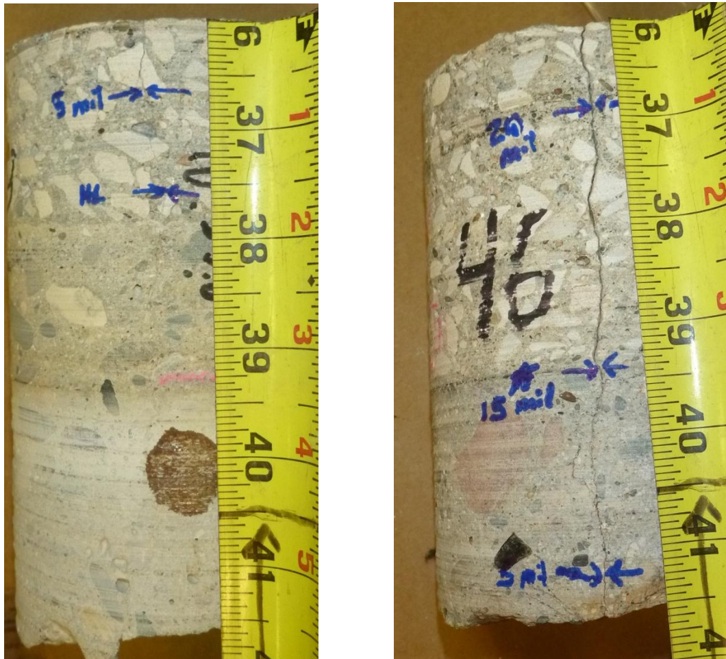
Figure 8.7. Comparison of crack width versus depth for Cores 33 and 46.
