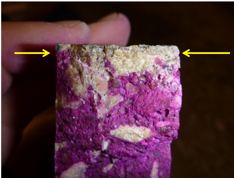
Figure 8.2. Phenolphthalein indicator on a freshly cracked surface of a core. The depth of carbonation is indicated by the arrow (pink color indicates pH > 9 ).
