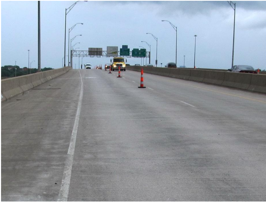
Figure 3.13. Deck surface showing surface texture and color variation between wheelpaths and surrounding deck.
