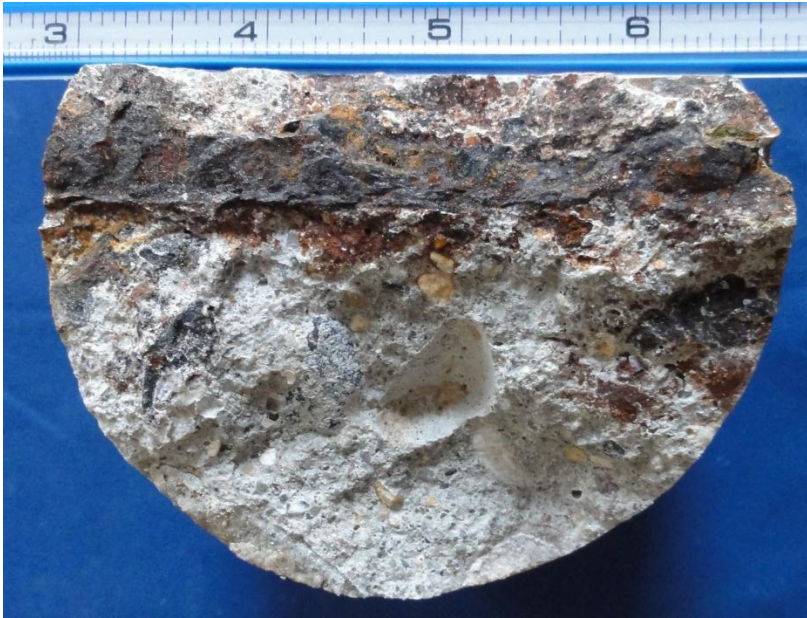
Figure 8. Core 42; corroded rebar in base concrete at one of the transverse cracks.
