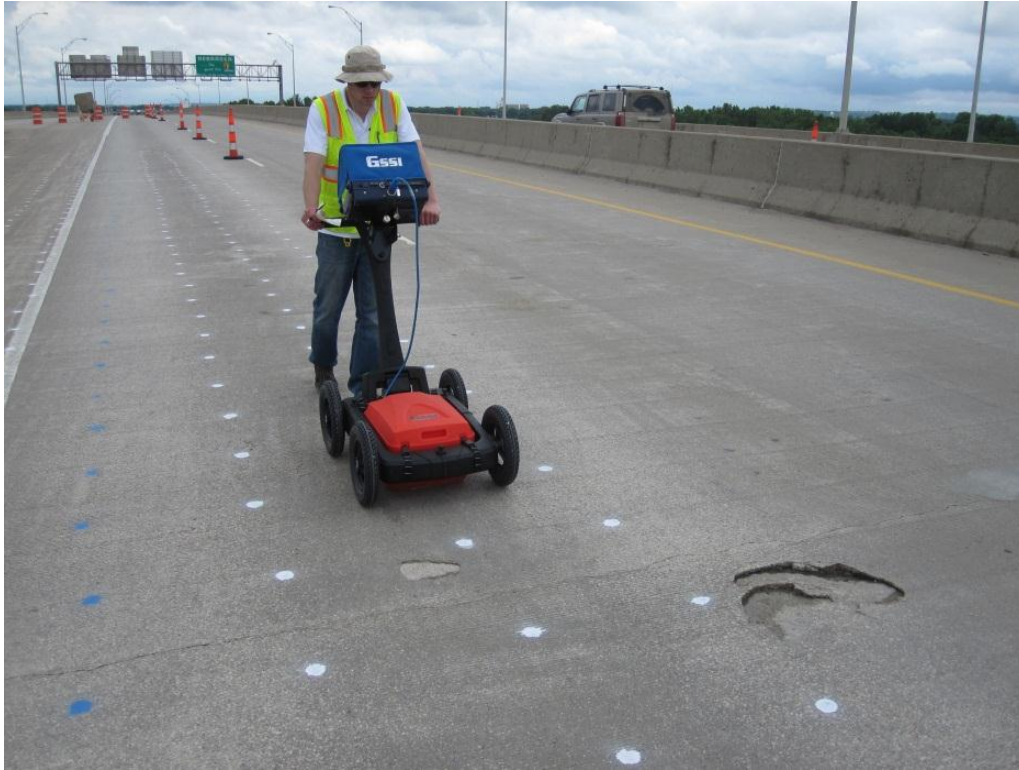
Figure 4.1. GPR data collection within the WB-2 study area using the GSSI Bridgescan system.
