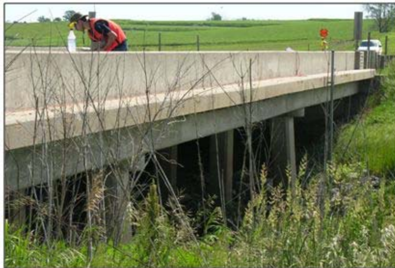
Figure 95. Side view of Bridge O5 showing full-depth (slab) deck construction between piers.
