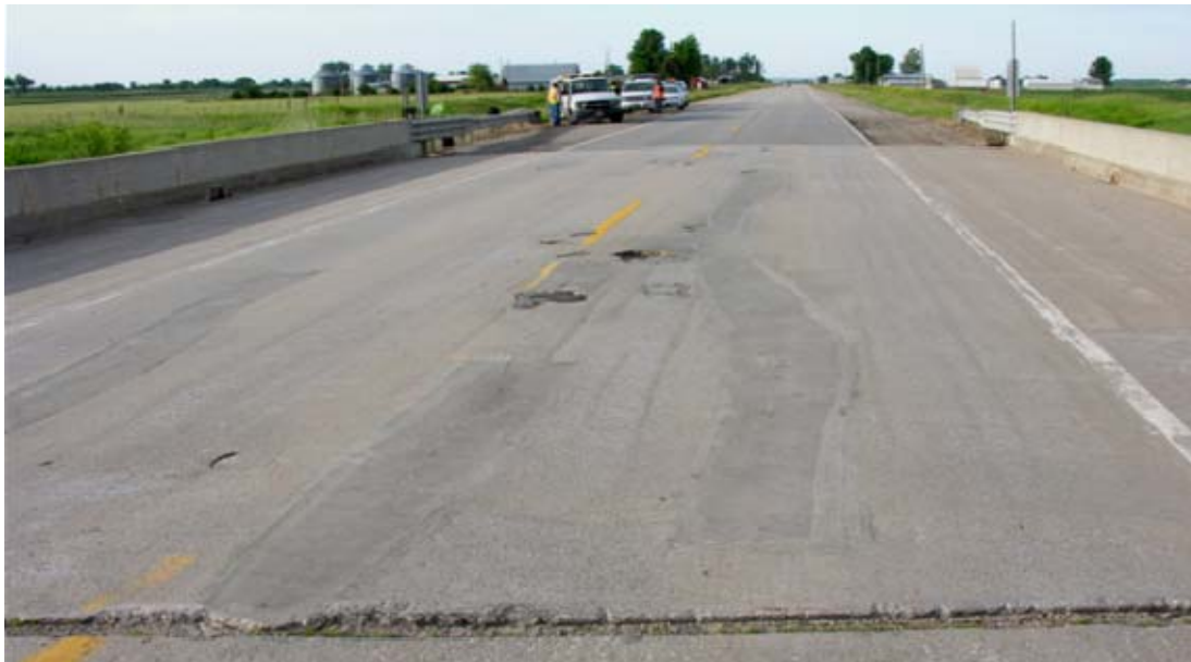
Figure 103. Perspective view of Deck O6, looking southbound, shows PC patches and spalls.
