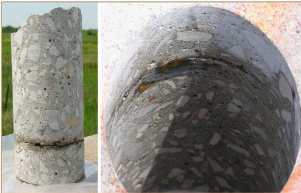
Figure 100. Core #1 – expected to be “fair to poor” – shows delamination, and core hole reveals “nicked” rebar, delamination and corrosion.
