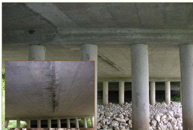
Figure 76. Rust stain almost full length between piers, roughly along centerline.
