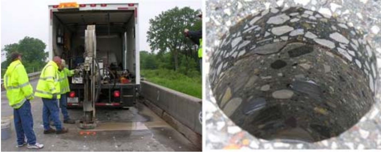
Figure 67. Core # 3 during extraction, where upper edge of delamination meets the debonded overlay just below the overlay, with both longitudinal and transverse rebars seen in the photo.
