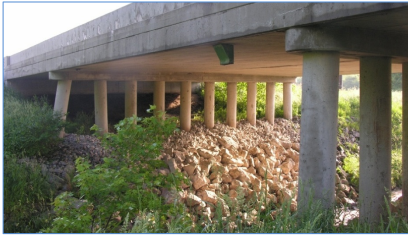
Figure 75 Side view of Bridge O3 showing full-depth (slab) deck construction between piers
