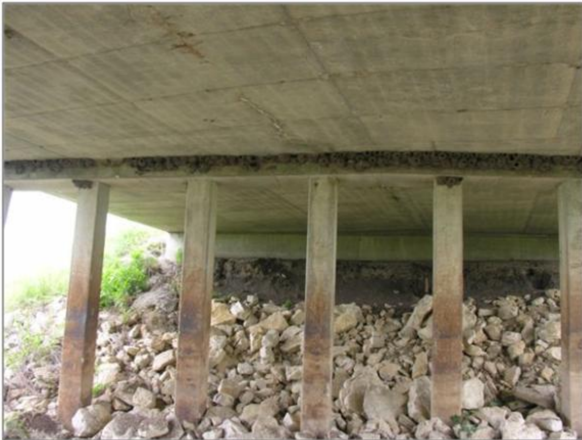
Figure 105. Bottom view of Deck O6 (continuous slab) shows rust staining, efflorescence and swallow nests along entire deck underside at pier.
