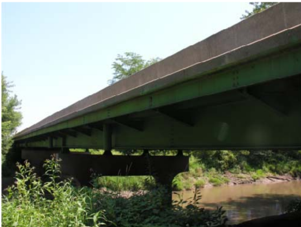
Figure 135. Side view of Deck R1 showing continuous slab construction on east face.
