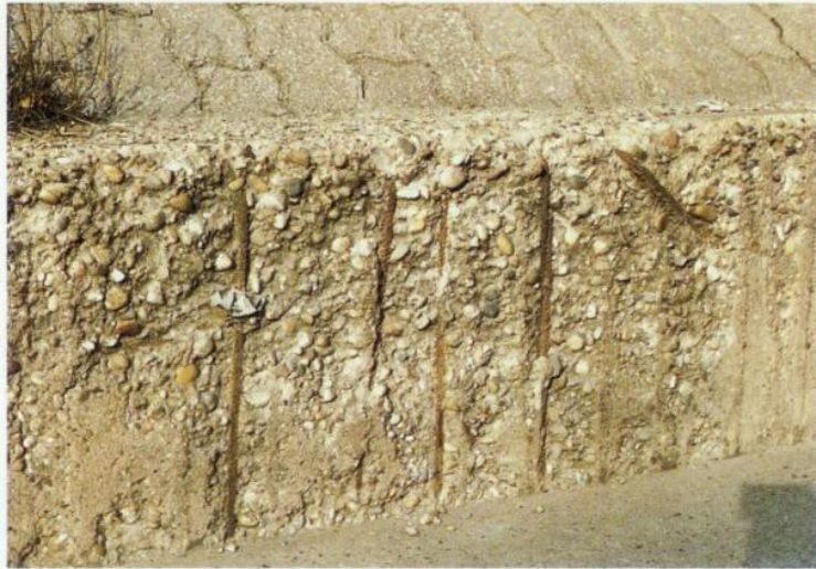
Figure 6. Crumbling and scaling of a concrete surface after freeze and thaw cycles (Nuernberger, 1995).
