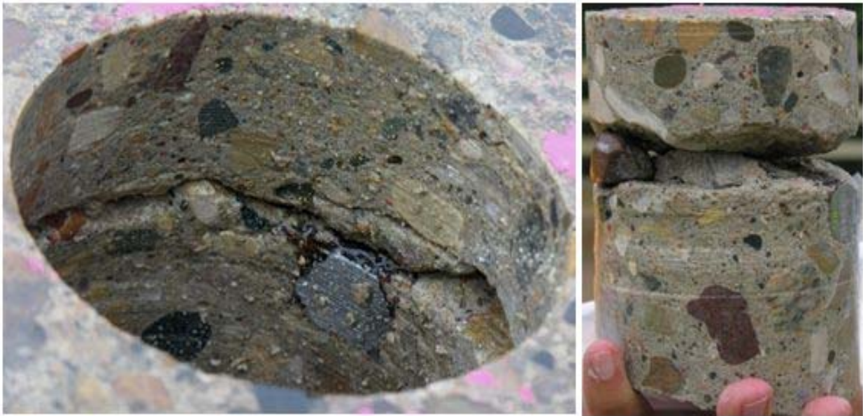
Figure 93. Hole and core sample (Core #3) with severe delamination and corrosion at top and sides of rebar.
