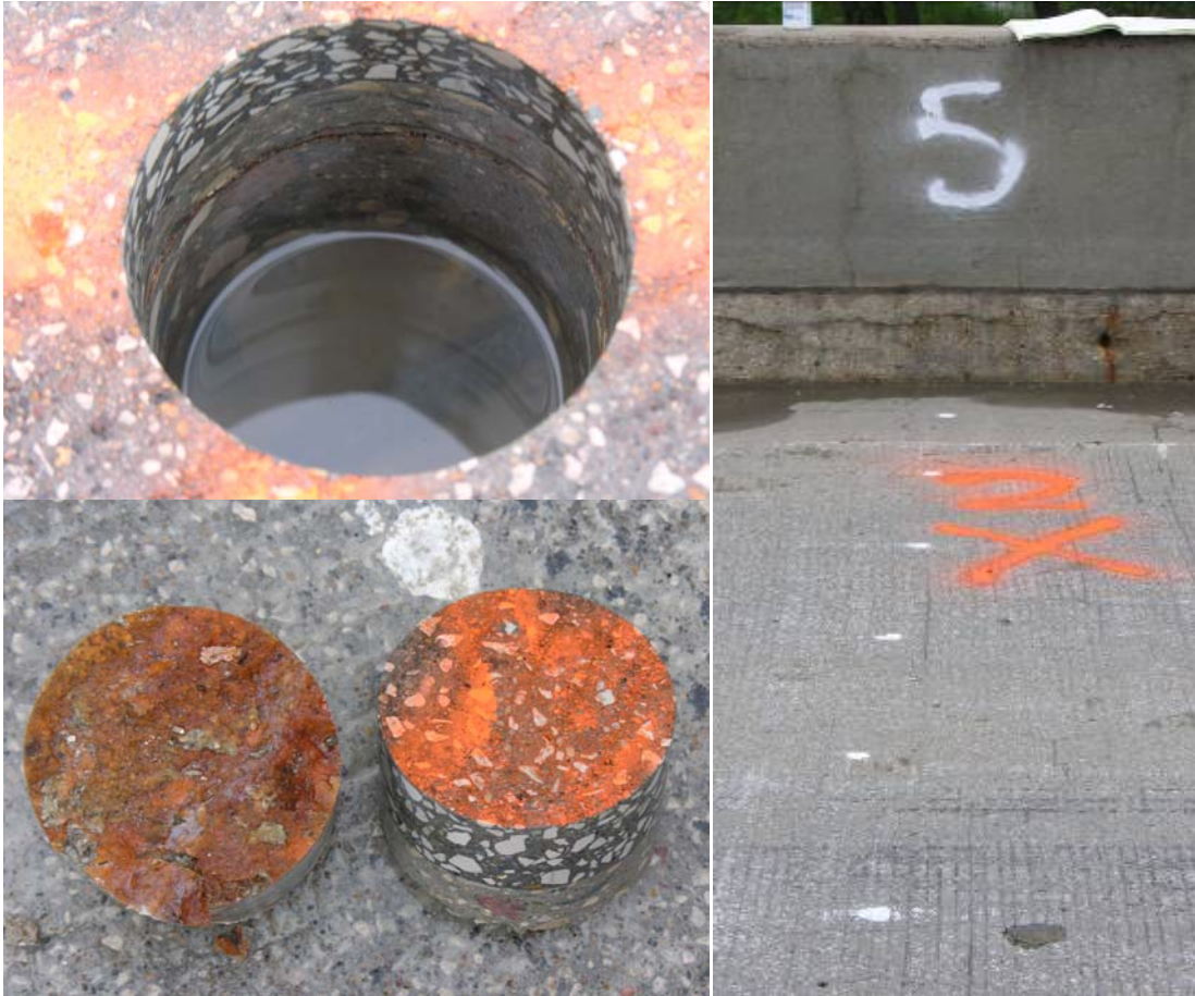
Figure 62. Photos of Core #2 location, showing extracted core, epoxy-filled delamination in core hole, and bonded overlay.
