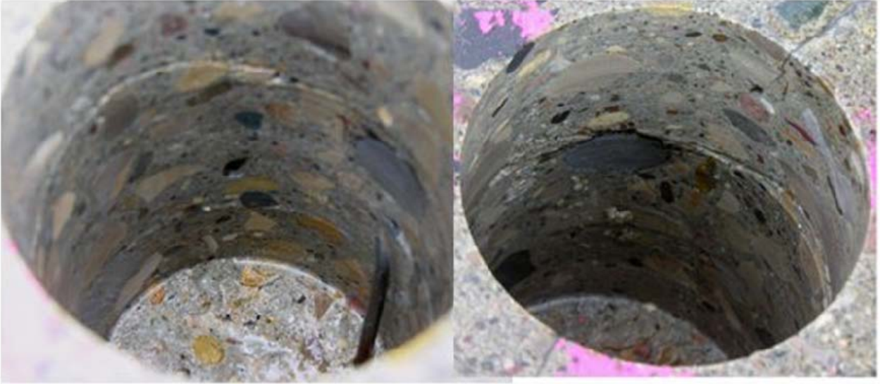
Figure 92. Hole from which Core #4 was retrieved, showing delamination in both photos, rebar chair beneath bar in left photo, and rebar with corrosion at top and sides in right photo.
