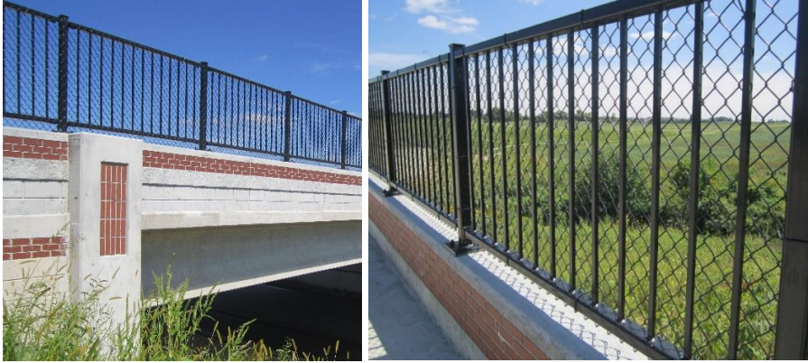
Figure 5.8.1.2.5-2. Example Welded Picket Railing with Chain Link Mesh (project shown is NHSX-100-1(93)—3H-57, Linn. Co. Design No. 915)
