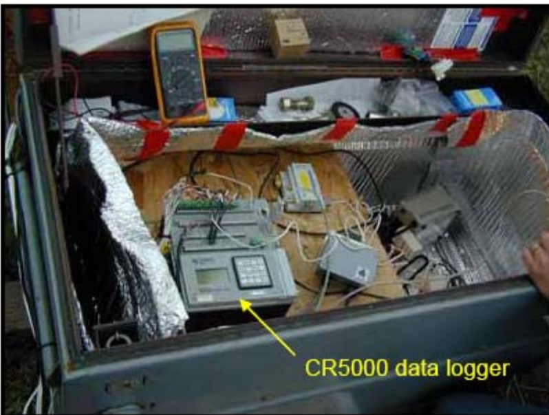
Figure 3-13. Data acquisition system at Pole 2
