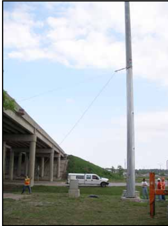
Figure 1.2 – Typical dynamic test of a retrofitted tower along I-29 in Sioux City, Iowa
