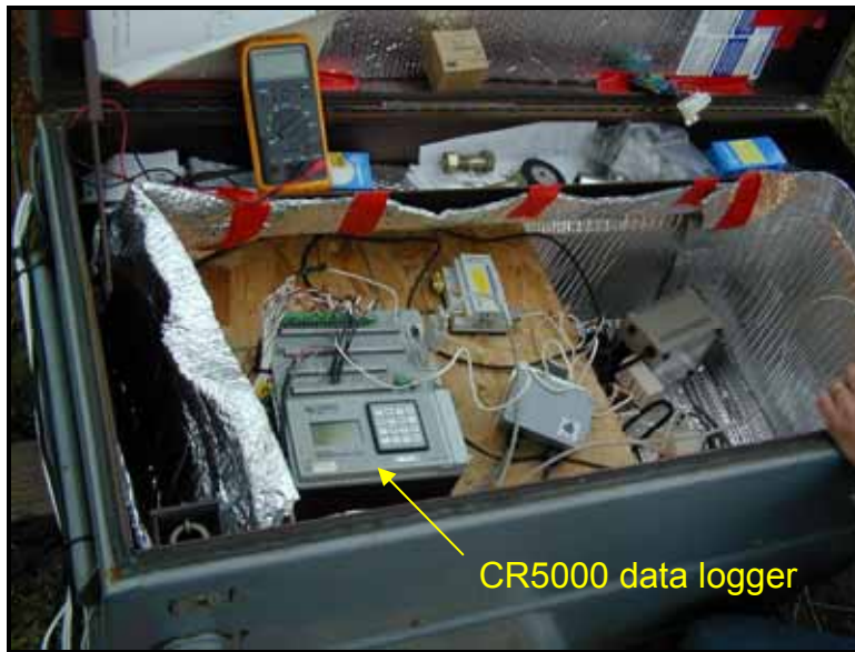
Figure 2.8 – View inside the weather-tight box at the Retrofit tower along US-18 in Clear Lake, IA
