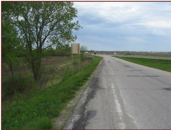
Photo 14. JASPER COUNTY RCB CULVERT AT EXIT 159 EASTBOUND EXIT RAMP NEAR INDIAN CREEK (FLOODING)- LOOKING WEST FROM F-48W EASTBOUND OFF RAMP
