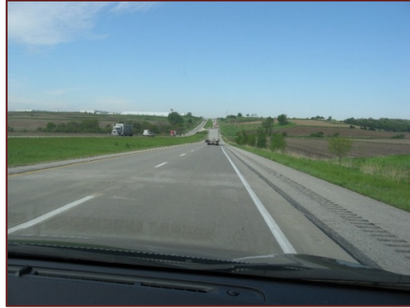
Photo 2. POTTAWATTAMIE COUNTY NEAR MP 35/SILVER CREEK (HIGH TEMPERATURE CHANGE) – I-80 WESTBOUND LANES LOOKING WEST
