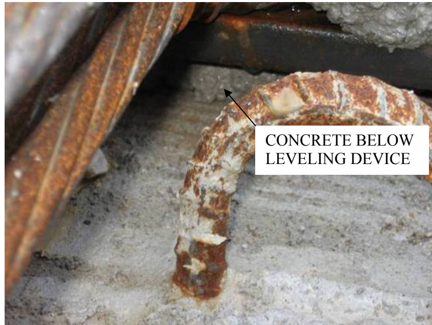
c) Concrete below the leveling device
