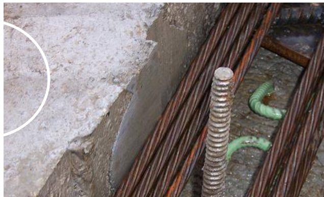
Figure 86. Concrete obstruction in Channel 1
