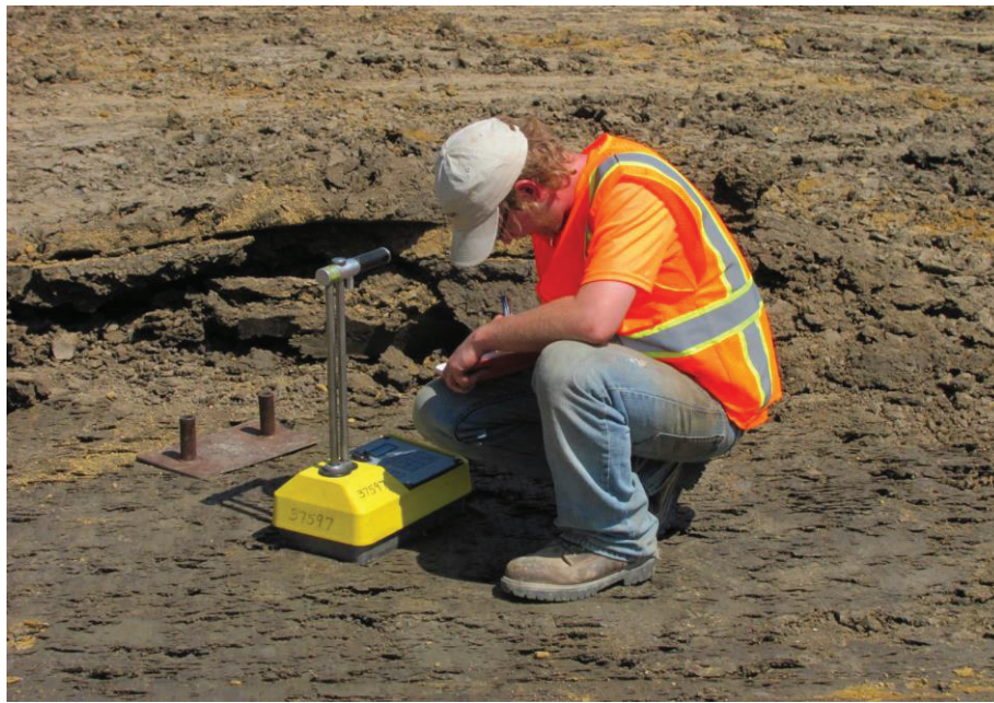
Figure 6-9: Nuclear gauge test used to determine in-place density of a compacted lift.
