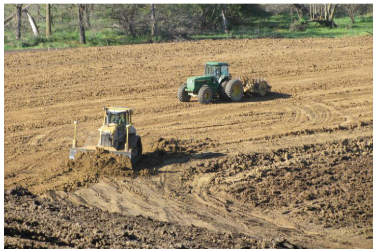
Figure 9-1: Pre-construction photo of a marsh-like area (top). Installation of granular working blanket (middle). First lifts being placed and compacted on top of the granular working blanket (bottom).
