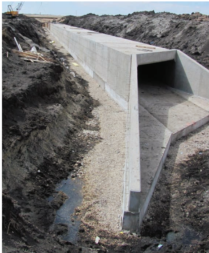
Figure 6-16: Contractor should not place backfill at box culverts until at least 14 days after concrete has been placed.
