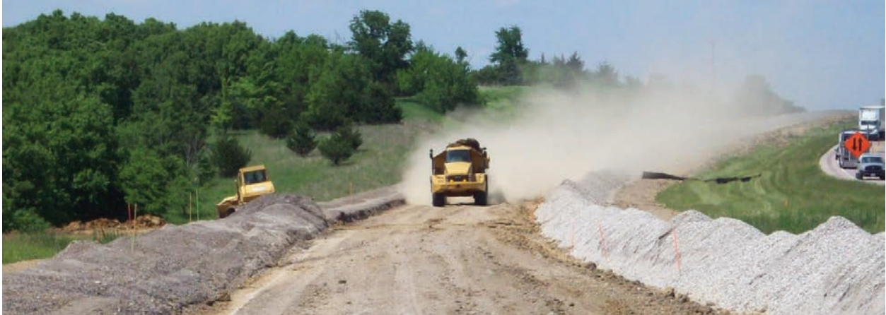
Figure 6-19: Haul roads or the project site may require application of water for dust control.
