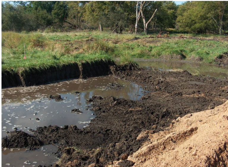
Figure 9-2: This photo shows a core-out to remove compressible soils as well as a sand blanket to be used to provide a workable platform from which to build the embankment.
