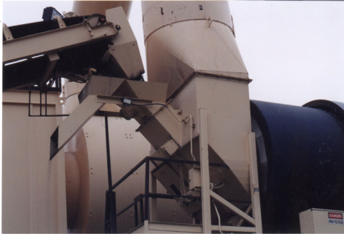
Fixed Chute Entry to Dryer with Vibrator on Chute
