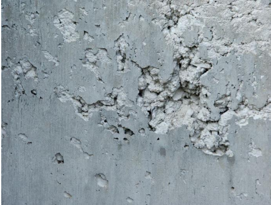
Figure 5-7 Bugholes and honeycombing at wall effected zone
