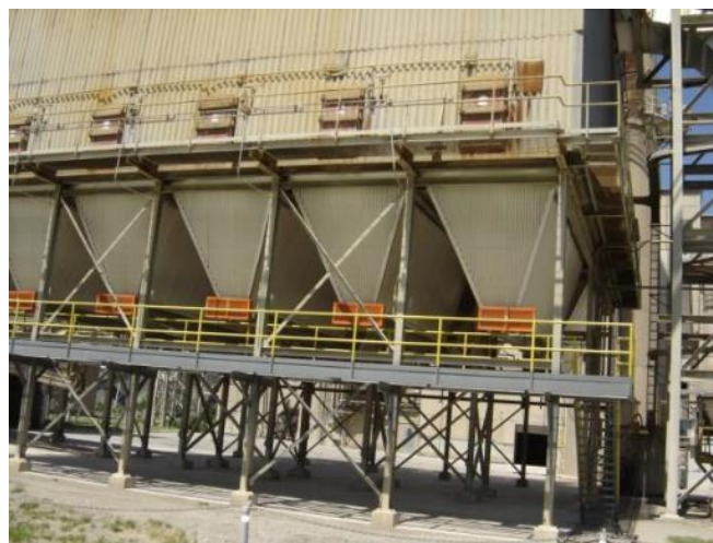
Figure 2-6 Bins used for blending operation
