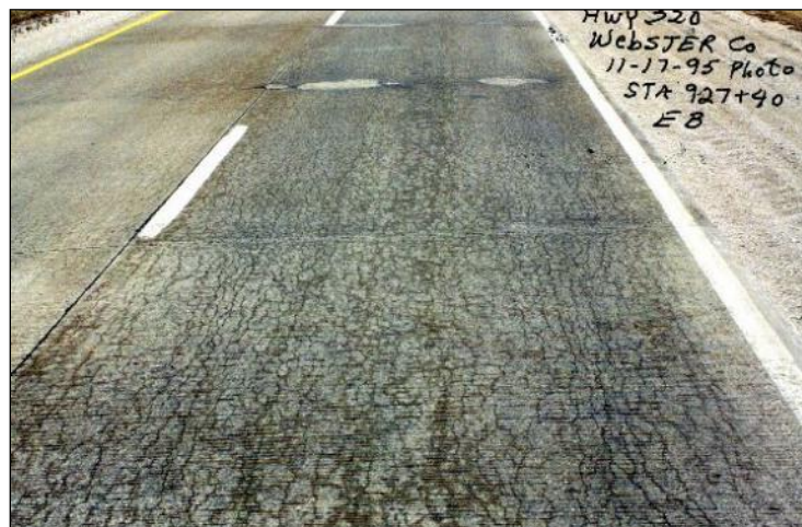
Figure 3-4 Example of freeze thaw damage on five-year-old pavement
