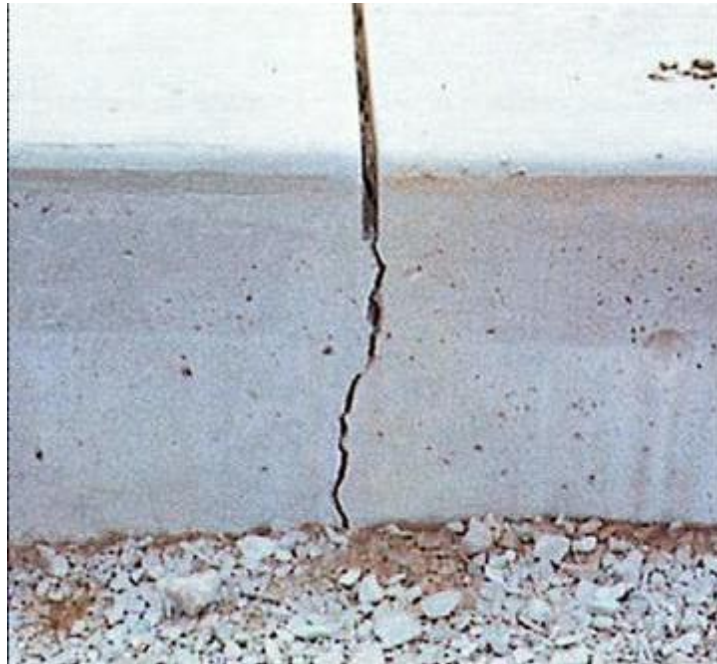
Figure 2-27 Drying shrinkage cracking controlled at joint
